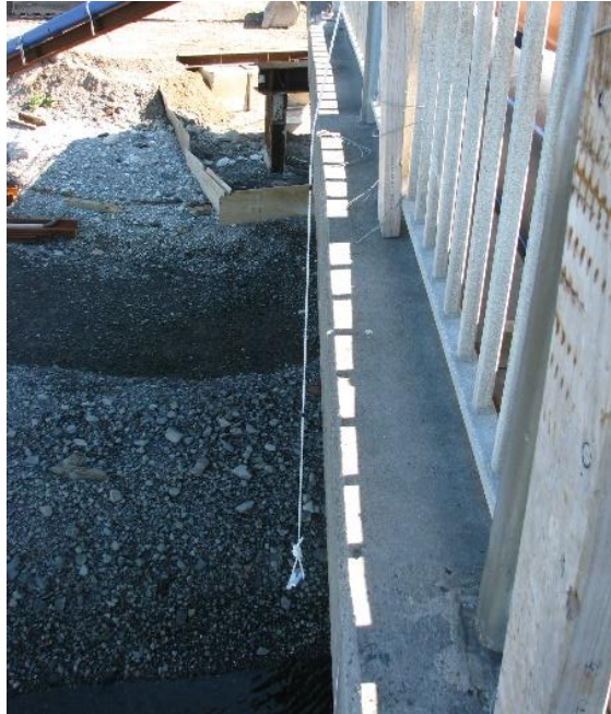
Figure 6-6 Sounding at South Brighton Bridge with construction work in the background on 19 March 2014.
