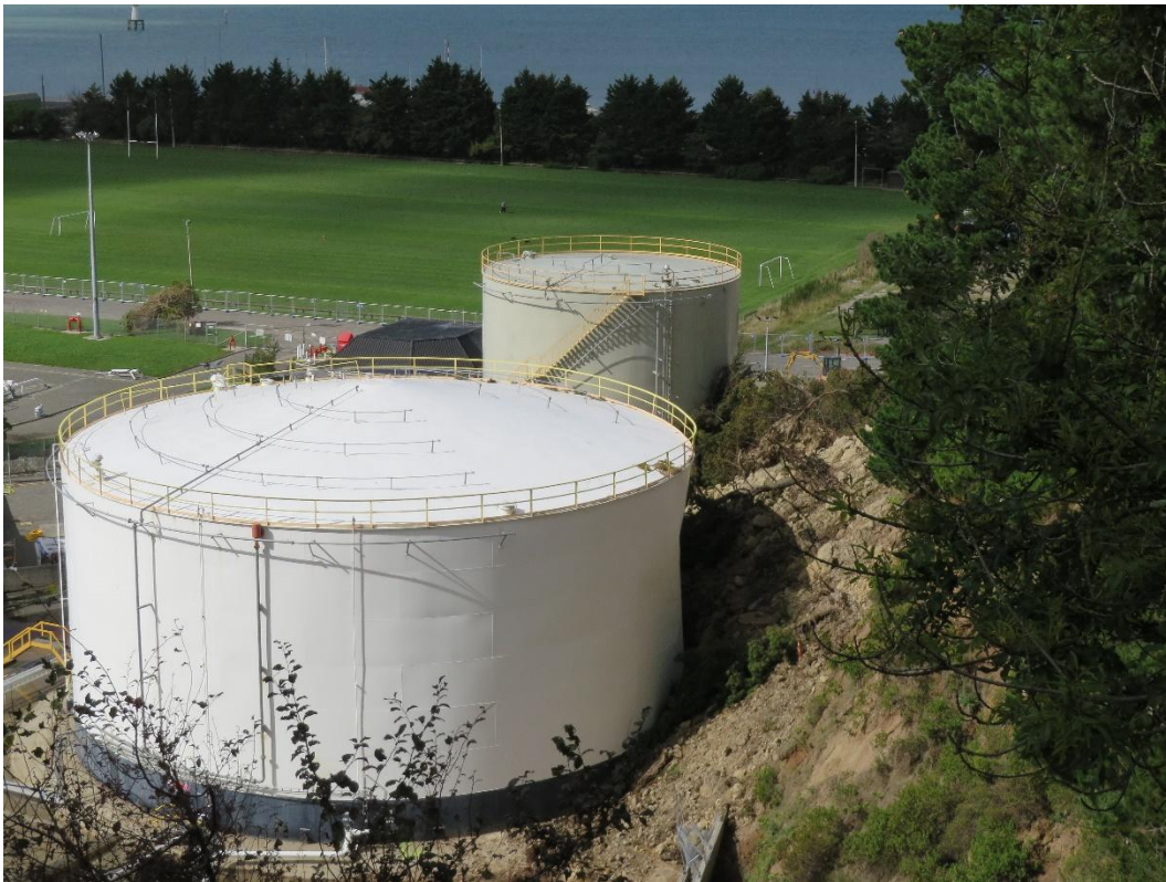
Figure 6-27 Tank impacted by landslide that initiated during periods of heavy rainfall.
