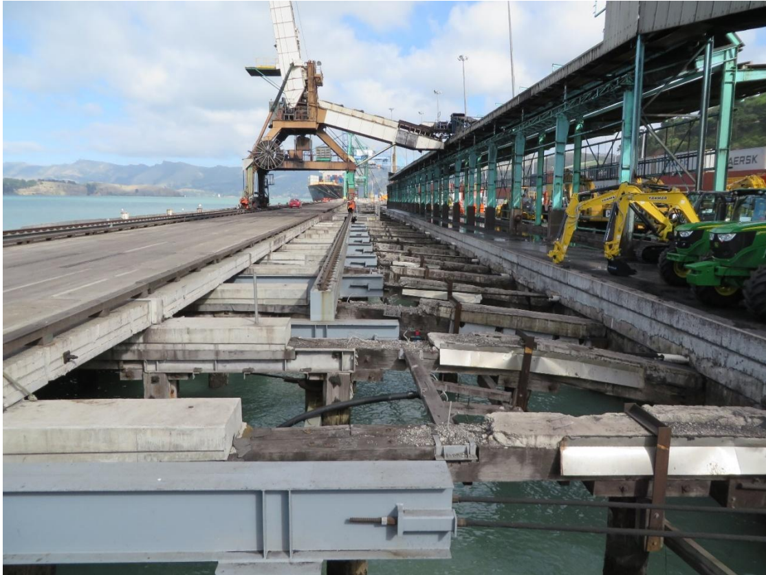
Figure 6-24 Example of visible earthquake induced damage to Cashin Quay in March 2014.
