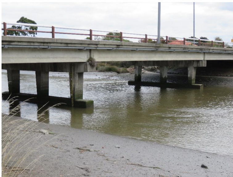
Figure 6-18 Heathcote River Bridge on 20 March 2014.
