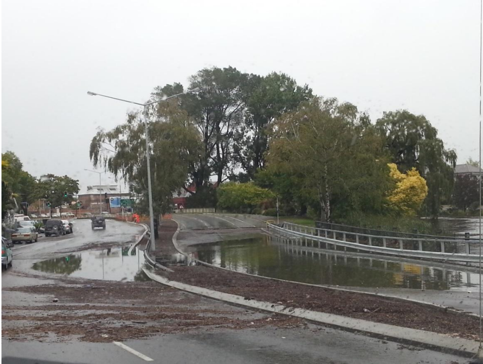
Figure 7-5 Avon River overflow causing surface flooding on Fitzgerald Avenue (-43.524078°, 172.650935°), Central City, Christchurch. This road demonstrates a post-earthquake reconstruction design error. The road should have been built at a higher elevation to avoid flooding. Photo courtesy of Su Young Ko.
