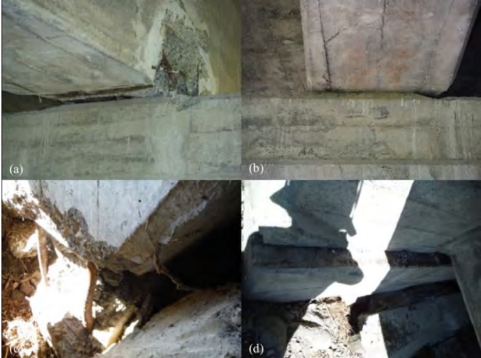
Figure 6.47: Damage at Flaxbourne River Bridge [-41.8085, 174.1458]: (a) Damage at deck-pier connection; (b) Residual transverse deck displacement; (c) Exposed and buckled reinforcement in abutment columns; (d) Residual longitudinal deck displacement.
