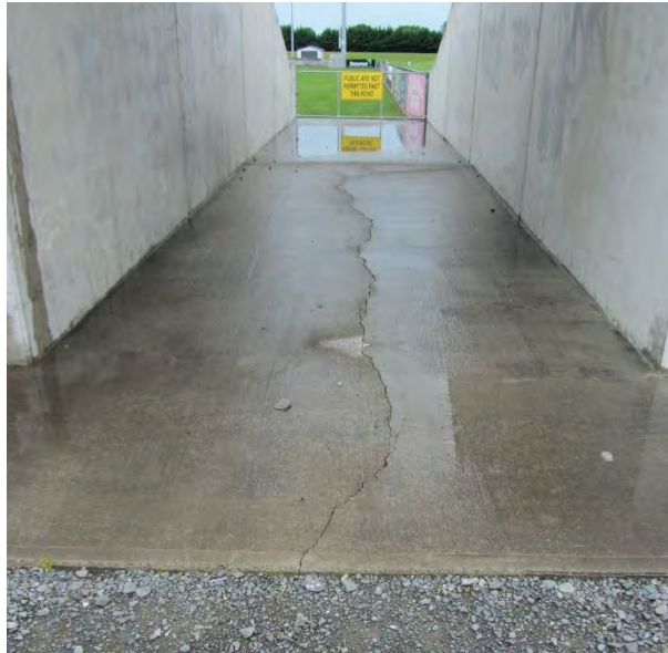
Figure 4.14: Crack in foundation slab on west stand (17 Nov 2016, S41.4993, E173.9569, facing E).
