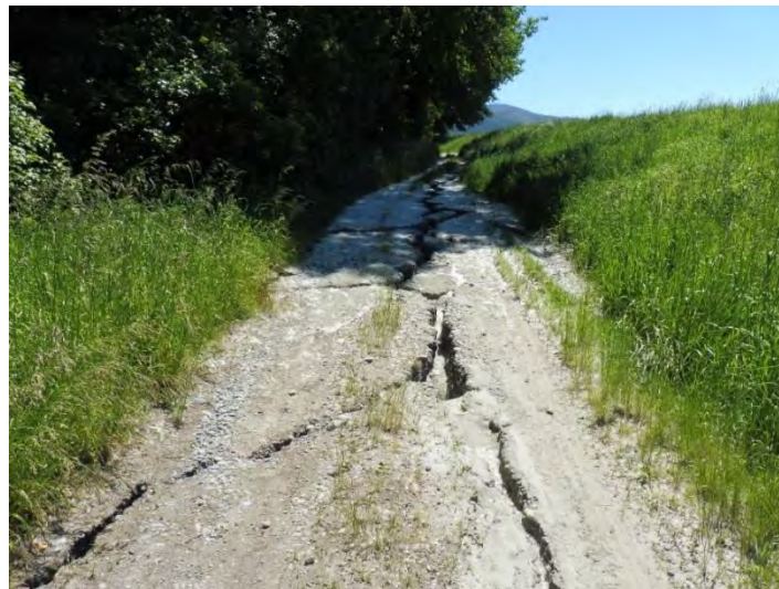
Figure 4.40: Group A cracking along the base of the secondary stopbanks (4 Dec 2016, S41.4487, E173.9738, facing NE).
