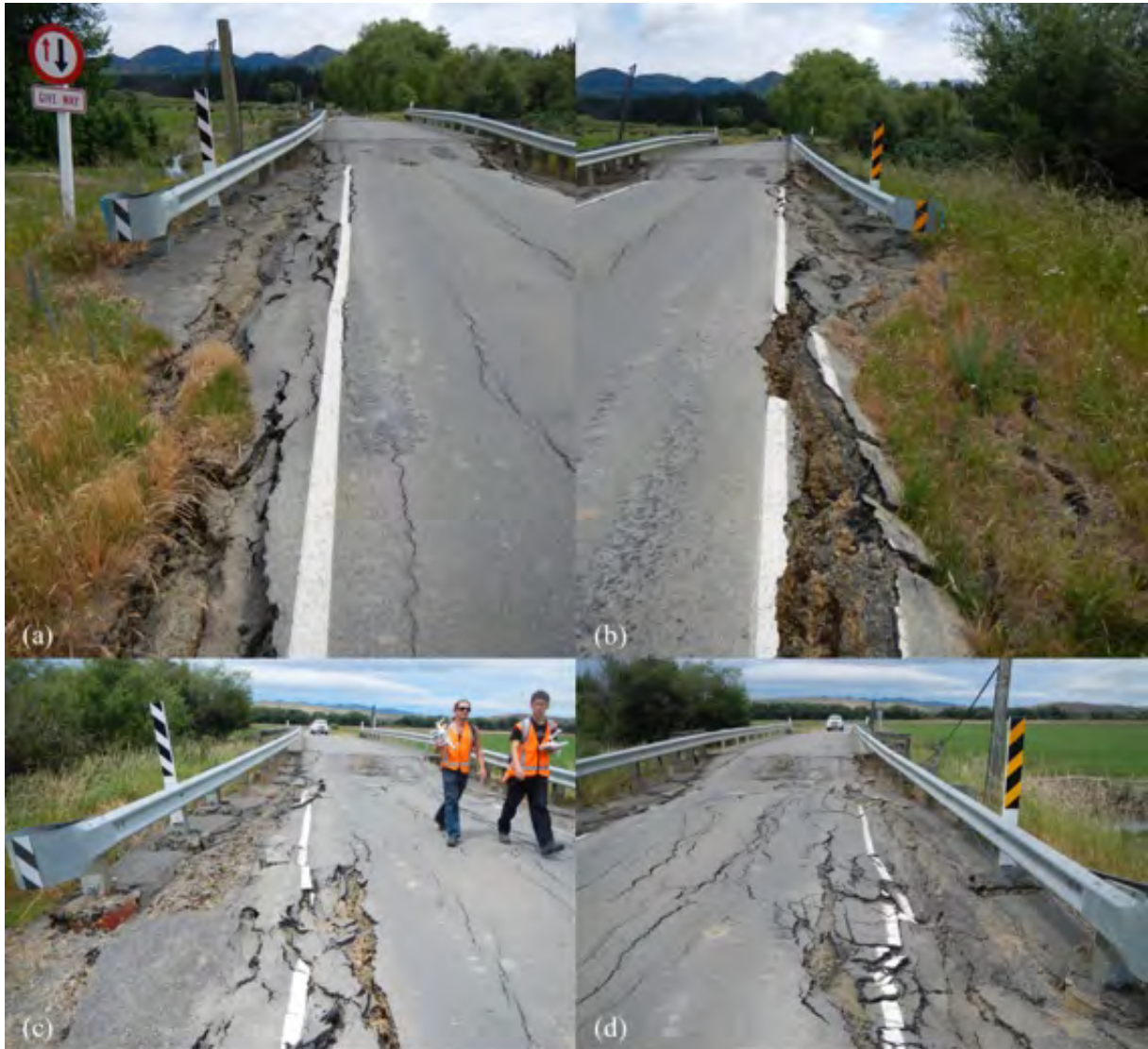
Figure 6.44: Settlement and cracking in approaches to Mt Paul Bridge [-42.6355, 172.9924]: (a) Southwest corner; (b) Southeast corner; (c) Northeast corner; (d) Northwest corner.
