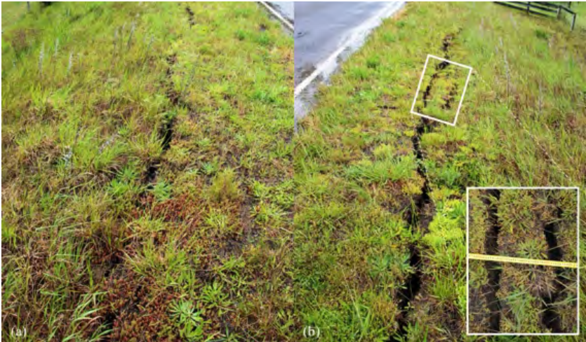
Figure 6.15: Cracks along edges of the western approach embankment for Mason Bridge (looking east towards bridge) [-42.6464, 173.04196]: (a) North side; (b) South side – inset shows close-up of cracks as indicated.
