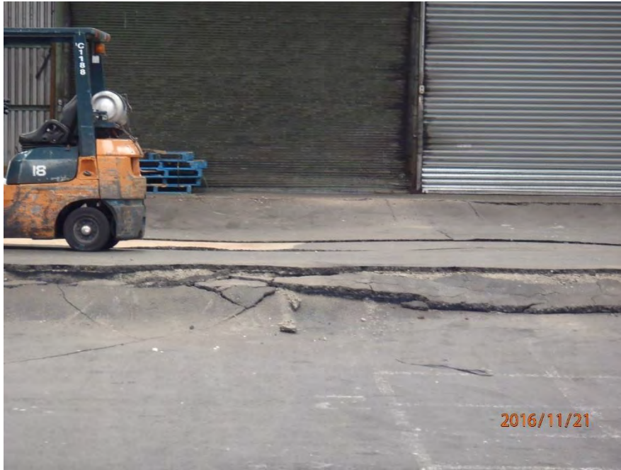
Figure 5.72: Looking west across inside of the S37 building. Approximately 400-550 mm of differential settlement between the ground and the buried precast concrete seawall that runs south-to-north through the center of the building. (S41.279065°, E174.785787°, taken at 1220 hrs on 21NOV16)
