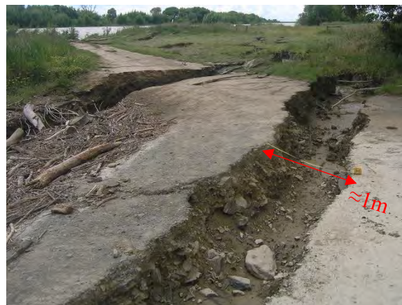
Figure 4.69: Lateral spreading at the east end of the rowing club site. Note: measuring tape set to 1m. (17 Nov 2016, S41.4882, E174.0105, facing E).
