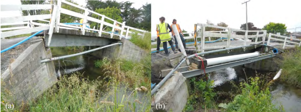
Figure 6.66: Back rotation of east and west abutments at Lyell Creek Bridge [-42.3892, 173.6773]: (a) Looking south at bridge; (b) Looking north at bridge.
