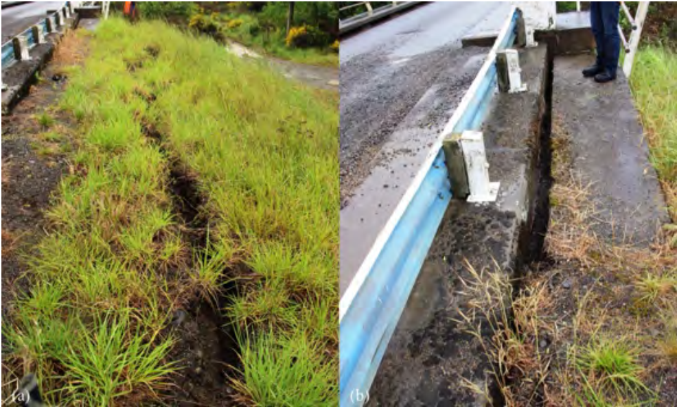
Figure 6.4: South side of western approach embankment to Waiiau River Bridge [-42.6556, 173.03]: (a) Lateral cracks in embankment side; (b) Settlement and outward movement at abutment wall.
