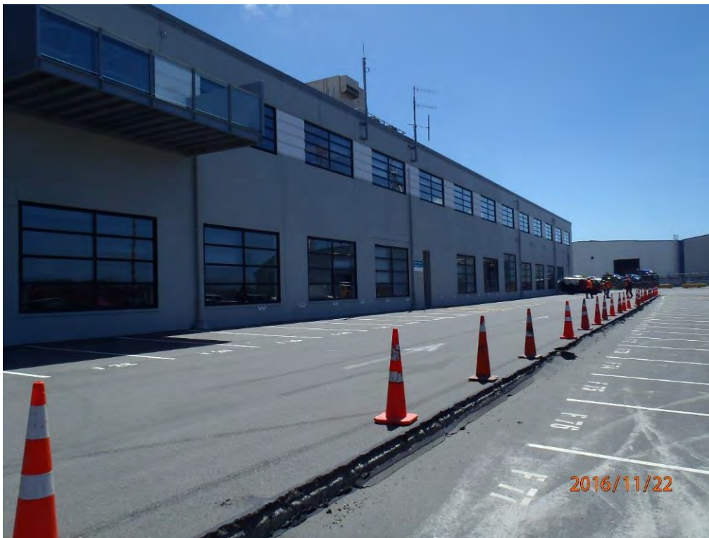
Figure 5.68: Southeast side of Building S39 and a buried segment of the Fryatt Quay Wharf deck parallel to the building. Fill to the south of the buried mass concrete seawall/wharf settled 220 mm relative to the pile-supported building and wharf deck. (S41.277984°, E174.785776°, taken at 1230 hrs on 22NOV16)
