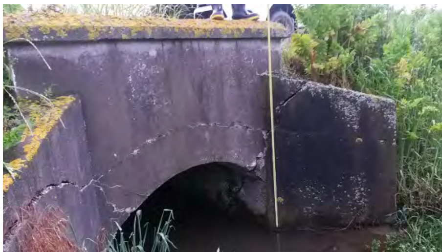
Figure 6.81: Cracking in the concrete at Hawthorne Road culvert (8 Dec 2016, facing northwest) [-42.3900, 173.6675].
