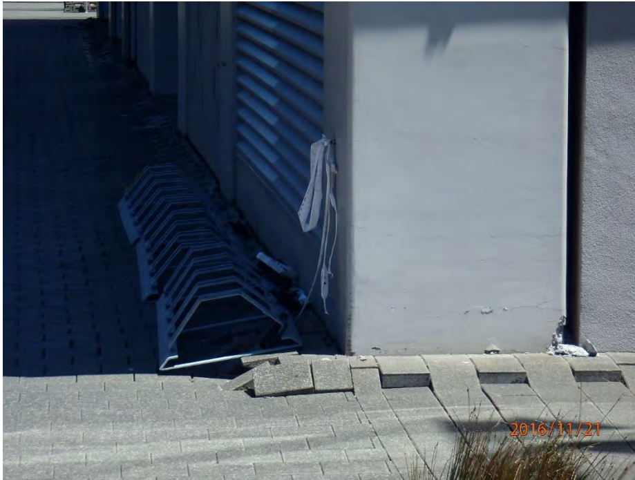
Figure 5.80: Looking west at southeast corner of the S building at which fill settled approximately 100 to 200 mm relative to pile-supported building. (S41.278285°, E174.784757°, taken at 1243 hrs on 21NOV16)
