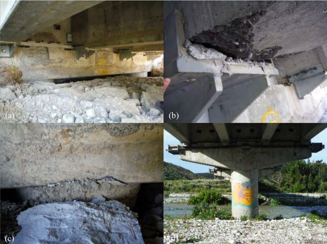
Figure 6.56: Damage at Waima River Bridge [-41.9021, 174.1122]: (a) South abutment facing south; (b) Damage to concrete beams around retrofit brackets; (c) Cracking at top of abutment pile; (d) Tilt of southernmost pier facing north.
