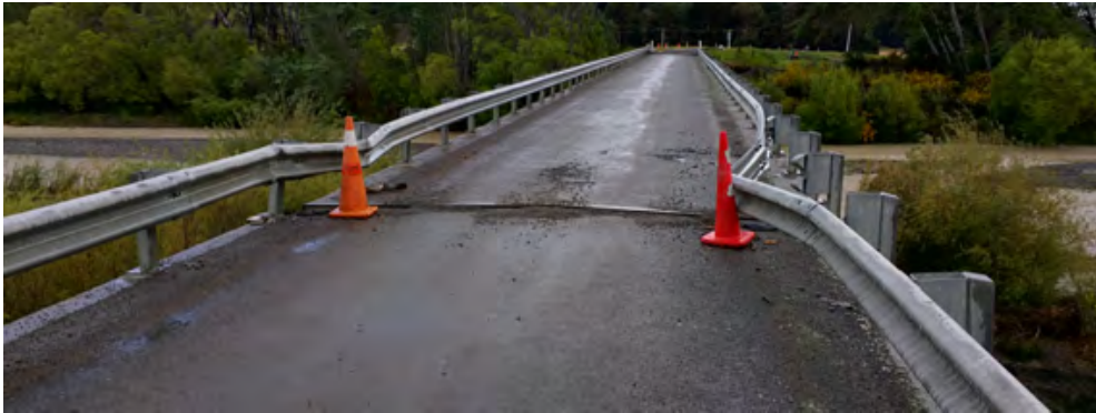
Figure 6.25: Buckling of guard rails at centre expansion joint of Lower Mason Bridge indicating that the two main deck sections have undergone permanent inward deformation. Photo facing south [-42.6343, 173.0664].
