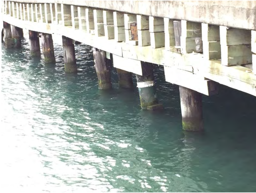
Figure 5.44: Looking west along southern end of King’s Wharf. Westward tilt of piles is visible. (S41.281281° W174.784097°, taken on 17NOV16)
