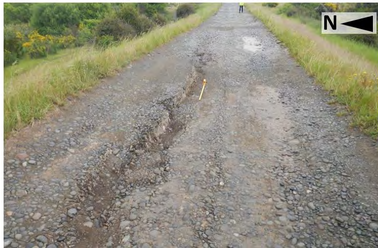
Figure 4.36: Cracking along the top of the southern stopbank of the Wairau Diversion (Tape set at 1 m) (17 Nov 2016, S41.4414, E174.0219, facing W)
