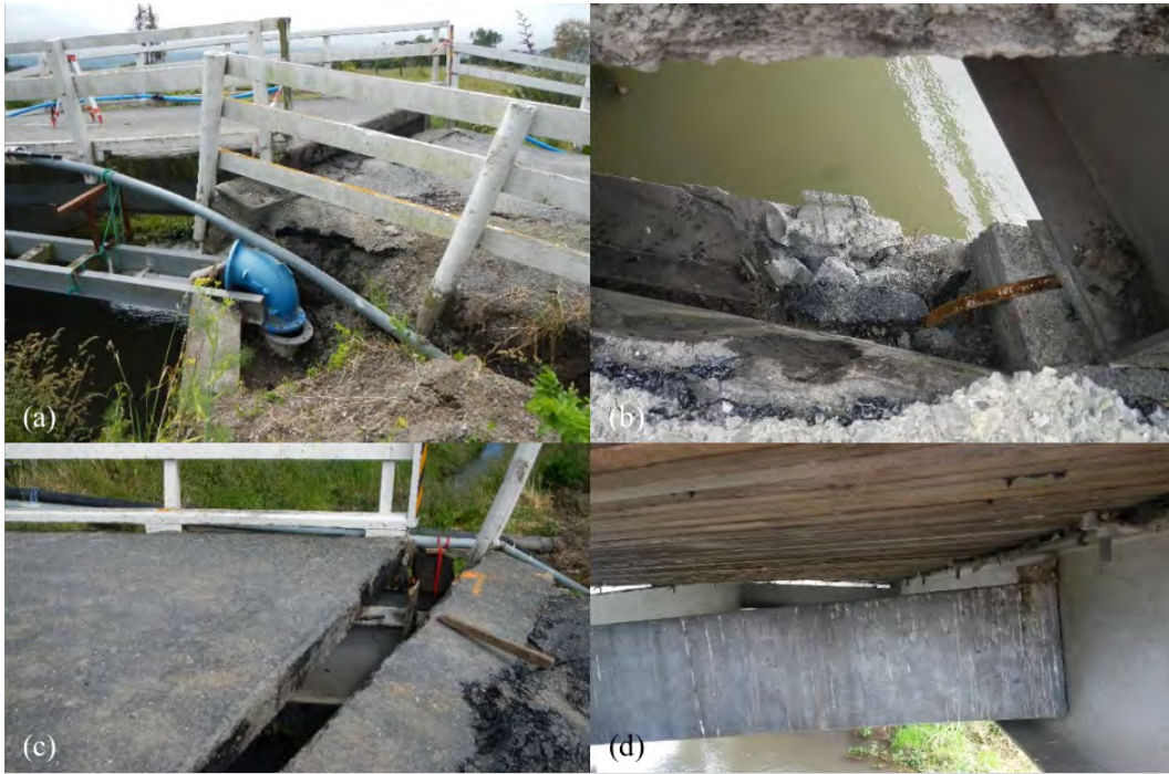
Figure 6.68: Damage at Lyell Creek Bridge [-42.3892, 173.6773]: (a) Eastern end of bridge looking north; (b) Bent anchor bars at east abutment-deck connection; (c) Gap between deck and west abutment looking south; (d) Twisting of deck beams.
