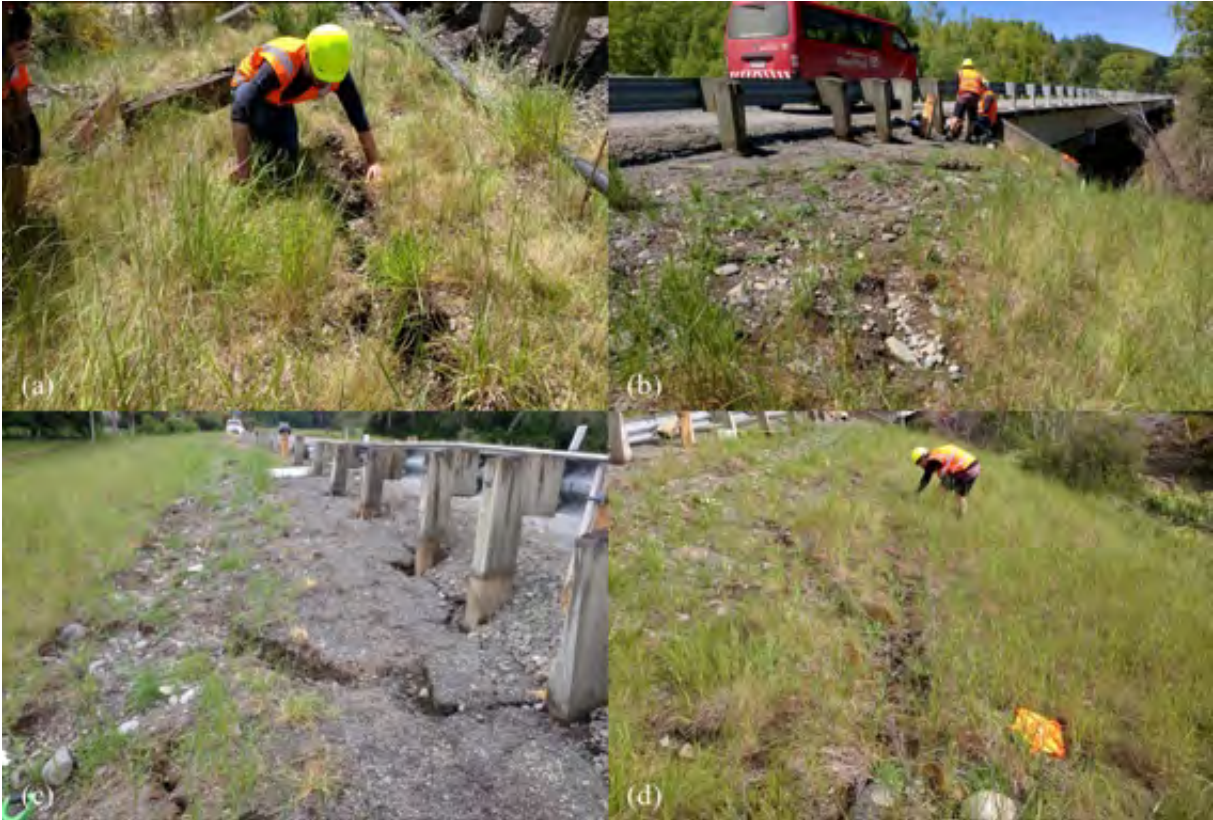
Figure 6.21: Cracking in sides of approach embankments at Lower Mason Bridge. (a) West side of south approach looking north [-42.6353, 173.0662]; (b) East side of south approach looking north [-42.6353, 173.0662]; (c) and (d) West side of north approach looking north and south, respectively [-42.6330, 173.0666].
