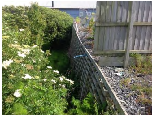
Figure 4.138: Failure of retaining wall (– date to be added in V2.0 of report, S42.3964, E173.6793, facing N). Note: Cracks visible in the car park on the retained side of the wall.
