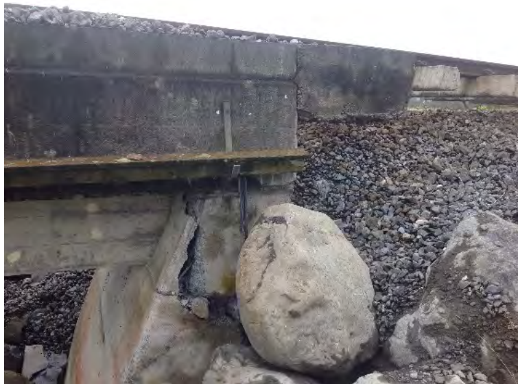
Figure 6.72: Damage to the north abutment of the Middle Creek Railway Bridge facing northwest [-42.3670, 173.6861].
