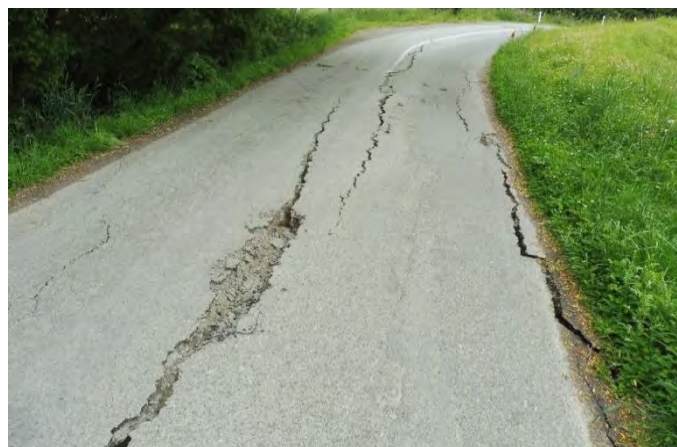
Figure 4.45: Cracks in the access road that crosses a historic river channel at the Equestrian Park (15 Nov 2016, S41.4436, E173.9790, facing E, Marlborough District Council 2016).
