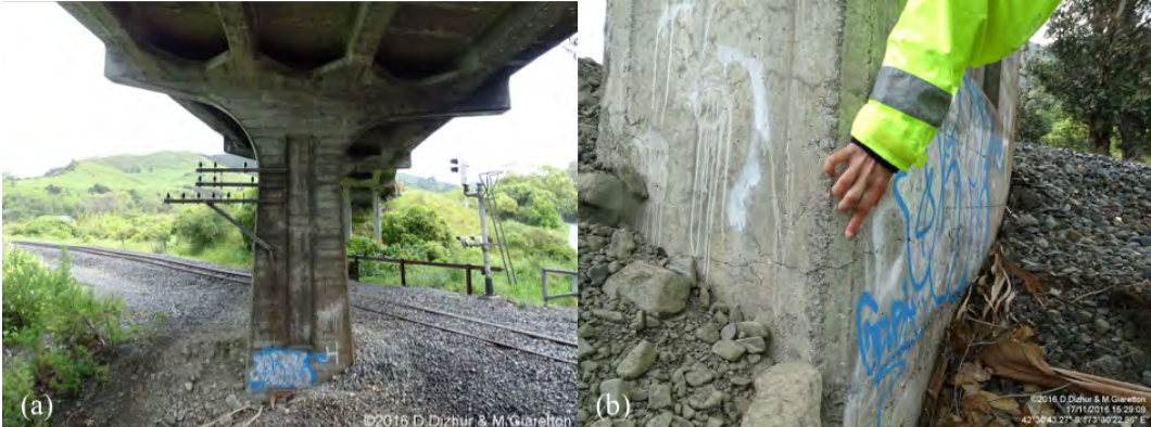
Figure 6.85: Damage at Oaro Overbridge [-42.512089, 173.506345]: (a) Northernmost central hammerhead pier looking south; (b) Flexural cracking at base of northernmost hammerhead pier. Photos courtesy of D. Dizhur and M. Giaretton.
