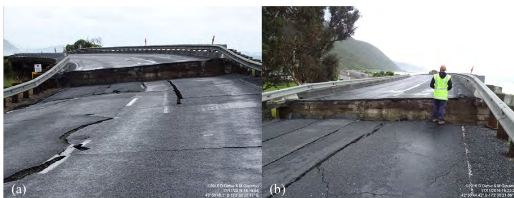
Figure 6.83: Settlement and severe approach roadway cracking at southern abutment to Oaro Overbridge [-42.5121, 173.5063] looking north. Photos by D. Dizhur and M. Giaretton.
