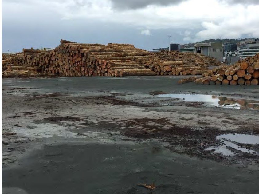
Figure 5.21: Sandy liquefaction ejecta in the log stacking area in the northeast corner of CentrePort (Sample S13). Area of hydraulic fill reclamation. (S41.274972°, E174.788347°, taken on 17 NOV16)
