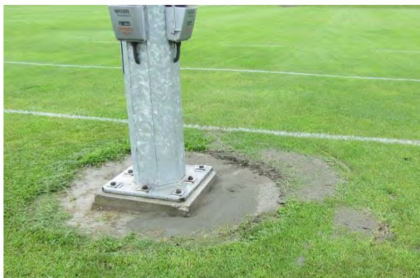
Figure 4.13: Liquefaction ejecta at flood light tower (17 Nov 2016, S41.5003, E173.9572, facing N).
