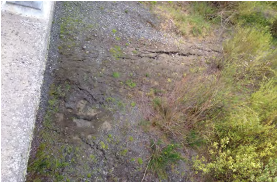
Figure 6.26: Cracks in northern river bank on eastern side of bridge. Photo taken from bridge deck. Riverward direction is down for this orientation [-42.6342, 173.0665].
