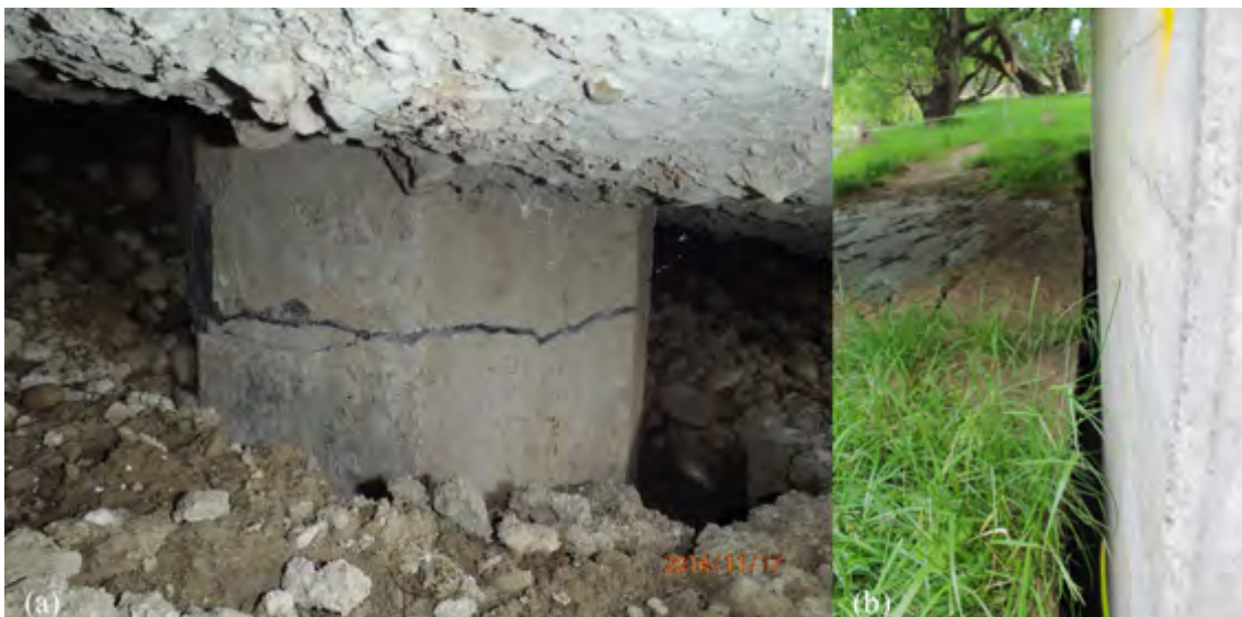
Figure 6.54: Pile and footing damage at Needles Creek Bridge [-41.8217, 174.1370]: (a) Crack in pile for south abutment; (b) Soil-footing gapping at pier 3.
