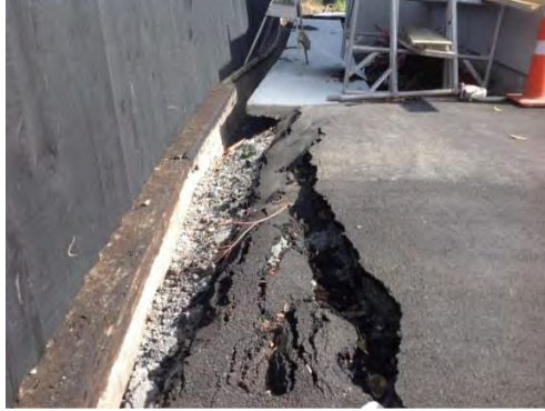
Figure 4.137: Cracks behind retaining wall (– date to be added in V2.0 of report, S42.3971, E173.6798, facing N).
