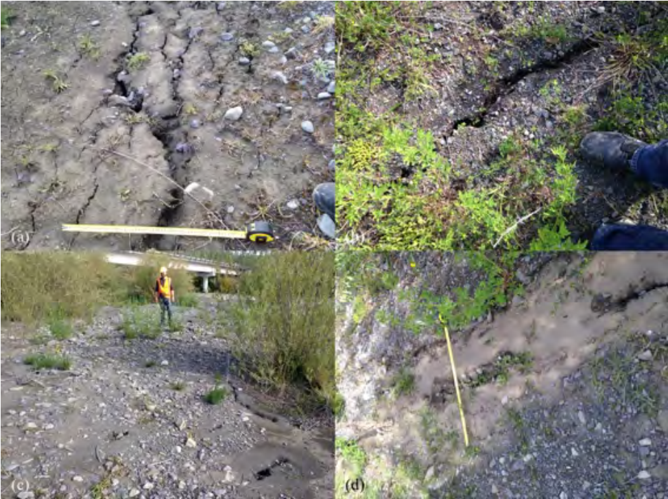
Figure 6.28: Representative photos of the lateral spreading cracking and liquefaction ejecta observed on the Northern river bank near the bridge in the areas indicated by Figure 6.19.
