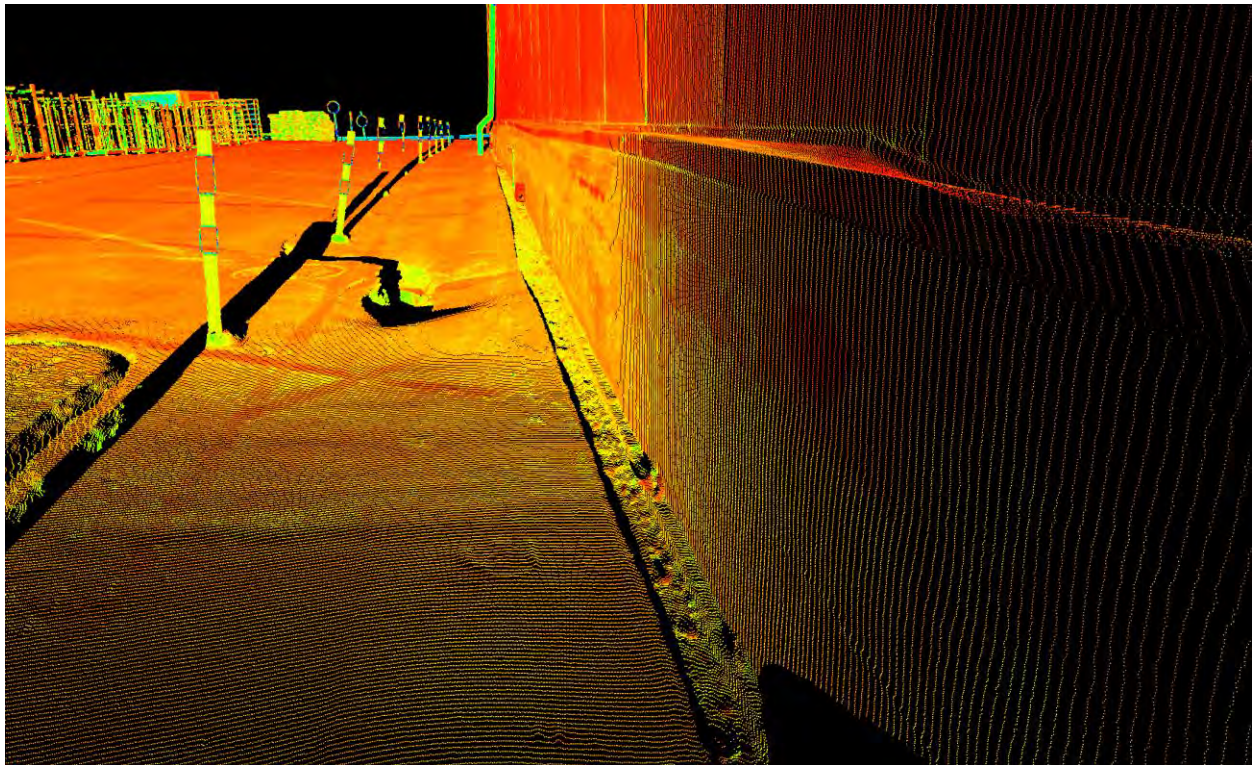
Figure 5.52: Perspective view of LiDAR scan looking westward showing the horizontal separation from building foundation and settlement of pavement observed on the south side of the CS building looking west (colored indicates intensity). The separation varies from 0.23 m wide to 0.03 m wide horizontally from the building's eastern side to its western side.
