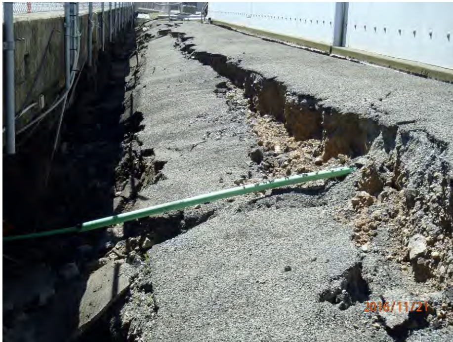
Figure 5.54: Looking north along the west wall of the CS building. The ground settled approximately 530 mm relative to the pile-supported bulkhead of King's Wharf, which is shown at the left side of the photograph. (S41.280923° E174.784389°, at 1411 hrs on 21NOV16)
