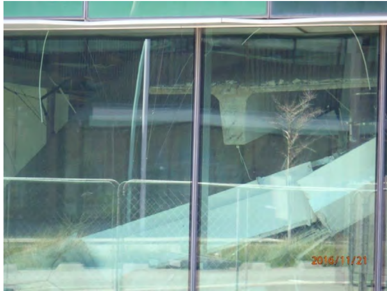
Figure 5.82: Pull-out and partial collapse of Level 1 floor slab in the S building taken along the west wall of the building. (S41.277982°, E174.784255°, taken at 1246 hrs on 21NOV16)
