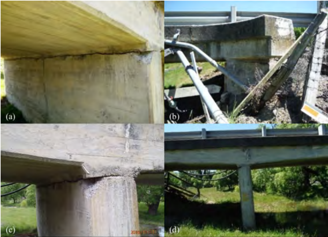
Figure 6.55: Structural damage at Needles Creek Bridge [-41.8217, 174.1370]: (a) Cracking across length of pier 1 looking south; (b) Deck sheared off of abutment 1 facing west; (c) Cracking at pier 1 facing east; (d) Tilting of pier 1 facing east.
