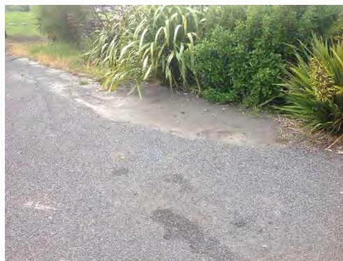
Figure 4.96: Liquefaction in driveway on Mt Fyffe Road (- date to be added in V2.0 of report, S42.3800, E173.6600).
