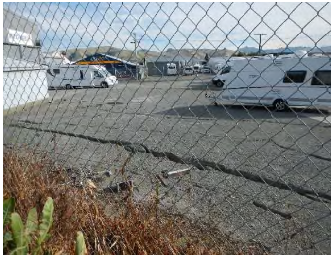
Figure 4.19: Ground damage to industrial properties along Park Terrace (5 Dec 2016, S41.5122, E173.9649, facing SE).
