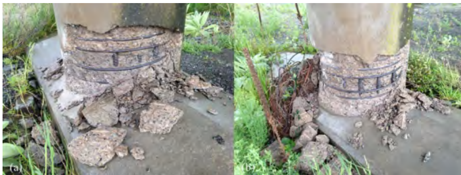
Figure 6.17: Severe examples of plastic hinging at base of Mason Bridge piers (looking north) [-42.6469, 173.0432].
