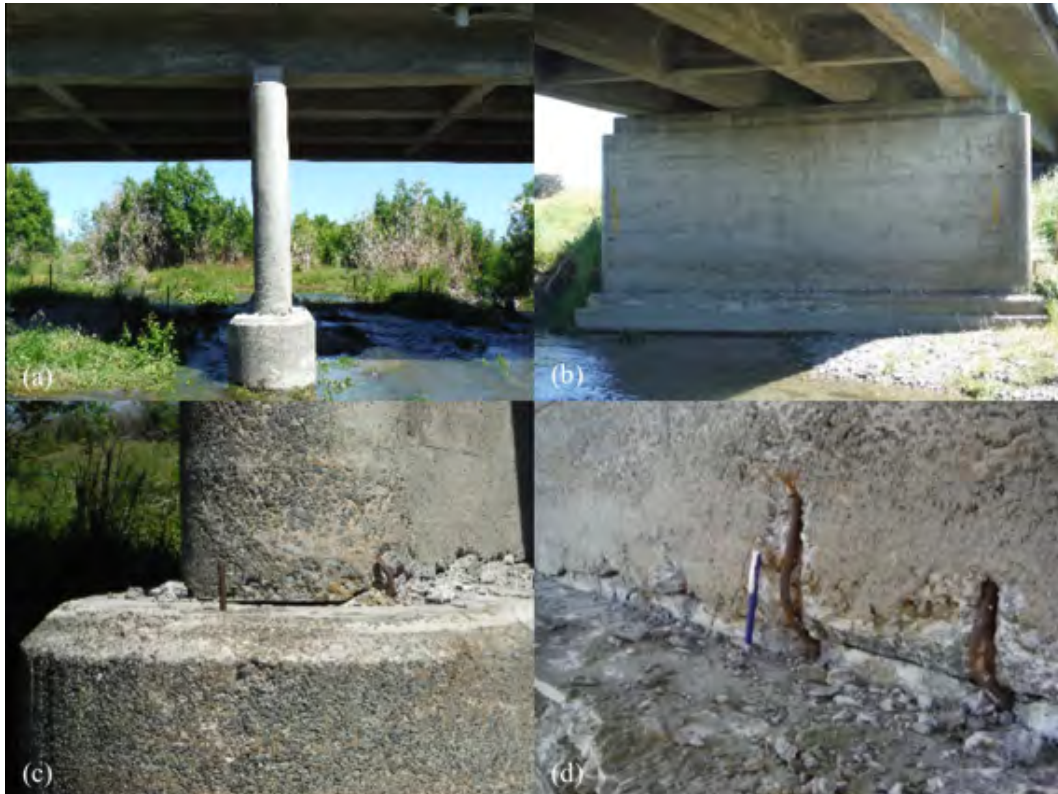
Figure 6.48: Substructure damage at Flaxbourne River Bridge [-41.8085, 174.1458]: (a) Tilted pier; (b) Cracking at pier base; (c) and (d) Cracking and exposed reinforcement at base of piers.
