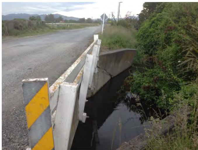
Figure 6.82: Failure of the northwest wingwall of the Lyell Creek culvert on Mill Road (8 Dec 2016, facing west) [-42.3765, 173.6788].
