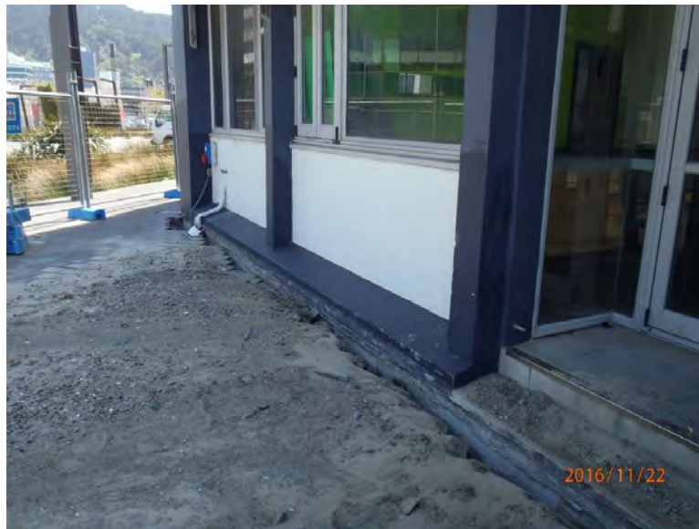
Figure 5.71: Southwest wall of TC building with liquefaction ejecta and 150 mm of ground settlement relative to building. (S41.277858°, E174.785081°, taken at 1246 hrs on 22NOV16)
