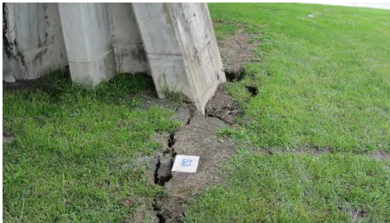
Figure 4.15: Cracking adjacent to the southern pier of the Opawa River Bridge (14 Nov 2016, S41.5006, E173.9616, facing N).
