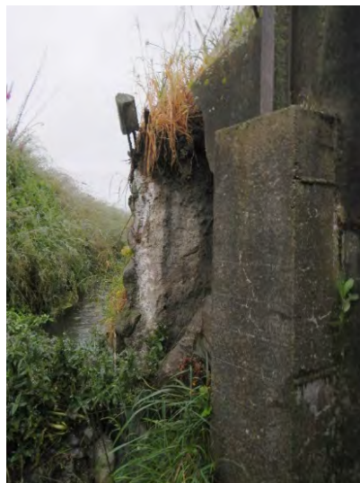
Figure 6.76: Damage to the north abutment on the west side of the bridge (8 Dec 2016, facing north) [-42.3692, 173.6547].
