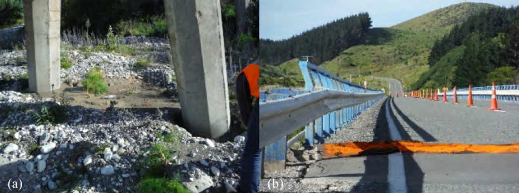
Figure 6.57: Geotechnical damage at Waima River Bridge site [-41.9021, 174.1122]; (a) Ejecta at piers of railroad bridge 50 m upstream; (b) Settlement at south approach looking north.
