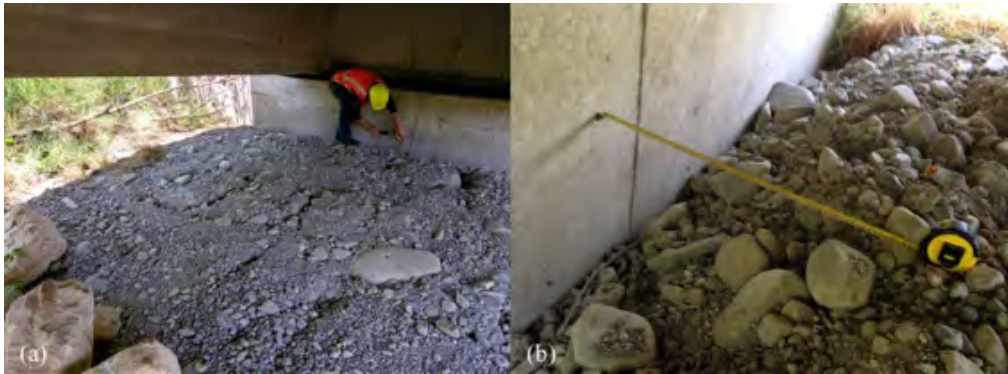
Figure 6.23: Cracking and gapping in fill below bridge deck at northern abutment to Lower Mason Bridge indicating riverward movement of the fill [-42.6334, 173.0666]: (a) Looking north; (b) 60 cm gap between wall and fill.
