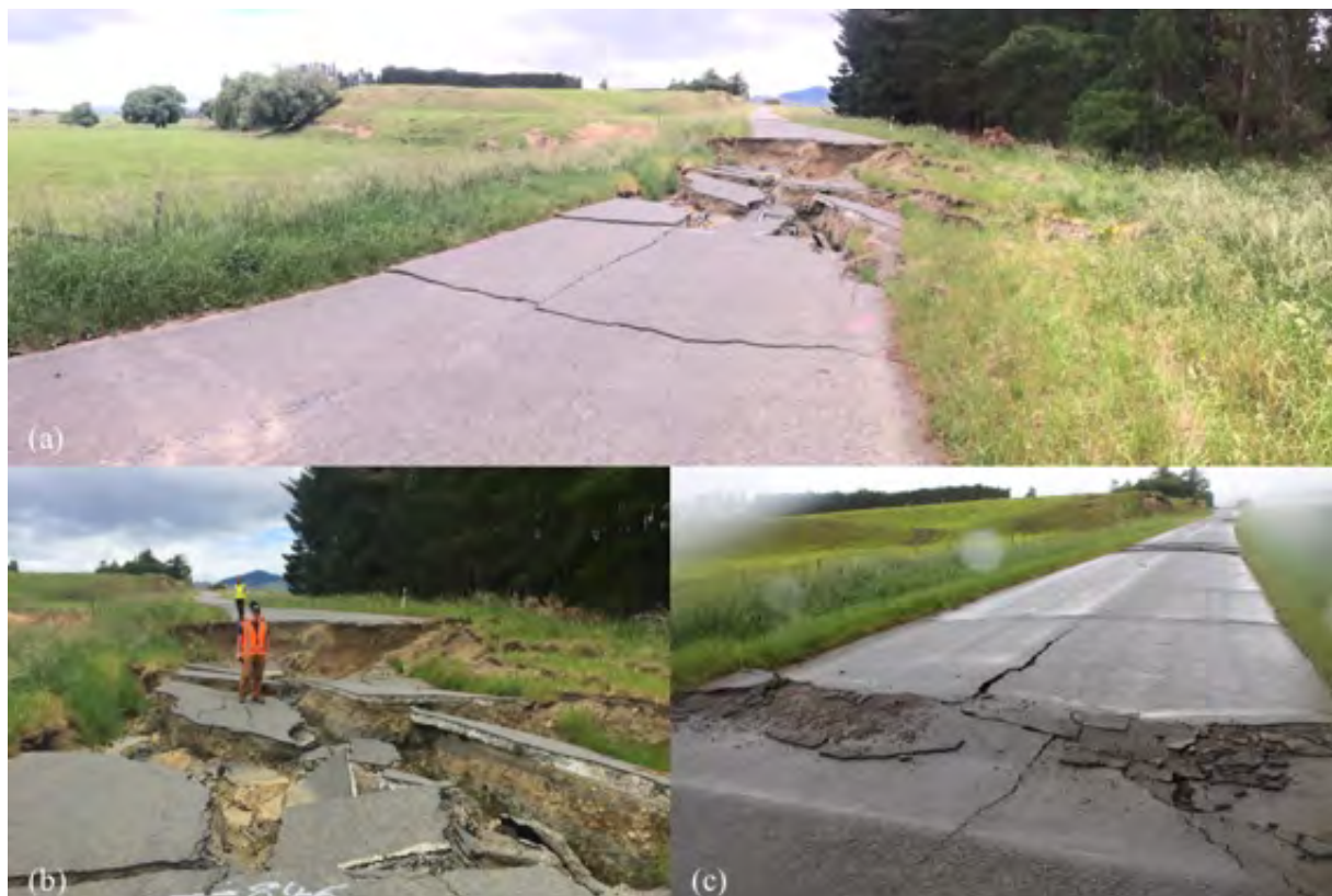
Figure 6.39: Failure and severe cracking on Leslie Hills Road (photos all taken looking west) [-42.6306,172.9895]: (a) Overview of major failure area; (b) Closer view of failure area; (c) Cracking to west of failure area.
