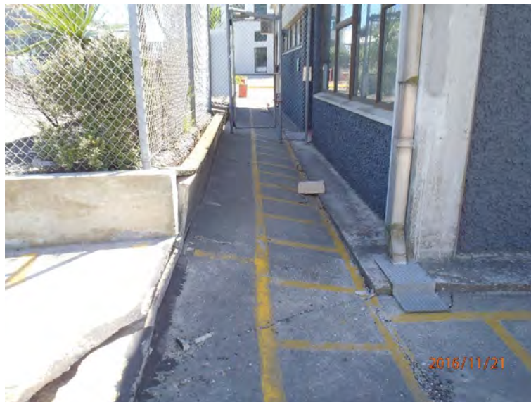
Figure 5.49: Uniform settlement (230-260 mm) of the building relative to ground supported on old bulkhead piles of Pipitea Wharf. Looking north along western wall of CPH building. The perimeter walkway slopes down towards the building at 11 degrees over 1.35 meters. (S41.278395° E174.785639°, taken at 1225 hrs on 22NOV16)
