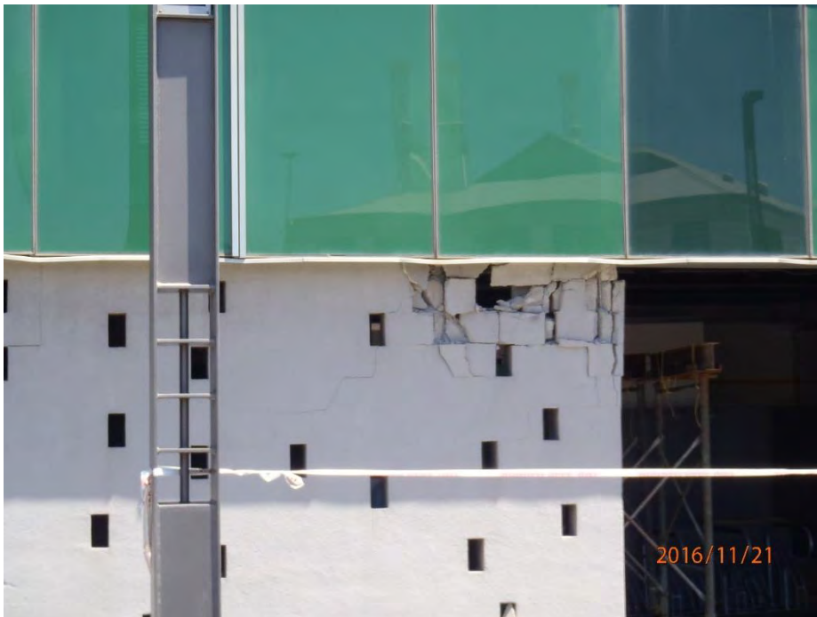
Figure 5.81: Damage to ground floor infill wall on the east side of the S building (S41.278114°, E174.784715°, 1241 hrs on 21NOV16)
