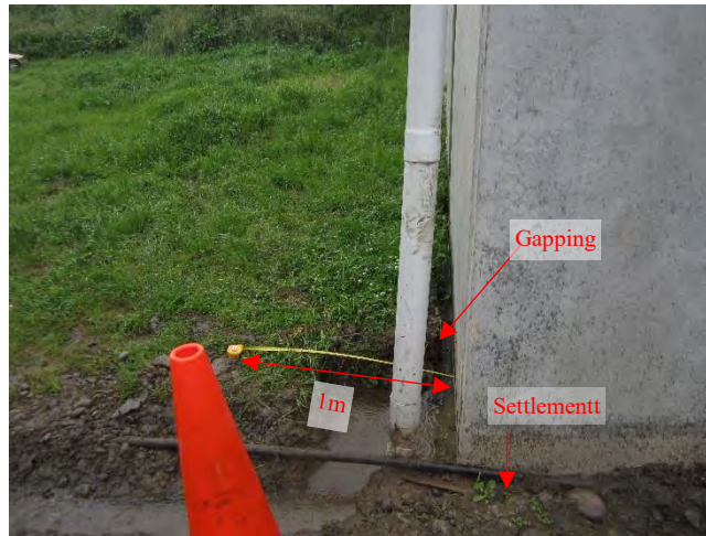
Figure 4.83: Gapping and settlement on northern side of club house (17 Dec 2016, S41.4767, E173.9851, facing E).
