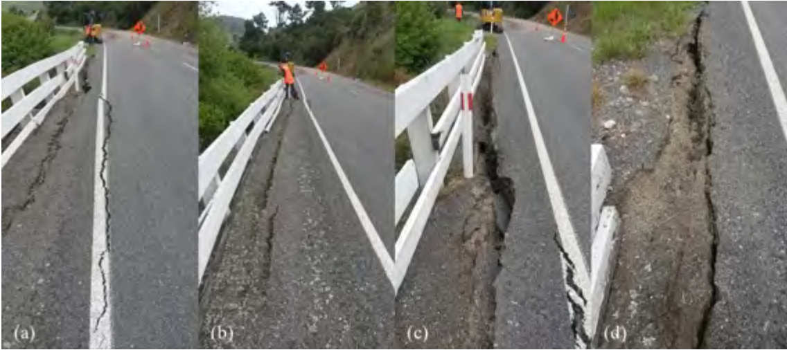
Figure 6.37: Cracks on free-face side of roadway on Highway 7 looking south [-42.6310, 172.7718]. Location and site layout shown in Figure 6.33.
