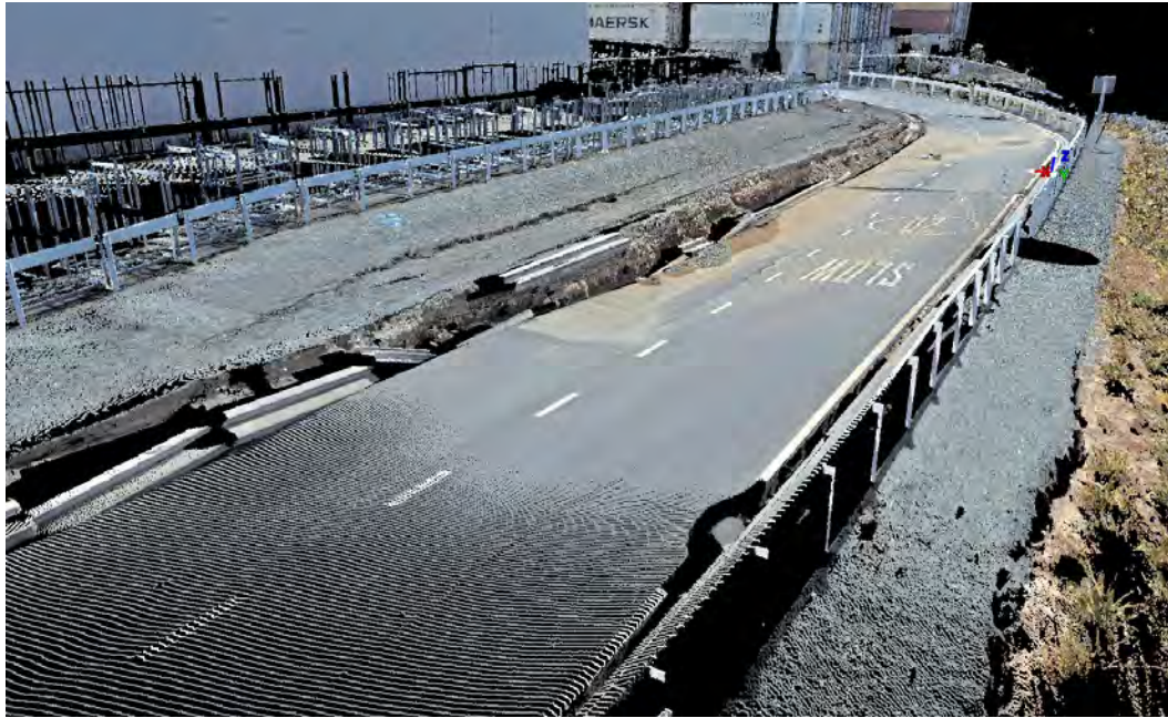
Figure 5.57: LiDAR scan of damage to the asphalt pavement and concrete curbs on the access road located south of the CS building. The vertical offset is approximately 1.1 m. This view is looking to the northeast.
