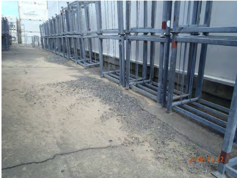
Figure 5.53: Gravelly liquefaction ejecta looking east along the northern wall of the CS building. (S41.280528° E174.784984°, taken at 1651 hrs on 22NOV16)
