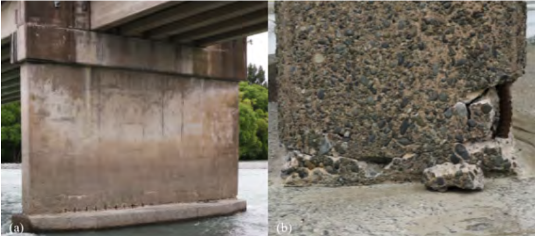
Figure 6.8: Structural damage to base of piers for Waiau River Bridge [-42.6553, 173.0351]: (a) Cracking at pile cap interface; (b) Exposure and buckling of longitudinal bars.
