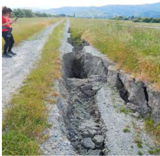
Figure 4.49: Damage to the secondary stopbank at Blind Creek (5 Dec 2016, S41.4407, E173.9791, facing W).
