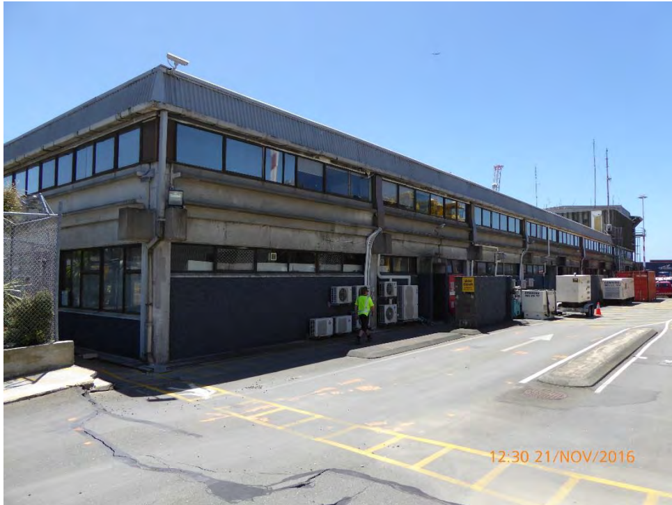
Figure 5.48: Uniform settlement of CPH building which is founded on shallow foundations that apparently displaced downward the same amount as the surrounding fill. This photo is looking northeast at the southwest corner of the building. (S41.278395° E174.785639°, taken at 1230 hrs on 21NOV16)
