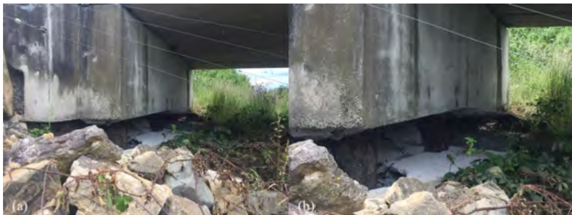
Figure 6.43: Settlement below abutment at Mt Paul Bridge [-42.6355, 172.9923].
