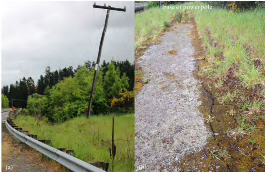
Figure 6.16: Northern side of eastern approach to Mason Bridge (looking west) [-42.6475, 173.04465]: (a) Power pole has moved down the slope of an embankment directly adjacent to bridge approach embankment; (b) Cracks parallel to roadway in embankment fill.
