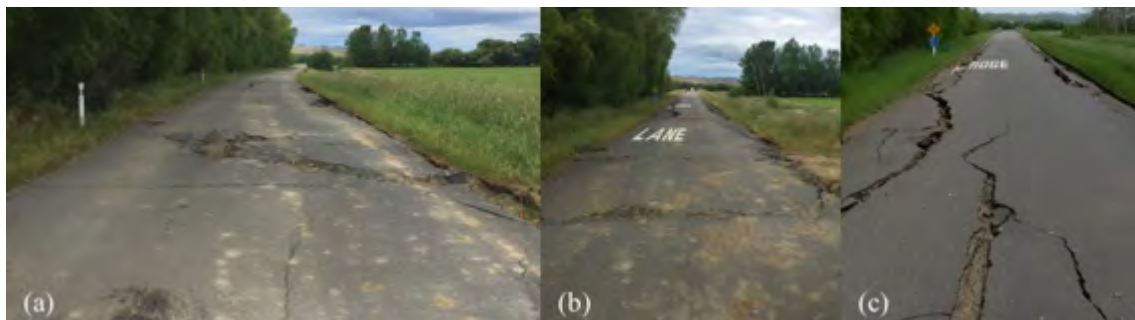
Figure 6.42: Cracking in roadway approaching Mt Paul Bridge from the north along Leslie Hills Road [-42.6355, 172.9924].
