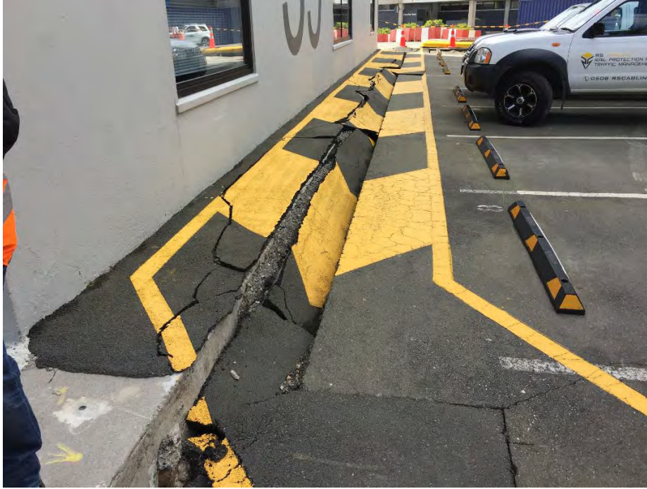
Figure 5.69: Looking southeast along southwest wall of S39. Fill settled approximately 190 mm relative to pile-supported building at the northwest corner of the building (shown on lower left corner of photo), and magnitude of settlement decreased south-eastward along this wall. (S41.277994°, E174.785467°, taken on 17NOV16)
