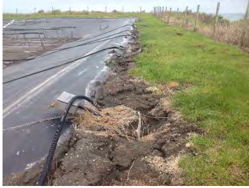
Figure 4.132: Rotation of the aeration-line control posts on the south side of KK-OPS (– date to be added in V2.0 of report, S42.3669, E173.6867, facing E).
