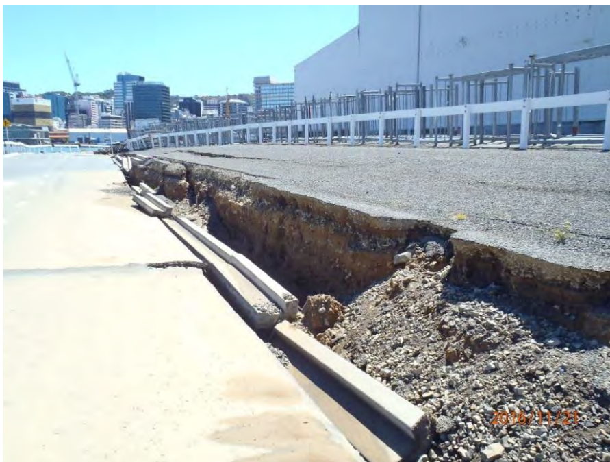
Figure 5.56: Approximately 1.1 m of vertical offset resulting from the southward lateral movement of the southern edge of CentrePort reclaimed land near its western side. Looking west near the southern wall of the CS building. (S41.281701° E174.785268°, taken at 1427 hrs on 21NOV16)
