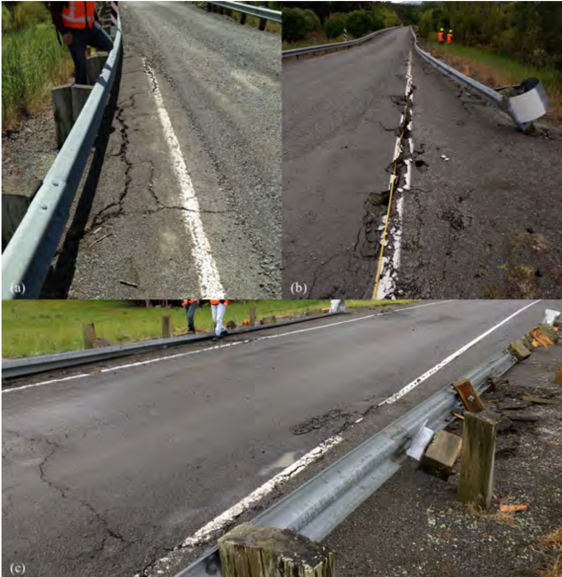
Figure 6.20: Cracking in approach roadways at Lower Mason Bridge: (a) Western side of south approach looking north [-42.6353, 173.0662]; (b) Eastern side of south approach looking north [-42.6353, 173.0662]; (c) North approach looking northwest across road [-42.6330, 173.0666].
