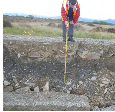
Figure 4.63: Measurement of vertical relative displacement along crack, tape set at 150 cm (17 Nov 2016, S41.5012, E174.0603, facing N).
