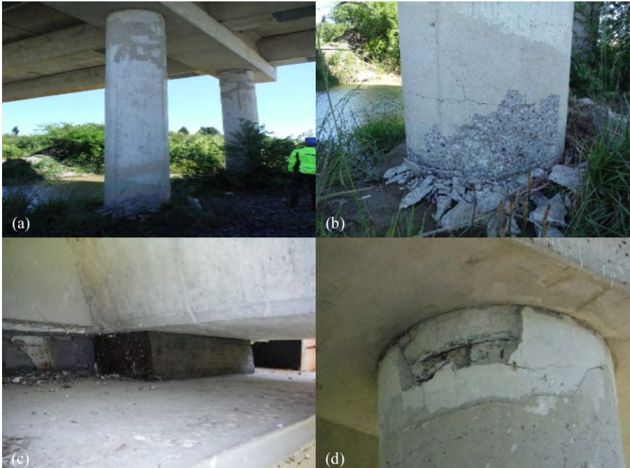
Figure 6.58: Damage at Awatere River Bridge [-41.6585, 174.077]: (a) Flexural damage at top and bottom of pier column near middle of bridge facing west; (b) Spalling of concrete at base of pier column; (c) Residual displacement in bearing pad at southern abutment; (d) Damage to previously grouted area.
