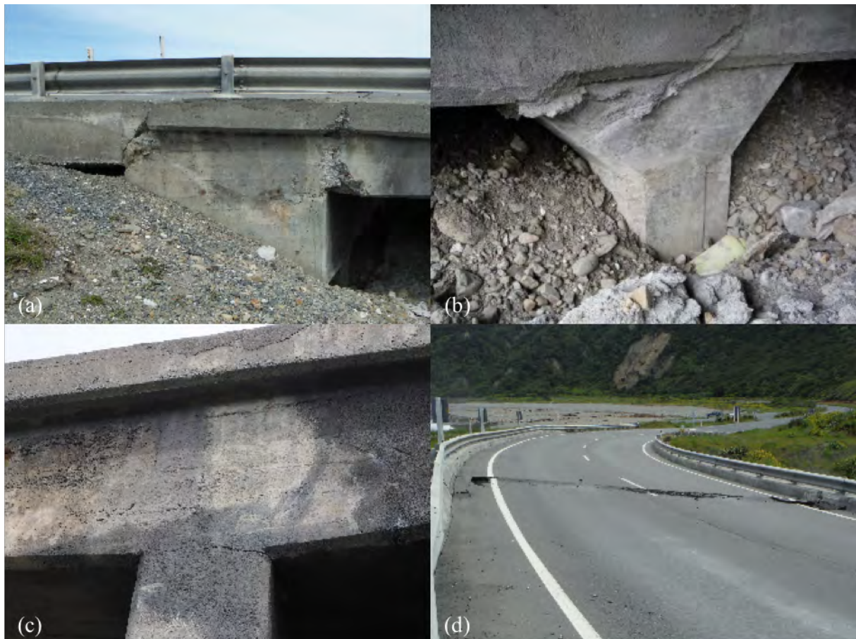
Figure 6.60: Damage observed at Mororimu Stream Bridge [-42.2173, 173.8673]: (a) Cracking in eastern abutment looking south; (b) Abutment column cracking; (c) Cracking at top of pier; (d) Settlement of eastern approach looking west.
