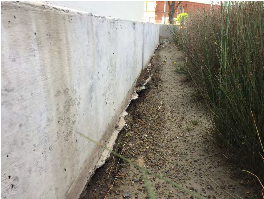
Figure 5.70: Looking southwest along northwest wall of S39. Fill settled 50-100 mm relative to pile-supported building. (S41.277882°, E174.785371°, taken on 17NOV16)
