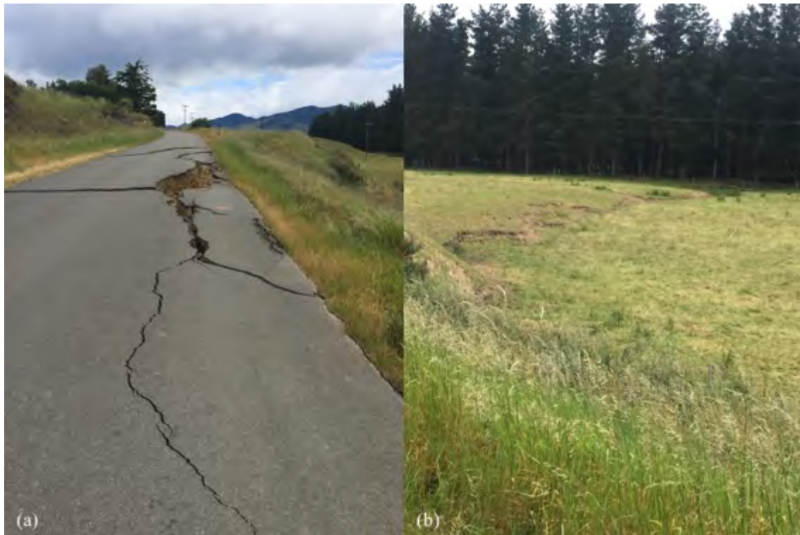
Figure 6.40: Damage west of failure area on Leslie Hills Road (both photos taken looking west) [-42.6306,172.9895]: (a) Cracking and failure of the road on free face of embankment; (b) Adjacent cracking through paddock.
