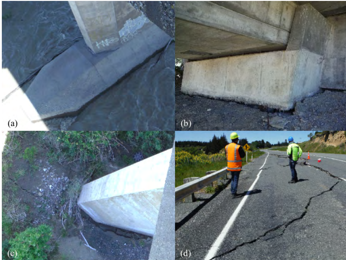
Figure 6.63: Damage at Clarence River Bridge [-42.1592, 173.9103]: (a) Cracking in top of footing; (b) Settlement of fill ahead of abutment; (c) Soil gapping at base of pier; (d) Spreading cracks in roadway at southern approach looking south.
