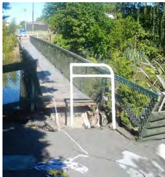
Figure 4.24: Damage to footbridge abutment at the end of Elizabeth Street (17 Nov 2016, S41.5087, E173.9636, facing W).
