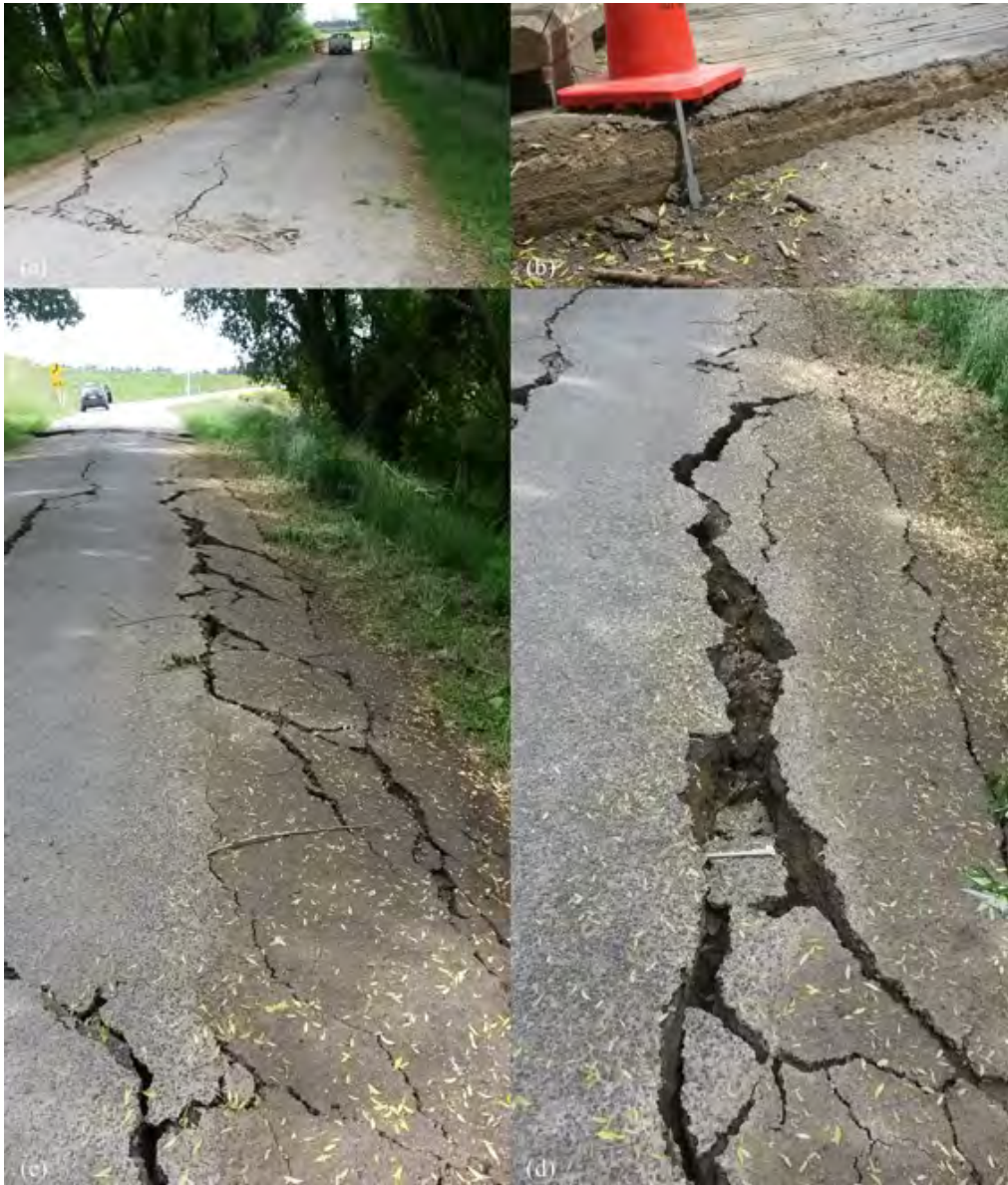
Figure 6.45: Damage at Emu Plains Bridge [-42.6394, 172.9149]: (a) Roadway damage looking west towards bridge; (b) Settlement at eastern abutment; (c) and (d) Significant cracking in roadway on eastern side of bridge (photos taken facing east away from bridge).
