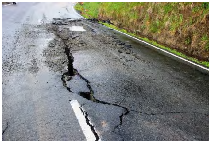
Figure 4.142: Large crack in middle of roadway on Rotherham Road. Crack width 20-30 cm. Vertical offset is approximately 4 cm (S42.6900, E173.9462, 17 Nov 2016).
