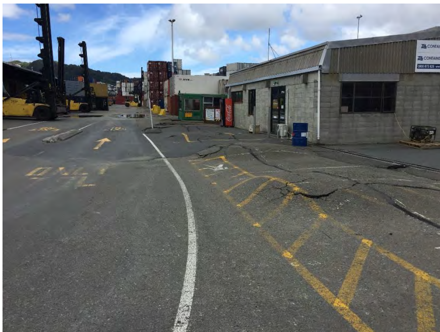
Figure 5.77: Looking south along western-most row of piles from partially demolished and buried Pipitea Wharf, which is approximately 16 m west of Building S37. Fill settled 300 mm relative to embedded piles (S41.278798°, E174.785186°, taken on 17NOV16). A cross section (LT1) is shown in Figure 5.29.
