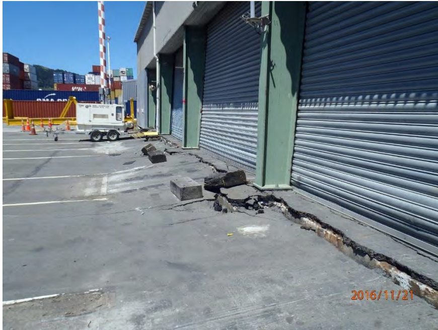
Figure 5.76: Looking south along east wall of Building S37, which shows approximately 375 mm of differential settlement between fill and pile-supported east wall of the building. (S41.279065°, E174.785787°, taken at 1220 hrs on 21NOV16)
