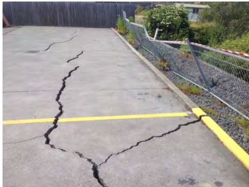
Figure 4.139: Cracks visible behind retaining wall (– date to be added in V2.0 of report, S42.3968, E173.6796, facing S).
