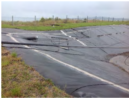
Figure 4.130: East side of KK-OPS. Note ripped geo-liner in line with crack by third post from left (– date to be added in V2.0 of report, S42.3667, E173.6875, facing SE).
