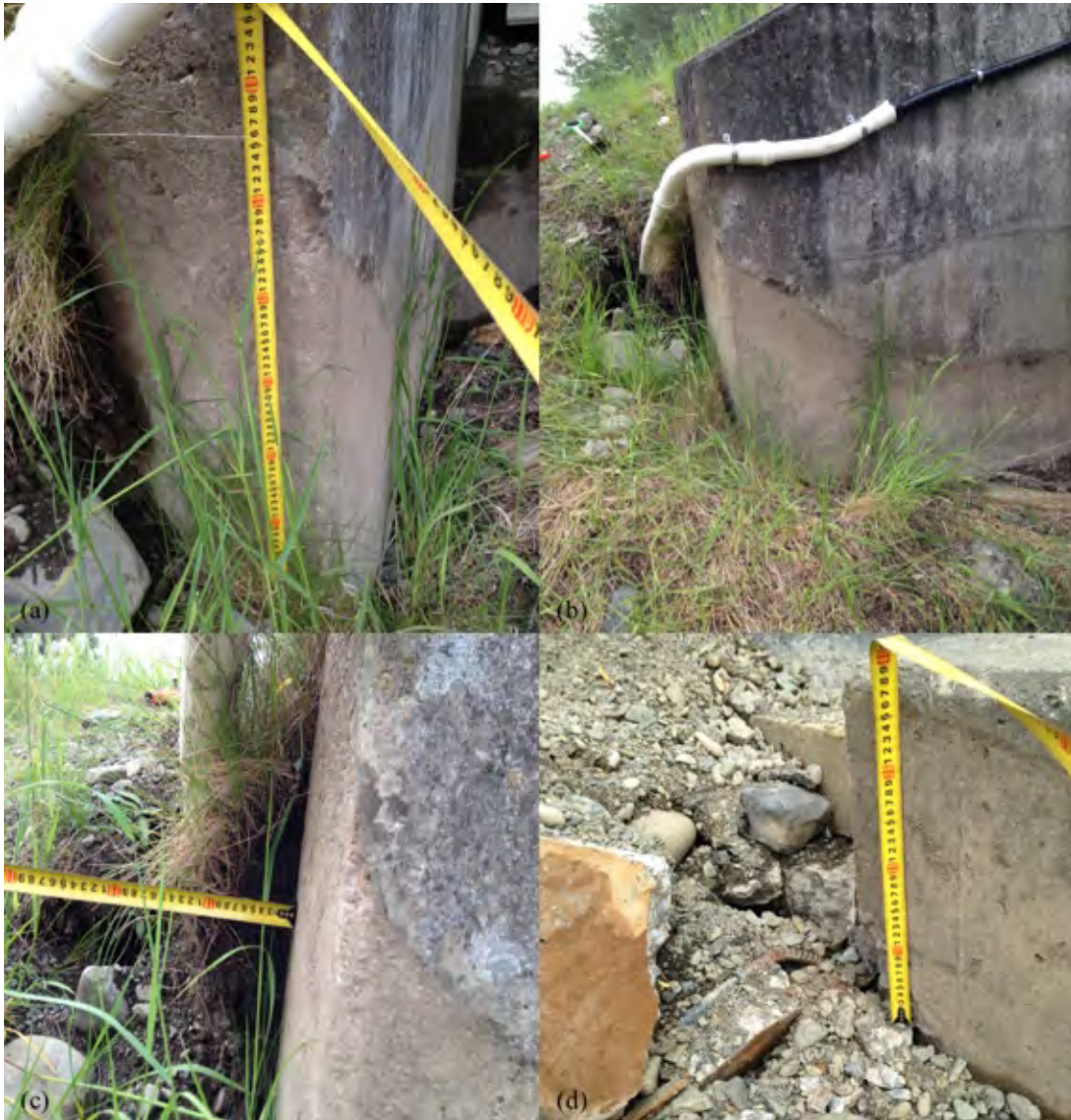
Figure 6.22: Settlement and outward movement at west side of north abutment to Lower Mason Bridge [-42.6334, 173.0666]: (a) Edge of abutment wall looking east; (b) Abutment wall looking north; (c) Edge of abutment wall looking north; (d) Embankment side of abutment wall near deck connection looking south.
