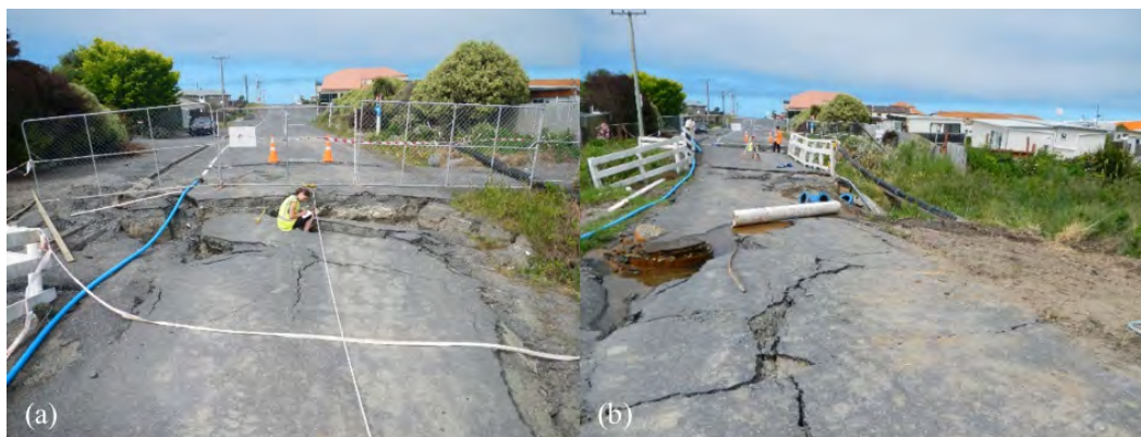
Figure 6.65: Approach cracking at Lyell Creek Bridge [-42.3892, 173.6773]: (a) Eastern approach looking east; Note: crack at 9, from the bridge abutment (location of field member) was 50 cm wide, and had a vertical offset of 30 cm. (b) Western approach looking east.
