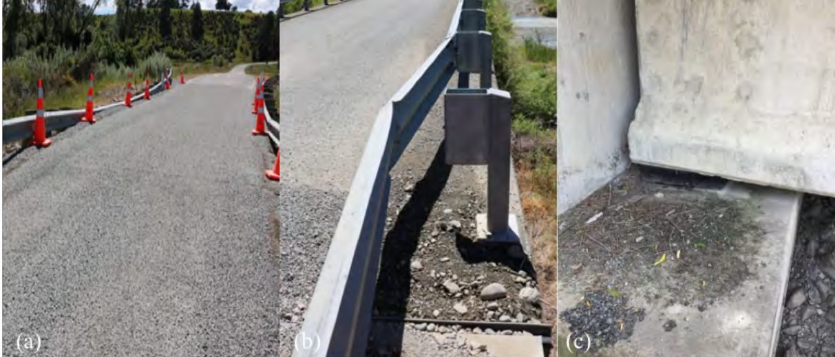
Figure 6.32: Damage at Lottery River Bridge [-42.6097, 173.0854]: (a) Gravel in-fill due to settlement and guardrail damage at northeast approach looking northeast; (b) Residual transverse offset of deck and abutment at northeast abutment looking southwest; (c) Residual displacement of bearing pad at southwest abutment looking west.
