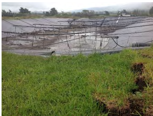
Figure 4.128: KK-OPS from eastern edge. Note geo-liner is ripped in foreground and uneven settlement on the west side is visible in the background (– date to be added in V2.0 of report, S42.3669, E173.6874, facing W).
