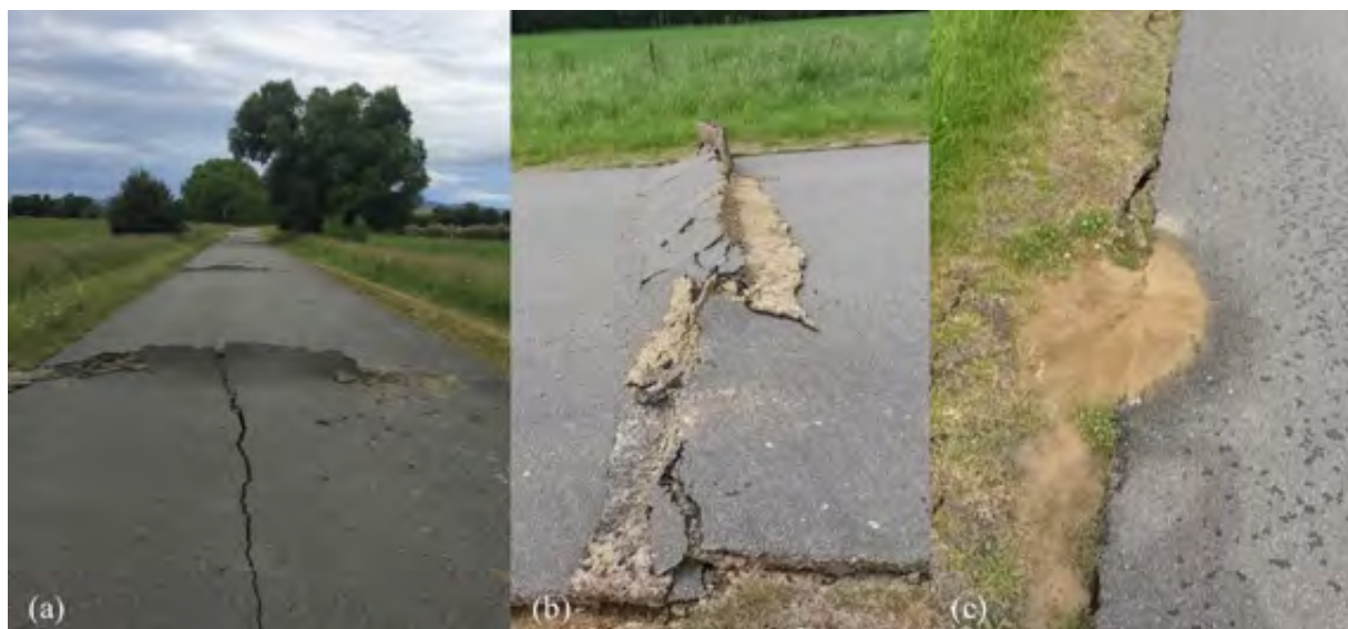
Figure 6.41: Damage observations east of Leslie Hills Road failure area [-42.6306,172.9895]: (a) Compression ridging in pavement material; (b) Side view of compression ridge; (c) Minor liquefaction ejecta.
