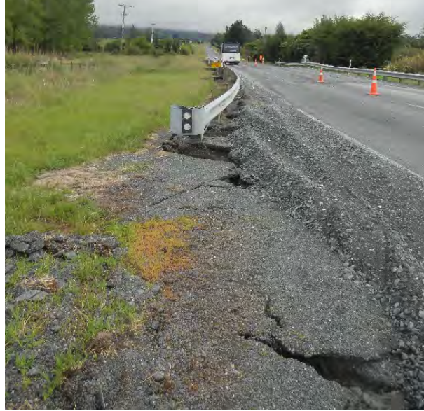
Figure 6.79: Cracking on the south side of the Waimagarara culvert on Athelney Road (9 Dec 2016, facing north) [-42.3606, 173.6765].
