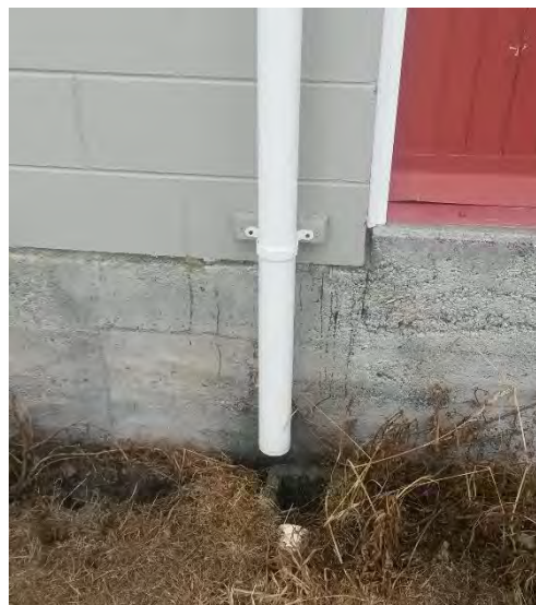
Figure 4.101: Misalignment of drain pipe and drain on east side of house on Schoolhouse Road (-9 Dec 2016, S42.3683, E173.6501).
