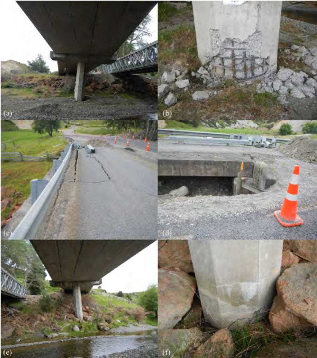
Figure 6.30: Structural damage to Wandle Bridge [-42.5864, 173.1003]: (a) South approach from under bridge; (b) Plastic hinging on pier near south approach; (c) Deck at southern end; (d) South abutment; (e) North approach from under bridge; (f) Minor hinging on pier near north abutment.
