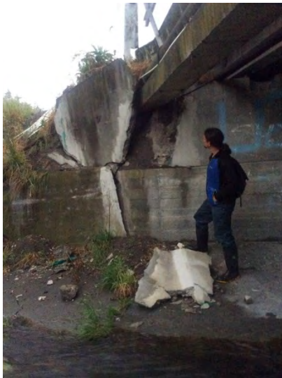
Figure 6.74: Damage to the south abutment on the east side of the bridge (8 Dec 2016, facing south) [-42.3692, 173.6547].
