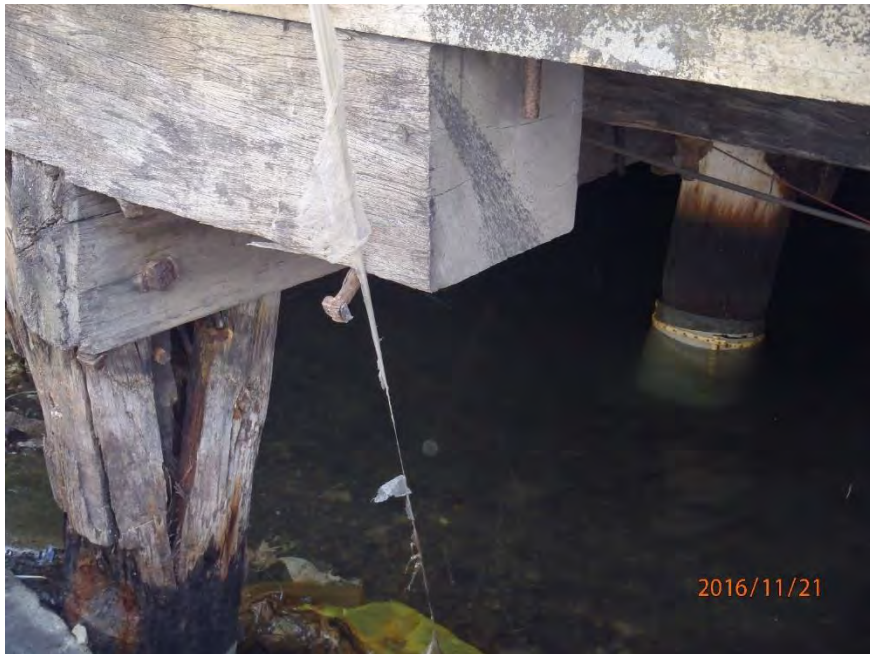
Figure 5.43: Looking under King's Wharf at an inland bulkhead pile. Timber pile is split from lateral movement (seaward/westward) of the deck relative to the pile. (S41.280900° E174.784375°, taken at 1412 hrs on 21NOV16)
