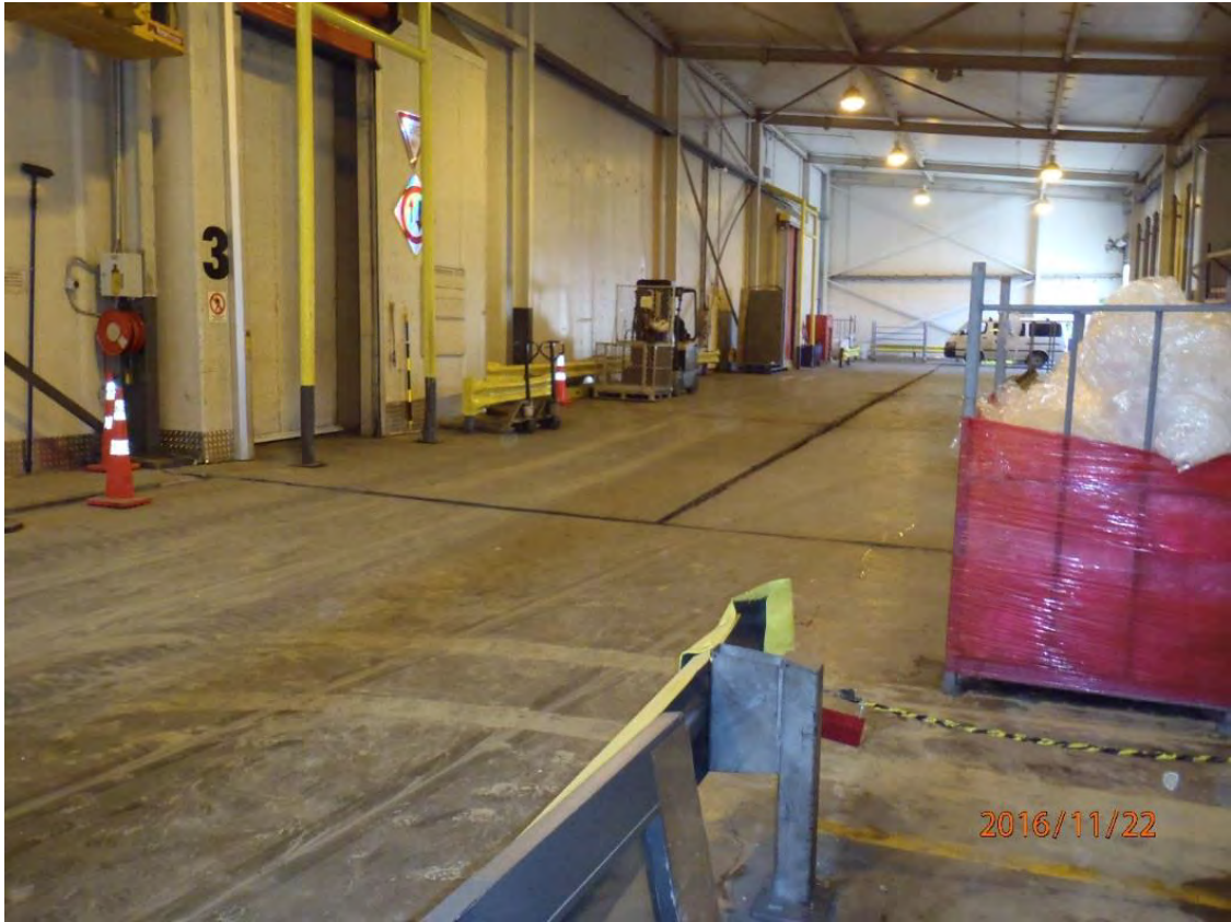
Figure 5.63: Contraction joint separation of ground floor slab inside the Shed of CS building looking south. As shown in photo, joint separations occurred in two orthogonal directions. (S41.281255° E174.784797°, taken at 1520 hrs on 22NOV16)
