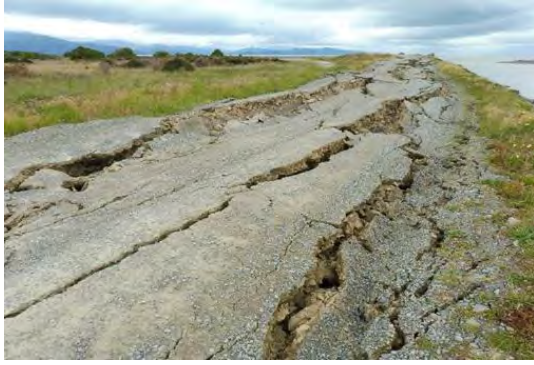
Figure 4.62: Severe cracking of levee (17 Nov 2016, S41.50122, E174.060071, facing E).
