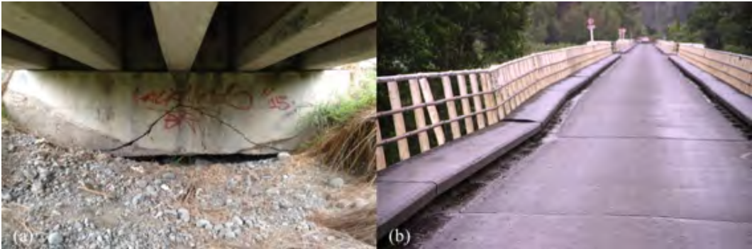
Figure 6.7: Structural damage at western approach area to Waiau River Bridge [-42.6556, 173.0302]: (a) Severe cracking in the abutment wall (looking west from under the bridge deck); (b) Differential settlement at second pier (looking east).
