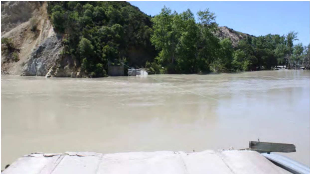
Figure 6.87: Collapse of Clarence Valley Road Bridge [-42.11066, 173.84156]. Photo taken from western side looking east (stuff.co.nz, 2016).
