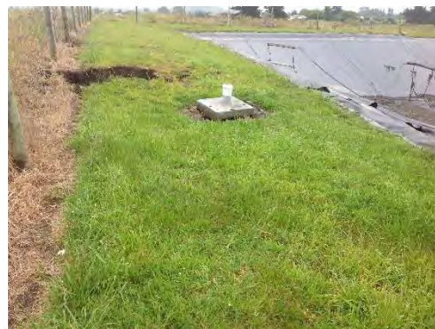
Figure 4.131: Protruding vent pipe on east edge of KK-OPS due to ground settlement (– date to be added in V2.0 of report, S42.3668, E173.6875, facing S).
