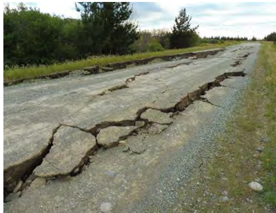
Figure 4.32: Lateral spreading induced cracking along top of northern stopbank (17 Nov 2016, S41.4387, E174.0214, facing E).
