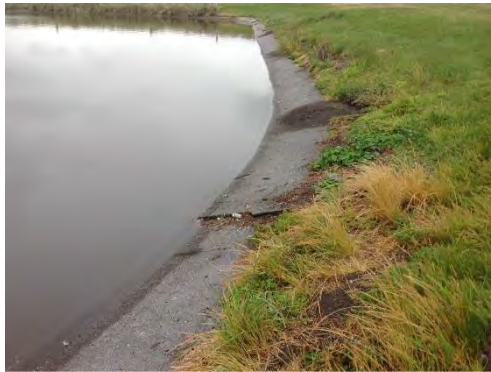
Figure 4.133: North edge of KK-OPN. Note cracking and overlayering of concrete. Ejecta visible on concrete. (– date to be added in V2.0 of report, S42.3647, E173.6884, facing W).
