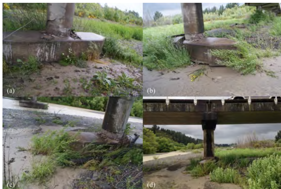
Figure 6.18: Ejecta near bridge piers and footings at Mason Bridge [-42.647, 173.043]: (a) Looking east; (b) Looking north; (c) Looking west; (d) Looking north.
