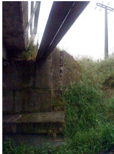
Figure 6.75: Damage to the north abutment on the east side of the bridge (8 Dec 2016, facing north) [-42.3692, 173.6549].
