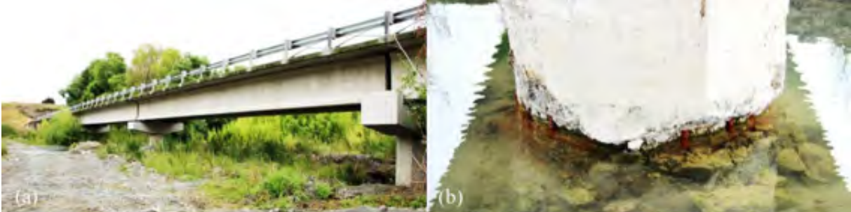
Figure 6.31: Lottery River Bridge [-42.6097, 173.0854]: (a) General layout; (b) Plastic hinge damage at base of pier.
