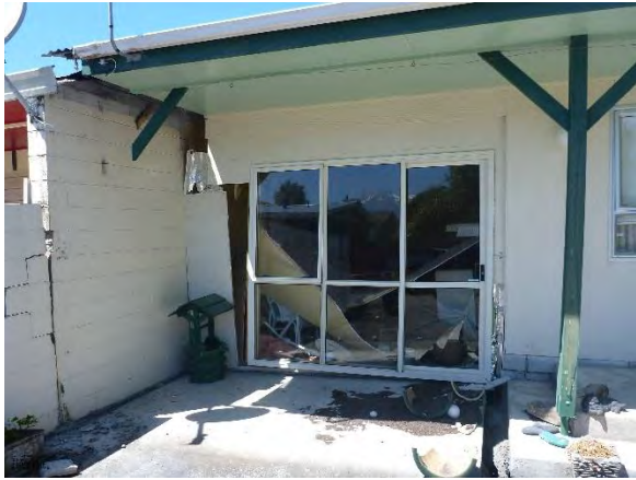
Figure 4.116: Cracks running through the house closer to Lyell Creek (– date to be added in V2.0 of report, S42.3857, E173.6783).
