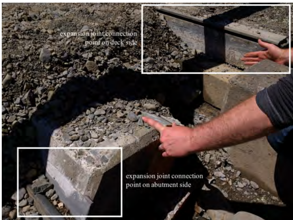
Figure 6.24: Damage to abutment-deck connection at Lower Mason Bridge due to relative movement of abutment wall and deck. The breakaway member to the left was pushed back away from the deck and rotated 180° such that the connection point for the expansion joint faces away from the deck [-42.6334, 173.0666].
