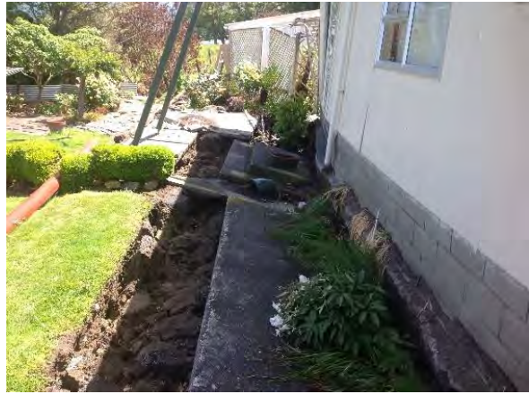
Figure 4.117: Gapping at the west side of the house closer to Lyell Creek (date to be added in V2.0 of report, S42.3857, E173.6783).
