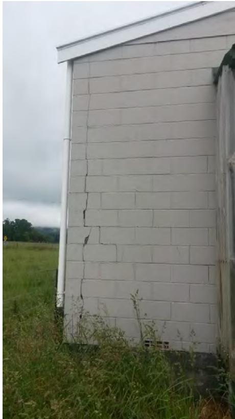
Figure 4.102: Cracking through brick work on SW corner of house on Schoolhouse Road (–9 Dec 2016, S42.3684, E173.6501, facing W).
