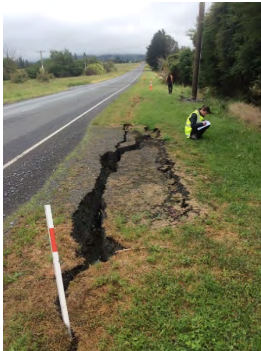
Figure 6.77: Lateral spreading cracks at the side of Athelney Road (9 Dec 2016, facing north) [-42.3598, 173.6765]. Note the drainage ditch to the right of the photo.
