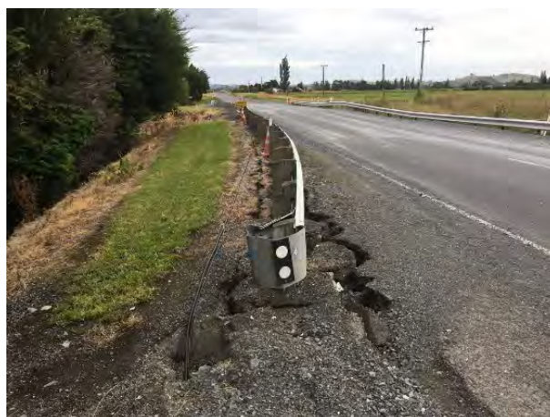
Figure 6.78: Cracking on the north-side of the Waimagarara culvert on Athelney Road (9 Dec 2016, facing south) [-42.3599, 173.6765].
