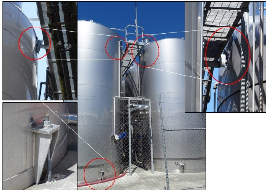
Figure 18. Damage to the walking platforms atop of tanks and anchoring connections due to tank movement (photos and annotations: Dmytro Dizhur).
