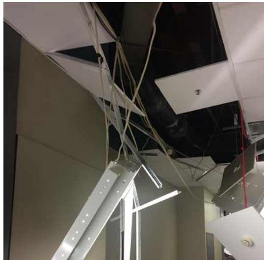
Figure 20. Typical ceiling damage observed in commercial buildings (photo: Helen Ferner).
