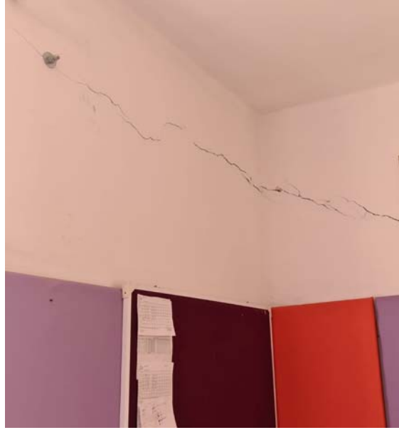
Figure 7.25. Interior wall damages in the school building
