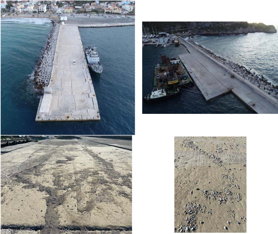
Figure 5.48. (top left) east quay wall of Karlovasi port, (top right) west quay wall of Karlovasi port, (bottom left) ejecta on the west quay wall, presumably product of liquefaction occurrence, and (bottom right) a detailed view of the ejecta, brownish to grey color, mostly sandy and silty with some gravels (aerial photographs courtesy of I.N. Spyrou and Prof. K. Ziotopoulou – to not be reproduced without permission from Prof. Ziotopoulou ).
