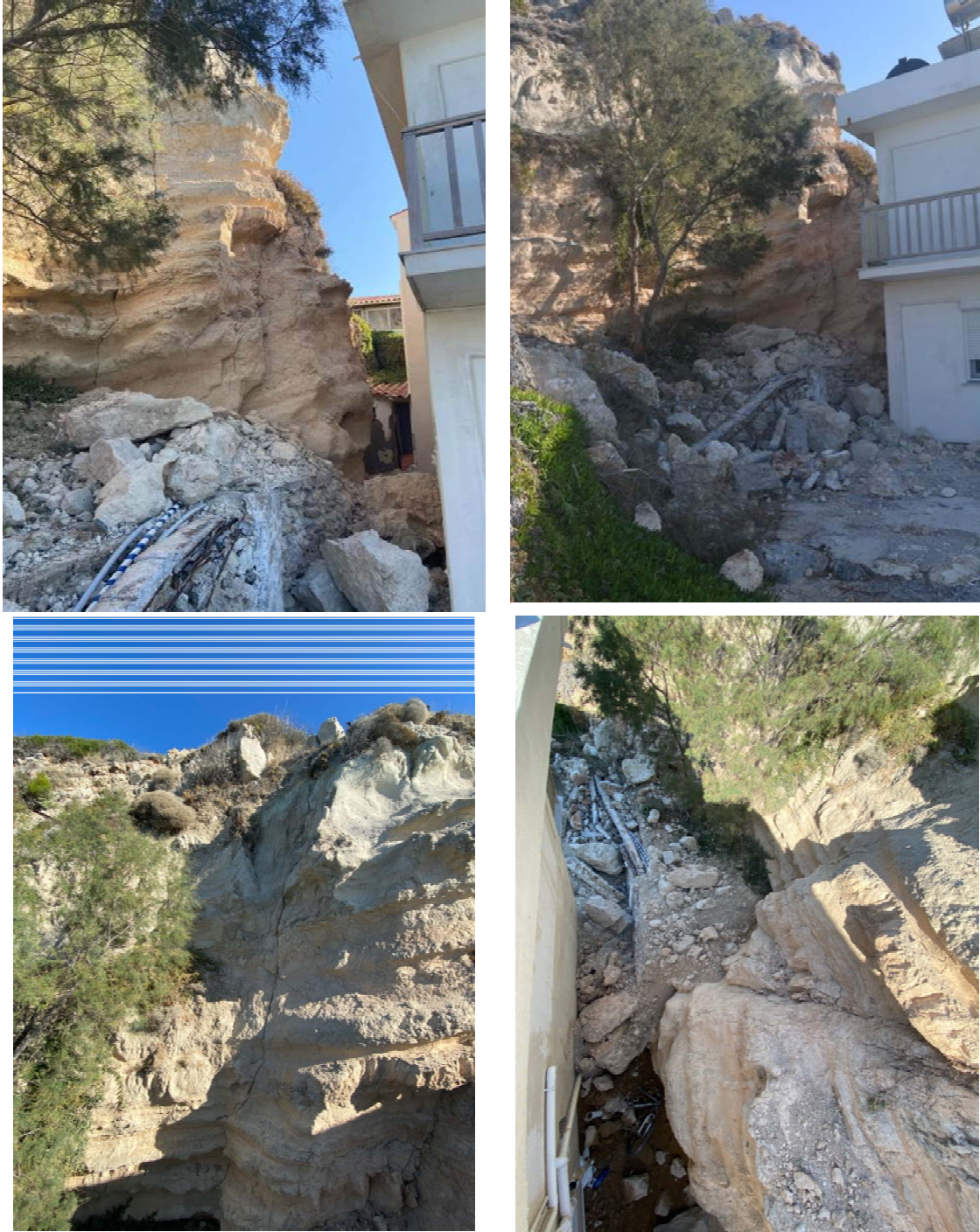
Figure 5.26. Detachment of sandy marls and marly limestones recorded very close to a residential building in the Kokkari region (photos taken by the HAEE reconnaissance team, 37°46'49.9"N, 26°53'35.0"E). Vertical open cracks are visible, clearly susceptible to detachment and overturning.
