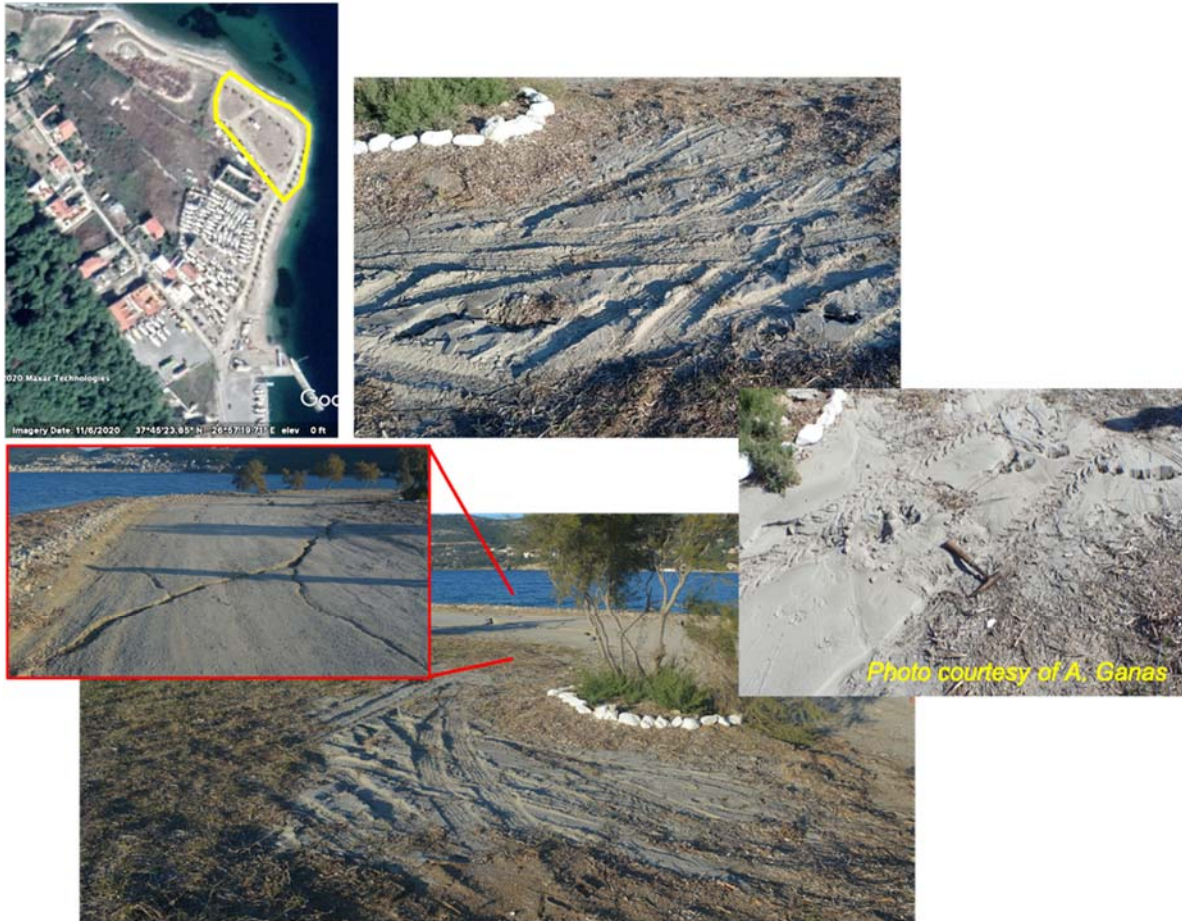
Figure 5.14. Surface manifestations of earthquake-induced soil liquefaction in the form of sand boils in Malagari (location: 37°45'24.6"N 26°57'28.8"E) [photos taken by the HAAE reconnaissance team and Dr. A. Ganas from NOA]
