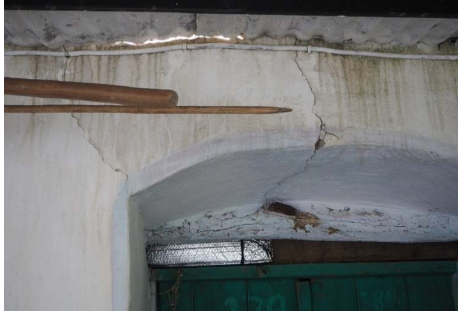
Figure 7.31. Cracking at the door opening
