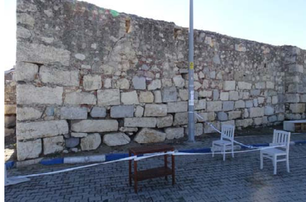
Figure 5.35. Deformed and cracked safety wall 38^{\circ}11'40.34''\text{N } 26^{\circ}47'3.22''\text{E} / 14:22 / 31.10.2020
