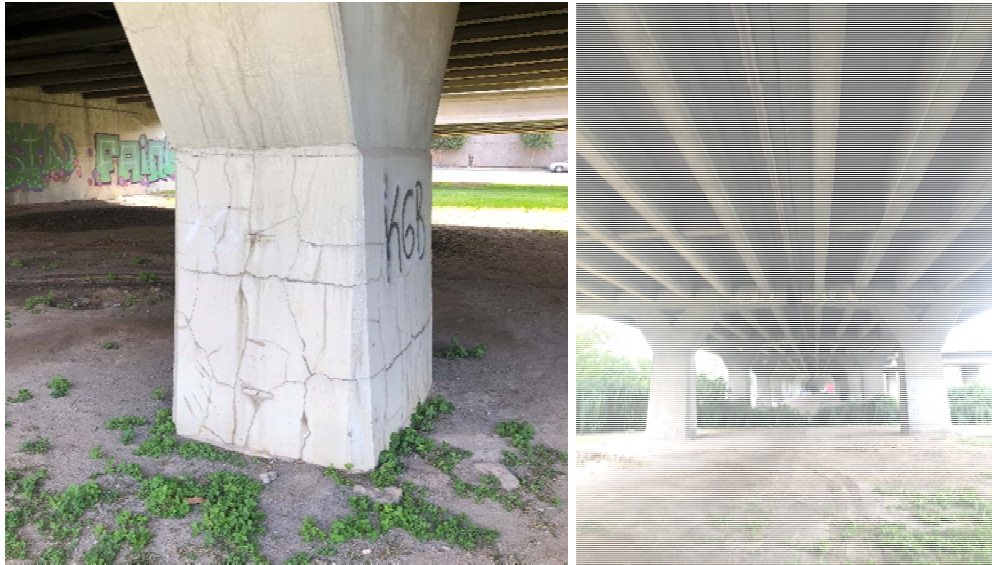
Figure 7.50. ASR based cracks (non-seismic) and general view
