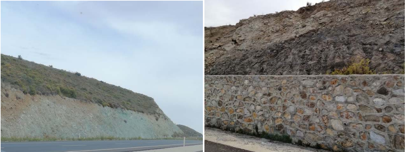
Figure 5.23. Views from a highway cuts with no signs of slope instability ( 38^{\circ}17'31.6''N 26^{\circ}40'14.6''E )
