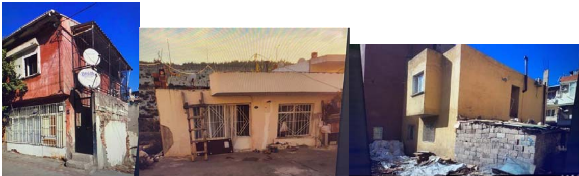
Figure 7.10. Examples of one- and two-story buildings designated as heavily damaged even though the damages due to earthquake are not severe
