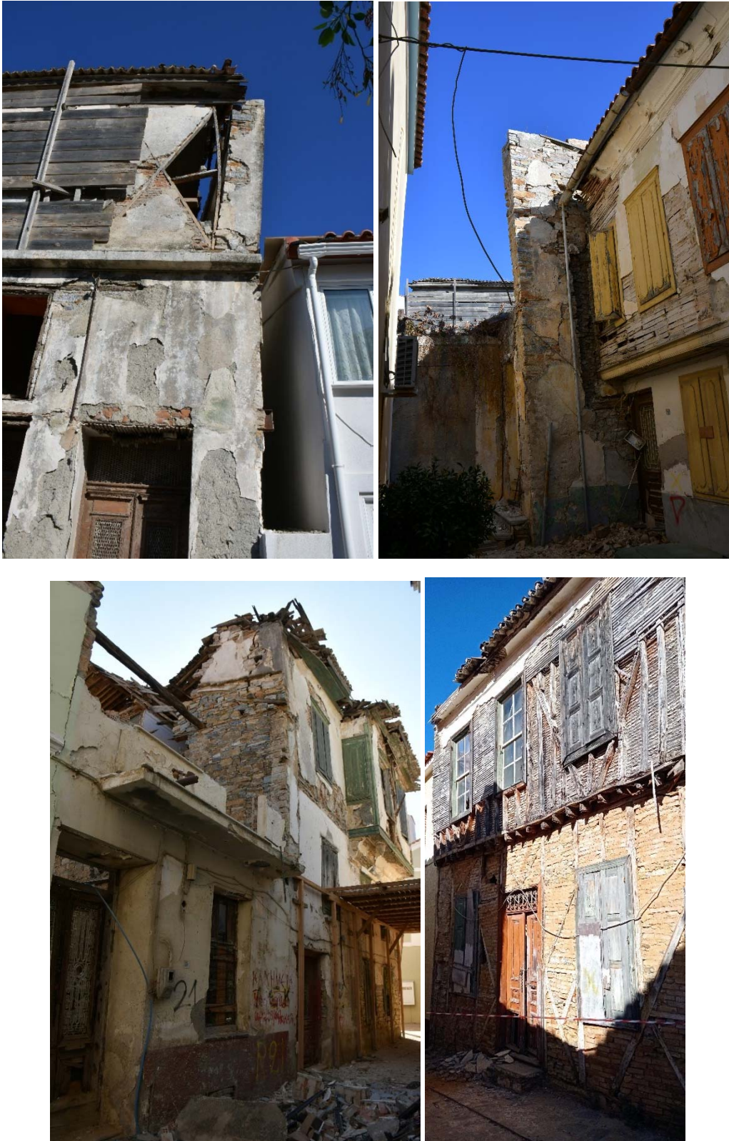
Figure 7.72. Buildings in which the ground floor is made of masonry and the upper story is made either of timber-framed masonry or timber walls.
