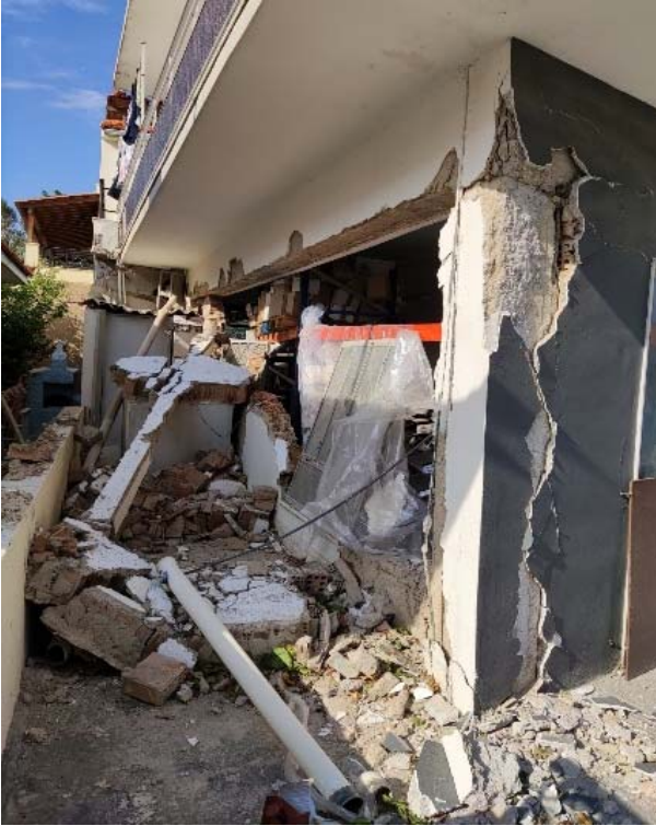
Figure 7.63. Separation and overturning of infill walls.
