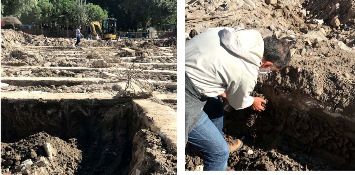
Figure 5.3. Two-way combined footing system of a heavily damaged building in Bayrakli
