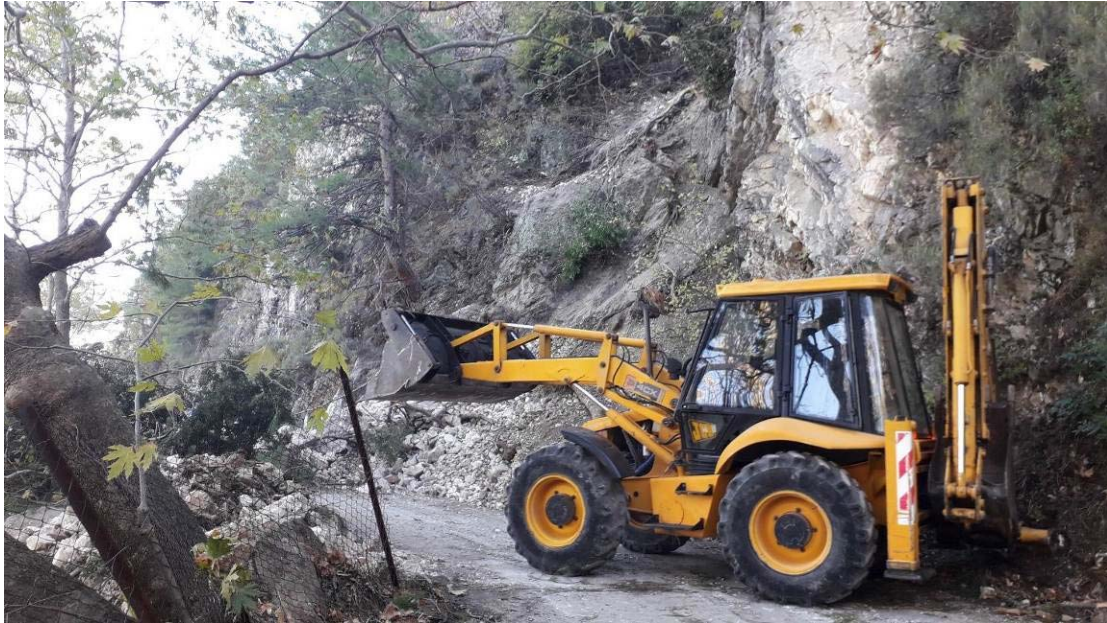
Figure 5.29. Slope failures close to the village Stavrinides (photo reported in HSGME 2020).
