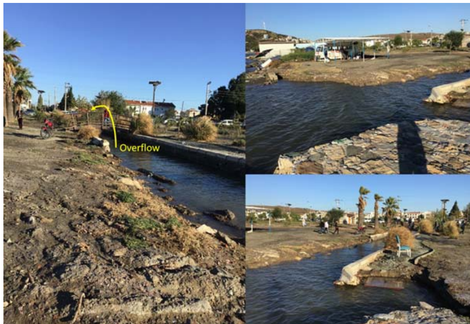
Figure 2.14. Azmak river in the East direction from Teos Marina where the tsunami overflowed the small bridge.
