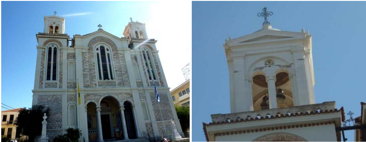
Figure 7.91. Shear failure at the bell tower of the Agios Spyridon Cathedral at Bathi.
