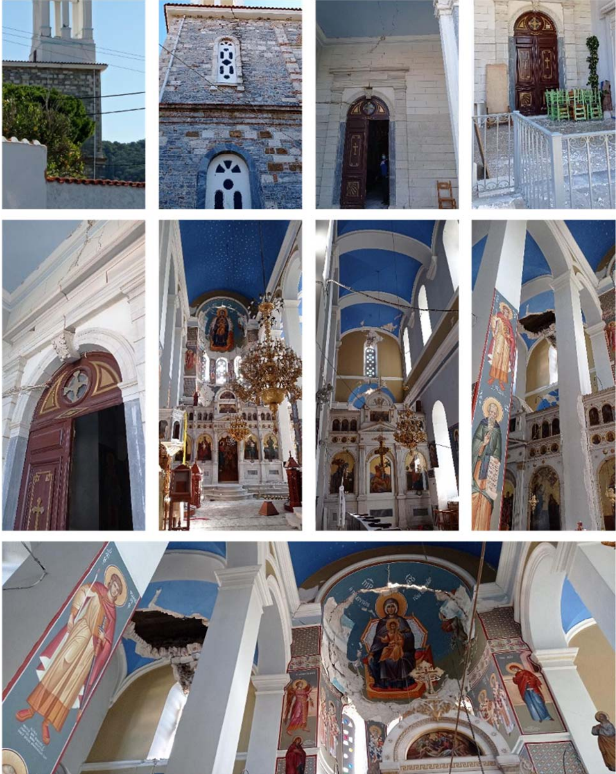
Figure 7.89. Extensive failures at the Church of Agios Nikolaos in Kokkari, the largest Church of Samos. Failure in arches, in the keystone of the two main entrances, cracks and complete failures in domes as well as damages in the bell tower.
