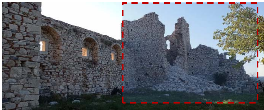
Figure 7.95. Partial collapse of the perimeter walls of the Castle of Lykourgos Logothetis.
