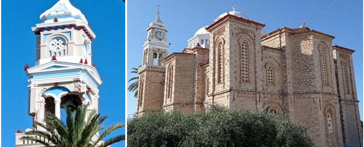
Figure 7.86. Cathedral of the Assumption of the Virgin Mary in Karlovasi. Heavy damage observed in both bell towers which were not built at the same time as the main part of the temple but were added afterwards.
