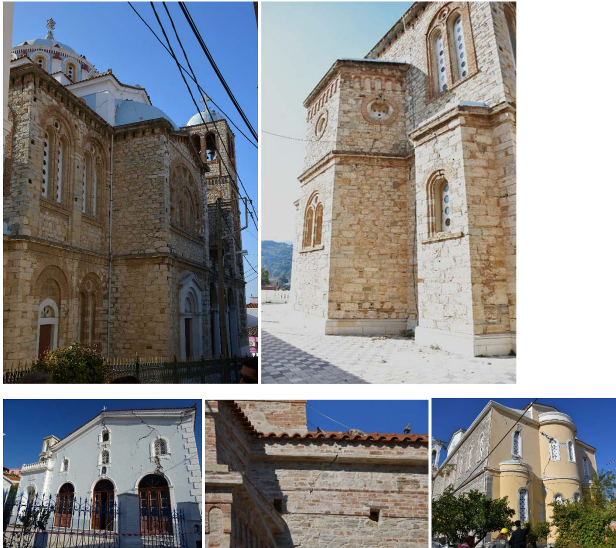
Figure 7.82. Perimeter walls of churches and damage observed.
