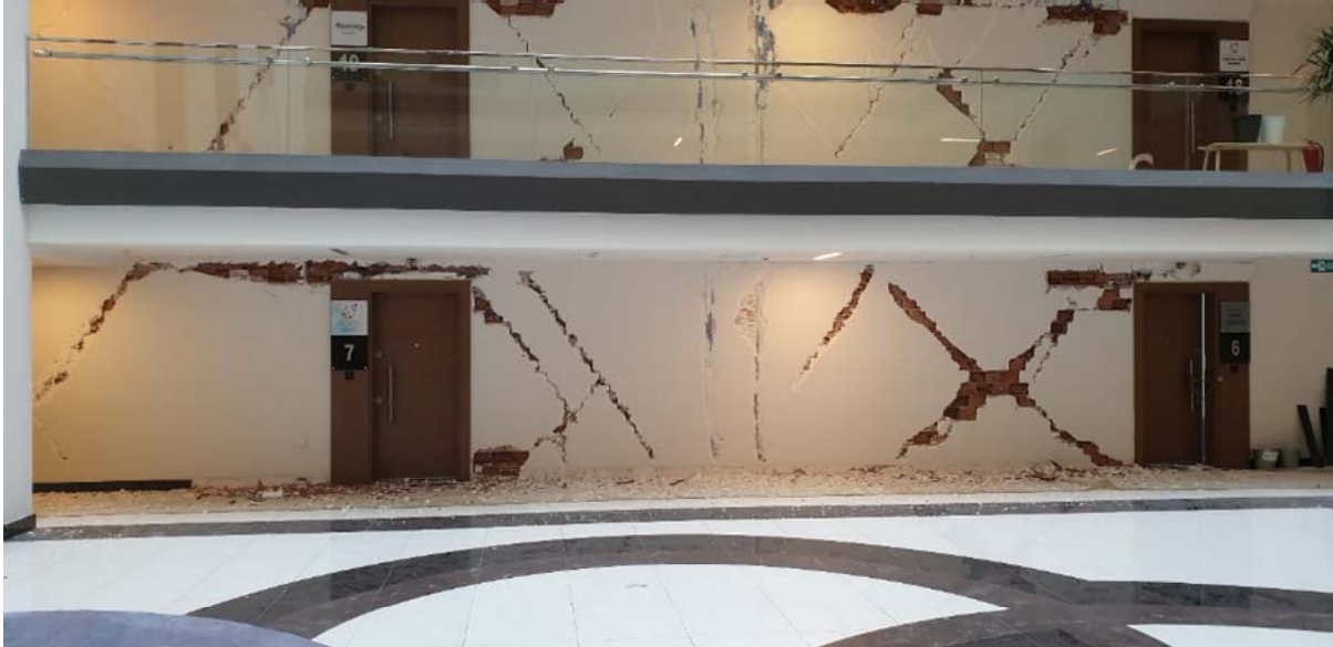
Figure 7.17. Non-structural damage due to large openings in slabs
