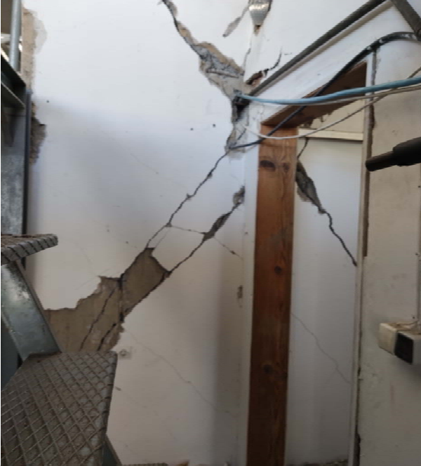
Figure 7.61. Shear failure of a shear wall in a soft story.
