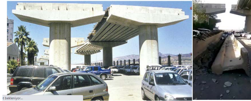
Figure 7.52. An incomplete bridge construction 20 years ago without providing a lateral girder stability at the site (10 years ago and now)
