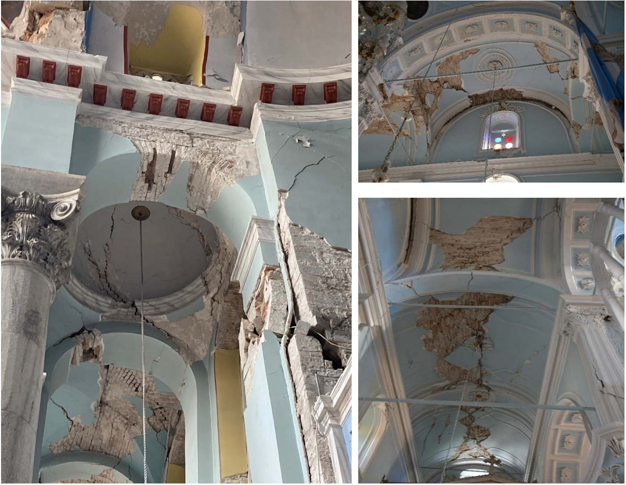
Figure 7.84. Severe damage of dome-and-arches roofs
