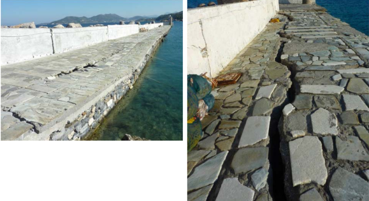
Figure 5.49. (left) clear trends of differential subsidence of the quay wall of Kokkari port with wide open cracks alongside and transversely, (right) close view of an open crack of 10 to 15cm alongside the sea front (HAEE reconnaissance report, 2020).
