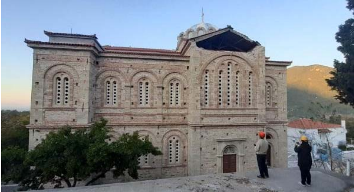
Figure 7.90. Out-of-plane failure of the gable below the roof of the Church of Genesis of Virgin Mary at Konteika, which dates back to the 19 th century.
