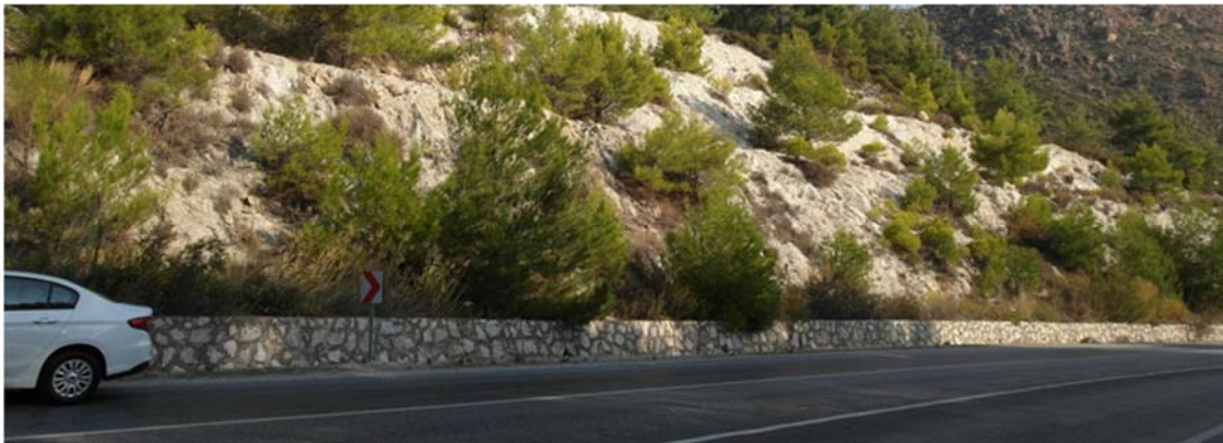
Figure 5.36. Short, stoned retaining walls on the toe of the highway cuts between Menderes and Gumuldur in the south of İzmir city center.
