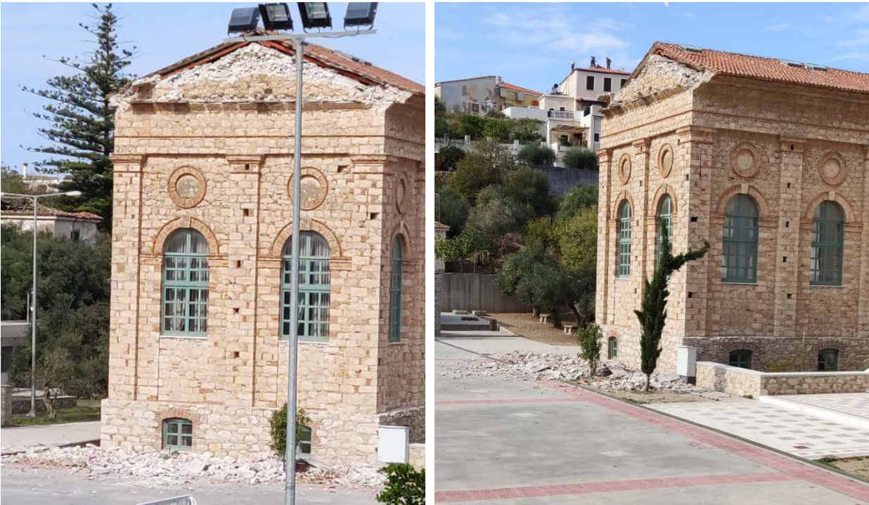
Figure 7.78. Primary school at Karlovassi (Porphyrriad School): damage to the triangular metope and the perimeter eaves, damage to the roof, and cracks inside the building.
