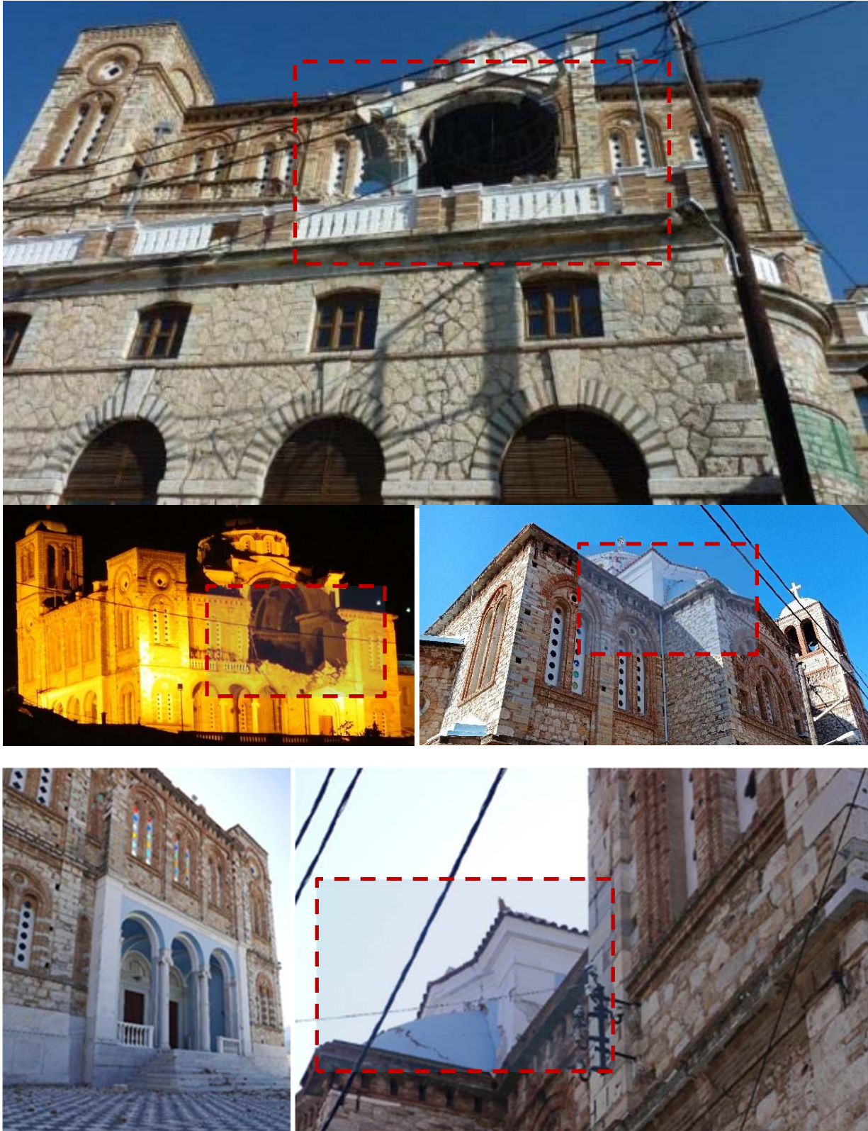
Figure 7.88. Out-of-plane failure of the south lateral wall which supports the dome of the Cathedral of the Assumption of Virgin Mary in Karlovasi. In this particular temple there was a collapse of the roof on the west side of the Temple.
