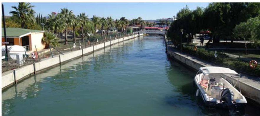
Figure 5.38. Sidewalls of the river canal in the Sığacık Marina (Photo: Courtesy of Gurel Özdemir). (38°11'33.86"N 26°47'4.07"E 14:16 / 31.10.2020)
