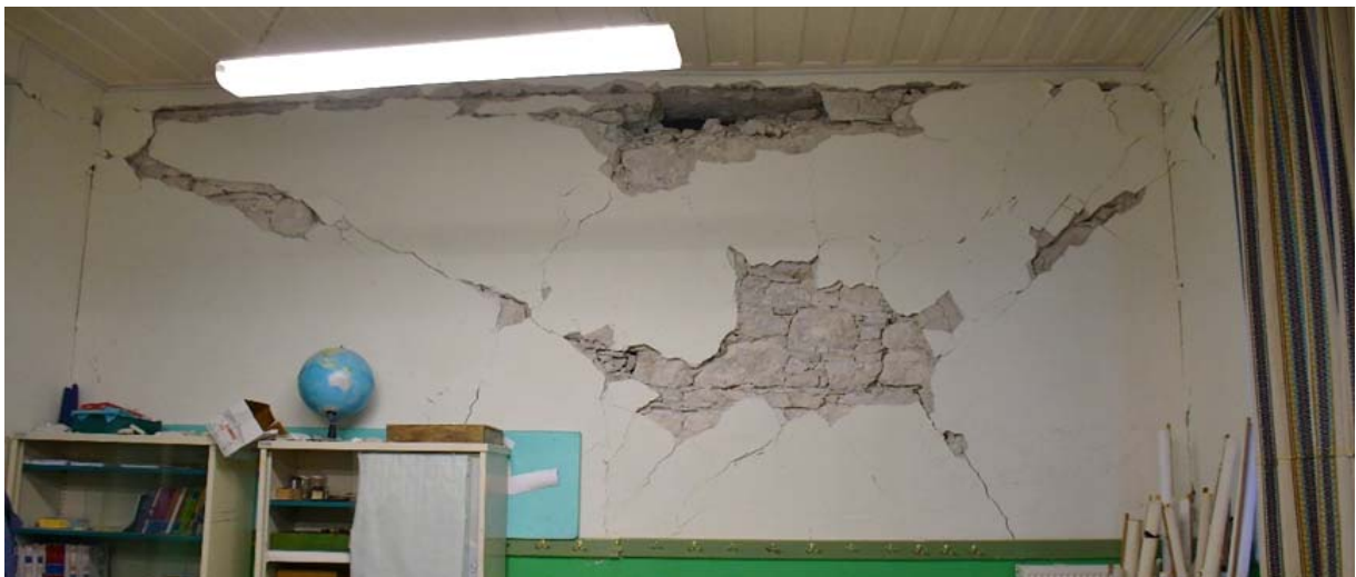
Figure 7.76. Primary school at Chora: Shear failure of masonry wall.
