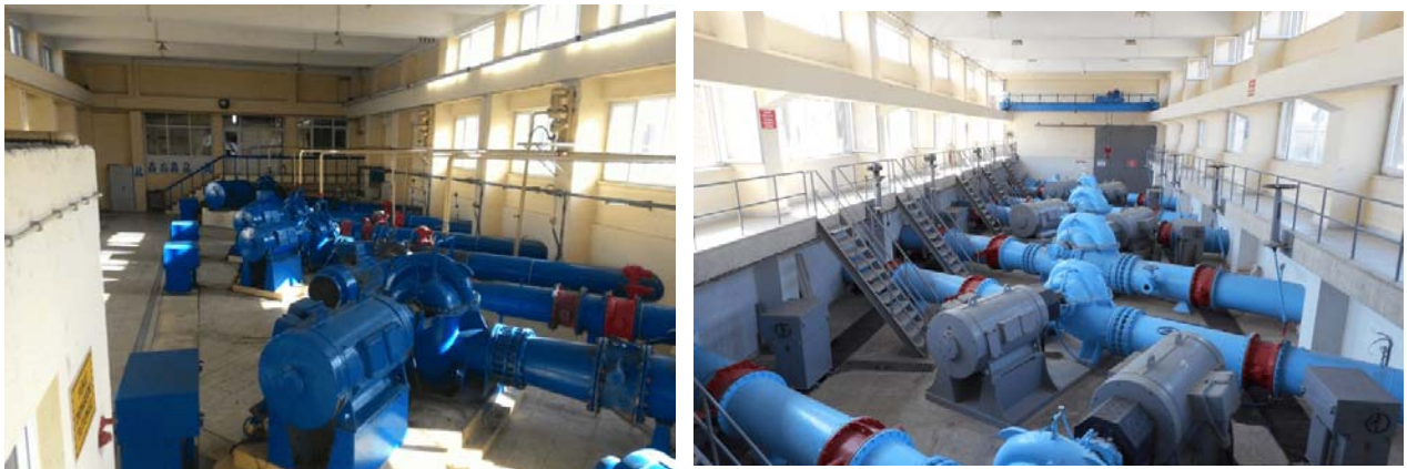
Figure 6.15. The Goksu (left) and Yahselli (right) pump stations in İzmir (Izsu, 2020)
