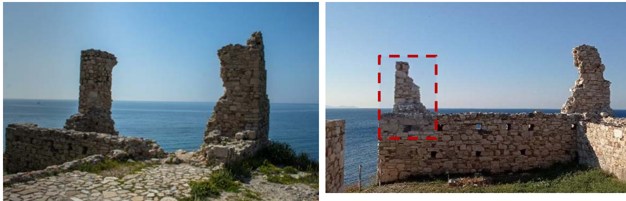
Figure 7.94. The Castle of Lykourgos Logothetis (a) before the earthquake 4 , (b) after the earthquake of the October 30th 2020, showing the partial collapse of the perimeter walls into the sea.
