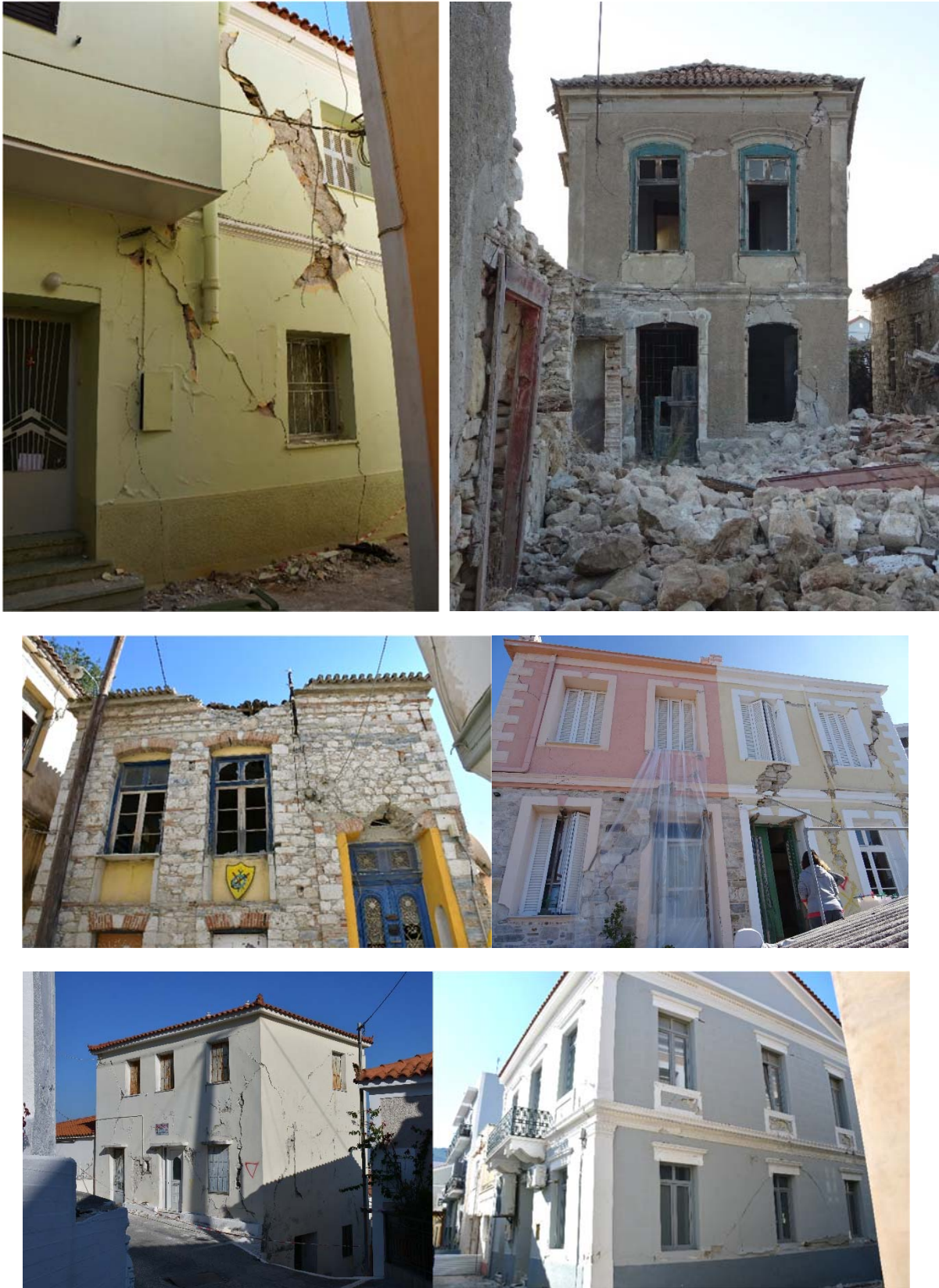
Figure 7.69. In-plane shear damage to walls and lintels.
