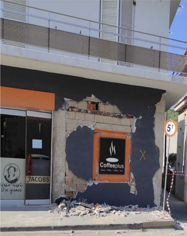
Figure 7.64. Cracking of infill walls due to out-of-plane bending.
