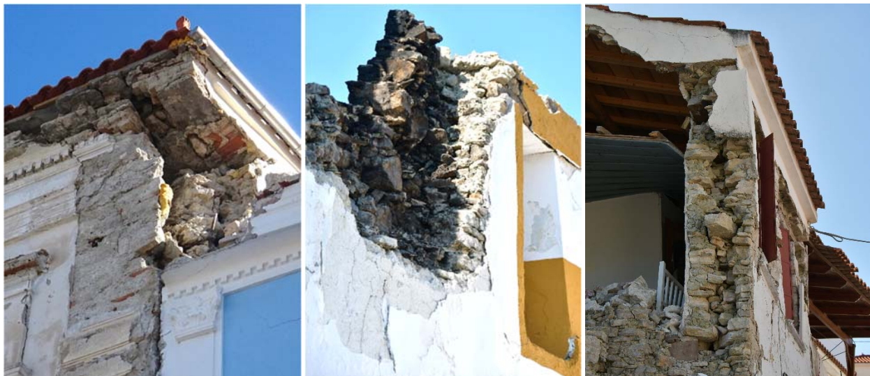
Figure 7.65. Poor-quality, three-leaf stone masonry building.
