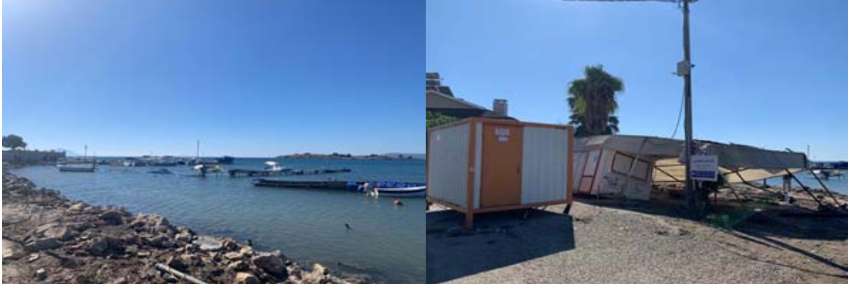
Figure 2.33. Observed damage in the floating piers used for berthing and mooring and the seafront harbor facilities in Akarca fishery shelter.
