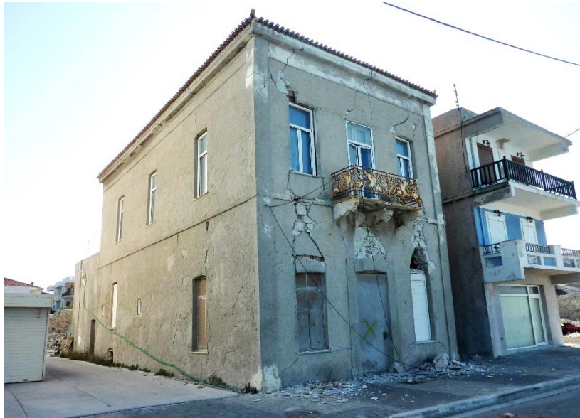
Figure 7.73. Masonry building with extensive damage adjacent to a concrete building with no damage.
