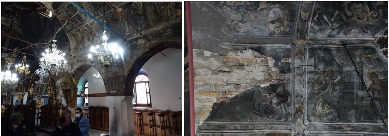
Figure 7.85. Steel ties were installed to alleviate the effect of the thrust of dome-and-arches roofs.
