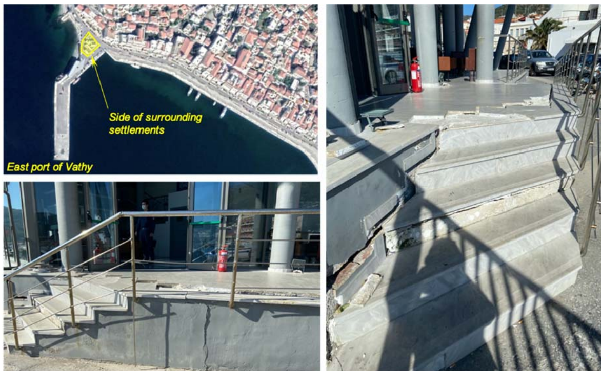
Figure 5.5. Damage observed around the Port authority building in Vathy, Samos (location: 37°45'27.0"N 26°58'15.4"E). The cracks indicate soil settlement/distortion around the building which remained intact and functioning 8 days after the earthquake (8th November 2020) [photos taken by the HAEE reconnaissance team]
