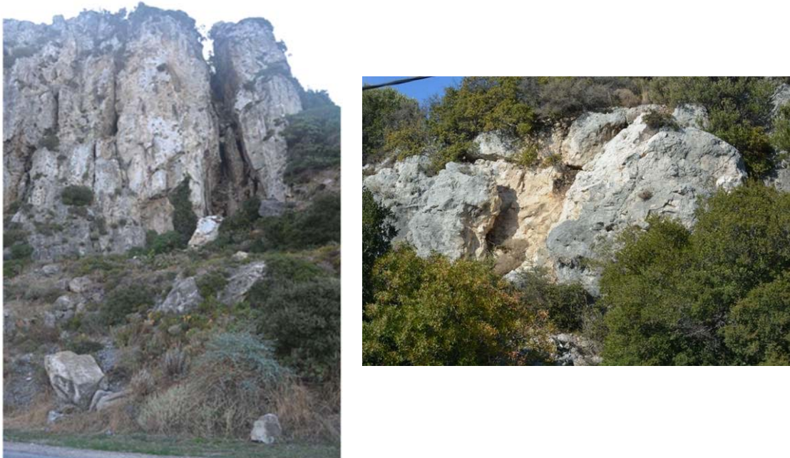
Figure 5.27. Left: Rockfalls recorded at the road network close to the village Potami ( 37^{\circ}47'17.6''\text{N} , 26^{\circ}40'00.5''\text{E} ), Right: Detachment of limestone segments close to the village Koumeika (photos taken by the HAAE reconnaissance team, 37^{\circ}42'33.7''\text{N} , 26^{\circ}44'52.9''\text{E} ).
