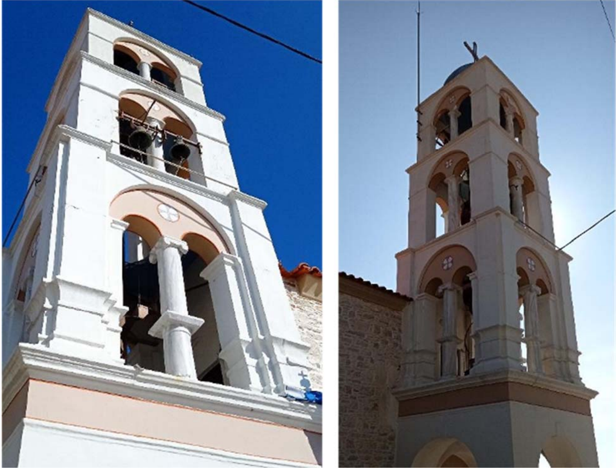
Figure 7.92. Shear failure at the bell tower of the Agia Paraskevi Church at Chora.
