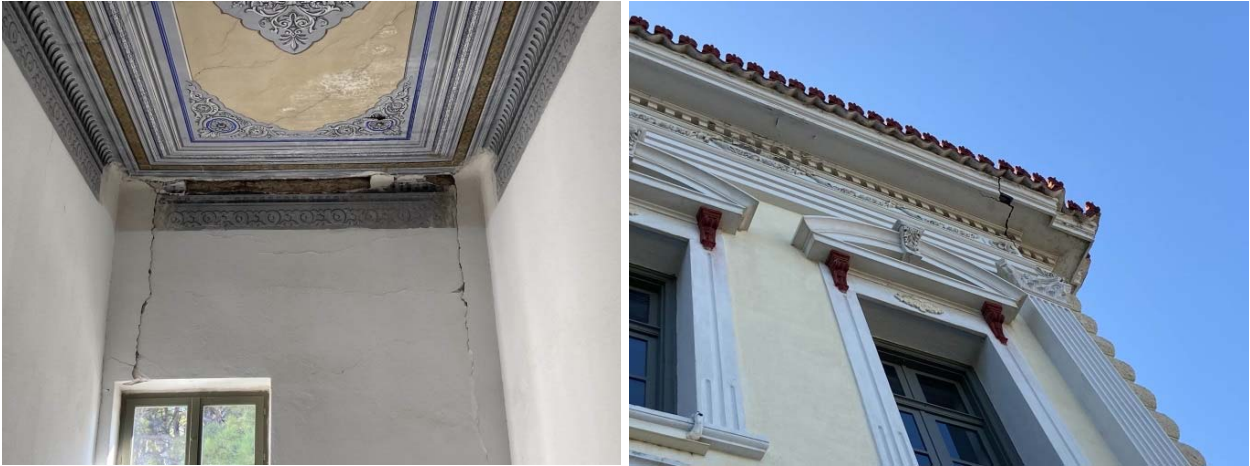
Figure 7.79. Out-of-plane masonry wall failure and corner detachment at the Lyberi building of the University of Aegean (School of Sciences).
