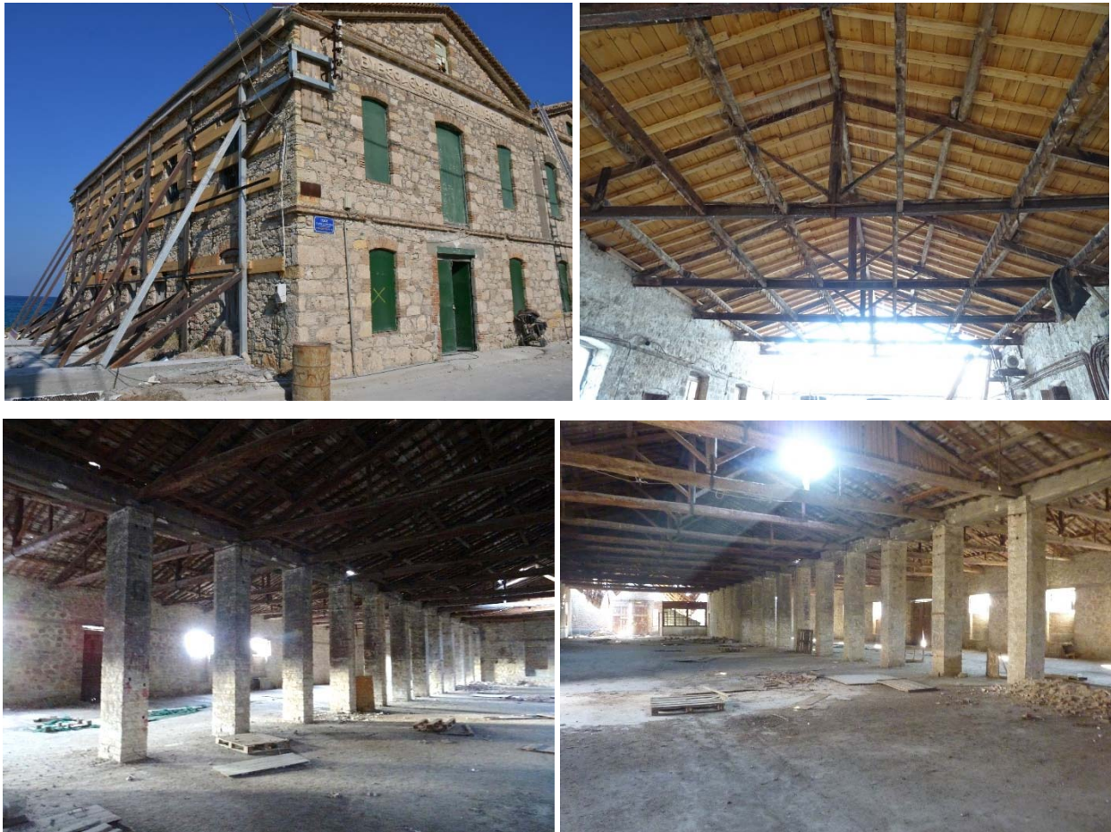
Figure 7.80. Typical tannery buildings at Karlovassi. Temporary out-of-plane support (top left).
