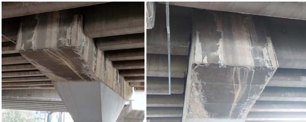
Figure 7.51. A typical before-and-after earthquake photo (December 2019 and November 2020)
