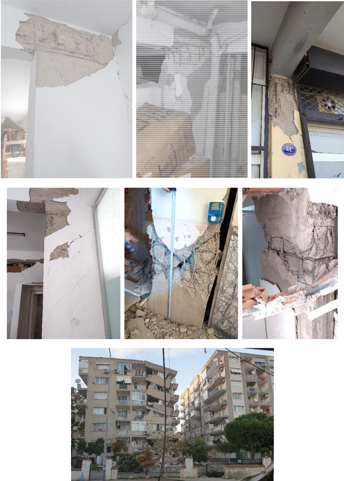
Figure 7.15. Severe column damages
