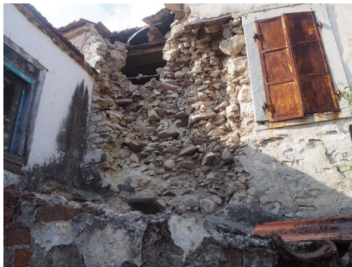
Figure 7.28. Collapsed portion of a wall
