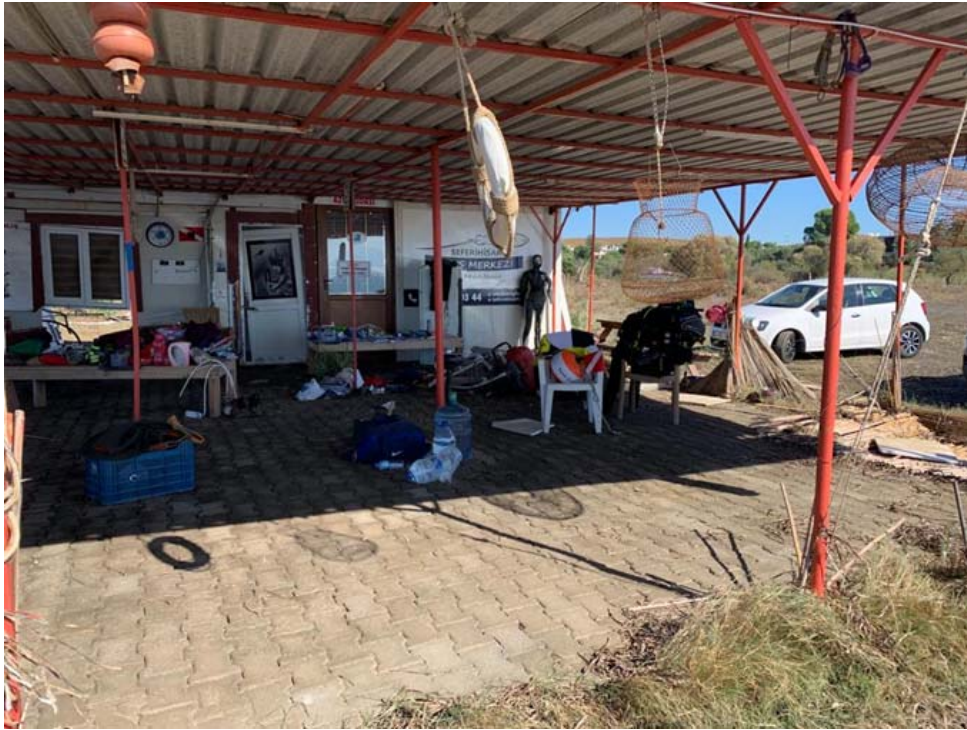
Figure 2.18. Tsunami damage on Seferihisar Diving Center (38.165683N 26.813717E).
