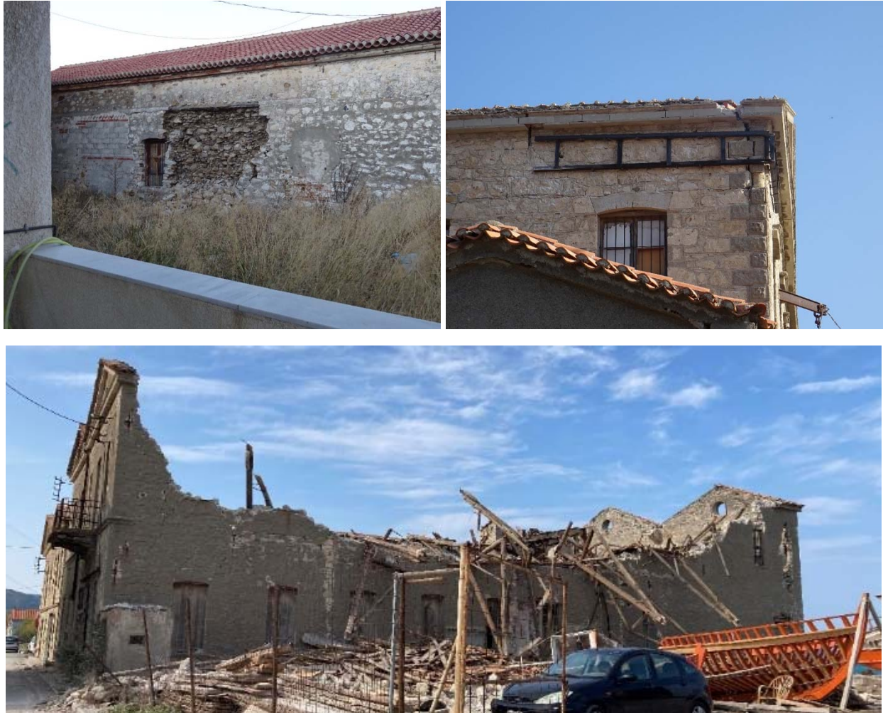
Figure 7.81. Typical damage in tannery buildings at Karlovassi.
