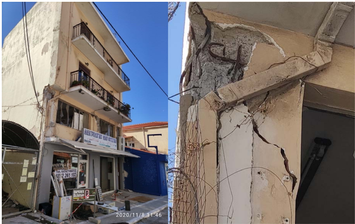
Figure 7.60. Short column (top) and beam-column joint failure of a 4-story building.
