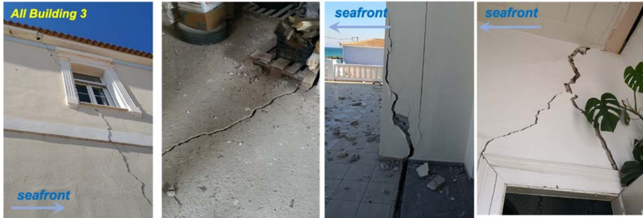
Figure 5.21. Building affected by lateral spreading towards the seafront in the neighborhood of Vyrsopepsia in Karlovasi ( 37^{\circ}48'01.1''\text{N} 26^{\circ}42'20.6''\text{E} ). The cracks observed running across the building indicate 3-5cm of movement. [Photos courtesy of Prof. K. Antonopoulos]
