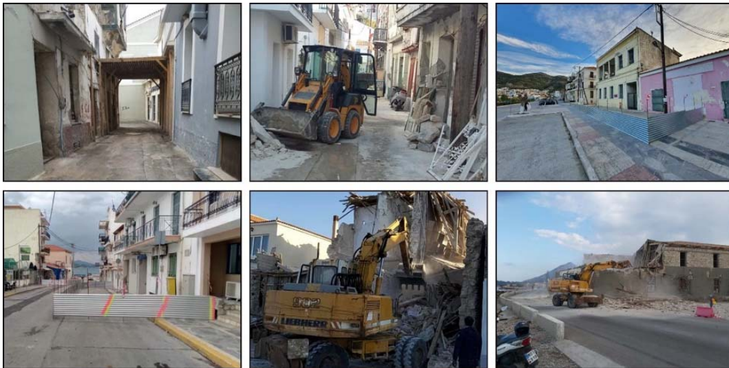
Figure 8.11. Actions for the mitigation of hazards the affected population and workers will likely encounter in the aftermath of the earthquake in Samos. Supporting of buildings, removing debris from roads and pavements, placement of markings and protective barriers to severely affected buildings in order to avoid approaching, demolition of unstable buildings dangerous for cars and passersby.
