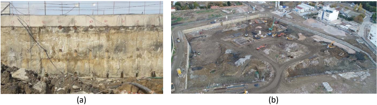
Figure 5.31. a) A picture taken earlier from the shored deep excavation located in the “new downtown” district (37°53'50.4"N 27°22'06.2"E, b) Plan view of the site
