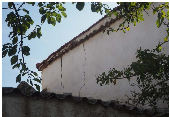
Figure 7.30. Cracking in the body of a wall
