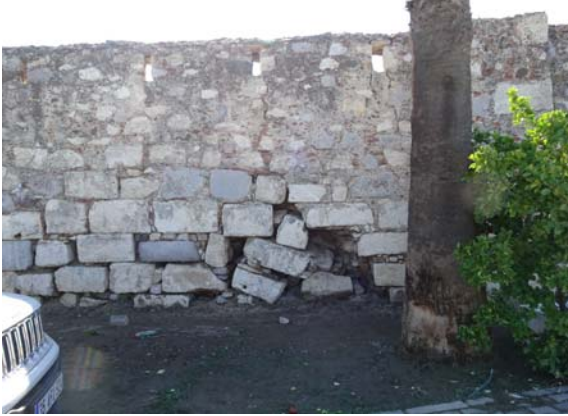
Figure 5.34. Deformed and cracked safety wall 38^{\circ}11'40.93''\text{N } 26^{\circ}47'3.47''\text{E} / 14:16 / 31.10.2020
