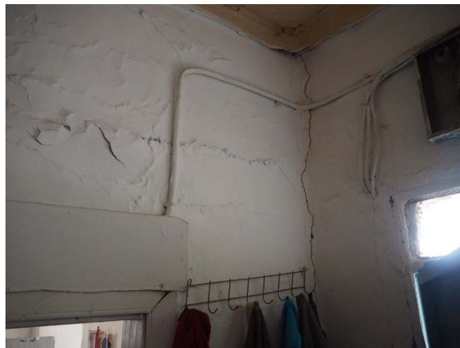
Figure 7.29. Separation at a wall-to-wall connection
