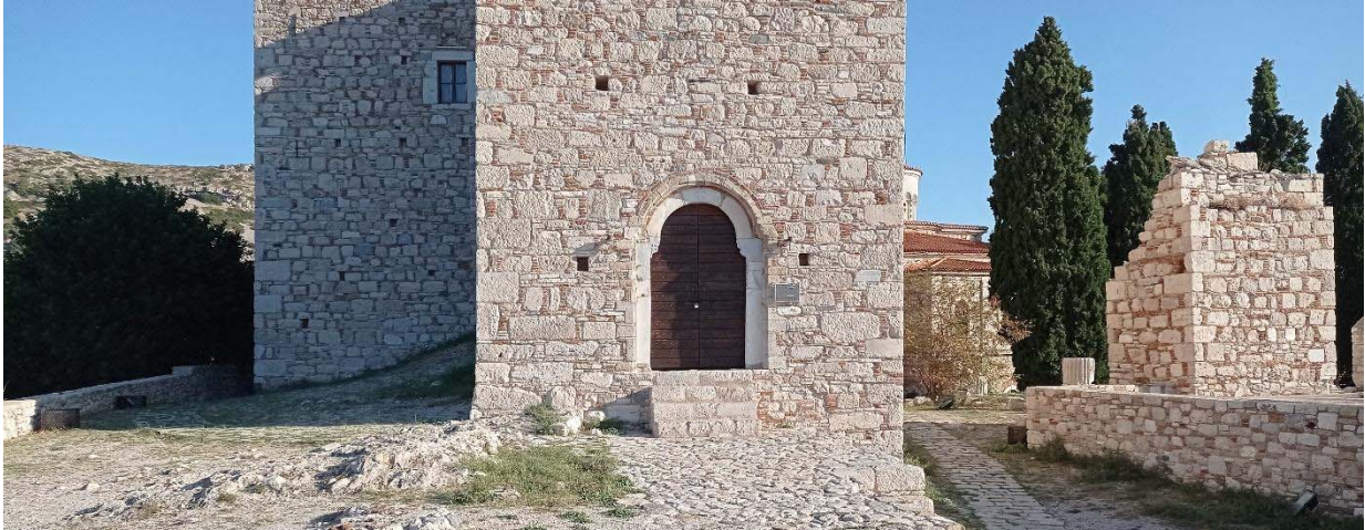
Figure 7.97. The Castle of Lykourgos Logothetis. No damage was observed; the seismic behavior of the structure was very good due to fact that it has been recently seismically rehabilitated.
