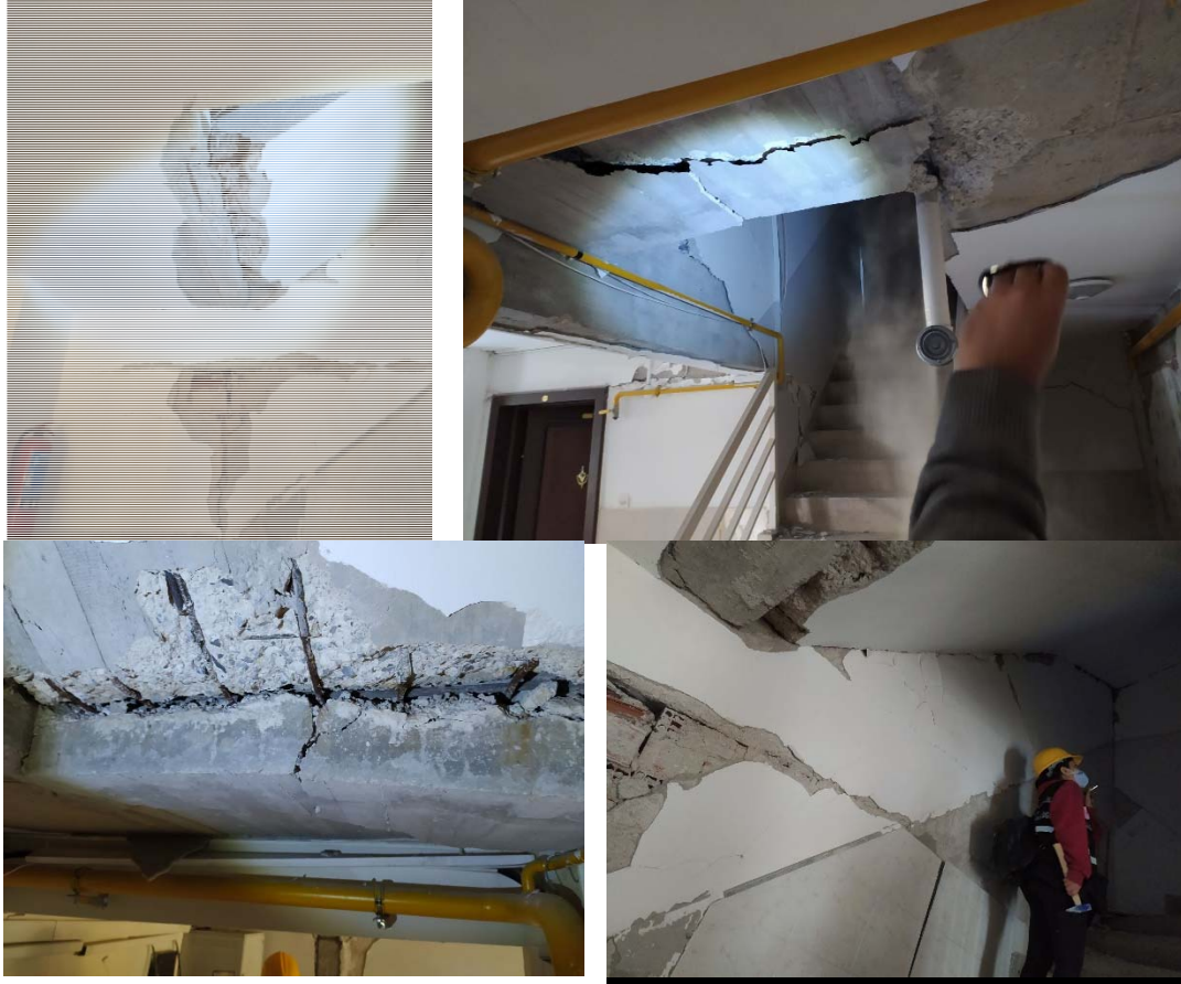
Figure 7.18. Observed staircase damages
