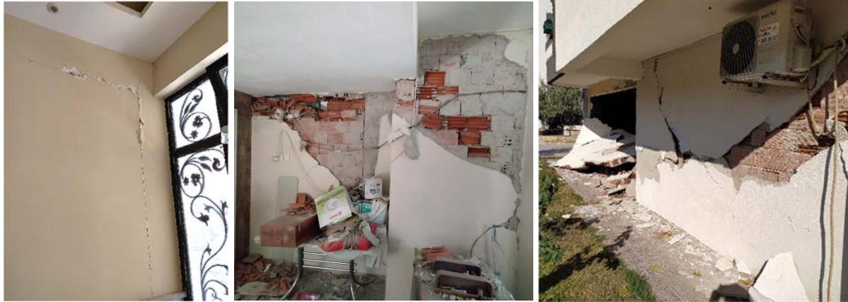
Figure 7.12. Infill wall damages
