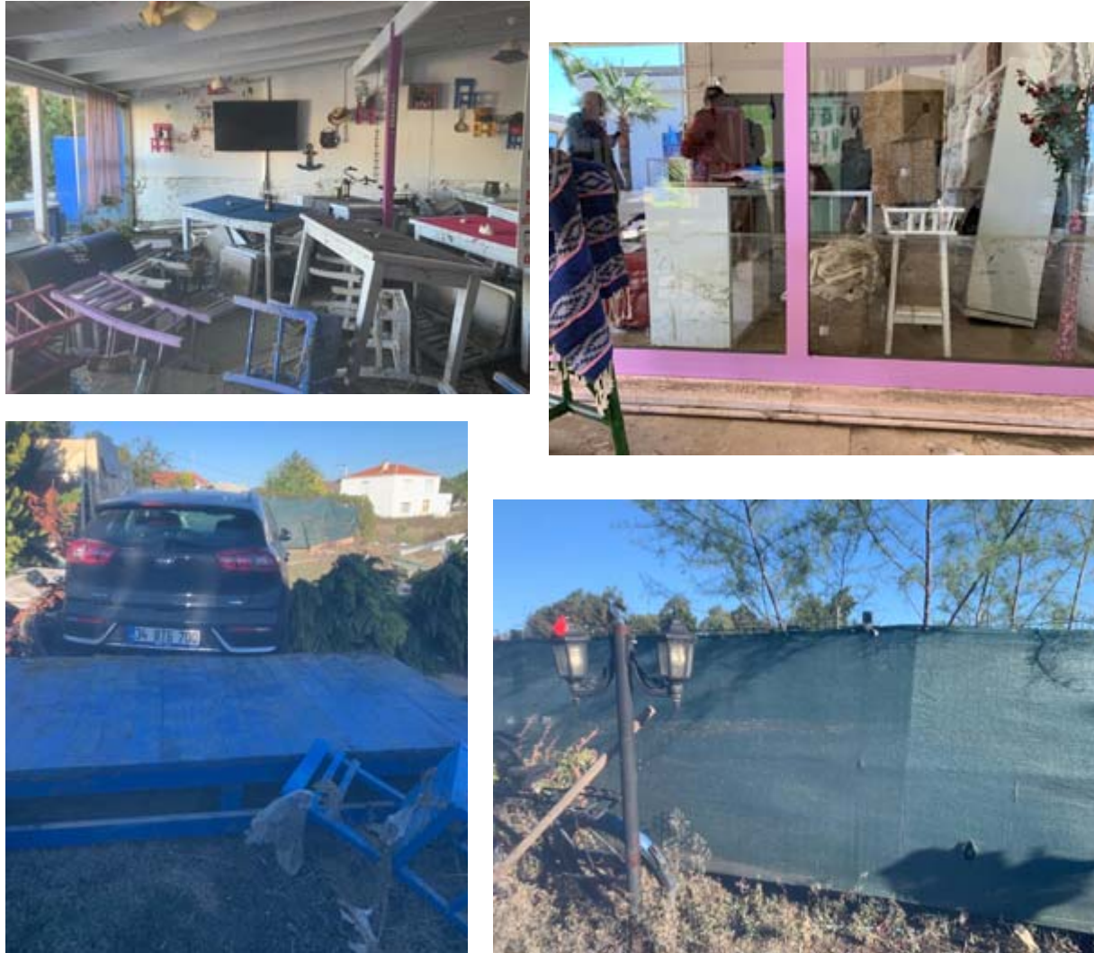
Figure 2.15. Damage on properties and tsunami traces in cafes and shops in Sigacik.
