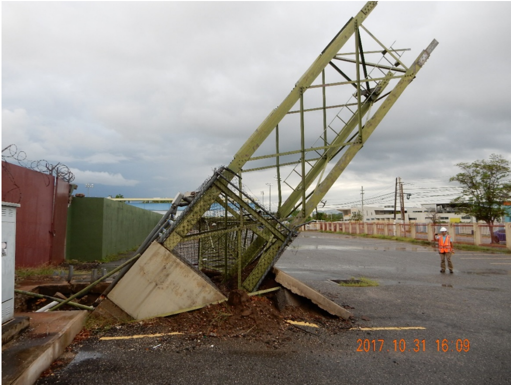
Figure E-4: Photo of foundation failure of illumination tower at Site F4 (Lat: +18.00207, Lon: -66.63098; 2017.10.31).
