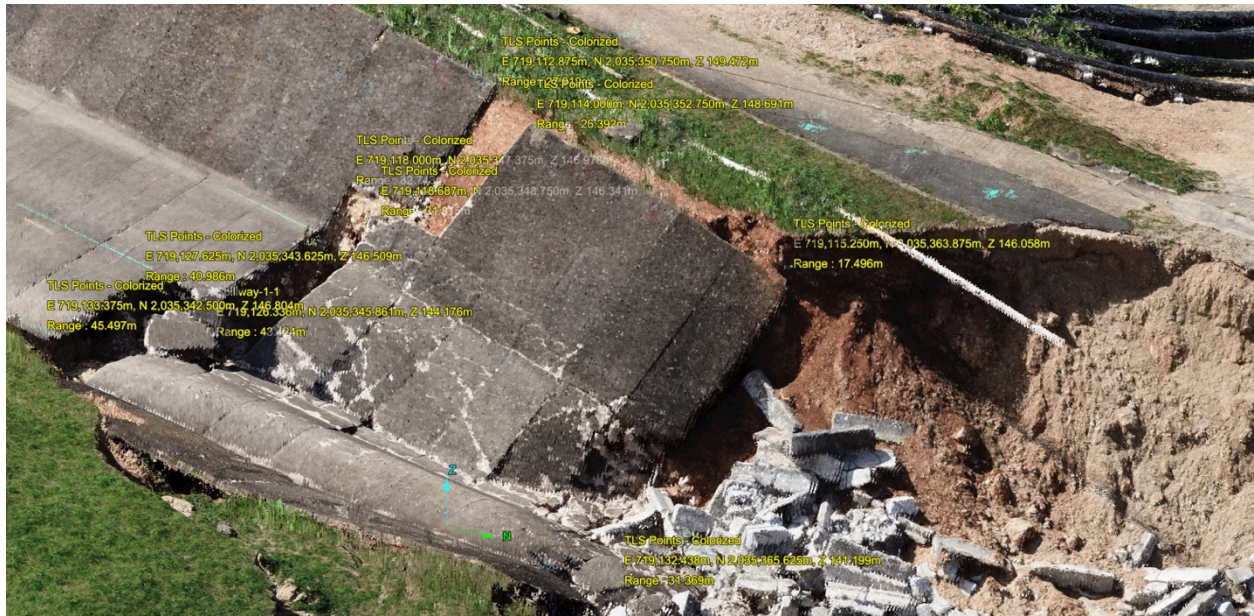
Figure G-5: Oblique view of the damaged section D of the spillway.
