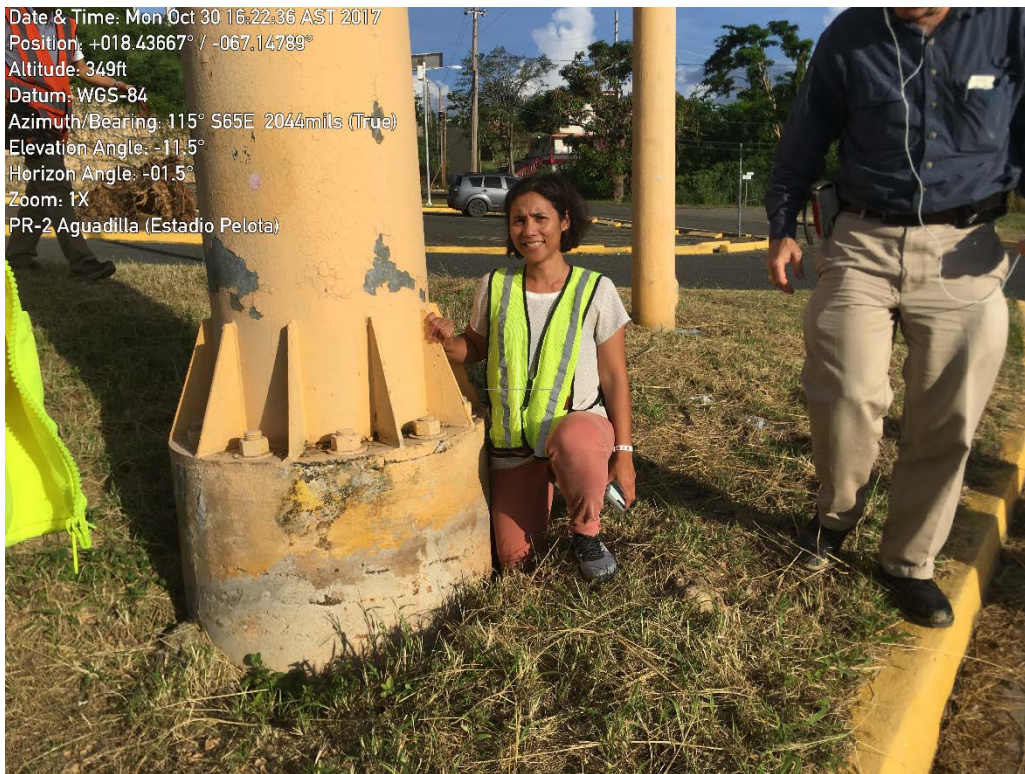
Figure E-2: Photo of drilled shaft of cantilevered traffic sign at Site F2 (Lat: +18.43681, Lon: -67.14776; 2017.10.30).
