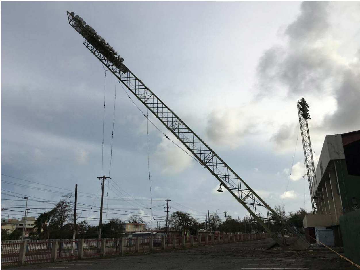
Figure 6-11: Photo of failed tower published by El Vocero 9/27/17 (Photo from Bartolomei, 2017) (Lat: +18.002275, Lon: -66.630714).
