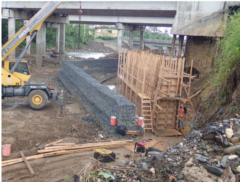
Figure 4-31: West abutment of westbound Highway 52 bridge over the Inabón River (Lat: +18.04003, Lon: -66.53795, October 31, 2017).
