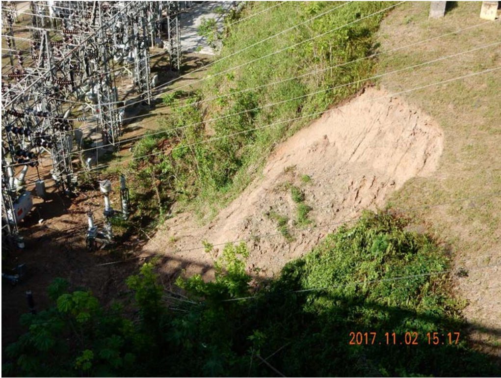
Figure B-9: Utuado, Dos Bocas Dam, Surficial slide near transformer's yard; Lat: +18.33541333, Lon: -66.66602664; 2017.11.02; #3940.
