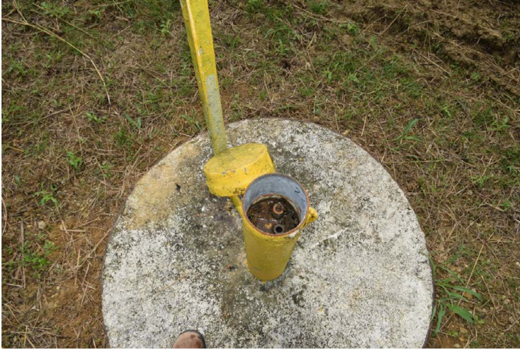
Figure 3-10: Water and debris in piezometer (Lat: +18.397658, Lon: -66.924462).
