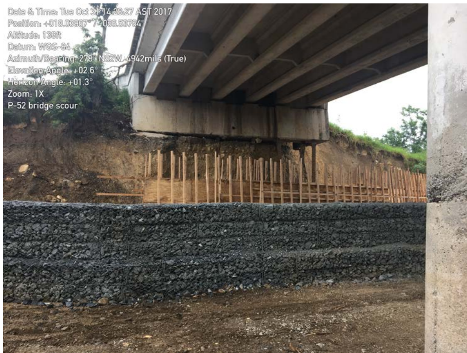
Figure 4-32: West abutment of westbound Highway 52 bridge over Inabón river (October 31, 2017). Photo shows erosion along this abutment and ongoing emergency repair work (Lat: +18.03967, Lon: -66.53764).
