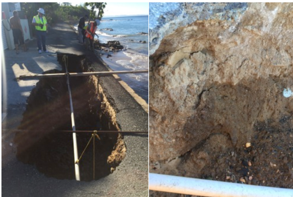
Left photo: Lat: +18.30246, Lon: -67.23669, 2017.11.3, 08:22 AST; Right photo: Lat: +18.30254, Lon: -67.23678, 2017.11.3, 08:19 AST. Seepage through seawall observed at the bottom of the sinkhole.
