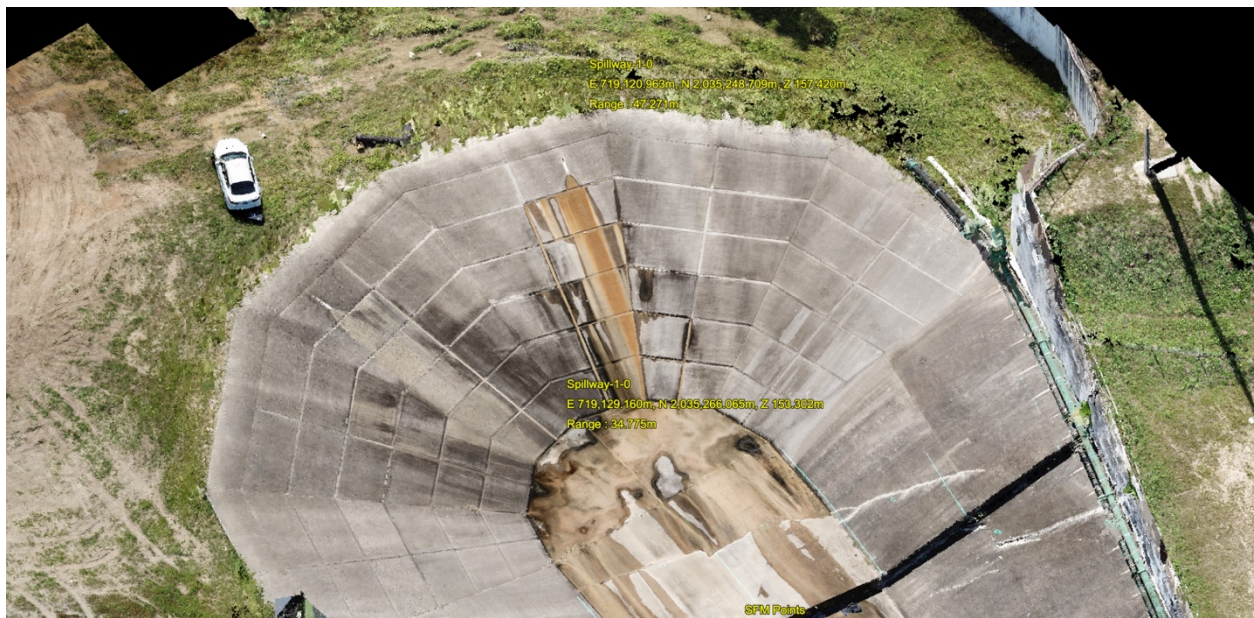
Figure G-7: Figure 7. Hybrid SFM-TLS model of the upper apron of the spillway, above section A. Reservoir waters pass over a soil bench before plunging down the apron when entering the spillway.
