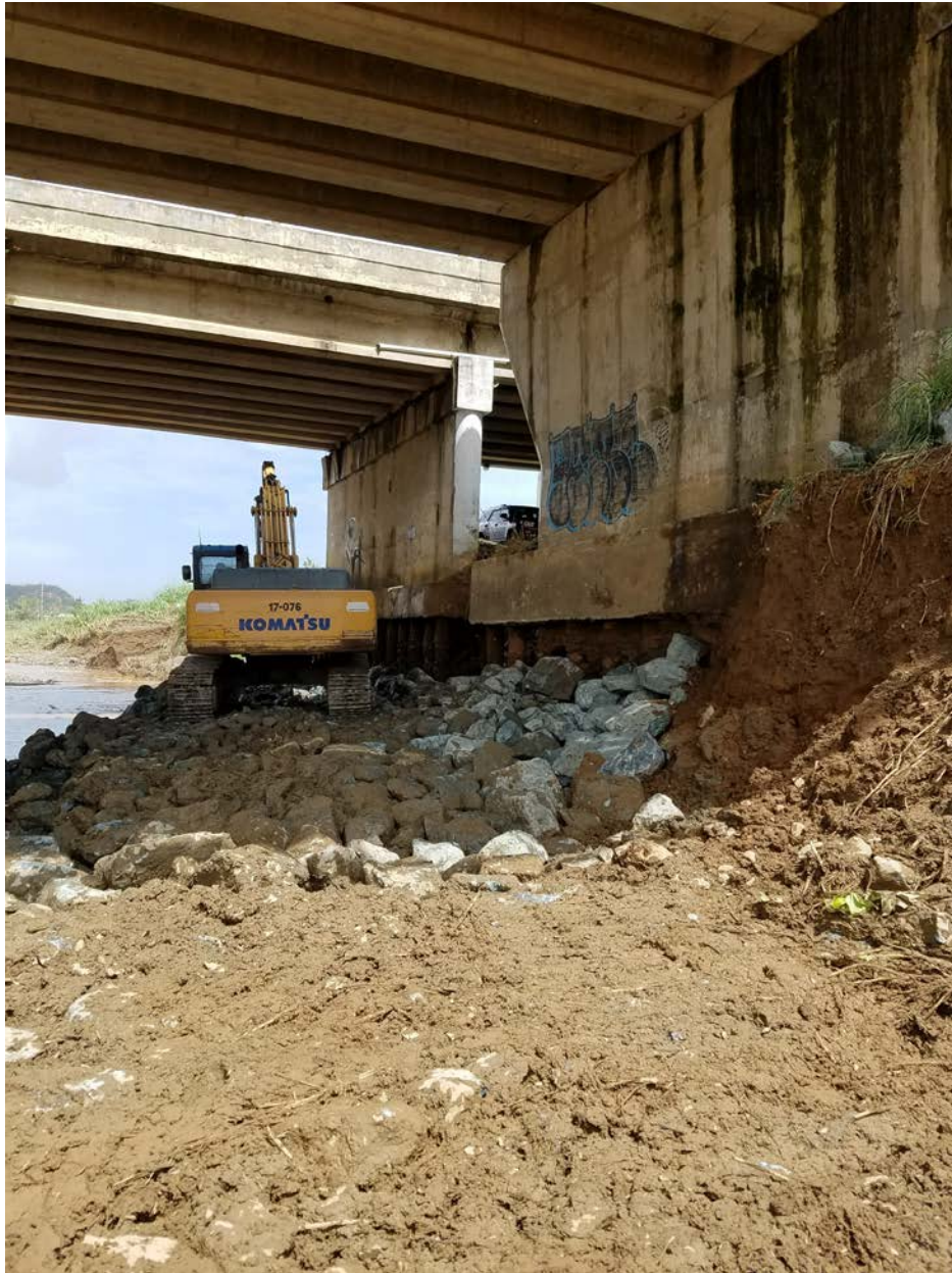
Figure 4-35: Erosion along pier foundation of bridges of Highway PR-177 in Bayamón, PR (Photo by Geo-Cim) (Lat: +18.38384, Lon: -66.13571).
