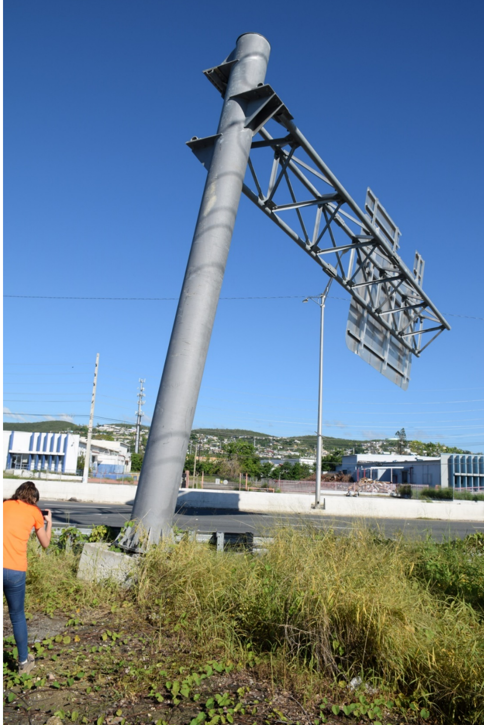
Figure E-3: Photo of cantilevered traffic sign at Site F3 (Lat: +17.987991, Lon: -66.648788; 2017.11.1).
