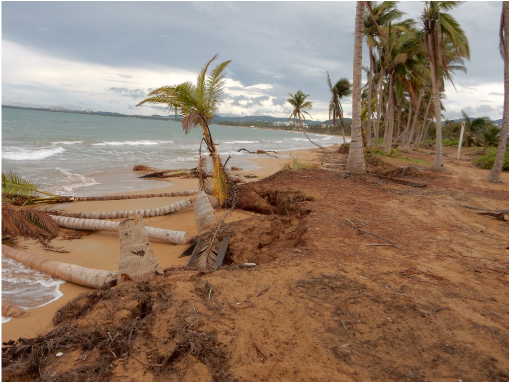
Figure C-2: Coastal Erosion, Yunque Mar, Rio Grande, PR; Lat: +18.39774, Lon: -65.76471; 2017.10.28; #3211.
