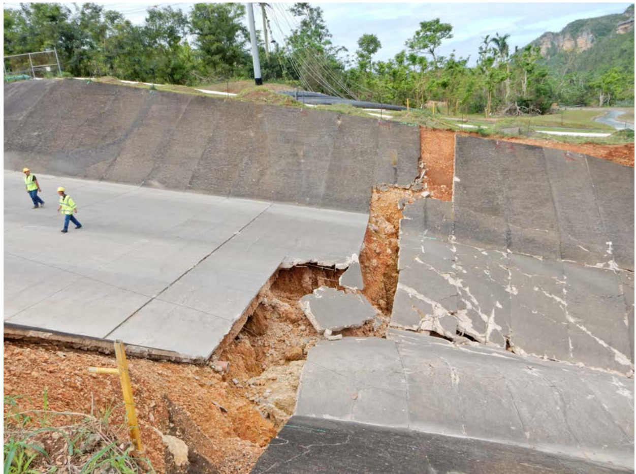
Figure 3-15: Displaced and damaged spillway (Lat: +18.39707, Lon: -66.92535).
