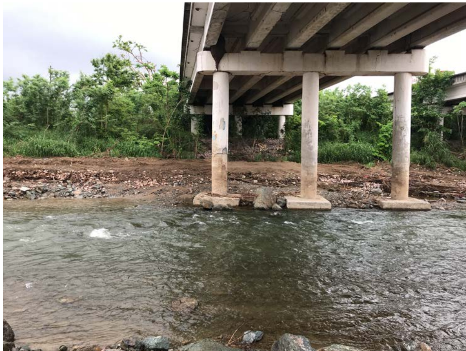
Figure 4-34: Erosion along pier foundation of westbound Highway 52 bridge over the Inabón River (Lat: +18.03992, Lon: -66.53754, October 31, 2017).
