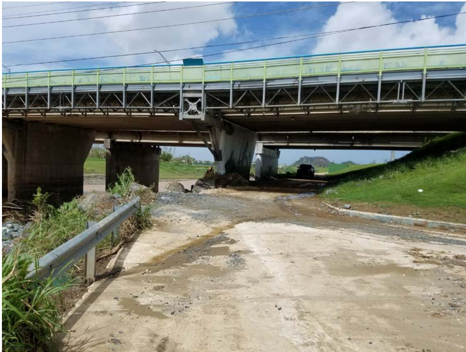
Figure 4-36: Erosion along pier foundation of bridges of Highway PR-177 in Bayamón, PR (Photo by Geo-Cim) (Lat: +18.3838, Lon: -66.13557).
