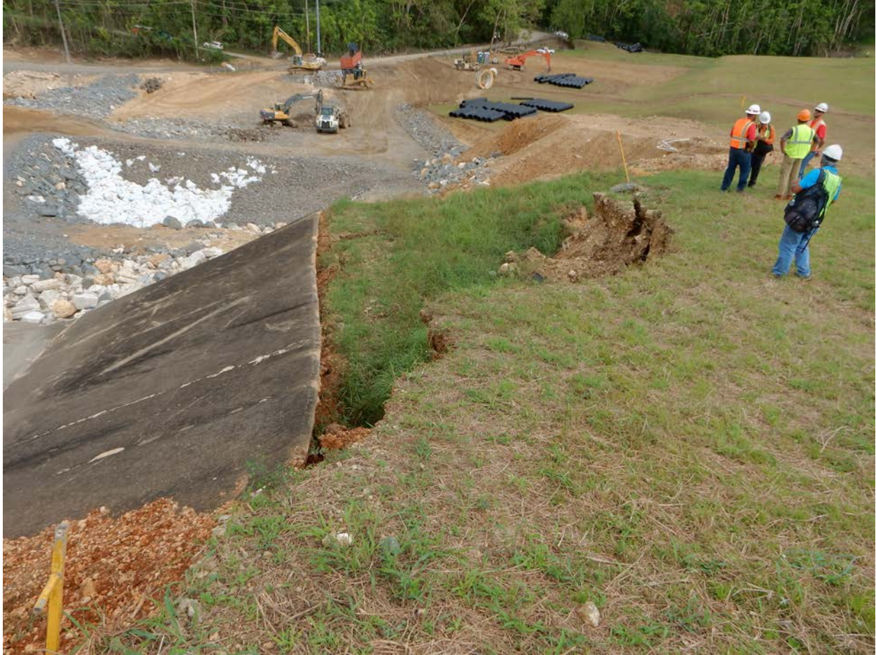
Figure 3-16: Scarp adjacent to the spillway (Lat: +18.39702, Lon: -66.92540).
