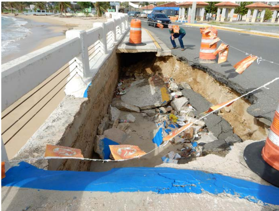
Figure 4-20: Coastal erosion Site CE5 – Collapse of sidewalk along coastal avenue in Aguadilla Town Center (Lat: +18.43159, Lon: -67.15529).
