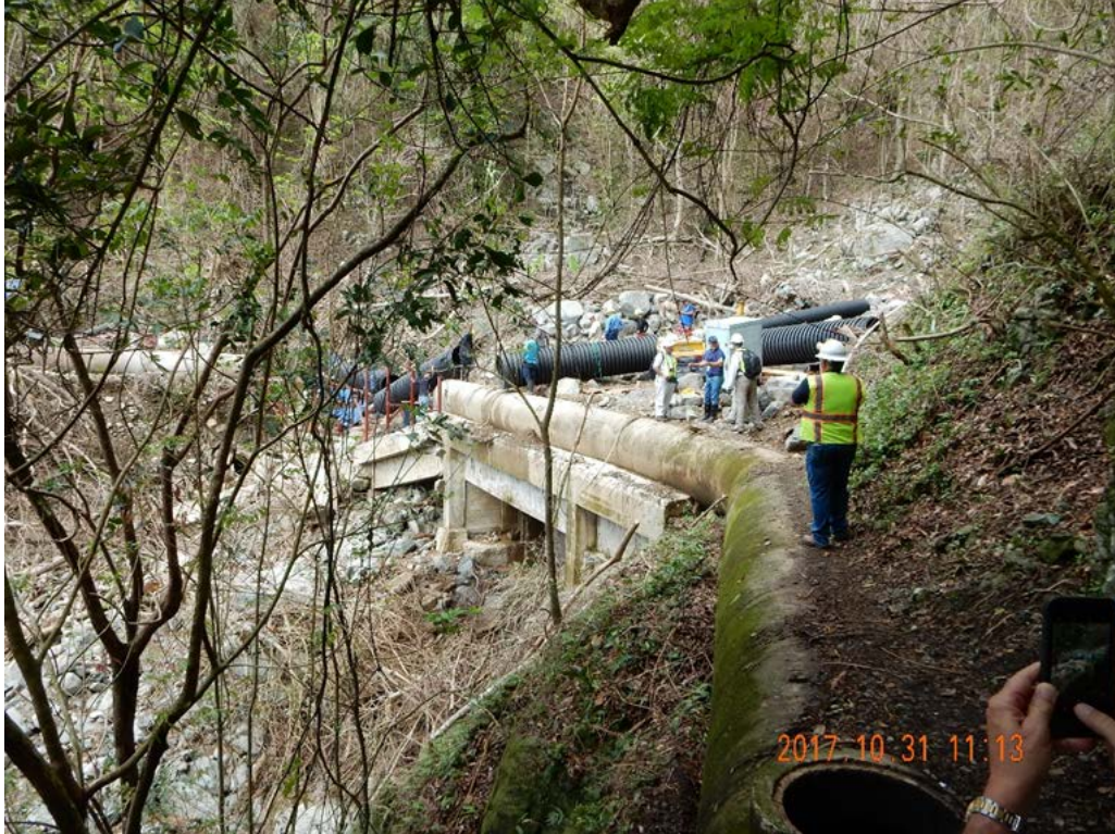
Figure A-14: Raw water line severed by debris flow, Carillo, Villalba, PR-149, Km 59.1; Lat: +18.15855, Lon: -66.49808; 2017.10.31; #3500.
