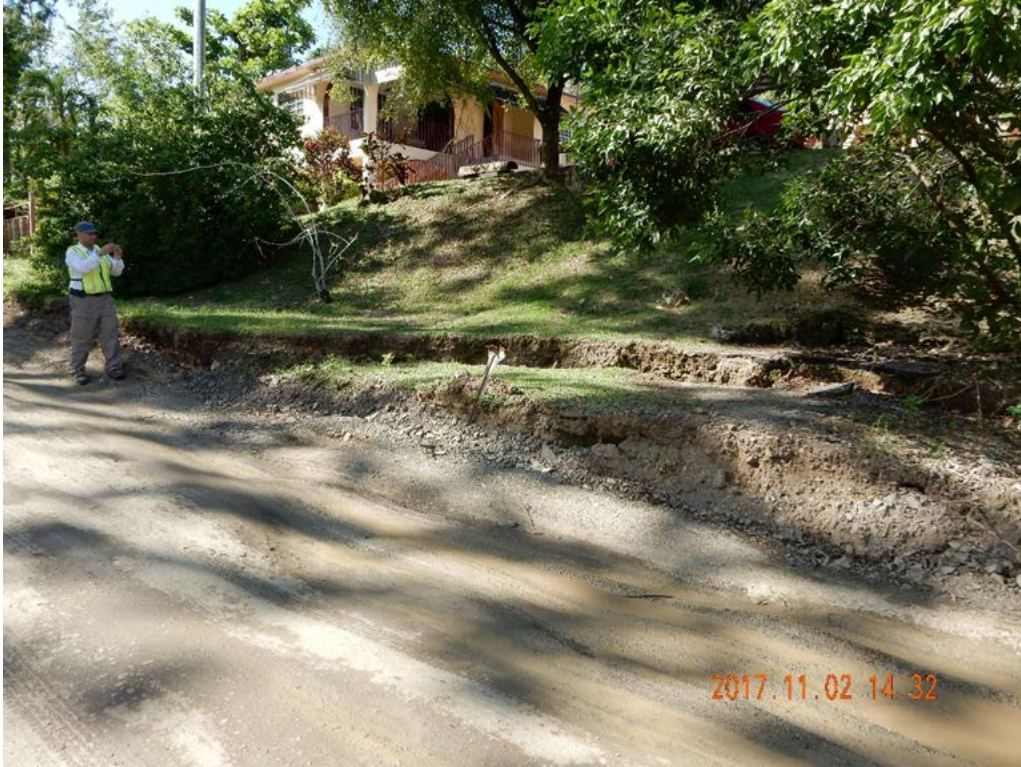
Figure A-31: Utuado, PR-146, Km 9.3, Rio Limón Slide, Head Scarp; Lat: +18.32294444, Lon: -66.599125; 2017.11.02; #3929.
