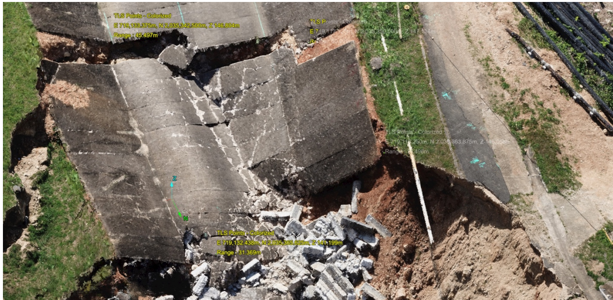
Figure G-6: Oblique view of the damaged section D of the spillway.
