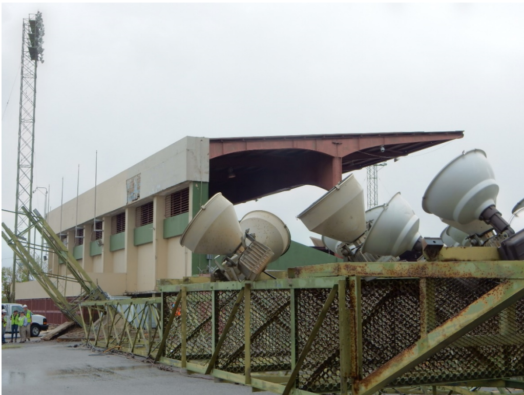
Figure E-8: Photo of portion of the structure of the failed illumination tower (Lat: +18.00207, Lon: -66.63098; 2017.10.31).
