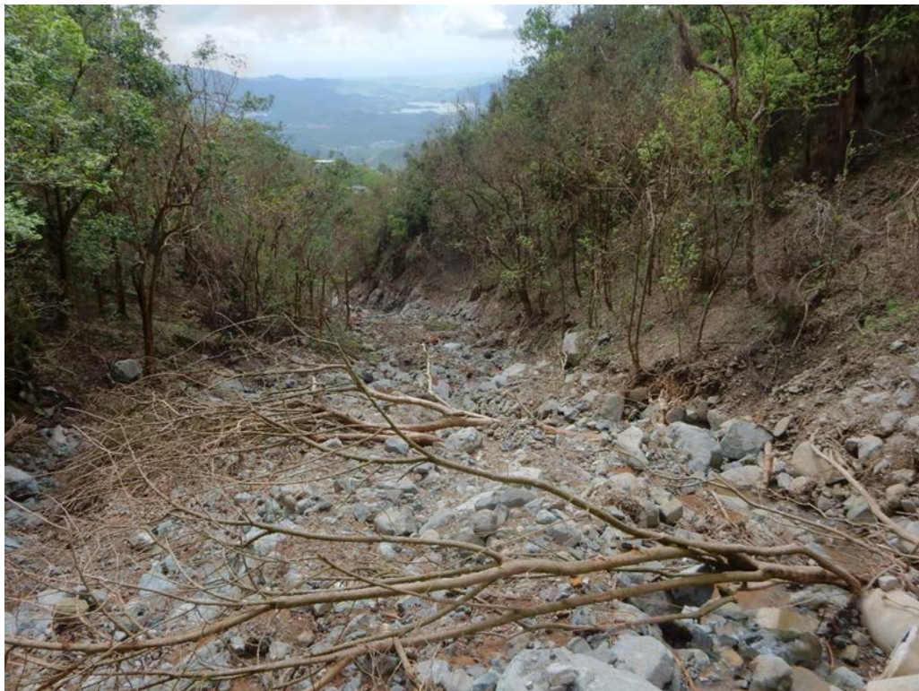
Figure A-17: Downstream of raw water line break, Carillo, Villalba, PR-149, Km 59.1; Lat: +18.15849, Lon: -66.49821; 2017.10.31; #3515.
