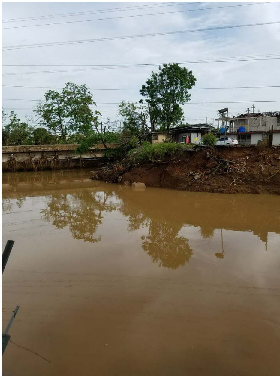
Figure 4-40: River bank erosion failure of Guaynabo River at Site RE3 (Photo by Geo-Cim) (Lat: +18.37307, Lon: -66.13248).
