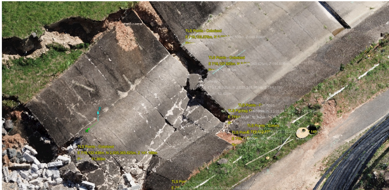
Figure G-4: Oblique view of the damaged section D of the spillway.
