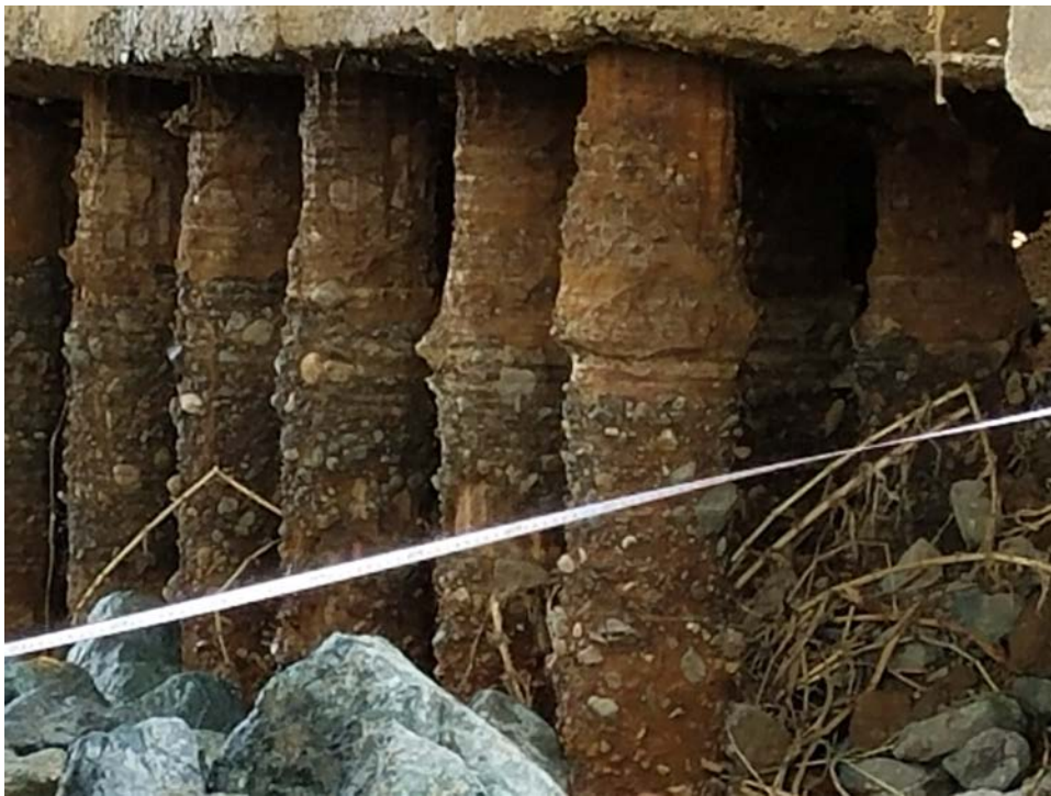
Figure 4-37: Erosion along pier foundation of bridges of Highway PR-177 in Bayamón, PR (Photo by Geo-Cim) (Lat: +18.38389, Lon: -66.135562).
