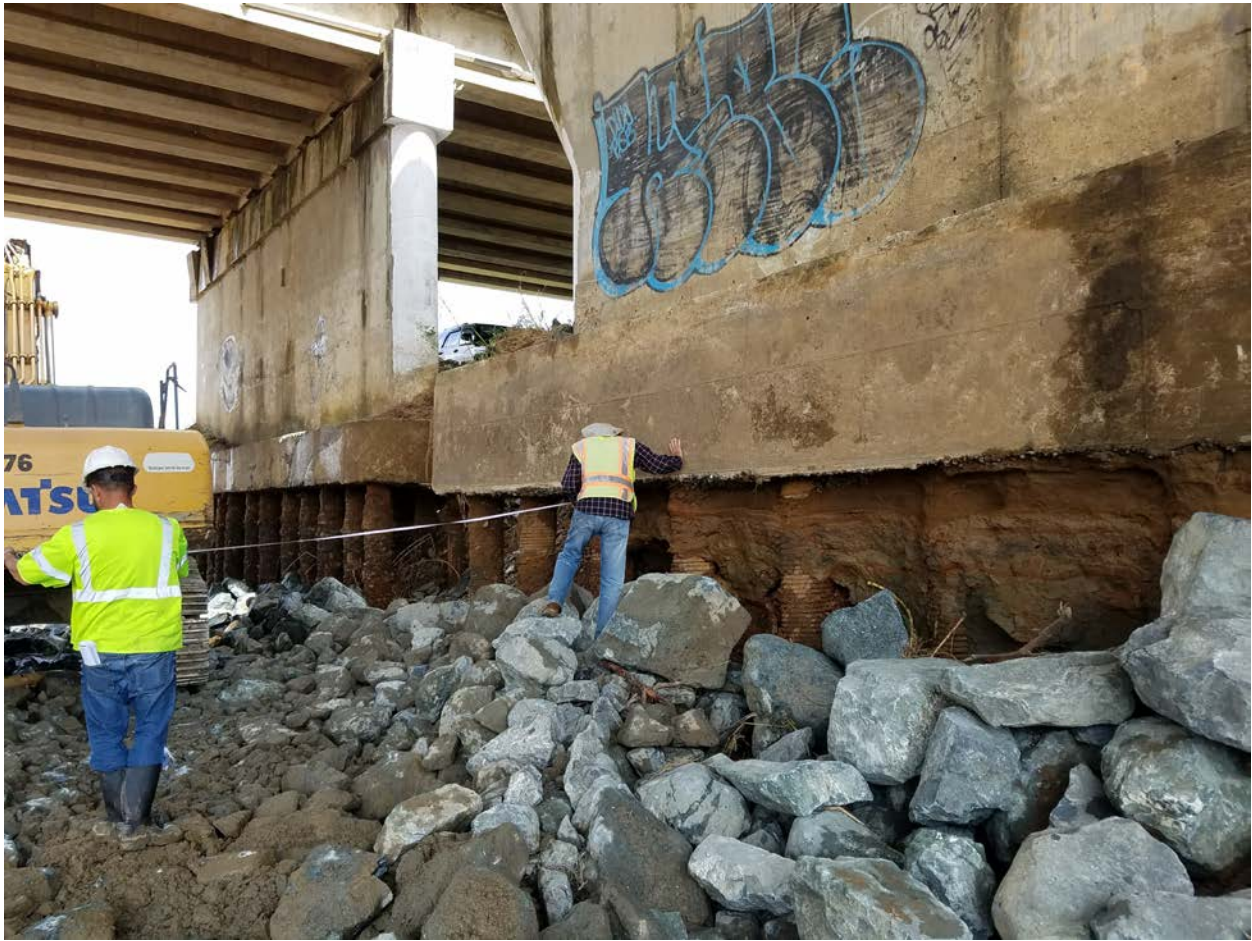
Figure 4-38: Erosion along pier foundation of bridges of Highway PR-177 in Bayamón, PR (Photo by Geo-Cim) (Lat: +18.38392, Lon: -66.13581).
