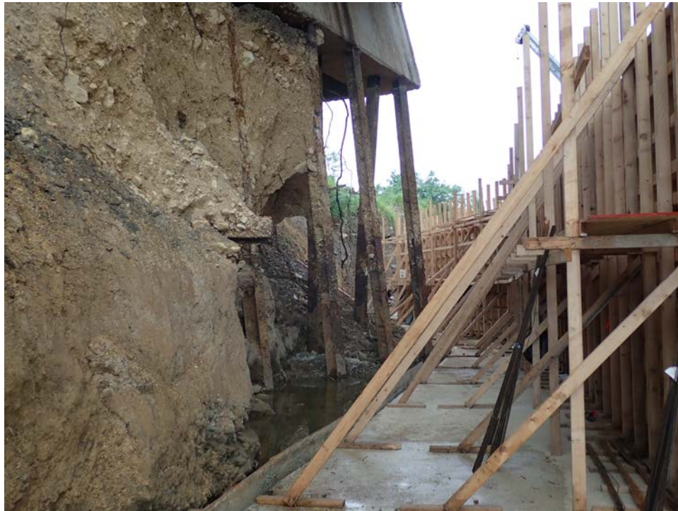
Figure 4-33: Erosion damage at west abutment of westbound Highway 52 bridge over the Inabón River (Lat: +18.03962, Lon: -66.53767, October 31, 2017).
