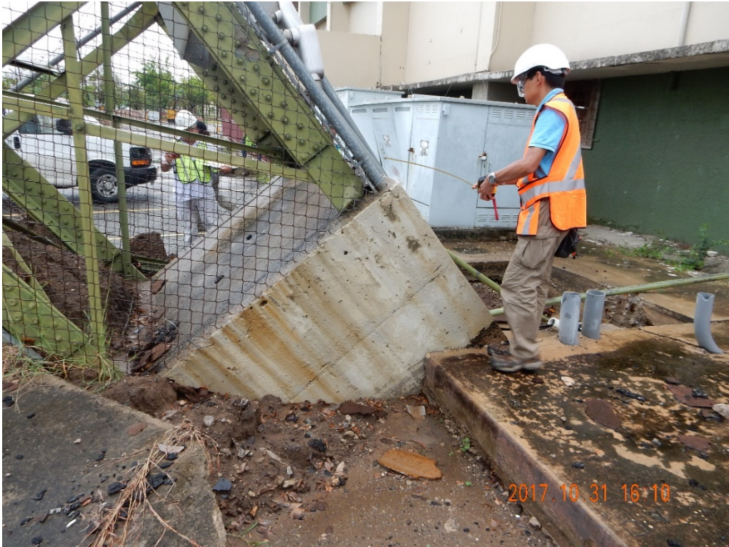
Figure E-5: Photo of illumination tower foundation pedestal at Site F4 (Lat: +18.00207, Lon: -66.63098; 2017.10.31).
