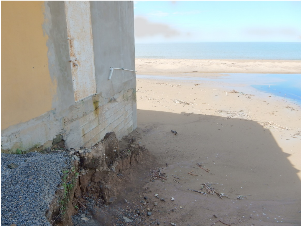
Figure C-11: Coastal erosion at El Maní, Mayagüez; Lat: +18.24732, Lon: -67.17516; 2017.11.04; #4175.
