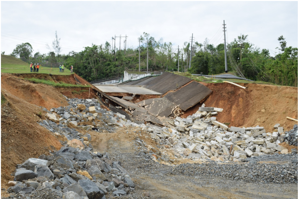
Figure 3-13: Damaged spillway (Lat: +18.39724, Lon: -66.92554).
