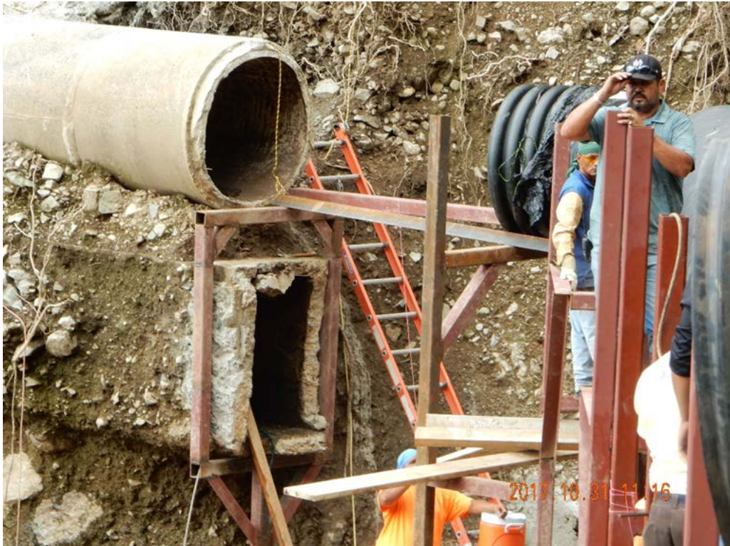
Figure A-15: Raw water lines, rectangular section about 100 years old; Lat: +18.15848, Lon: -66.49798; 2017.10.31; #3503.
