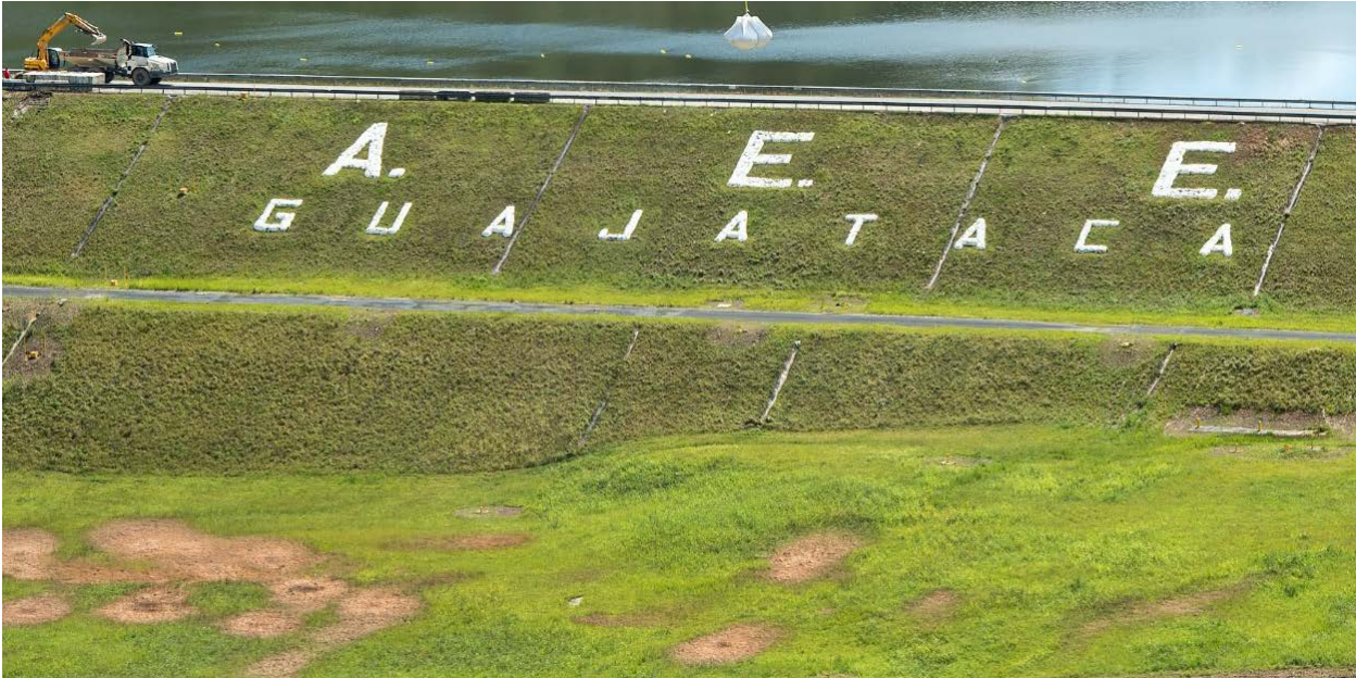
Figure 3-9: Sand boils downstream of the dam toe (photographs from the Pennsylvania National Guard).
