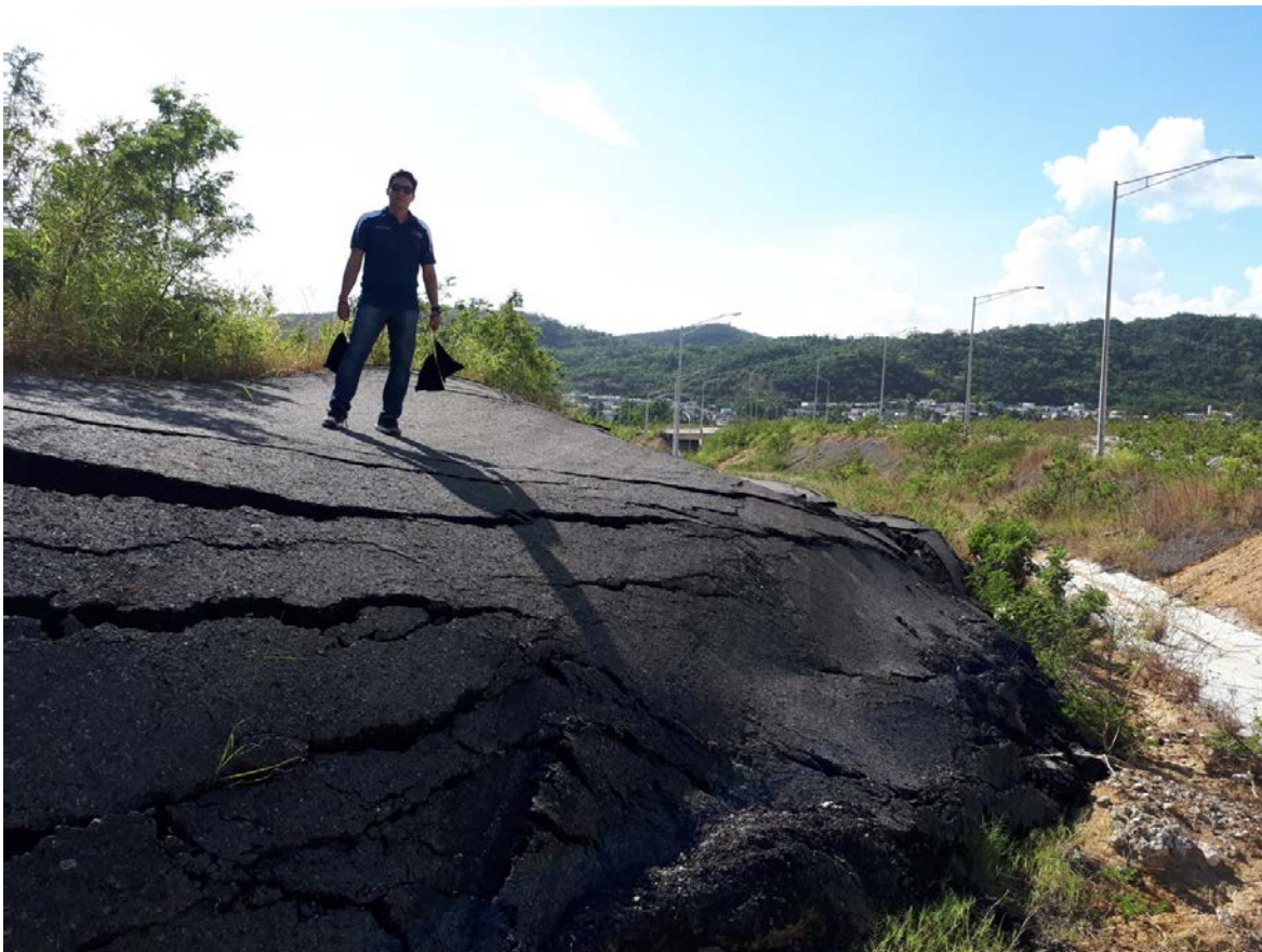
Figure 2-18: Photo of Toe of PR-9 landslide in January 2018 (Lat: +18.033145, Lon: -66.637579).
