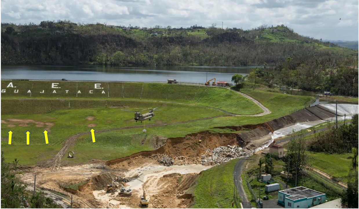
Note: Yellow arrows show location of sand boils downstream of the dam toe.
