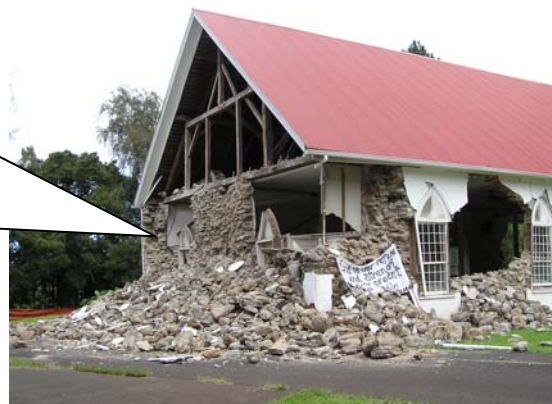
Figure 36: Location 21, Kalāhikiola Congregational Church, Kapa’au. Weakly cemented stacked rock walls failed dramatically.
