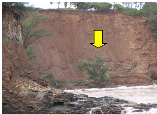
Figure 22: Location 19, Keokea Bay. Cliffs failed during the earthquake: Note displaced trees (arrow) and slide scars.
