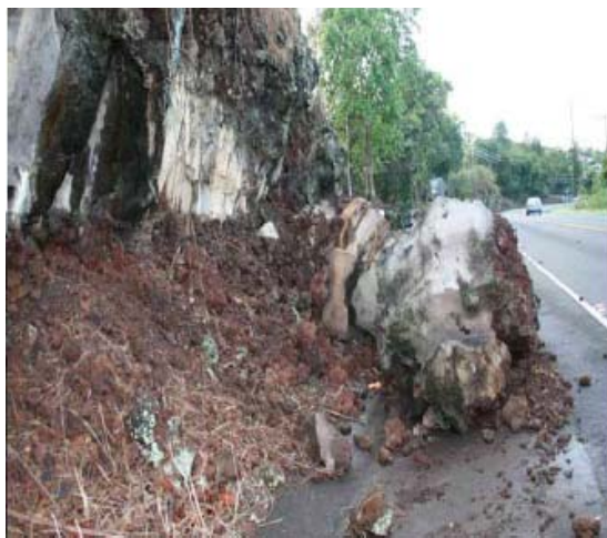
Figure 5: Failed rock cut: massive a'a block undermined by raveled a'a clinker (Chock, 2006; after Robertson et al, 2006)
