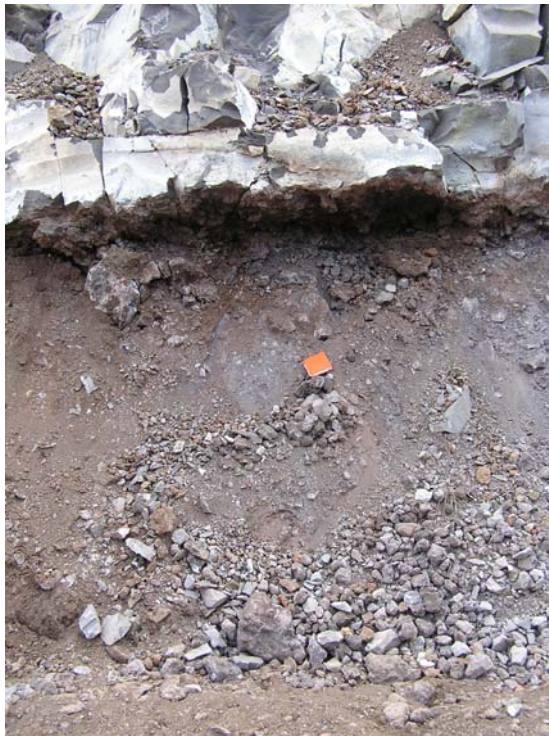
Figure 8: Location 25, Hwy 270 north of Kawaihae. Cantilevered block of massive a'a basalt, undermined by raveled clinker
