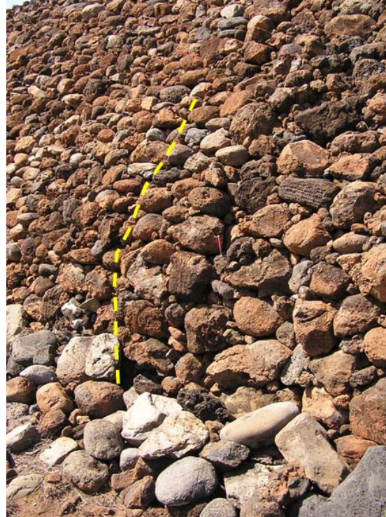
Figure 35: Location 29, NE corner Puukohola Heiau. Bulging of rock face approaches 90 degree inclination as indicated by yellow line. Bulge is clearly seen in stereo (see Appendix).
