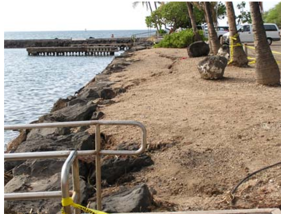
Figure 27: Location 27, Kawaihae Small Boat Harbor, showing ground crack resulting from lateral spreading.
