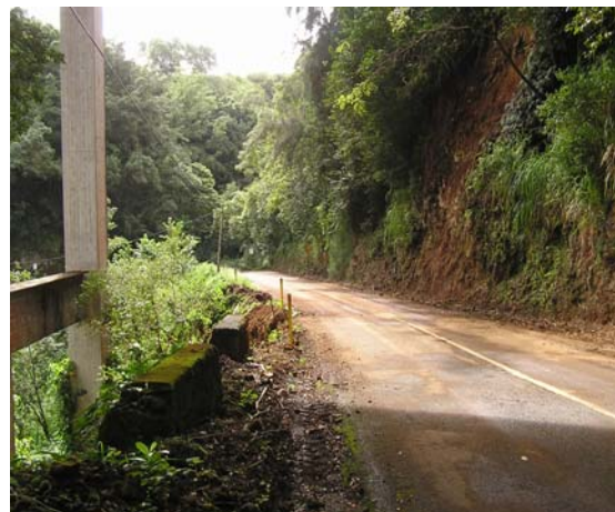
Figure 17: Location 4, old Hwy 11 near Ookala, Modern Hwy 11 viaduct above. Soil slide in very steep road cut in vicinity of abutment of viaduct, typical of many slides along this road.
