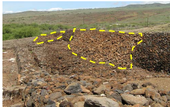
Figure 33: Location 29, Mailekini heiau. Significant raveling and slumping of interior face of the eastern wall (outlined).
