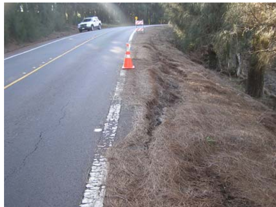
Figure 40: Location 15, north of Mile Post 9.4 Hwy 250. Slump failure of embankment on makai (west) side road.
