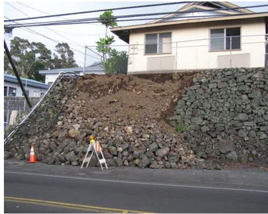
Figure 38: Location 35, Captain Cook. Failed stacked rock retaining wall.
