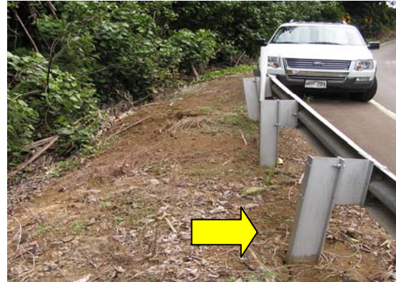
Figure 41: Location 18, Hwy 270 near Makapala, makai side. Arrow indicates tension cracks and short head scarp (12 inches) at crest of steep and high fill slope.
