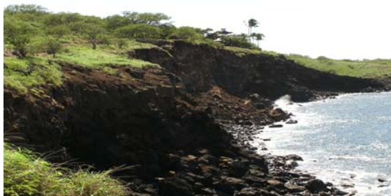
Figure 24: Location 23, failed cliff south of Honoipu Landing (Kuakini Trail).
