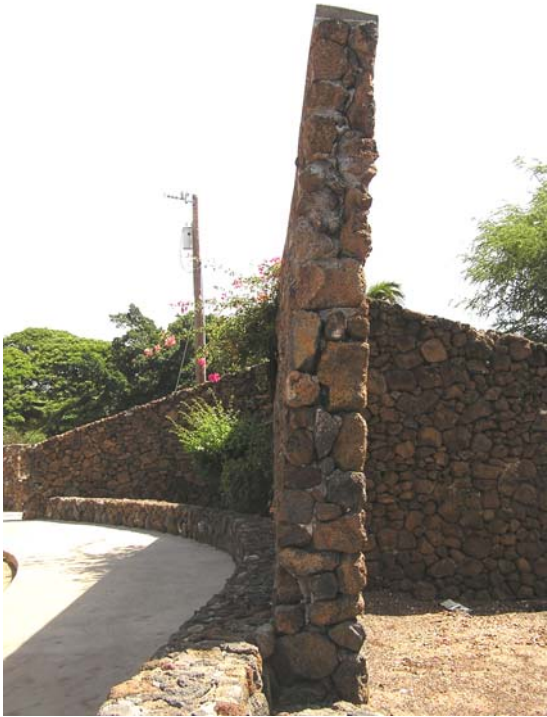
Figure 37: Location 30, Spencer Beach Park, south of Kawaihae. Apparent earthquake damage of partially mortared rock wall.
