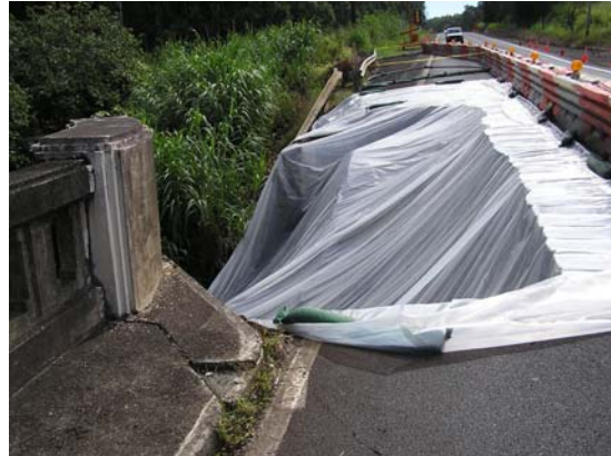
Figure 39: Location 6, Mile Post 35, Hwy 11 near Pa’auilo. Failure of fill at makai (east) side of southern approach to bridge.
