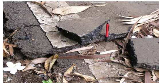
Figure 43: Location 20, bridge at approximately MP 28, Hwy 270. Thrusting of AC pavement.
