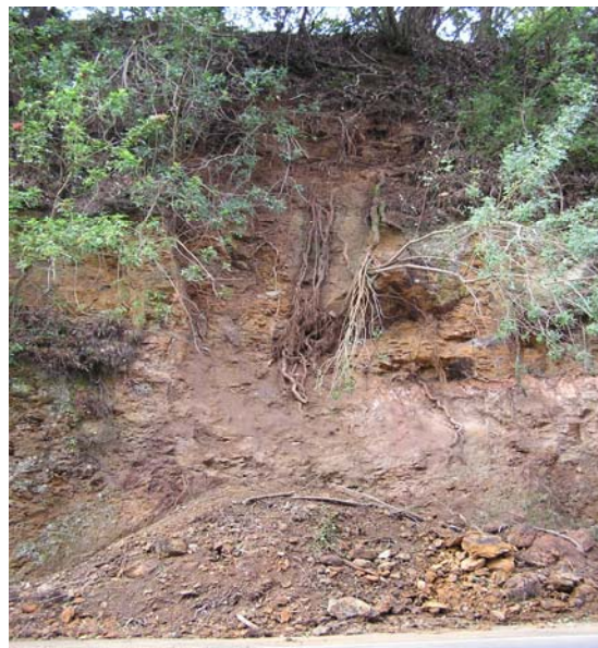
Figure 19: Location 16, Near Kapaau (Kohala), Hwy 270. Tree roots within fractures influenced instability in road cuts in soil.
