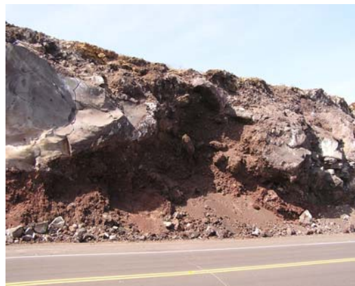
Figure 9: Location 32, Hwy 11. Failure of massive basalt rock overlying weaker weathered rock (baked zone).
