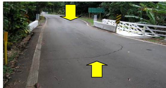
Figure 42: Location 20, bridge at approximately MP 28, Hwy 270. AC pavement cracked at approximately the cut/fill transition lines of underlying subgrade (cracks in AC).
