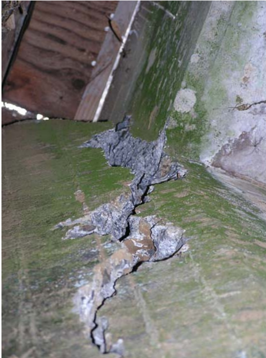
Figure 44: Location 20, bridge at approximately MP 28, Hwy 270. At SW corner of bridge, looking upward. Wooden plank sidewalk above. Significant spalling of bridge abutment headwall.
