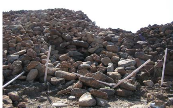
Figure 32: Location 29, Pu'ukoholā heiau, north side: Earthquake caused collapse of access step structure.
