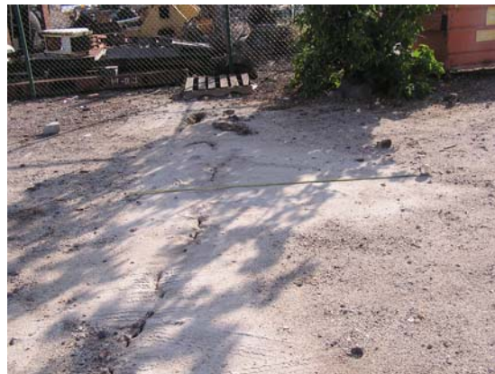
Figure 28: Location 27, Kawaihae Small Boat Harbor parking lot, adjacent boat yard at south side. Liquefied (white) sand was ejected from ground crack.
