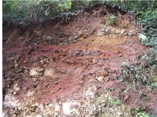
Figure 18: Location 4: old Hwy 11 near Ookala. Failure of soil above rock. Note inclusions of rock within soil.
