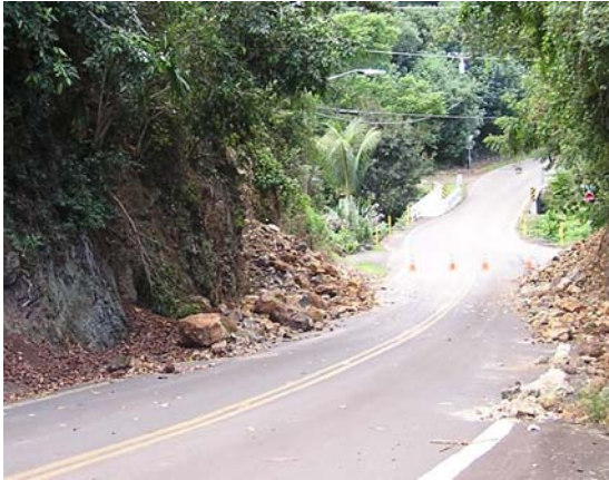
Figure 4: Hwy 270, near Keokea Bay Beach Park access road: Highway blocked by rock fall.
