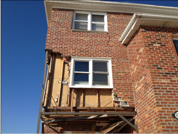
Figure 6.19 Damage to brick siding, Sea Gate, Brooklyn (November 9, 2012 – MRCE in collaboration with NYCDOB)
