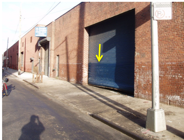
Figure 7.28 High water mark approximately five feet above sidewalk along Imlay Street, Red Hook, Brooklyn (40.680721° N, 74.010008° W, November 4, 2012).
