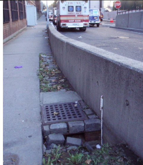
Figure 7.26 Washout at storm drain inlet, East 26 th Street (40.737767° N, 73.974794° W, November 3, 2012).
