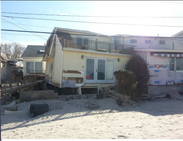
Figure 6.43 House washed off of CMU wall foundation, Breezy Point, Queens (November 5, 2012 – MRCE in collaboration with NYCDOB)
