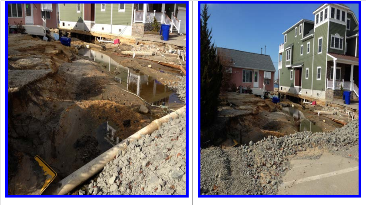
Figure 6.94 Sinkhole due to broken water/sewer line (Ocean County Engineering, 2012)
