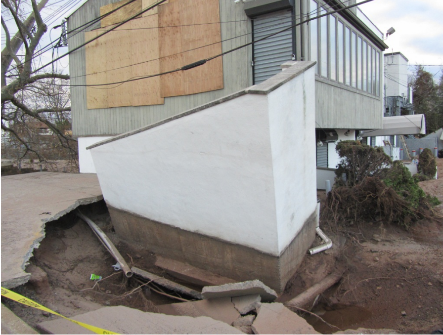
Figure 6.12 Scour undermining stair foundation and foundation drain, Seaver Ave and Father Capodanno Blvd, Staten Island (40.575944° N, 74.083015° W, November 4, 2012).
