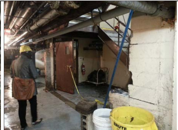
Figure 7.45 Unreinforced CMU wall overcome by flood water. The door to the stairwell had been closed, allowing water to fill the stairwell.
