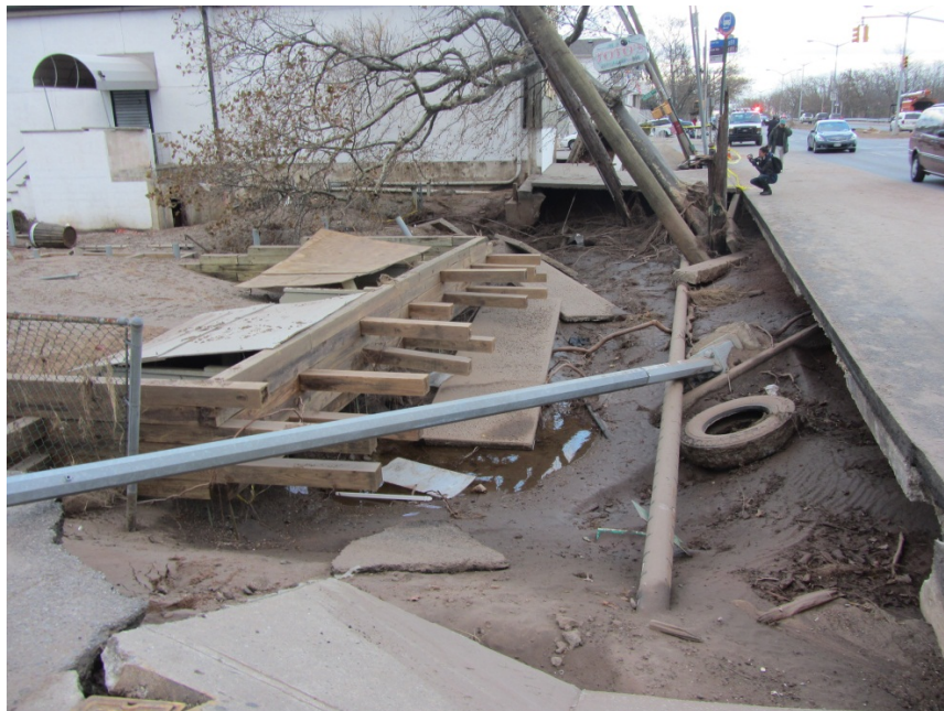
Figure 6.11 Scour undermining sidewalk, infrastructure utilities, and light pole foundation, Seaver Ave and Father Capodanno Blvd, Staten Island (40.575944° N, 74.083015° W, November 4, 2012).
