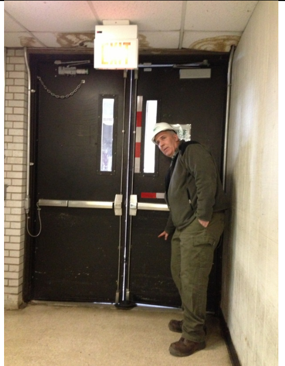
Figure 7.41 Flood level reached at aeration blower building door. This door was pushed open by flood water.
