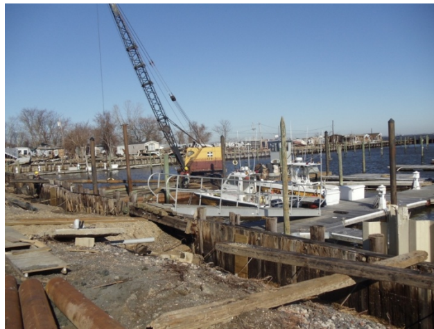
Figure 6.113 Erosion of sandy soils behind bulkhead (40°24'36"N, 74°00'02"W).
