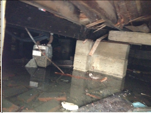
Figure 6.66 Basement flooding, Howard Beach, Queens. (November 16, 2012 – MRCE in collaboration with NYCDOB)
