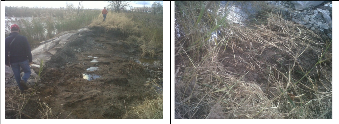
Figure 6.106 Breached section of the earthen berm showing remnants of sections with crushed stone (40°49'43.45"N, 74° 2'19.87"W).
