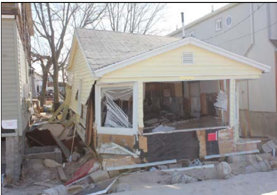
Figure 6.44 Collapsed CMU wall foundation, Breezy Point, Queens (November 5, 2012 – MRCE in collaboration with NYCDOB)
