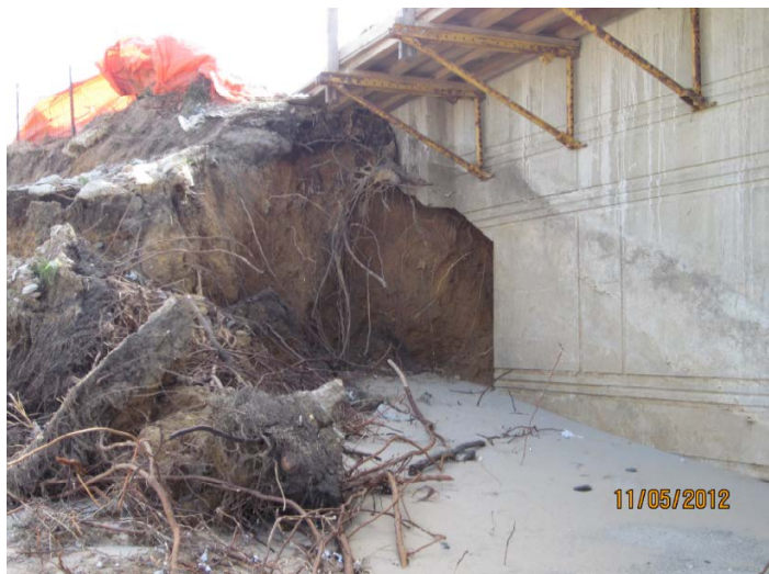
Figure 5.3 Erosion at the southeast abutment wingwall (NJDOT 2012a)
