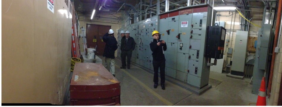
Figure 7.48 Electrical feeder and MCC room not flooded thanks to sandbagging measures.
