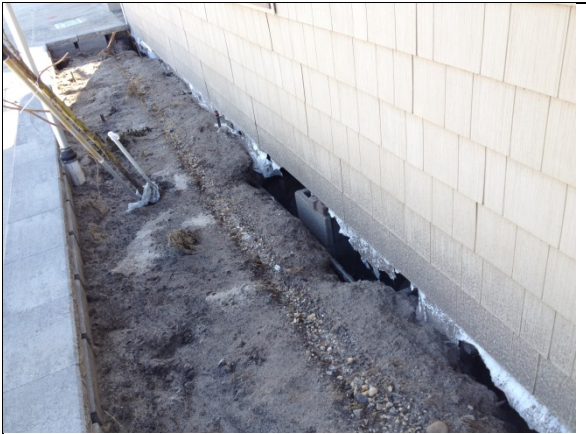
Figure 6.35 Erosion at CMU foundation wall, Rockaway, Queens (November 17, 2012 – MRCE in collaboration with NYCDOB)
