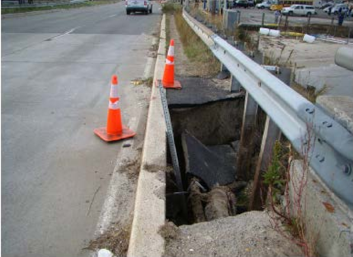
Figure 5.12 Erosion along the northwest abutment of the Tunney Bridge (westbound Route 37) 39° 56.9610" N, 74° 06.8341 W (NJDOT 2012a)
