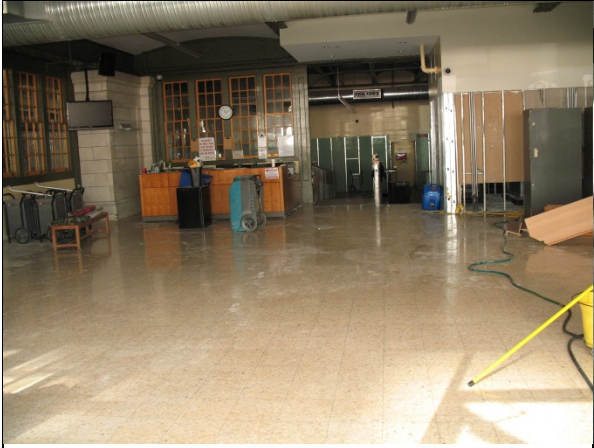
Figure 7.4 Flood damage, Governors Island ferry terminal (40.701061° N, 74.01177° W, November 3, 2012)
