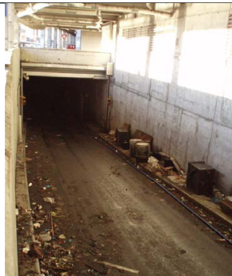
Figure 7.13 Evidence of flood inundation, Bellevue Hospital, East 30 th Street (40.73983° N, 73.973263° W, November 3, 2012).
