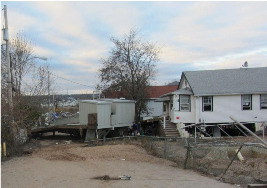
Figure 6.13 Damaged CMU block foundation, distressed timber frame house, and relocated wood deck, Staten Island (40.575944° N, 74.083015° W, November 4, 2012).
