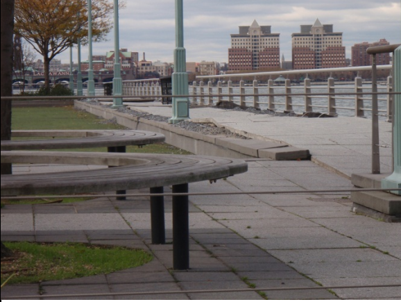
Figure 7.21 Heaved paving stones at Pier 46, west side of Manhattan (40.734326° N, 74.01092° W, November 2, 2012).
