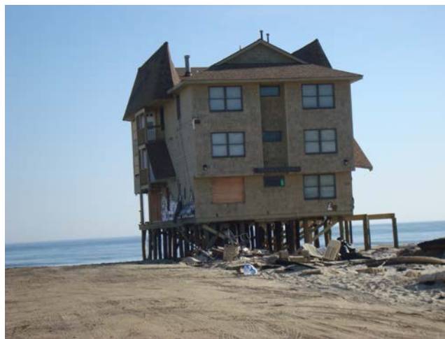
Figure 6.103 Buildings on deep foundations survived with serious structural damage
