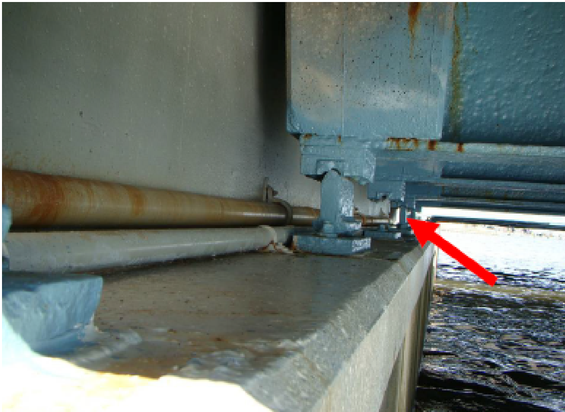
Figure 5.11 Mathis Bridge (eastbound) looking north showing a missing bearing for Stringer 3 (NJDOT, 2012a)
