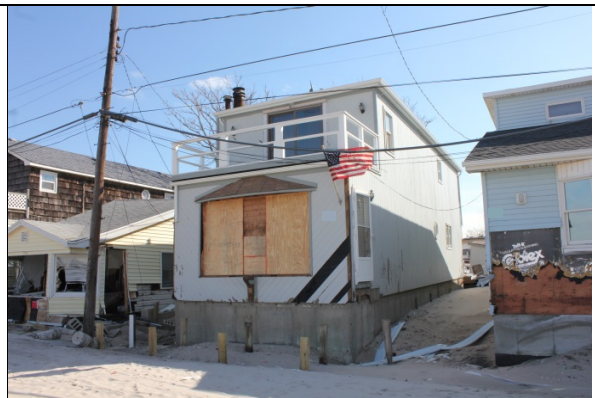
Figure 6.45 Concrete wall foundation with minor structural damage, Breezy Point, Queens (November 5, 2012 – MRCE in collaboration with NYCDOB)
