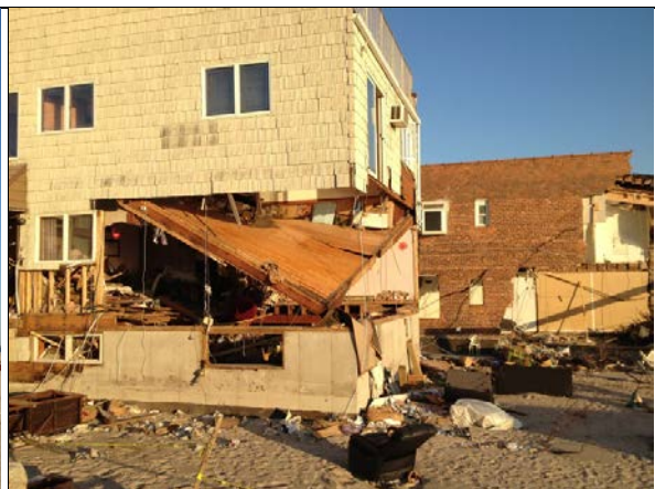
Figure 6.22 Partial wall and floor collapse, wood building on concrete wall foundation. Sea Gate, Brooklyn (November 9, 2012 – MRCE in collaboration with NYCDOB)
