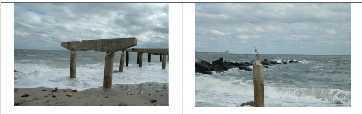
Figure 6.73 Damaged concrete piers that served as the supports for the boardwalk.
