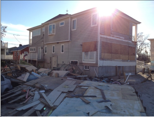
Figure 6.42 Concrete wall foundation with minor structural damage, Breezy Point, Queens (November 5, 2012 – MRCE in collaboration with NYCDOB)
