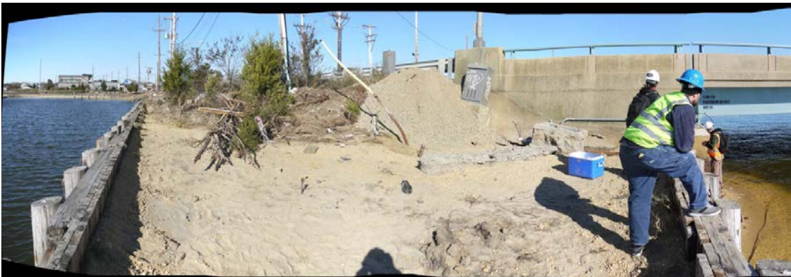
Figure 5.15 Erosion along the southwest abutment of the Mathis Bridge (eastbound Route 37) 39° 56.9610" N, 74° 06.8341 W
