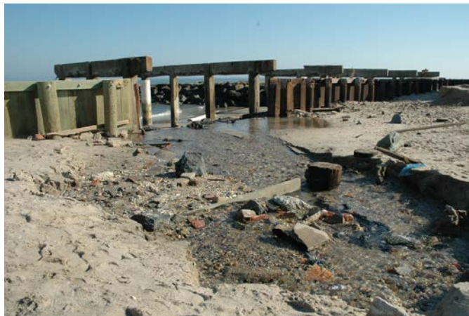
Figure 6.69 One of the breaches in the bulkheads along the coastline; in the backdrop are the remains of the boardwalk.
