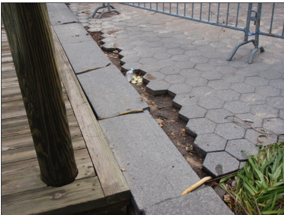
Figure 7.19 Displaced paving stones along Lower Manhattan waterfront, typical (40.706952° N, 74.01892° W, November 1, 2012).
