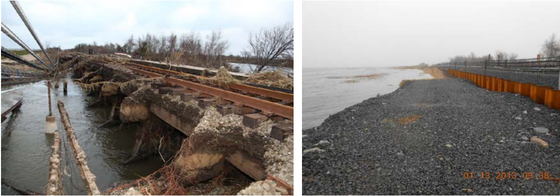
Figure 7.29 Washouts in Queens, along Rockaway subway [A] line after Sandy (left) and post mitigation work (right). Damage to earth embankment exposed old LIRR infrastructure (left). Photos credit: Khinda, J.S., ed., 2013.
