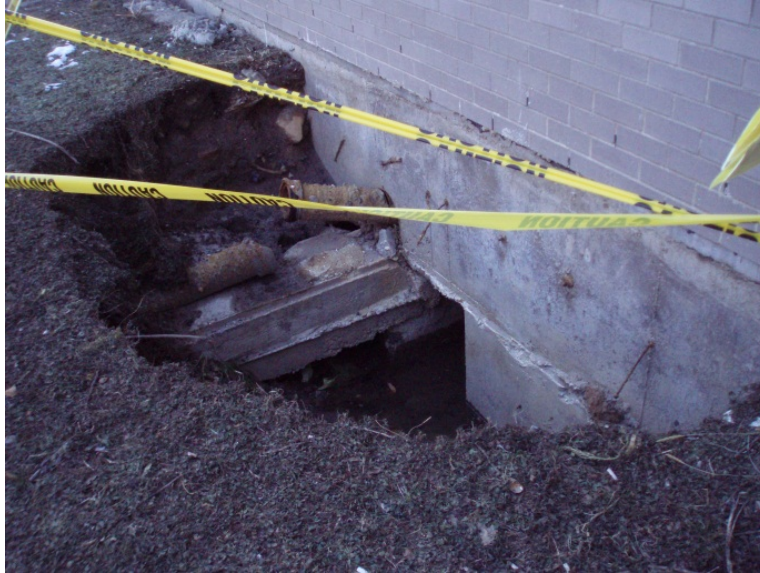
Figure 6.24 Sinkhole created by erosion and piping of flood water into building crawl space, Coney Island, Brooklyn. Note broken utilities undermined by the sinkhole.
