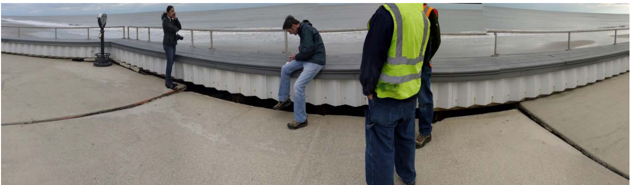
Figure 6.82 Settlement along the top of the seawall (39.41440 ° N, 74.35395 ° W, November 3, 2012)
