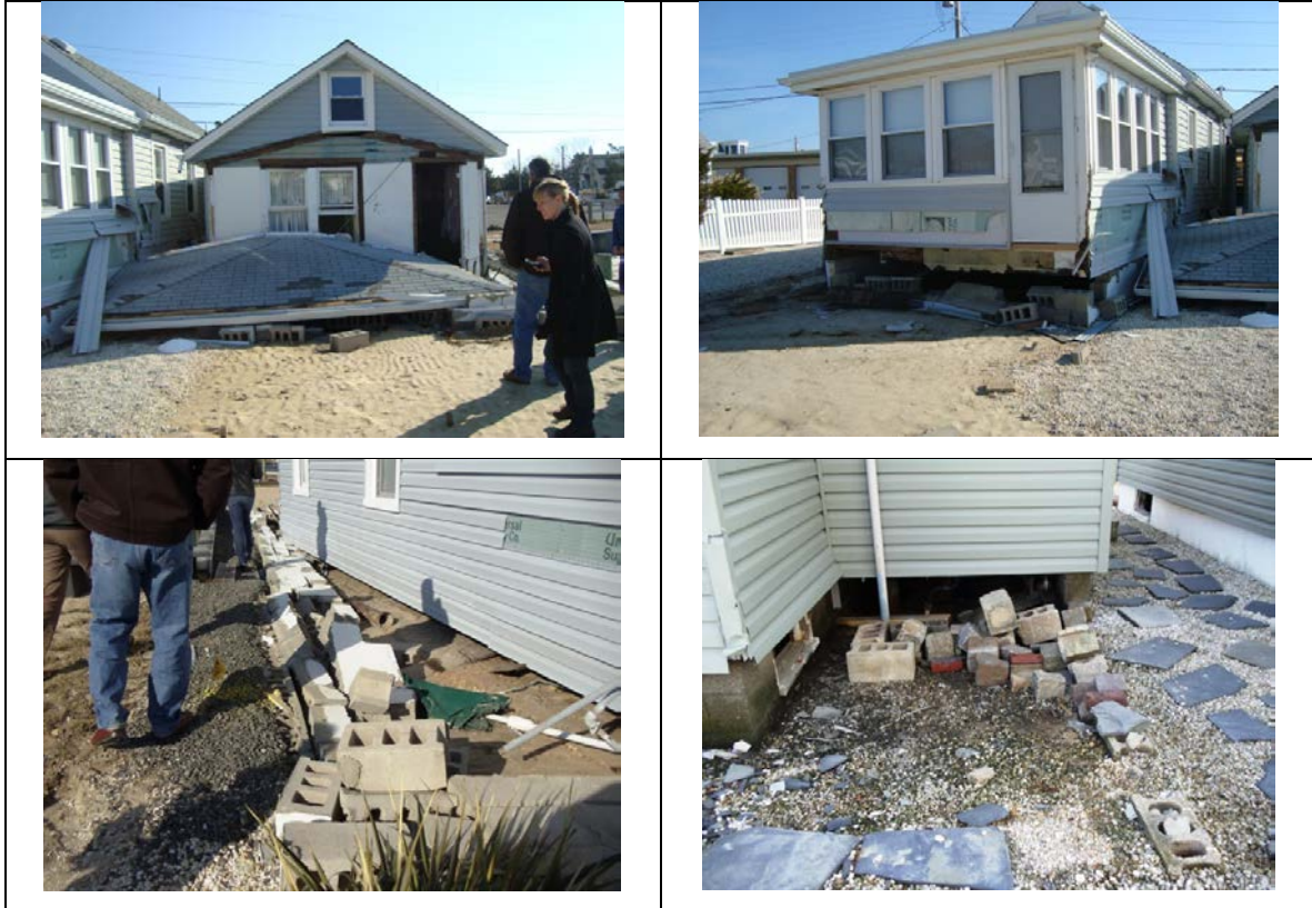
Figure 6.84 Damage to older structures on shallow foundations (39°38'41.15"N, 74°11'7.01"W)
