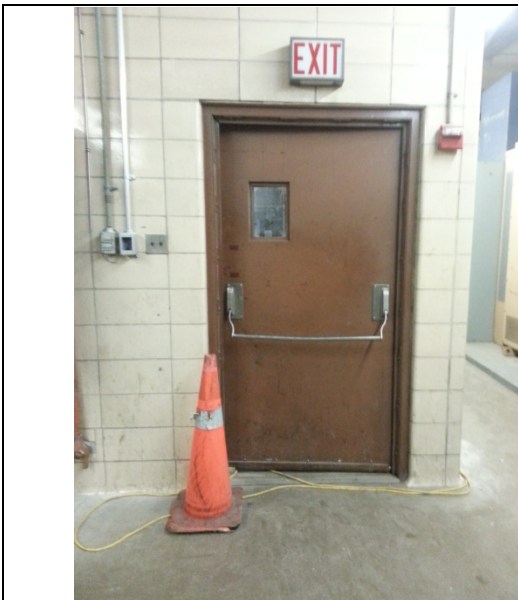
Figure 7.46 Door to electrical feeder and MCC room which was successfully sandbagged.
