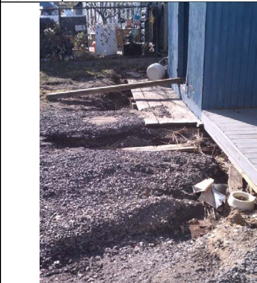
Figure 6.62 Soil washout, Broad Channel, Queens (November 6, 2012)
