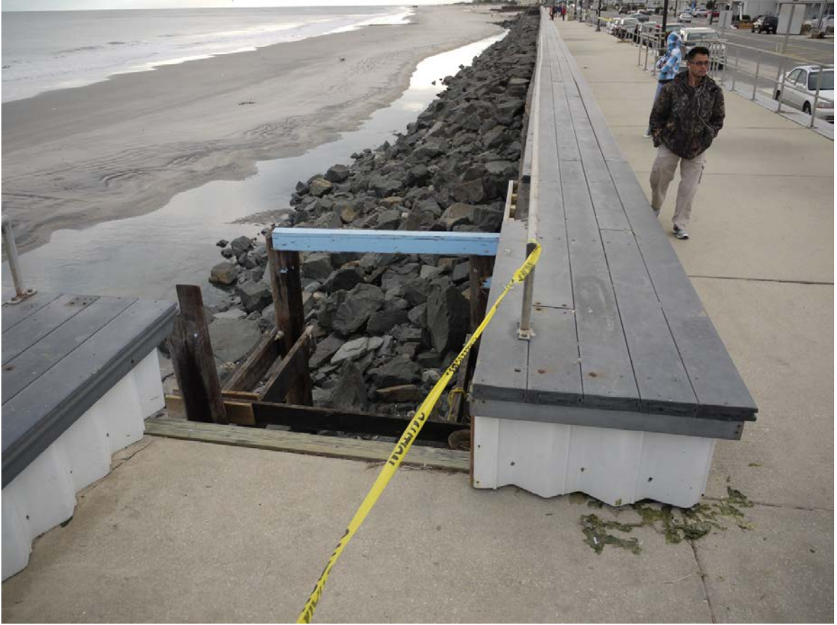
Figure 6.81 Washed-out stair on seawall (39.41387 ° N, 74.35460 ° W, November 3, 2012)
