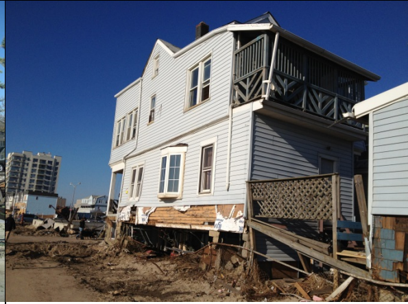
Figure 6.34 Void in CMU block foundation wall; wood frame building still standing, Rockaway, Queens (November 17, 2012 – MRCE in collaboration with NYCDOB)
