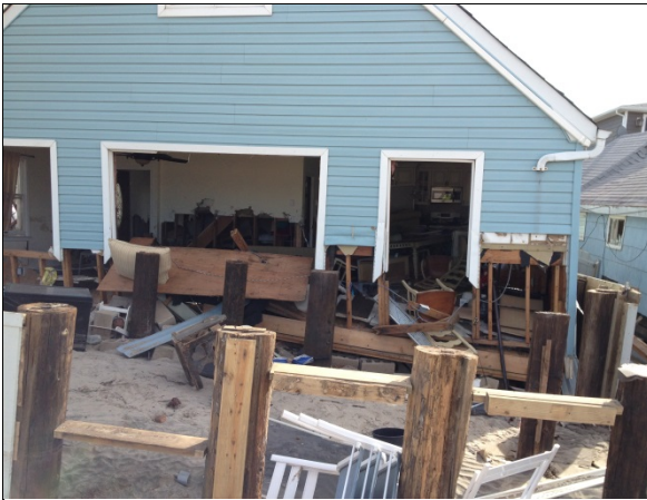
Figure 6.40 House washed off of pile foundations, Breezy Point, Queens (November 5, 2012 – MRCE in collaboration with NYCDOB)
