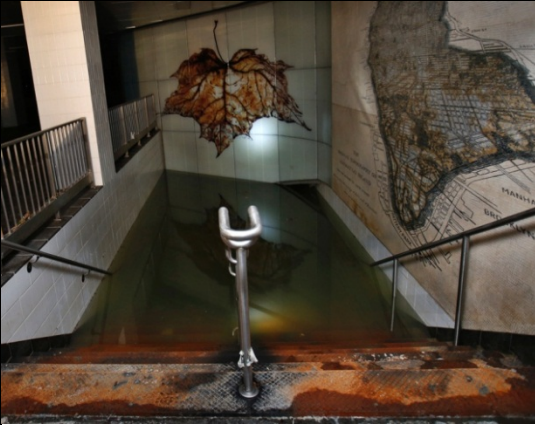
Figure 7.14 Flooding at South Station subway station, Lower Manhattan (Reuters, 10-29-12, Mike Segar).
