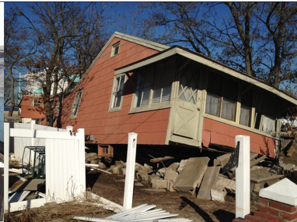
Figure 6.41 Destroyed CMU wall foundation, Breezy Point, Queens (November 5, 2012 – MRCE in collaboration with NYCDOB)
