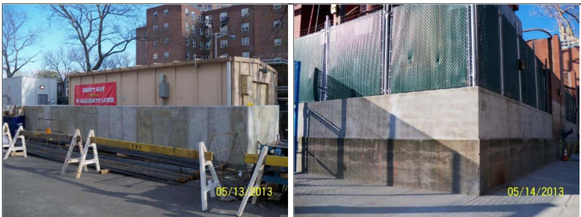
Figure 7.32 Examples of raised walls around critical equipment installed by Consolidated Edison soon after Hurricane Sandy for storm hardening. Photos provided by L. Villani (Consolidated Edison), May 2013.
