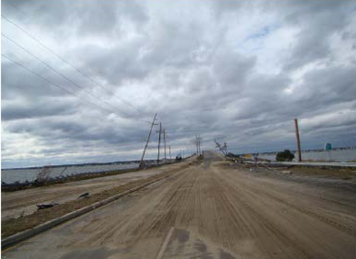
Figure 5.16 Damaged utility poles along eastern approach of Mathis and Tunney Bridges (westbound Route 37) (NJDOT 2012a)
