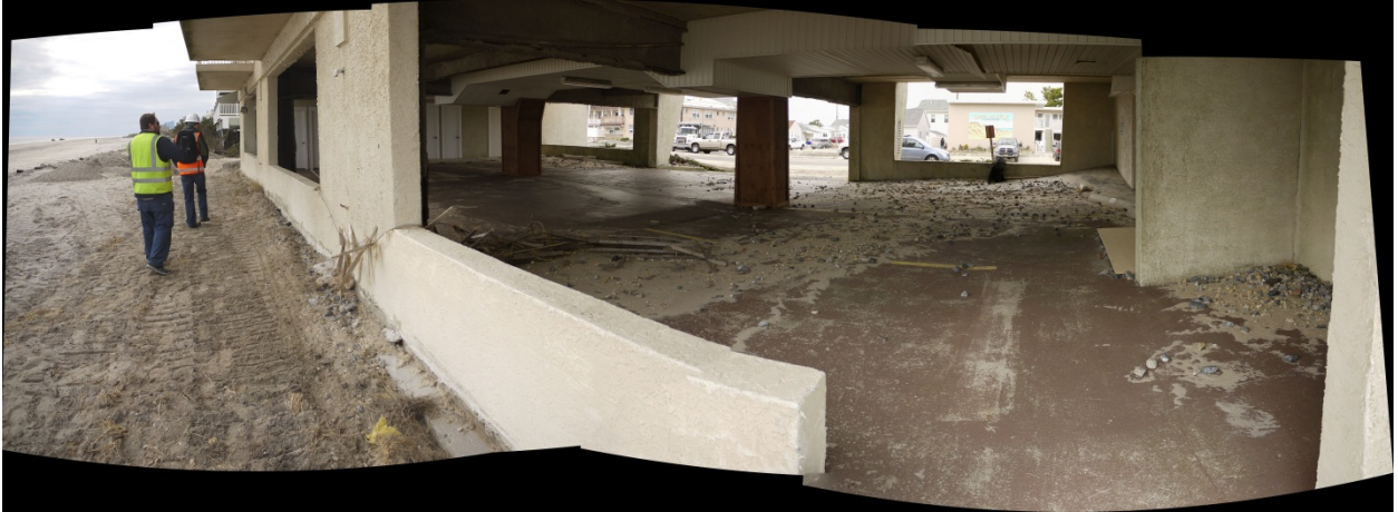
Figure 6.79 Sand deposition in the first floor garage of that same condo (39.41112 ° N, 74.35811 ° W, November 3, 2012)
