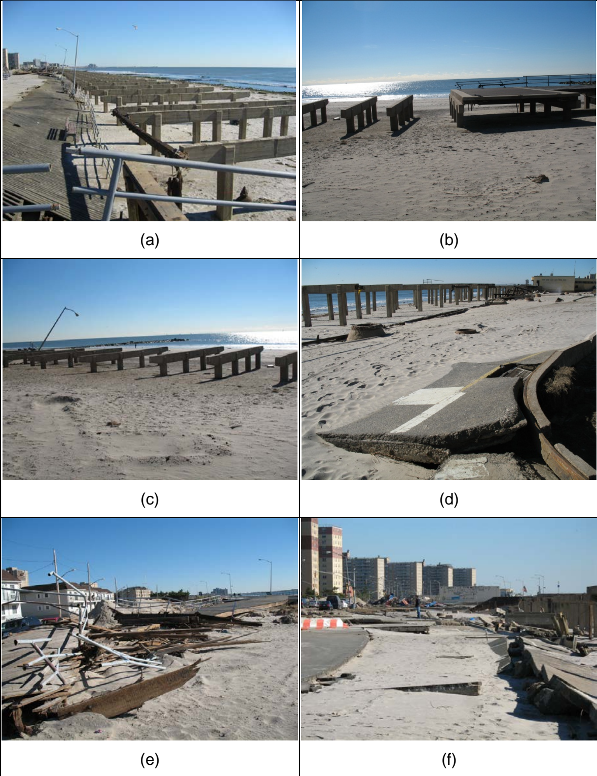
Figure 6.37 Typical damage to boardwalk and shore front road, Beach 95 th Street, Rockaway Beach, Queens (40.583445° N, 73.815529° W, Nov. 4, 2012)
