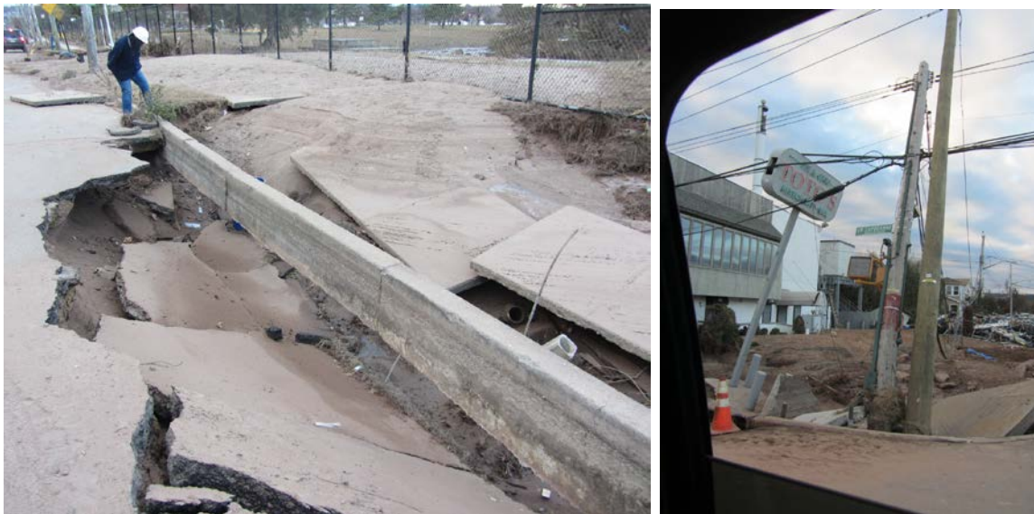
Figure 6.9 Scour undermining street, curb, sidewalk, and utilities, Seaview Blvd and Father Capodanno Blvd, Staten Island (40.579283° N, 74.077849° W, November 4, 2012). GEER team co-leader Dr. Sissy Nikolaou in background.
