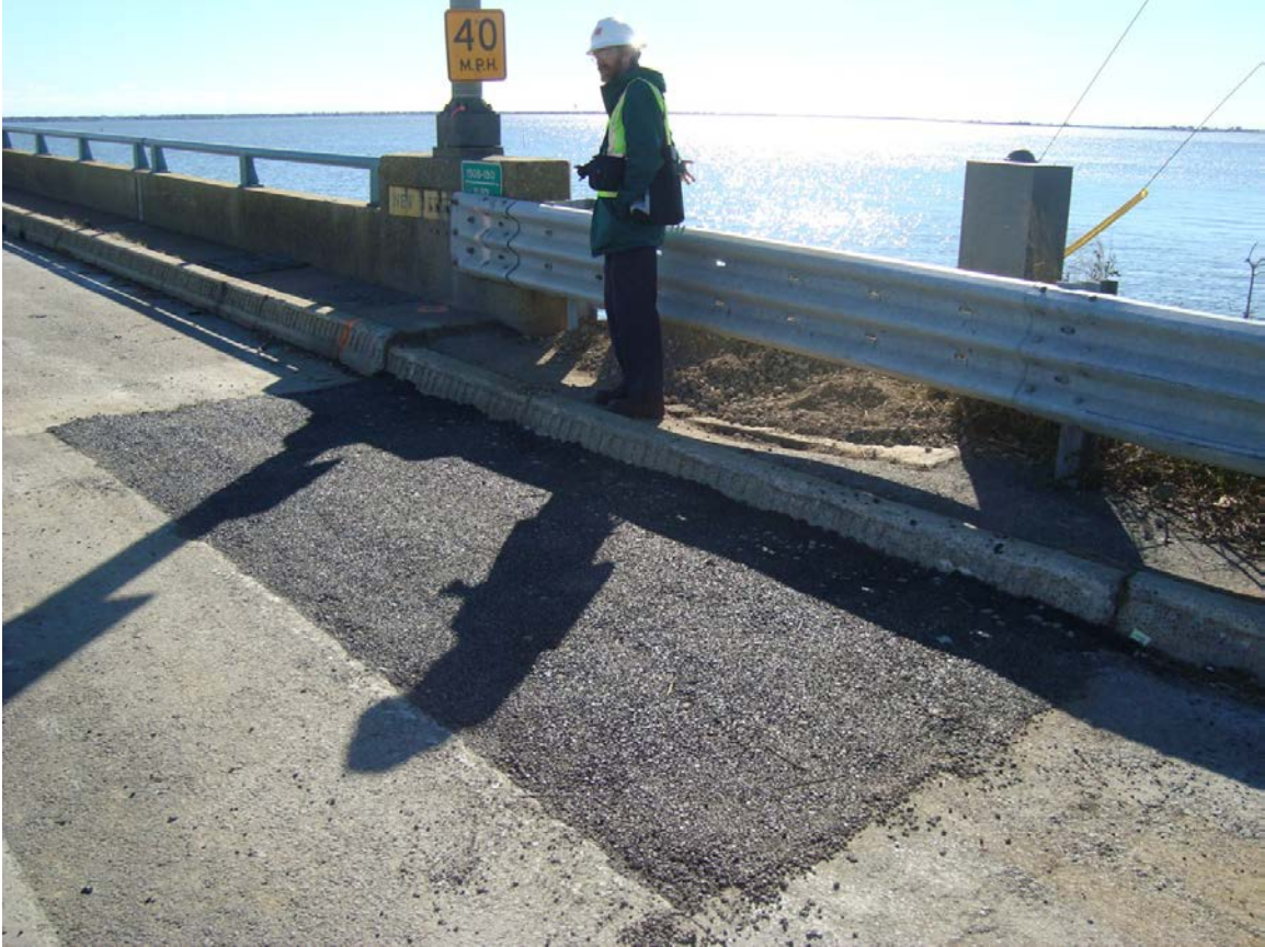
Figure 5.14 Evidence of erosion and recent repair of roadway along the southwest abutment of the Mathis Bridge (eastbound Route 37) 39°56.9610" N, 74° 06.8341 W
