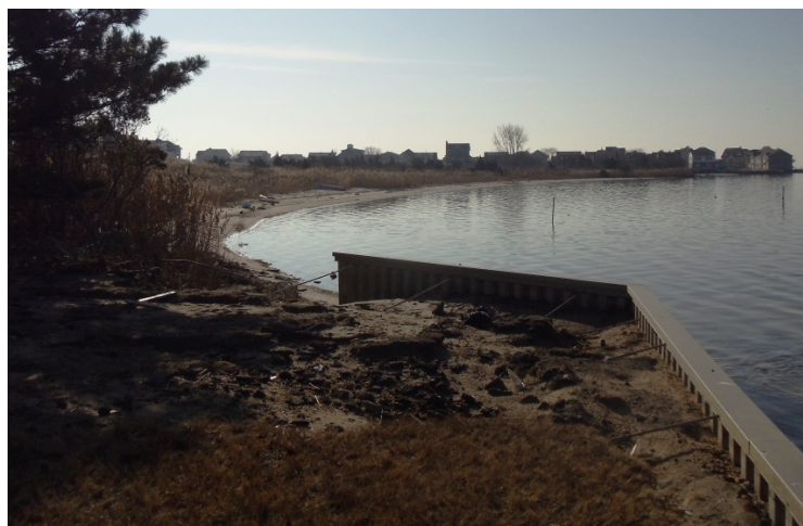
Figure 6.89 Erosion exposing steel tie-back anchors for bulkhead, bayside (39°37'17.62"N, 74°11'55.88"W)
