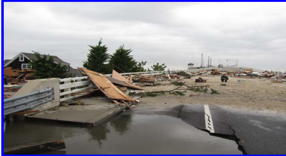
Figure 5.20 Damage to the east abutment of the bridge due to erosion undermining the foundation (40° 2'24.21" N, 74° 3'6.79" W , Ocean County Engineering, 2012)
