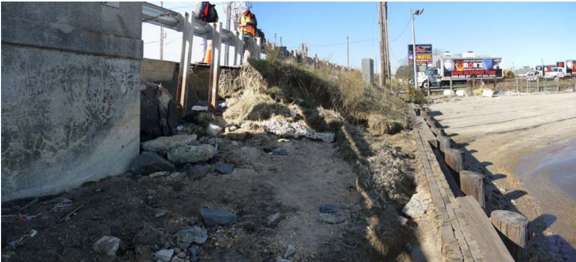
Figure 5.13 Erosion along the northwest abutment of the Tunney Bridge (westbound Route 37) 39° 56.9610" N, 74° 06.8341 W
