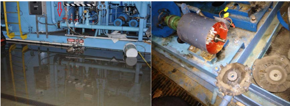
Figure 7.53 Syncon Resins Superfund Site Treatment Plant. Arrow shows high water mark (left). Motor cleaning and drying (right).
