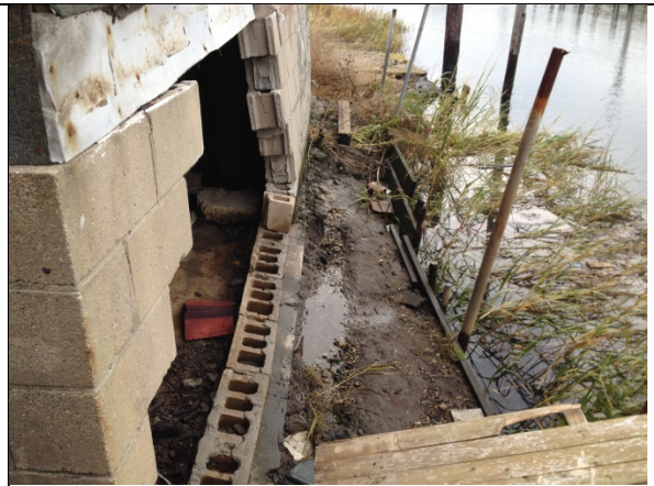
Figure 6.68 Partial collapse of CMU foundation wall, possibly related to erosion at footing, Howard Beach, Queens. (November 16, 2012 – MRCE in collaboration with NYCDOB)
