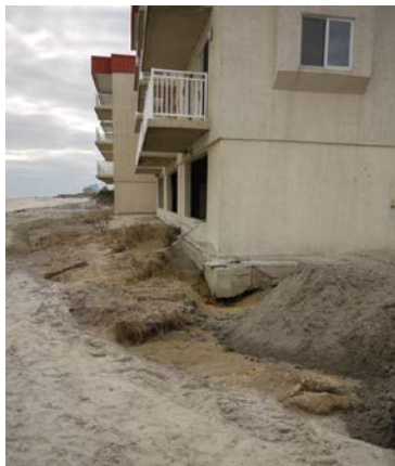
Figure 6.78 Erosion around the foundation of a beachfront condo at a location with little or no barrier dune (39.41112 ° N, 74.35811 ° W, November 3, 2012)
