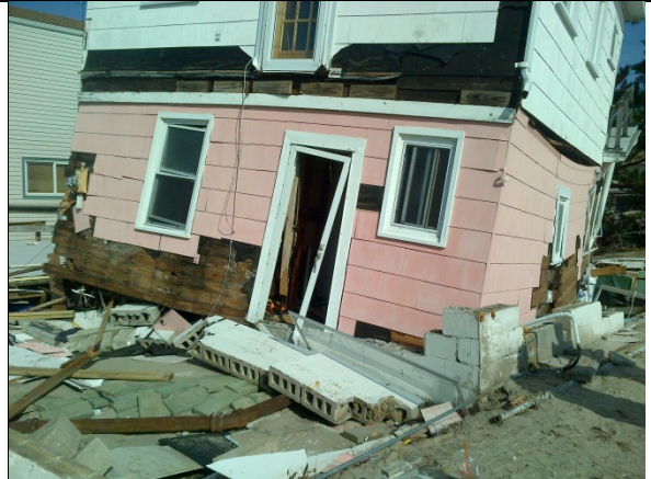
Figure 6.47 Destroyed CMU wall foundation, Breezy Point, Queens (November 12, 2012 – MRCE in collaboration with NYCDOB)
