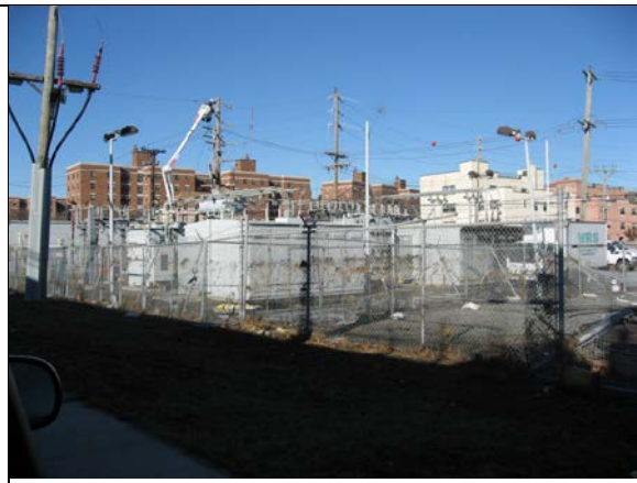
Figure 6.27 Electrical substation at Beach 53 rd Street with high water mark at 4.8 feet on fence, Arverne, Queens (40.592752° N, 73.783396° W, November 4, 2012)
