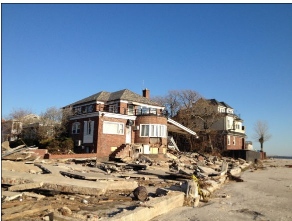
Figure 6.21 Undermining of beachfront retaining wall and loss of retained soil, Sea Gate, Brooklyn (November 9, 2012 – MRCE in collaboration with NYCDOB)
