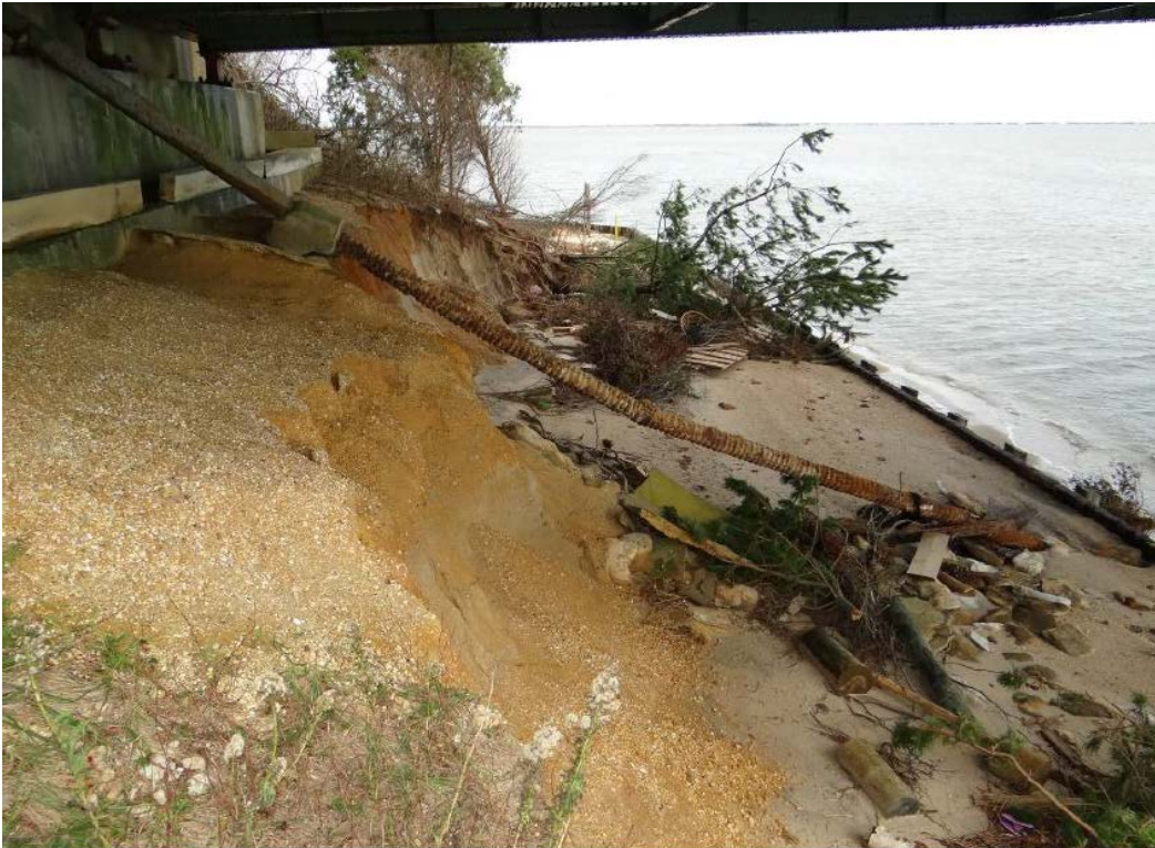
Figure 5.26 Severe erosion observed at the Rt. 72 east abutment, looking north (NJDOT 2012a).
