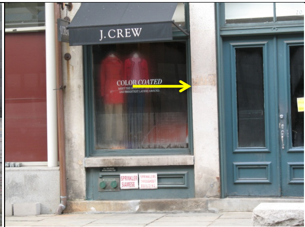
Figure 7.7 High water line at 5.7 feet on storefront window, South Street seaport (40.706935° N, 74.003322° W, November 3, 2012).
