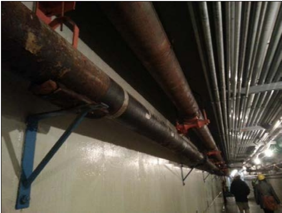
Figure 7.44 Insulated pipes required stripping and re-insulation.
