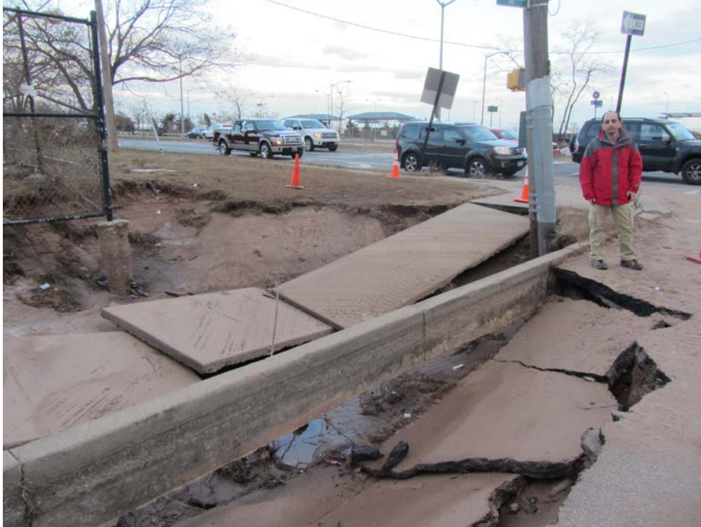
Figure 6.10 Scour undermining overhead power pole and sign, Slater Blvd and Father Capodanno Blvd, Staten Island (40.576173° N, 74.082629° W, Nov. 4, 2012). GEER team co-leader Dr. Youssef Hashash in background.
