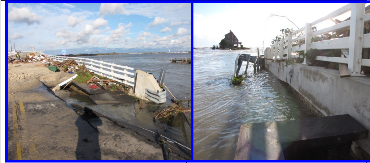
Figure 5.22 Damage to the north side of the east abutment due to erosion caused the T-wall to settle 4 ft (40° 2'24.21" N, 74° 3'6.79" W, Ocean County Engineering, 2012)
