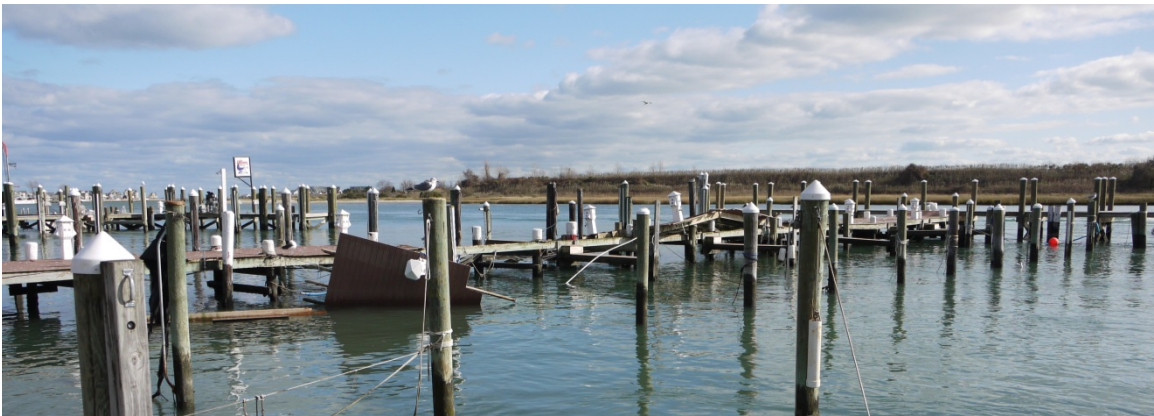
Figure 5.5 Damage to boat piers north of Manasquan River railroad drawbridge (40.10700°N, 74.04998°W, November 5, 2012)
