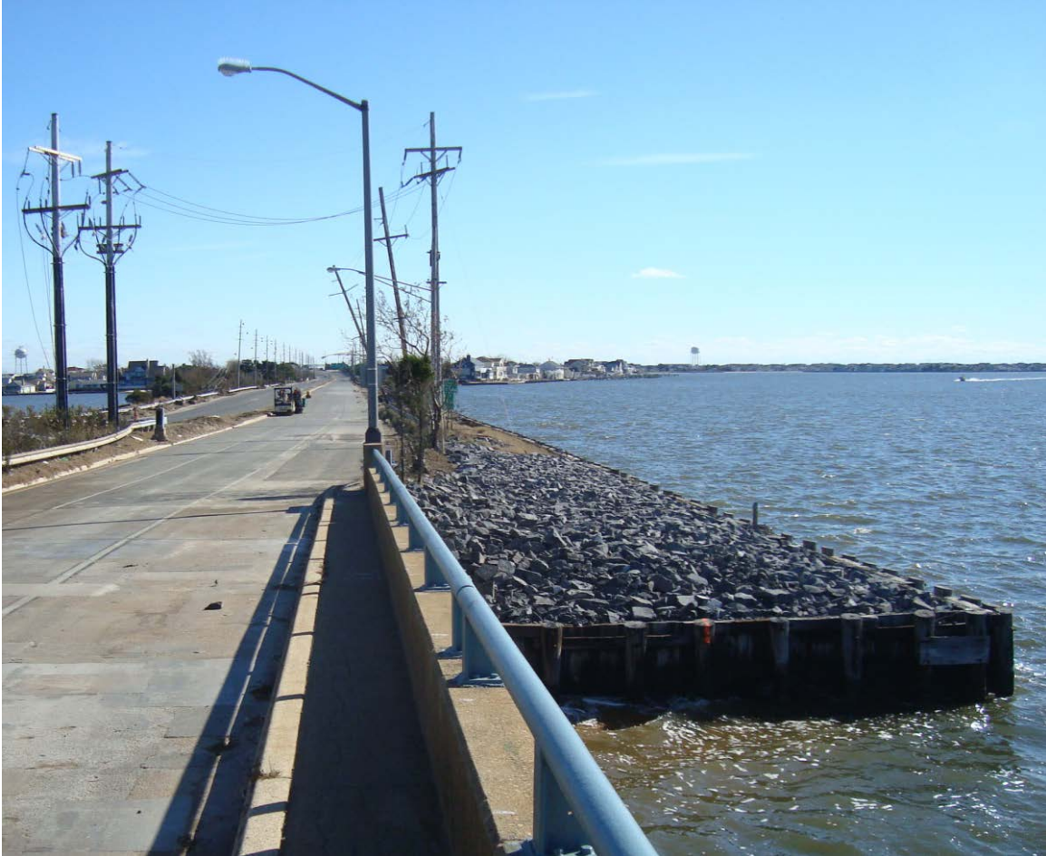
Figure 5.18 Condition of the southeast abutment of Mathis Bridge during the GEER visit (eastbound Route 37)
