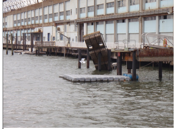
Figure 7.22 Damage to floating dock at Hudson River Park, Pier 40, west side of Manhattan (40.728161° N, 74.011395° W, November 2, 2012).
