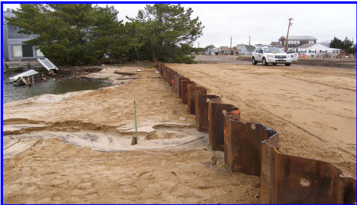
Figure 6.96 Bulkheads and roadway that was washed away at Brinley Avenue, Ortley Beach (39°57'41.63"N, 74° 4'38.29"W, Ocean County Engineering, 2012)
