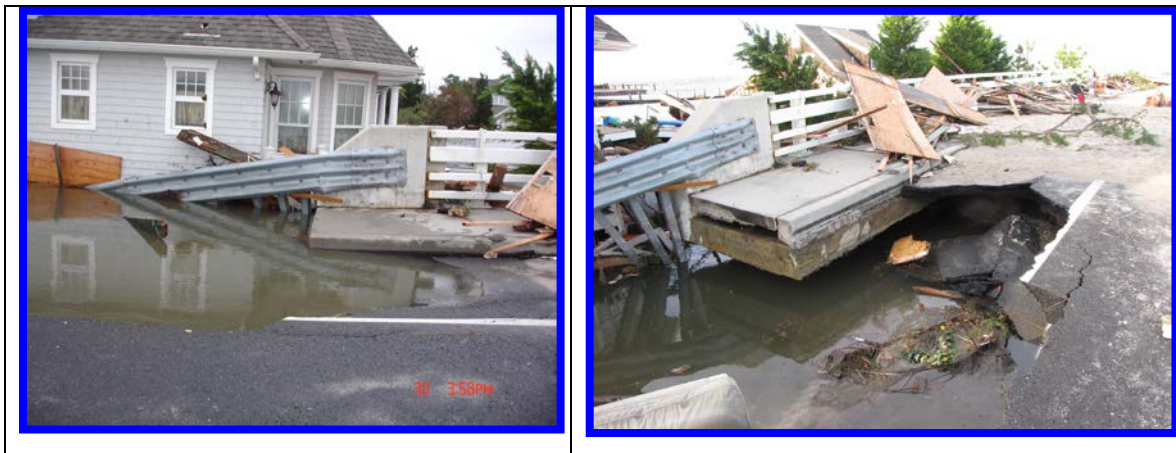
Figure 5.21 Damage to the south side of the east abutment due to erosion and large floating debris such as homes caused the loss of the T-wall, which allowed the coping and sidewalk to be cantilevered out approximately 10 ft (40° 2'24.21" N, 74° 3'6.79" W , Ocean County Engineering, 2012)
