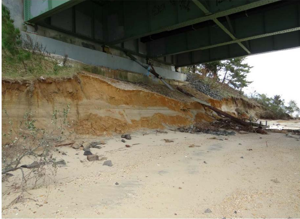
Figure 5.27 Severe erosion observed at Rt. 72 east abutment, looking south-east (NJDOT 2012a).
