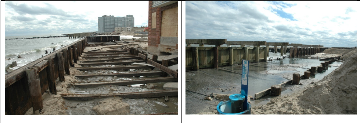
Figure 6.70 The backfill soil had been washed away exposing the severely corroded tie rods.
