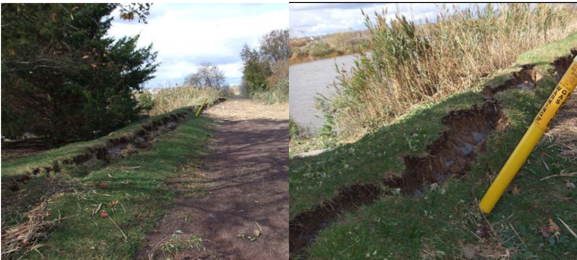
Figure 6.110 Pipeline exposed soon after Hurricane Sandy
