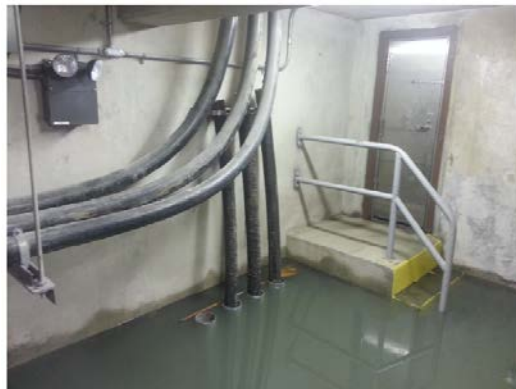
Figure 5.7 Flooding in the submarine cable room of the NJ 35 Manasquan River Draw Bridge (NJDOT, 2012a)
