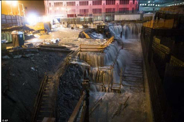
Figure 7.15 Flooding at World Trade Center site, Lower Manhattan (©Associated Press).
