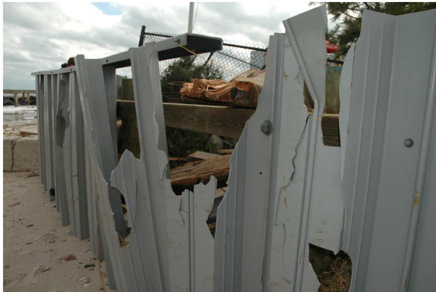
Figure 6.71 Damaged vinyl sheeting surrounding a children's playground.
