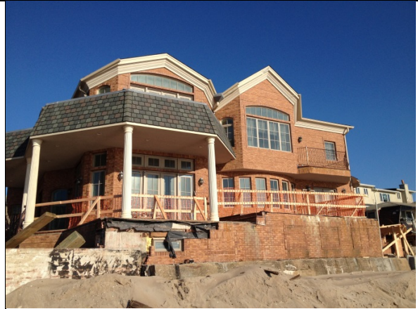
Figure 6.20 Brick veneer building on concrete wall foundation, Sea Gate, Brooklyn (November 9, 2012 – MRCE in collaboration with NYCDOB)
