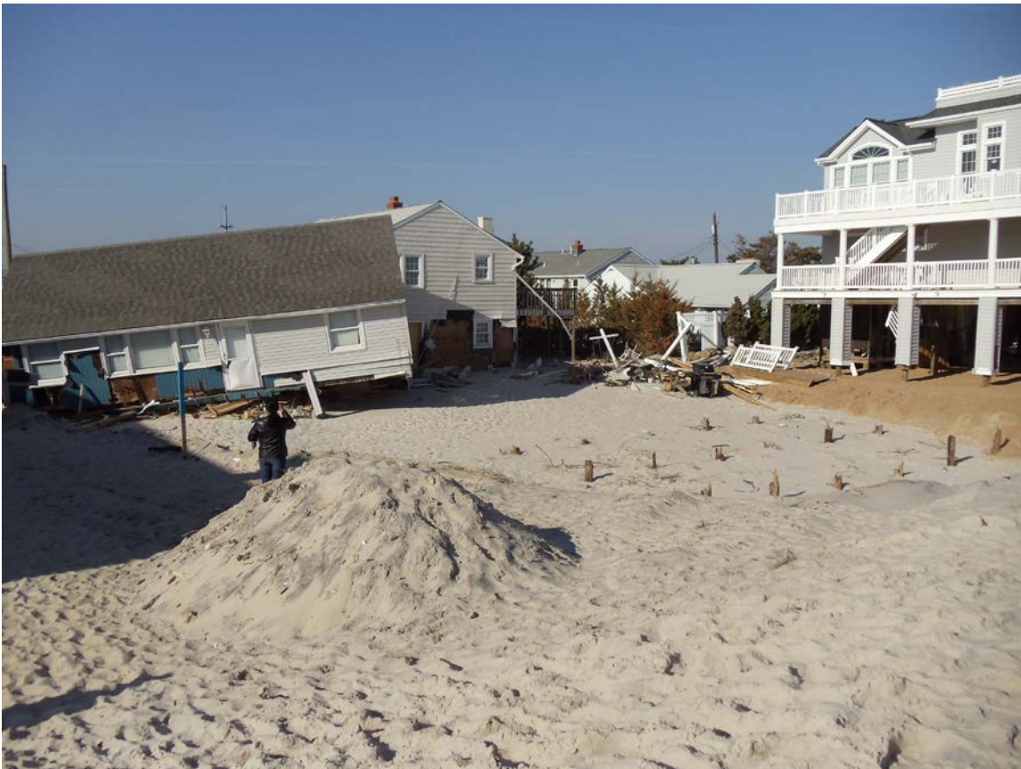
Figure 6.90 Timber pile foundation remains after home was sheared off, ocean-side in Pehola Park (39.610016, -74.206657)
