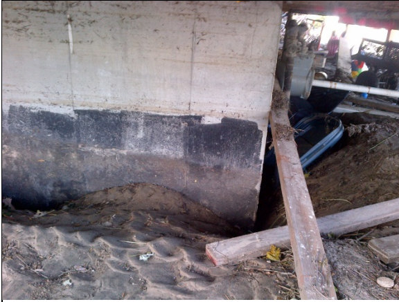
Figure 6.46 Scour and erosion at concrete wall foundation, Breezy Point, Queens (November 5, 2012 – MRCE in collaboration with NYCDOB)
