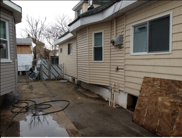
Figure 6.65 Typical home with flooding damage, Howard Beach, Queens. (November 16, 2012 – MRCE in collaboration with NYCDOB)
