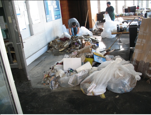
Figure 7.5 Flood damage, Pier 11 water taxi terminal (40.703277° N, 74.006237° W, November 3, 2012)
