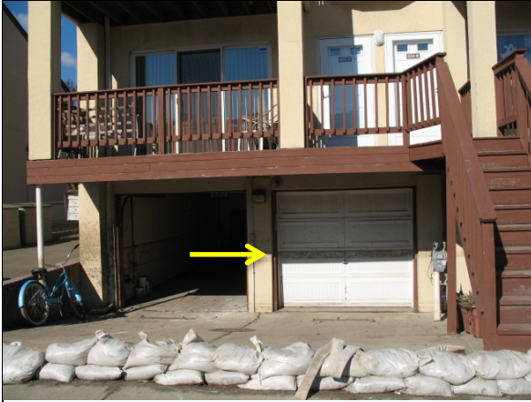
Figure 6.56 Sandbags and high water mark on garage door, East Broadway, Long Beach (40.584989 °N, 73.644769 °W, November 4, 2012)
