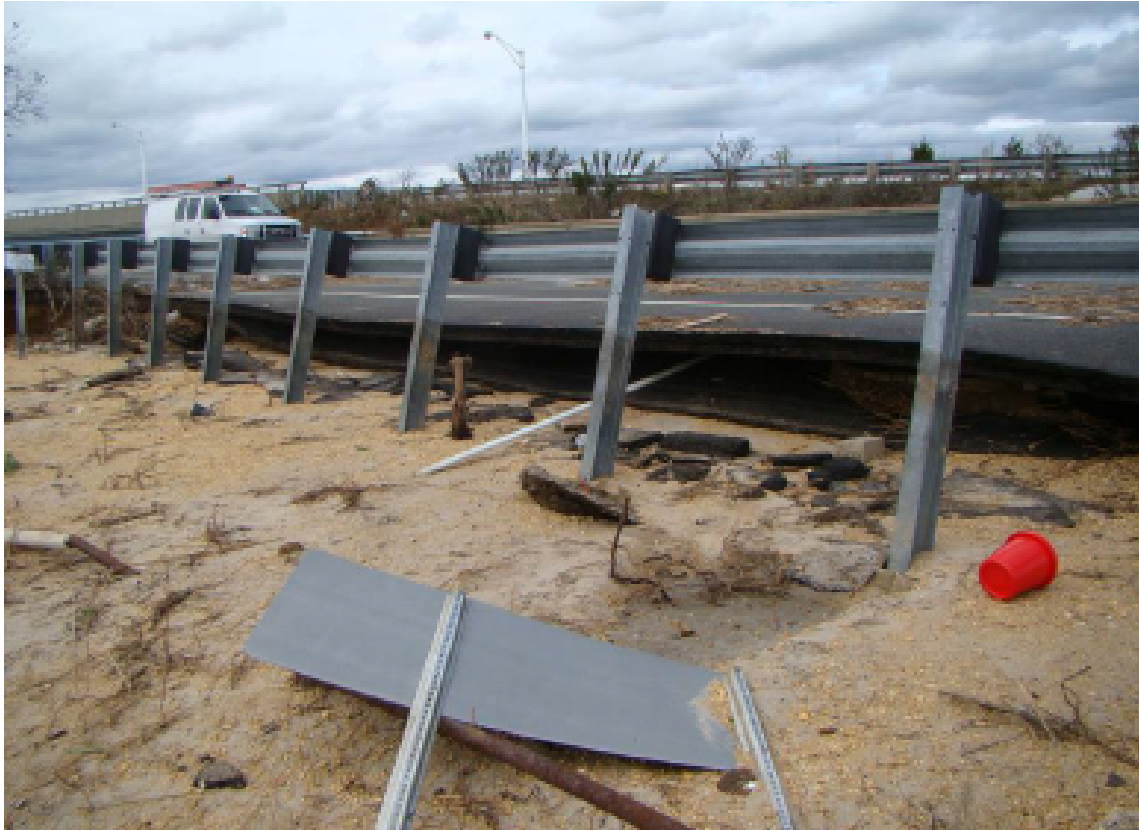
Figure 5.17 Erosion of embankment and roadway along southeast approach of Mathis Bridge (looking northwest) (NJDOT 2012a)
