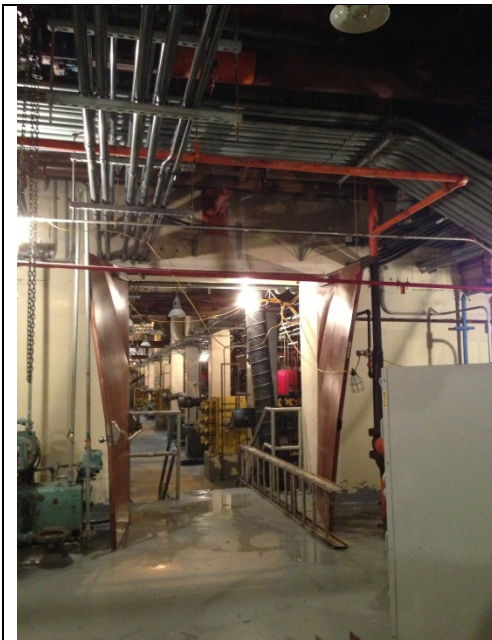
Figure 7.42 Steel doors twisted open by flood water.
