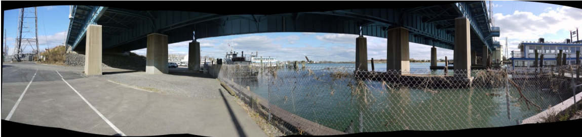
Figure 5.6 North abutment of Route 35 draw bridge over Manasquan River. Note possible high water debris in fence. (40.10495°N, 74.05422°W, November 5, 2012)
