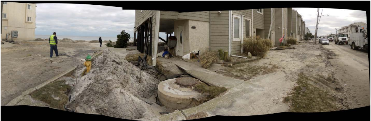
Figure 6.80 Erosion around utilities on landside of beachfront structures, again at a location with no barrier dune (39.41081 ° N, 74.35887 ° W, November 3, 2012)
