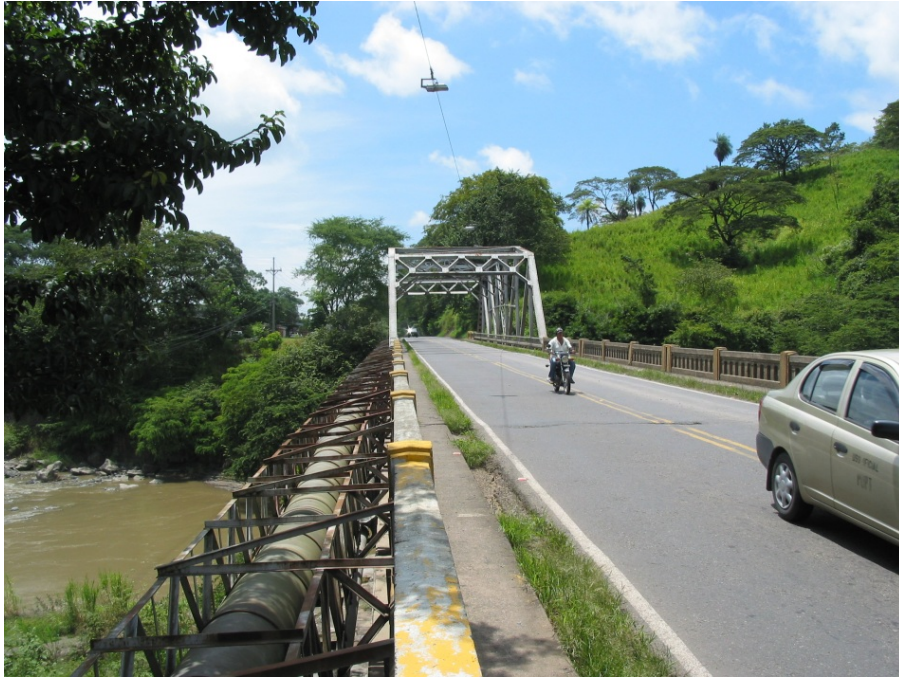
Fig. 4.5 - Crooked water pipe adjacent to the south side of the bridge (9.99705° N 84.69412° W).
