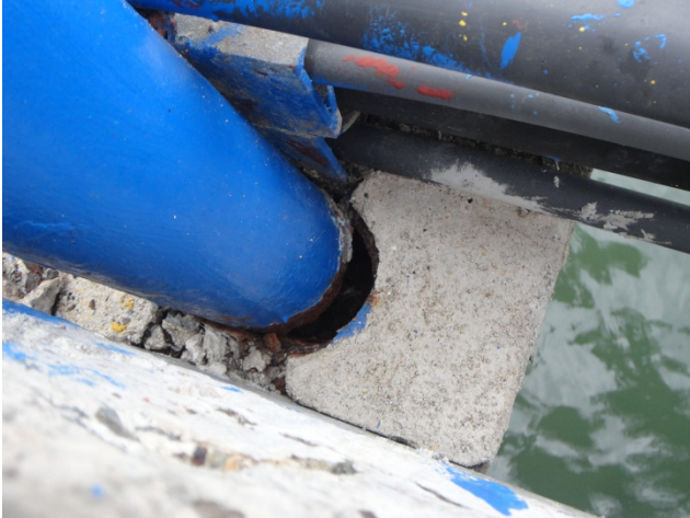
Fig. 3.10 - Damaged connection between a guardrail post and the pier (9.97213° N 84.83079° W).
