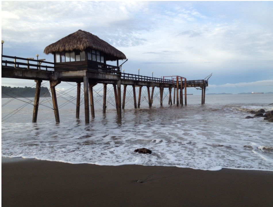
Fig. 3.15 - Pier with additional support piles to stabilize the pier during repairs. (9.96812° N 84.74150° W).
