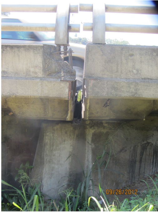
Fig. 4.14 - Possible evidence of pounding beneath the guardrail at the west abutment (10.00193° N 84.31131° W).
