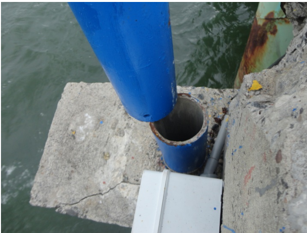
Fig. 3.11 - Sheared weld on a damaged guardrail post. Similar damage was observed on nearly every post (9.97214° N 84.83070° W).
