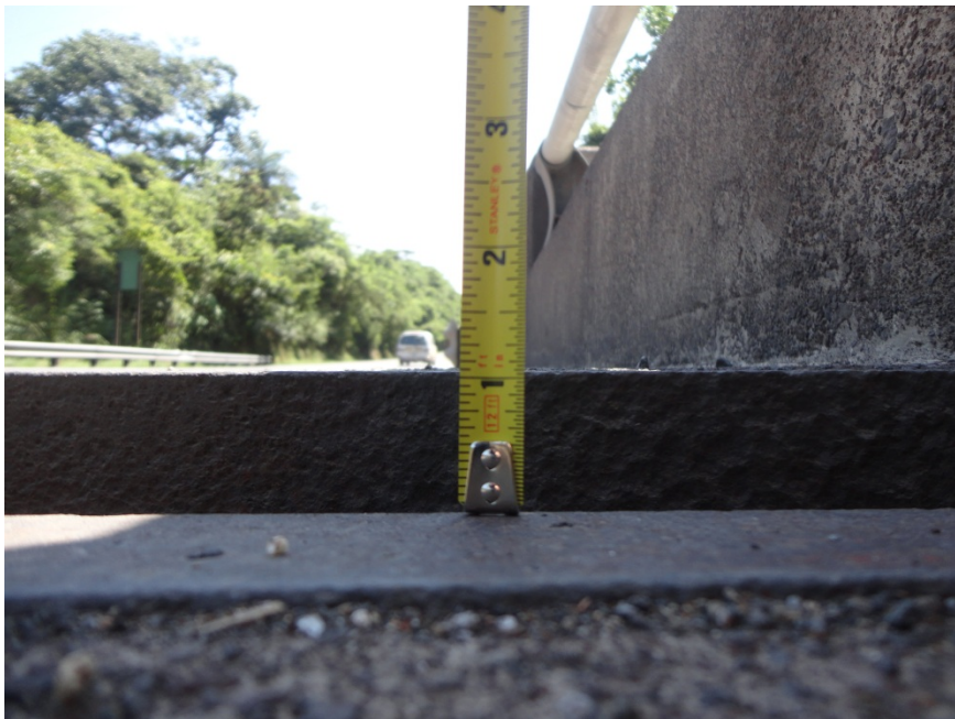
Fig. 4.13 - Vertical offset of about 25 mm (1 inch) at the east abutment.
