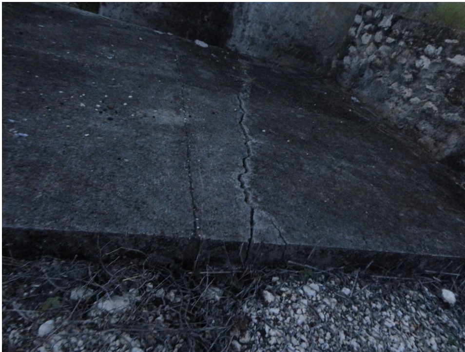
Fig. 4.20 - Transverse crack observed across the abutment slab at the east abutment (10.24889° N 85.24262° W).
