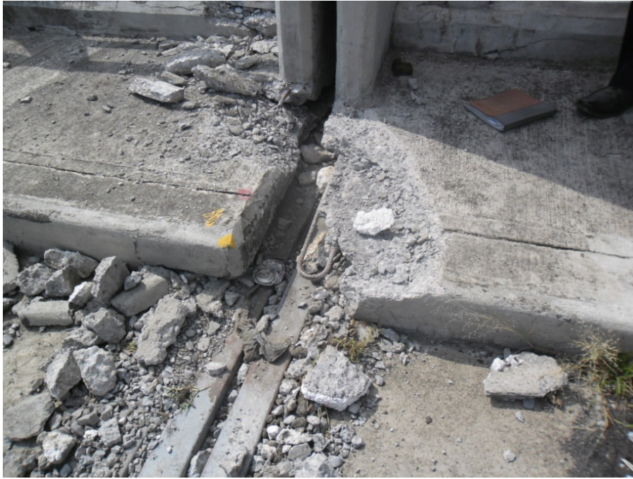
Fig. 4.17 - Spalled concrete and exposed rebar due to pounding between the cable-stayed bridge and the box girder bridge (courtesy of the Costa Rica Ministry of Transportation) (10.24678° N 85.24685° W).
