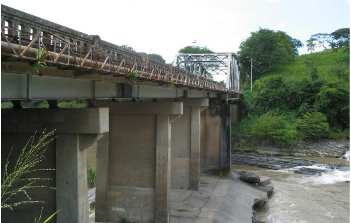
Fig. 4.1 - Photo taken of the Rio Barranca Bridge near the east abutment (9.99717° N 84.69409° W).
