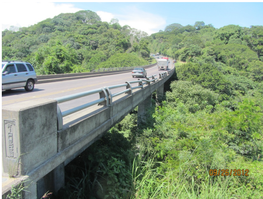
Fig. 4.9 - Photo taken of the Poas River Bridge adjacent to the east abutment (10.00238° N 84.31026° W)
