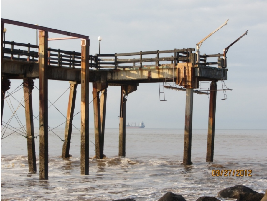
Fig. 3.14 - Failure of the pile to deck connection at four piles near end of pier. (9.96779° N 84.74181° W).
