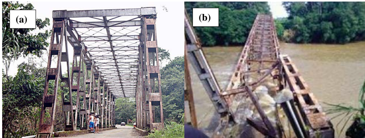
Fig. 4.28 – Photographs in the longitudinal direction of the De Hierro Sobre bridge over the Sarapiquí river (a) before and (b) after the earthquake. The bridge collapsed into the river during the earthquake despite relatively low acceleration level. (photos courtesy of Yamil Herrera ) (10.39000° N 84.13736° W)
