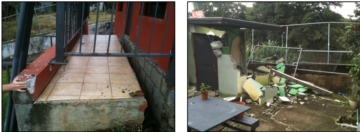
Fig. 5.5 – Structures became inhabitable. (a) Rear access porch became detached from structure, no apparent structural tie of porch to structure; (b) The shear displacement near retaining wall caused masonry construction to collapse in back patio of lower house.
