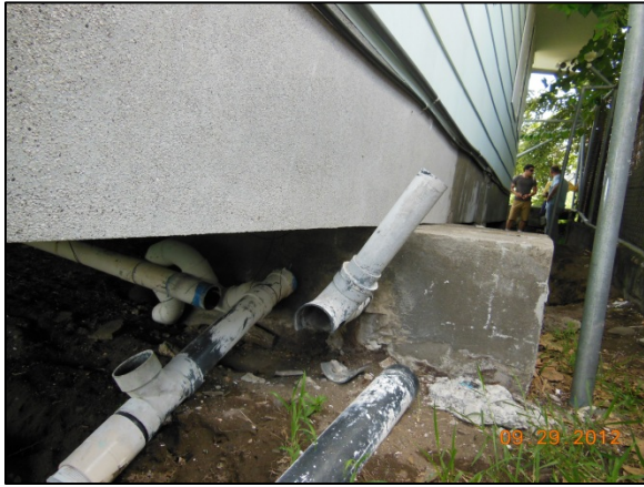
Damaged water and sewer utilities that served the Capitanía building office.
