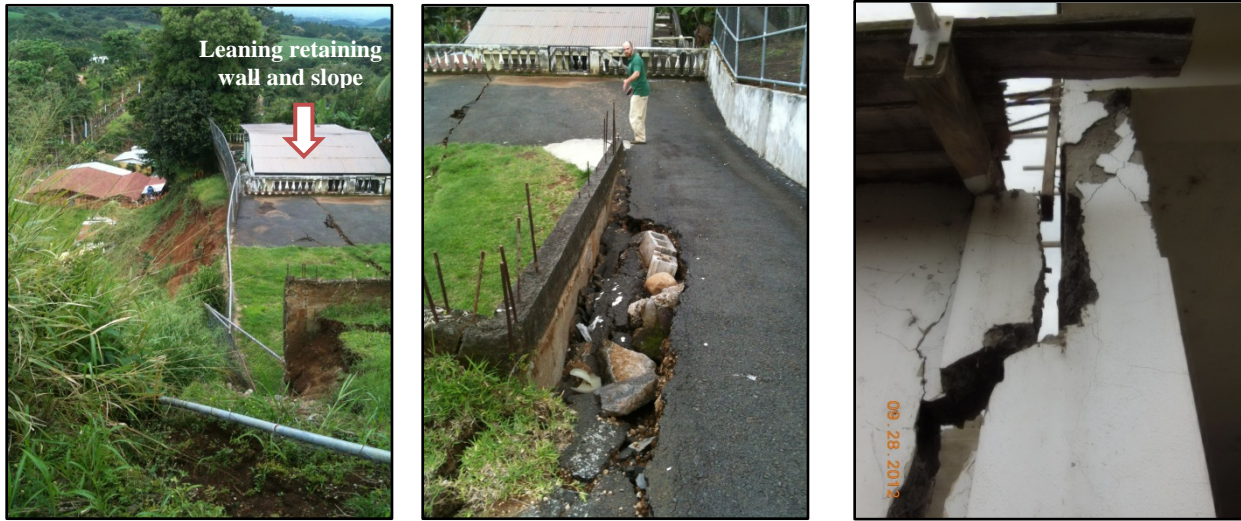
Fig. 5.4 – Construction near steep slopes: retaining walls and slope failure (a) Leaning retaining wall and large deformations caused evacuations; (b) Large crack openings parallel to the alignment of wall, (c) detached stairwell of structure built near a slope, minor reinforcement.
