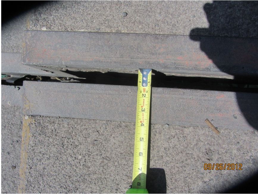
Fig. 4.12 - Longitudinal offset of about 25 mm (1 inch) at the east abutment (10.00231° N 84.31025° W).
