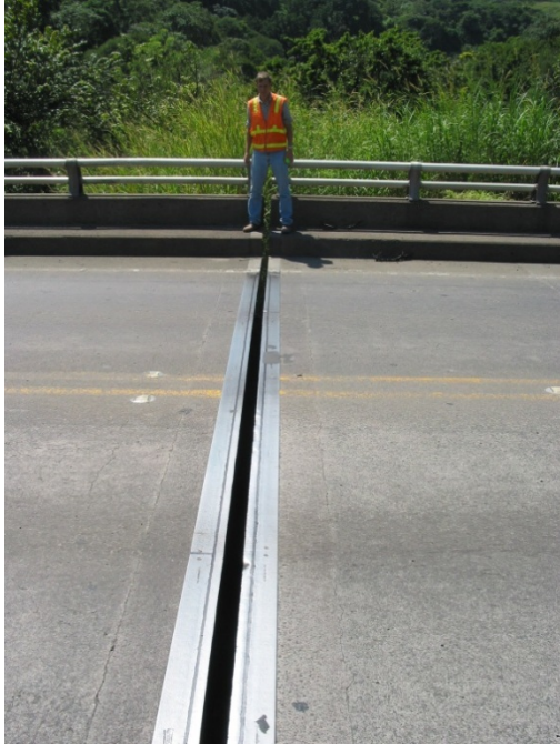
Fig. 4.10 - Longitudinal offset at the west abutment (10.00188° N 84.31129° W).
