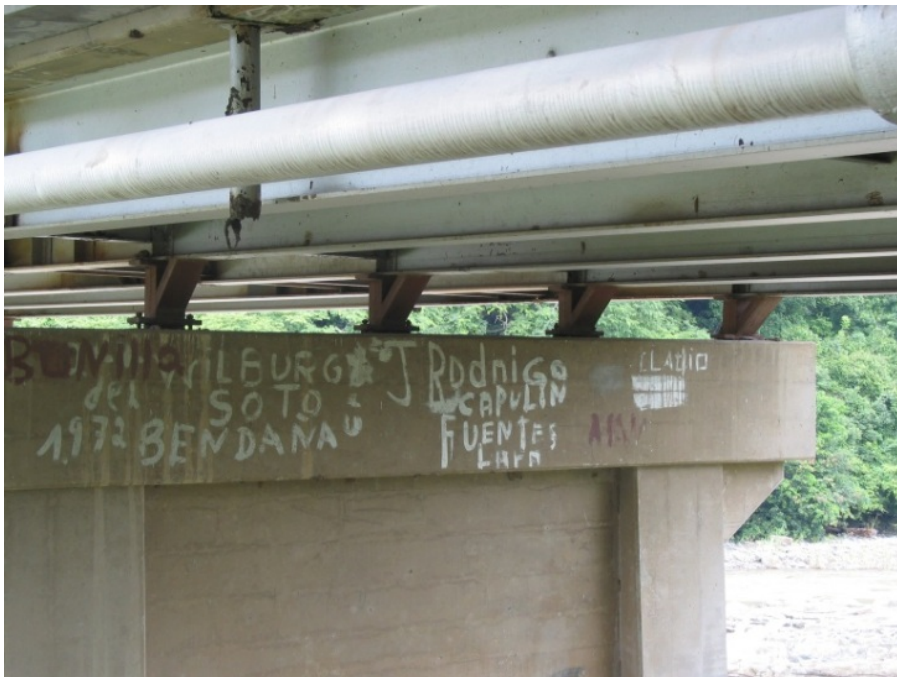
Fig.4.4 - Pull-out of the connections between the deck and the bent on the southern half of the bridge (9.99706° N 84.69436° W).
