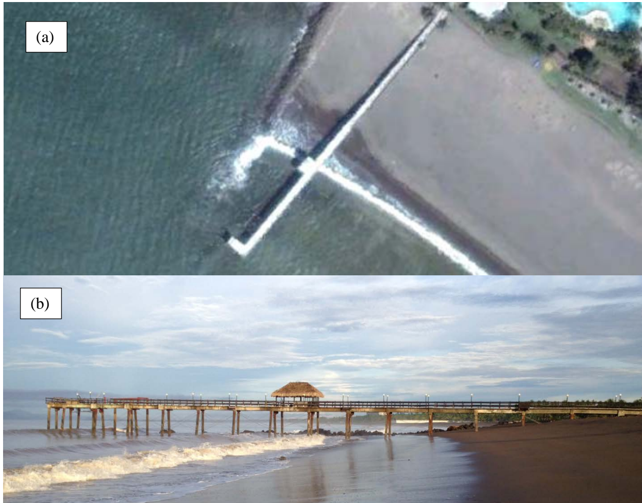
Fig. 3.13 - (a) Plan (Google Earth) and (b) elevation views of the damaged pier at Doubletree hotel in Puntarenas
