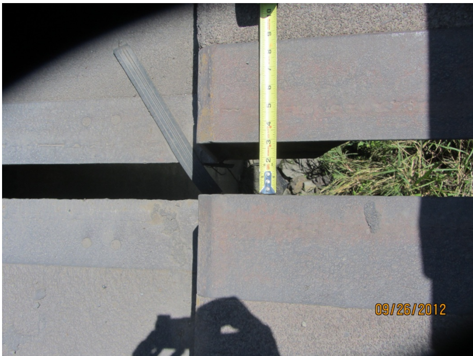
Fig. 4.11 - Longitudinal offset of about 76 mm (3 inches) at the west abutment.
