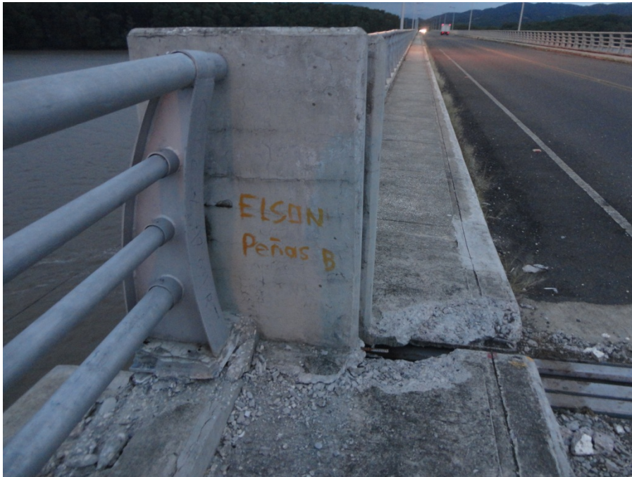
Fig. 4.18 - Evidence of pounding observed by the reconnaissance team at the joint between the box girder section and the cable-stayed section of the bridge (10.24678° N 85.24685° W).
