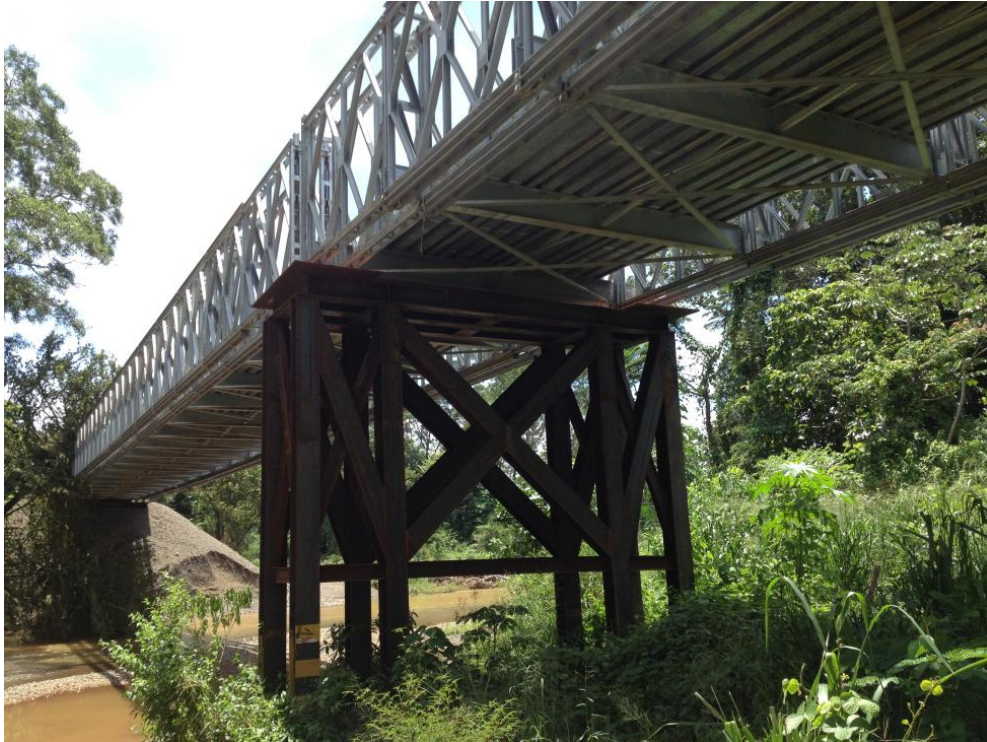
Fig. 4.29 Single span steel bridge in Nosara which performed without damage despite peak ground accelerations of 1.38g in the vicinity owing to the proximity to the fault rupture. Pile foundations at the abutment were in the same configuration as for this central pier.
