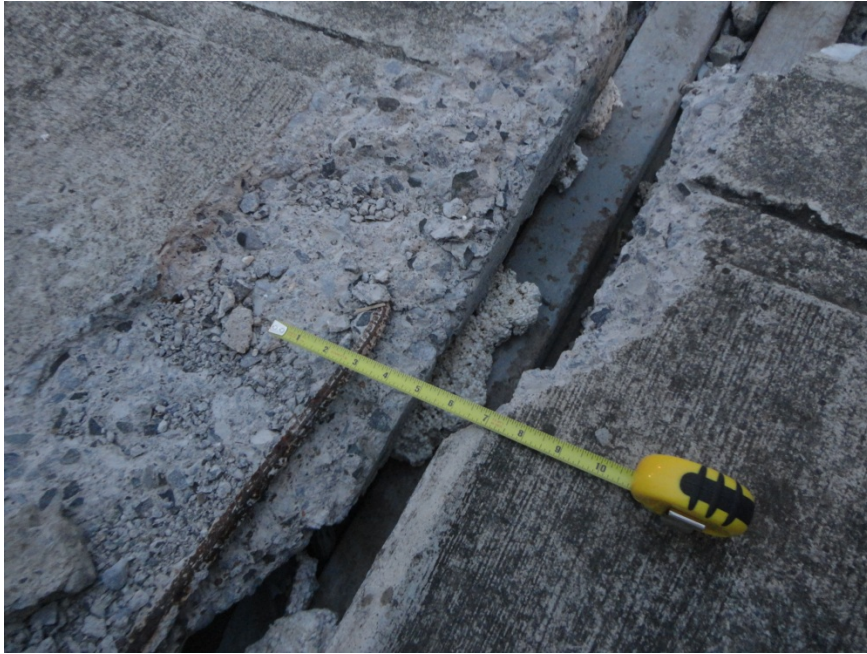
Fig. 4.19 - Gap of approximately 25 mm (1 inch) between the box girder and cable-stayed sections (10.24670° N 85.24682° W).
