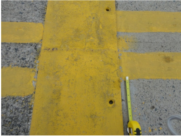
Fig. 3.7 - Lateral offset between the pile- and caisson-supported sections of the pier (9.97177° N 84.83068° W).
