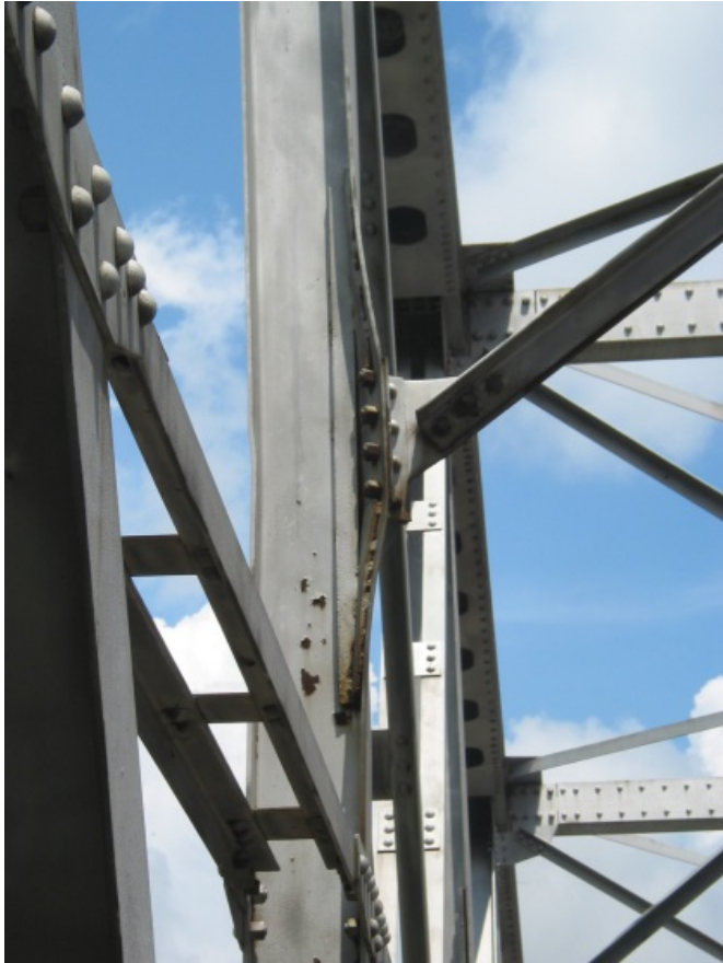
Fig.4.3 - Torsional buckling in certain members of the truss bridge (9.99704° N 84.69480° W).
