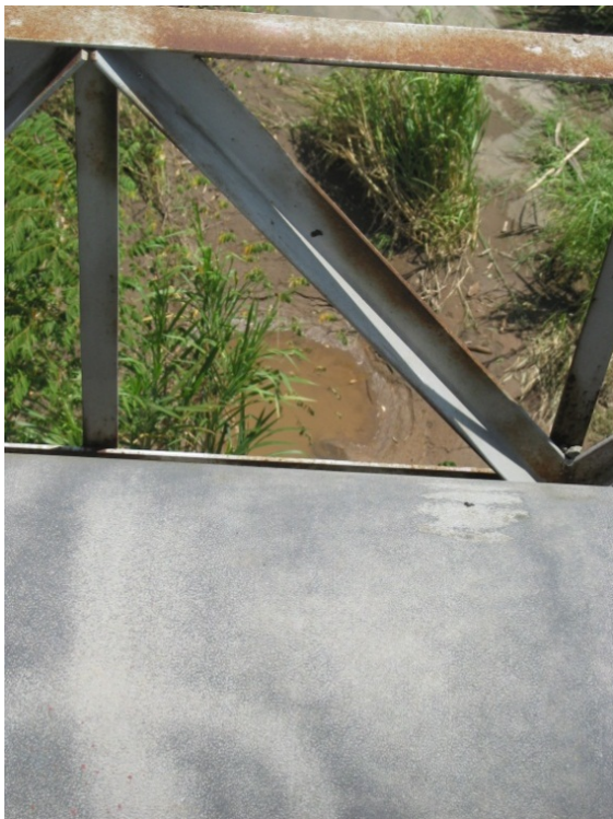
Fig. 4.6 - Evidence of a subsided sand boil due to liquefaction (9.99688° N 84.69438° W).
