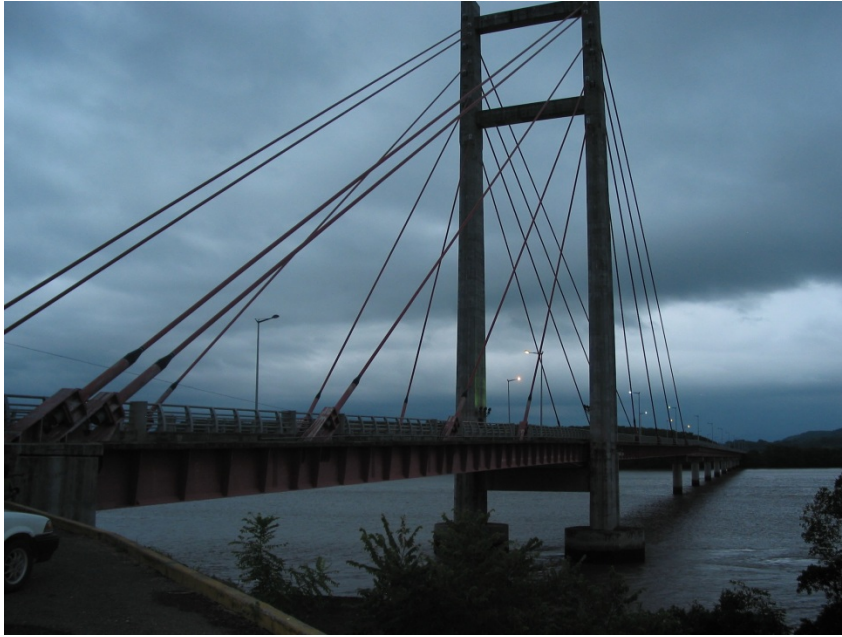
Fig. 4.16 - Photo of the bridge over the Rio Tempisque taken during our reconnaissance from near the west abutment (10.24555° N 85.24895° W).
