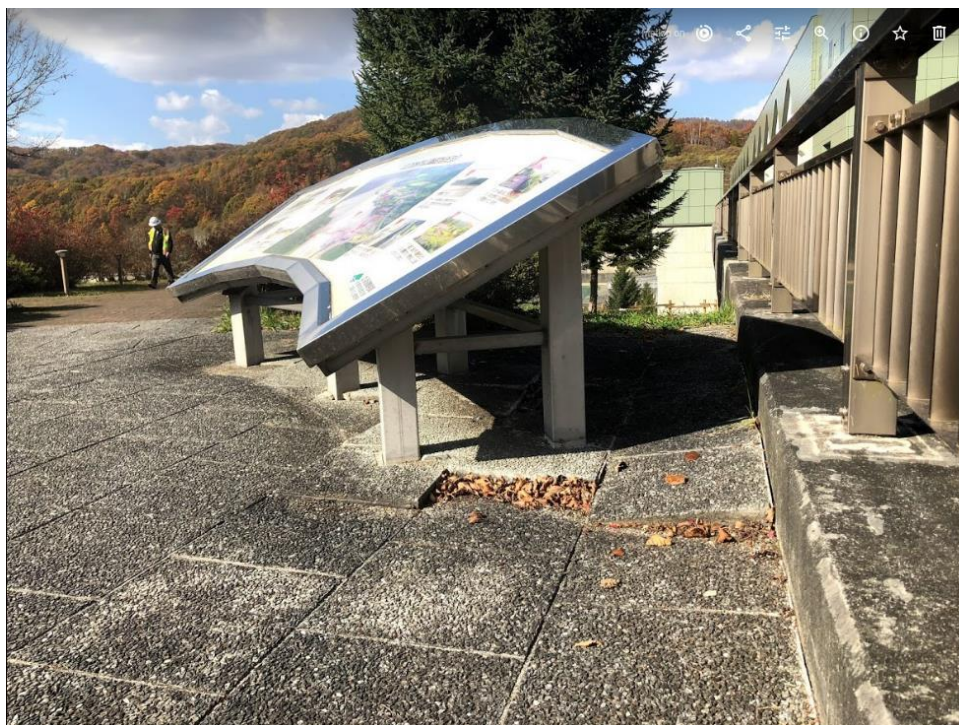
Figure 7-17. Differential settlement of the fill area 42.629302, 142.148654
