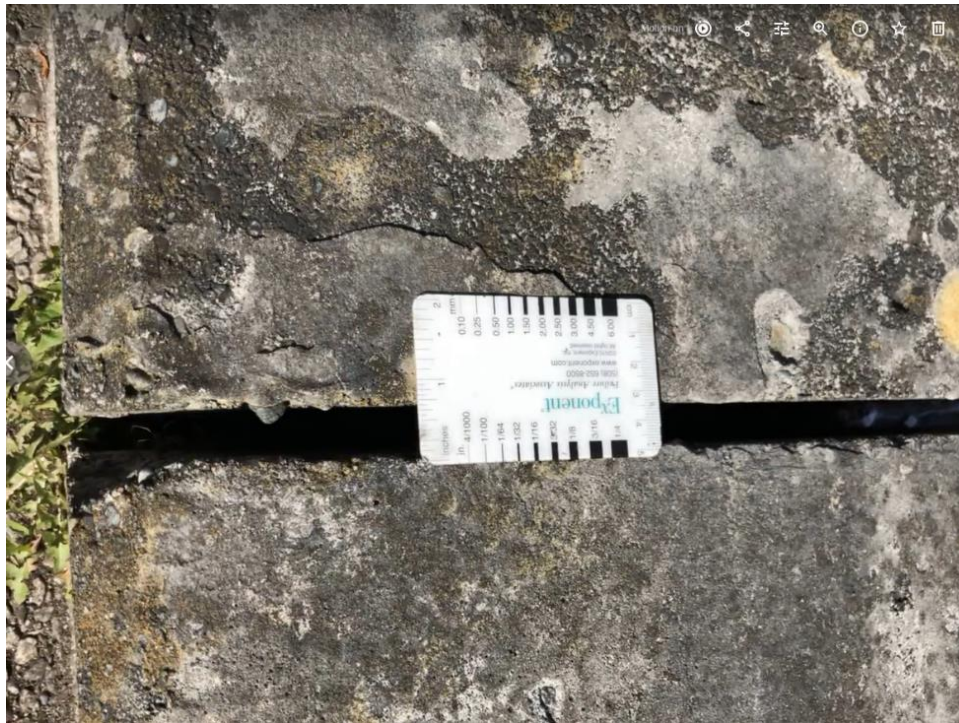
Figure 7-18. Separation of the concrete pavement 42.629302, 142.148654
