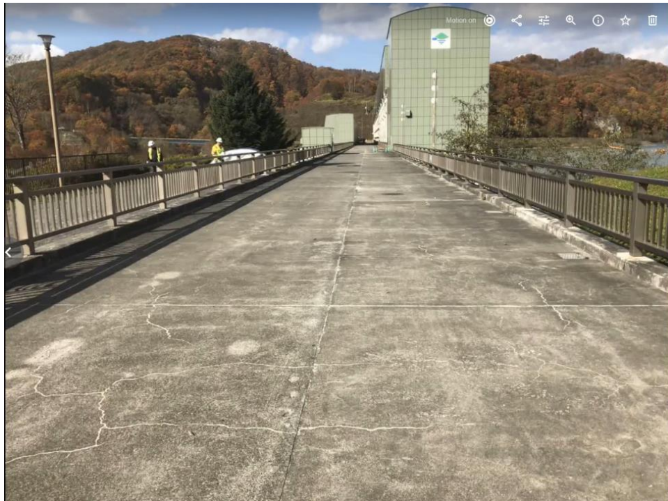
Figure 7-16. No damage to the deep foundation support bridge deck connect to the gates 42.629302, 142.148654
