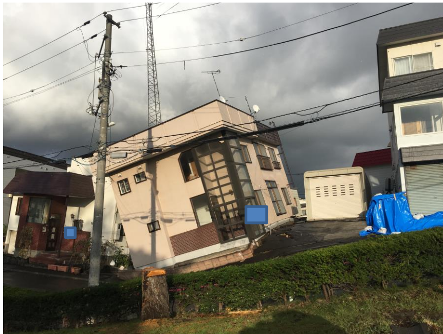
Figure 6-11. Significant rotation of a residential structure due to flow-failure-induced differential settlement
