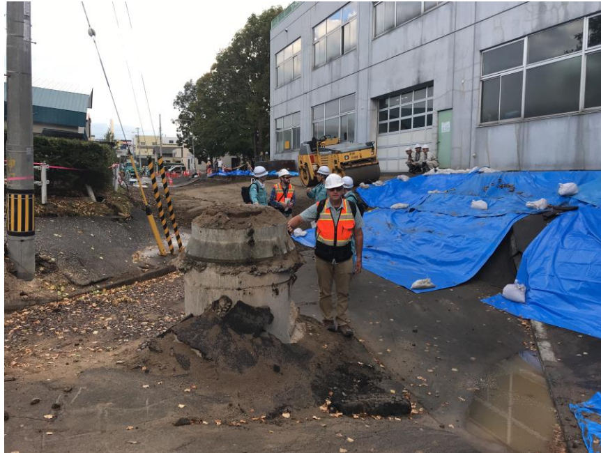
Figure 6-12. Manhole, founded on native non-liquefiable material at 10m depth. Surrounding pumice fill evacuated during flow-failure leading to significant vertical deformation shown here.
