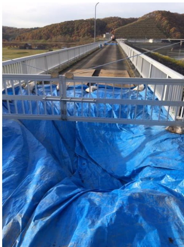
Figure 7-21. Sink hole near abutment bridge contact 42.629302, 142.148654
