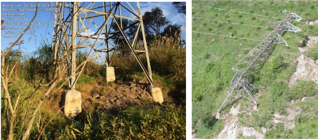
Figure 8-2. Electric power tower (a) at top of translational slide (Cow Slide) with no observable damage to foundation elements. Settlements at concrete footings range from 20-40 cm. (b) collapsed Iwachishi Line (66 kV) (November, 1, 2018 HEPCO report)
