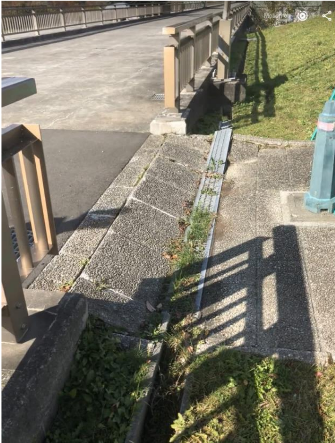
Figure 7-15. Differential settlement of bridge approach and adjacent fill area 42.629302, 142.148654
