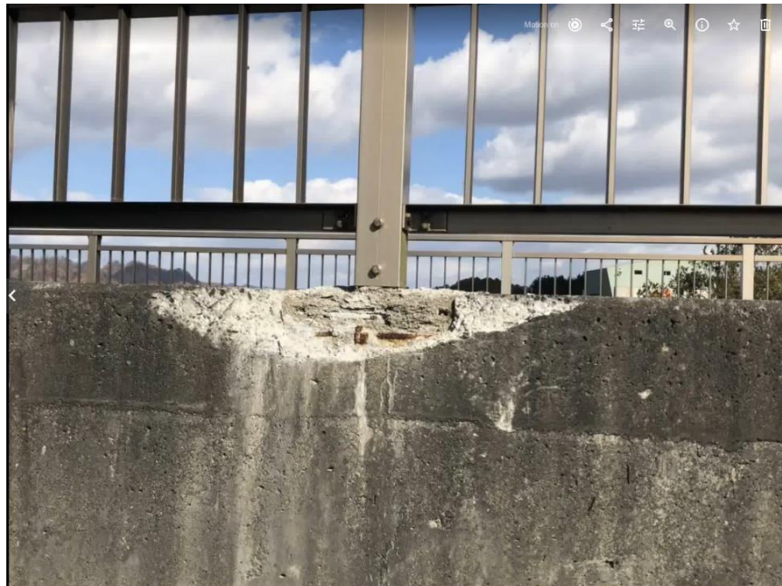
Figure 7-20. Damage of hand rail 42.629302, 142.148654
