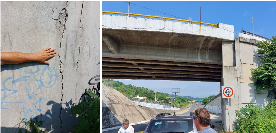
Figure 31. Vertical cracking in abutment of bridge, Boca de Iguanas, Jalisco. Waypoint Station 6 (Coordinates: 19.125082^\circ , -104.407973^\circ )
