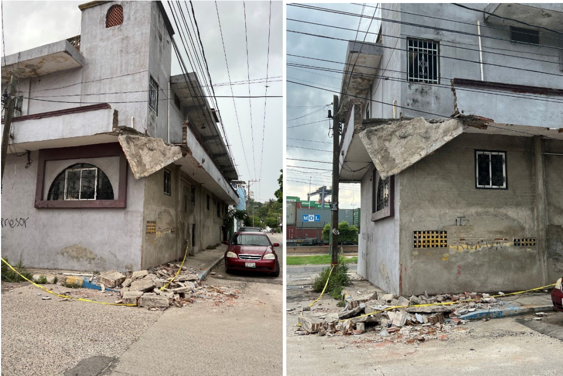
Figure 11. Partial collapse of balcony, Manzanillo, Colima Waypoint Station 9 (Coordinates: 19.058136°, -104.290446°)
