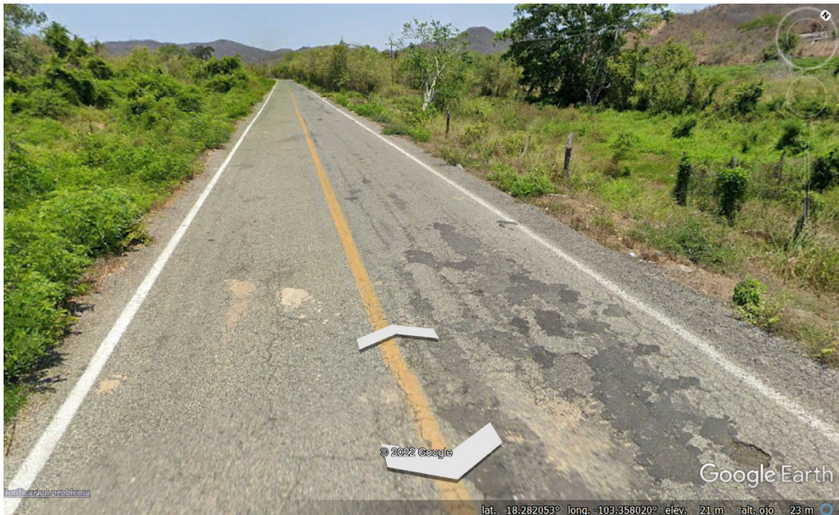
Figure 28a. Road before the earthquake, (Google Earth, image date: May 2022). (Coordinates: 18.282195°, -103.358294°)
