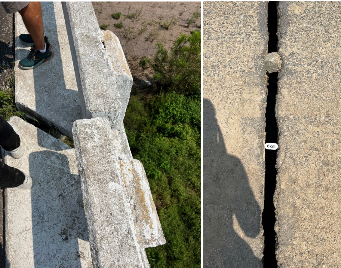
Figure 29. Gap of joints in decks of the bridge and lateral displacements, Campo Acosta, Jalisco.
