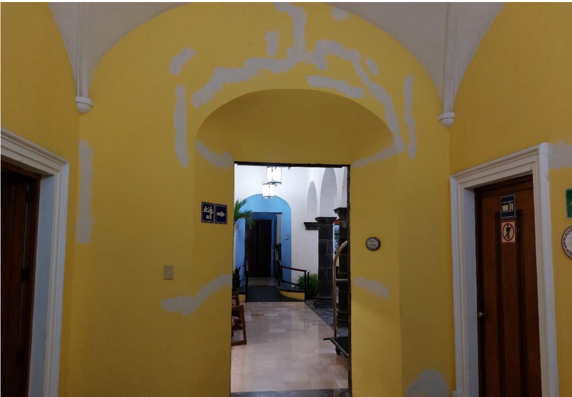
Figure 22. Damage and slight cracking in non-structural elements of multiple buildings in the center of the city, Colima, Colima. Waypoint Station 30 (Coordinates: 19.243584°, -103.728062°)
