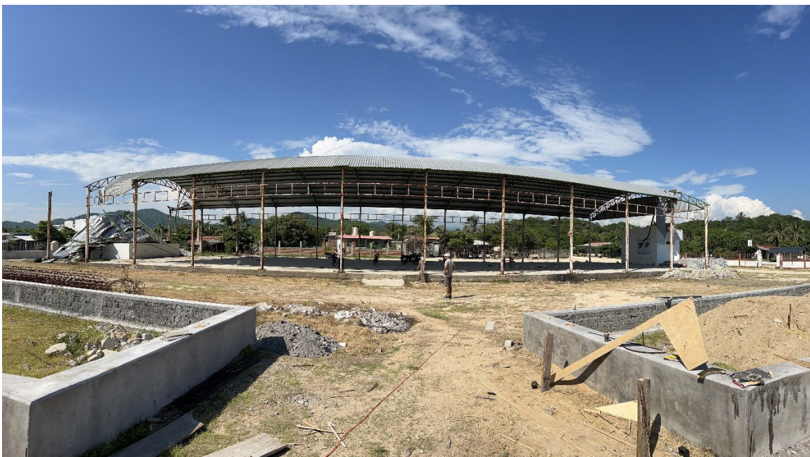
Figure 20. Partial collapse of a court cover roof. Structure had evidence of severe rust, Colola, Michoacan. Waypoint Station 26 (Coordinates: 18.298116°, -103.412856°)
