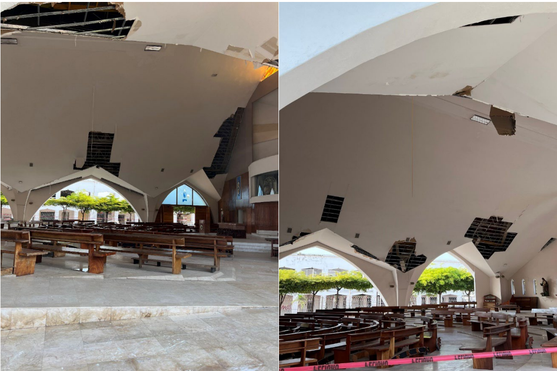
Figure 18. Damage to nonstructural elements in church, Tecoman, Colima Waypoint Station 16 (Coordinates: 18.910498°, -103.87244°)
