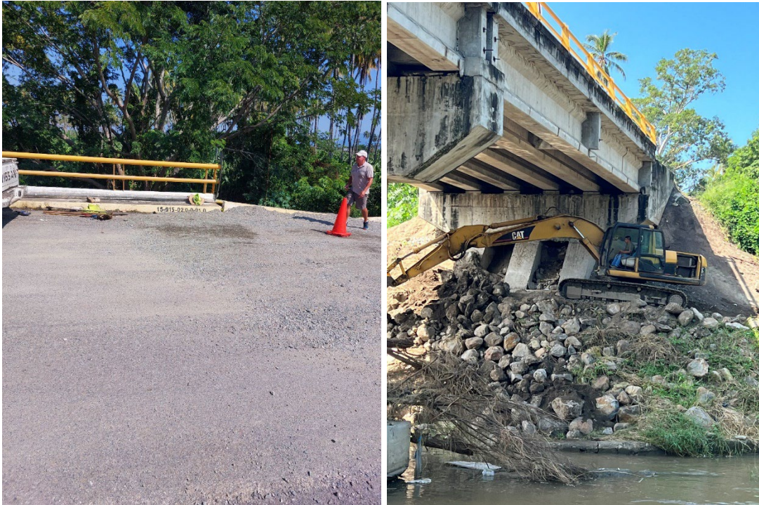
Figure 33. Lateral displacements of decks with damage in pier caps of the bridge and rotational failure of abutment, El Ticuiz, Michoacan. Waypoint Station 19 (Coordinates: 18.670031°, -103.681472°)
