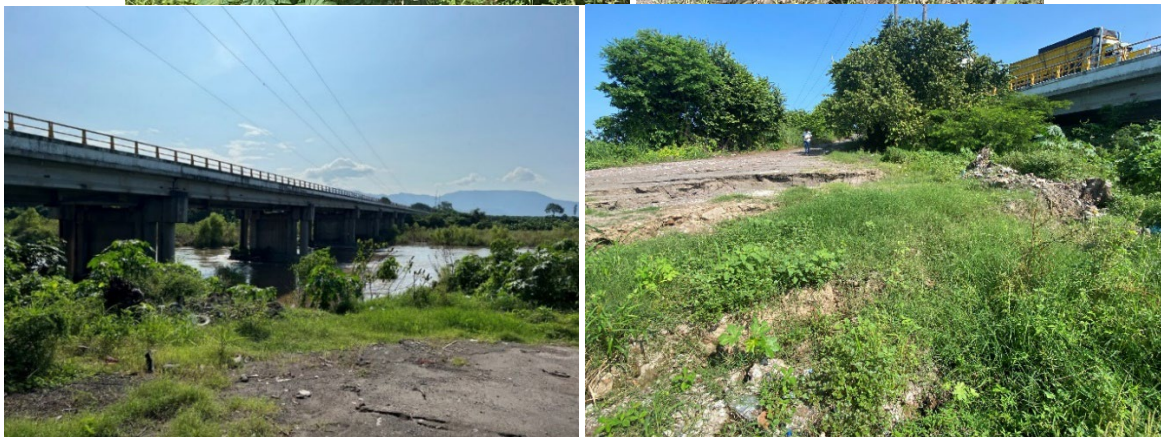
Figure 41. Lateral spread feature affecting a road along a natural levee, La Zapotera, Colima. Waypoint Station 18 (Coordinates: 18.717472°, -103.716876°)
