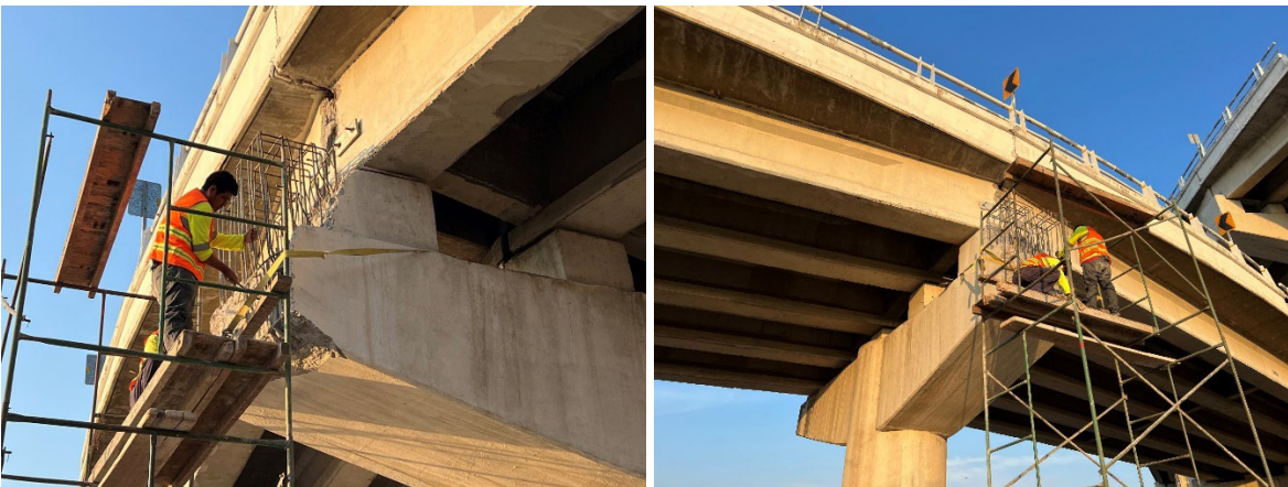
Figure 34. Lateral displacements of decks and damage in pier caps of bridge, Colima, Colima. Waypoint Station 31 (Coordinates: 19.213032°, -103.739473°)
