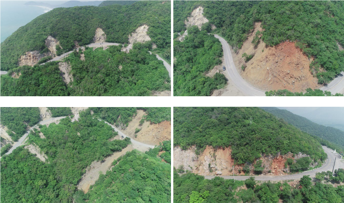
Figure 38. Multiple rockfalls and landslides on cutting slopes along the road, Las Brisas, Michoacan. Waypoint Station 23 (Coordinates: 18.566463°, -103.65394°)
