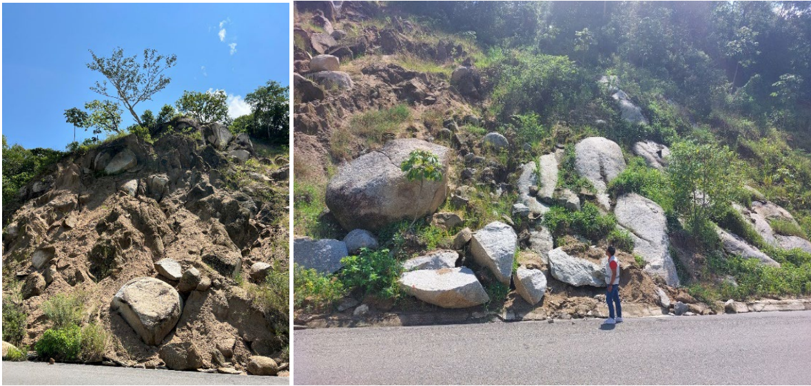
Figure 36. Rockfalls on cutting slope along the road, El Cono, Jalisco. Waypoint Station 1 (Coordinates: 20.240086°, -105.320644°)
