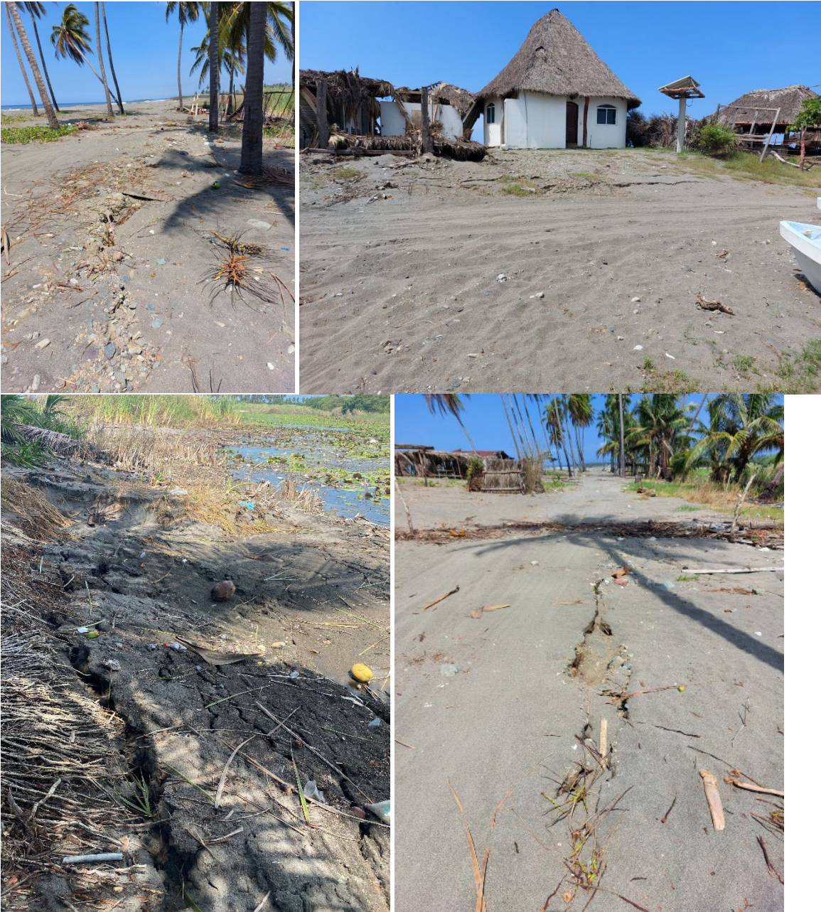
Figure 43. Lateral spreading in beach sands due to liquefaction, El Ticuiz, Michoacan. Waypoint Station 20 (Coordinates: 18.653076°, -103.700458°)
