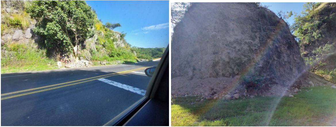
Figure 40. Rockfalls on cut slope along the road, Pialla, Jalisco. Waypoint Station 34 (Coordinates: 19.452558°, -103.469476°)
