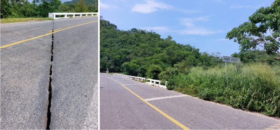
Figure 30. Gap of joints in decks of the bridge, Boca de Iguanas, Jalisco. Waypoint Station 4 (Coordinates: 19.321026^\circ , -104.817072^\circ )
