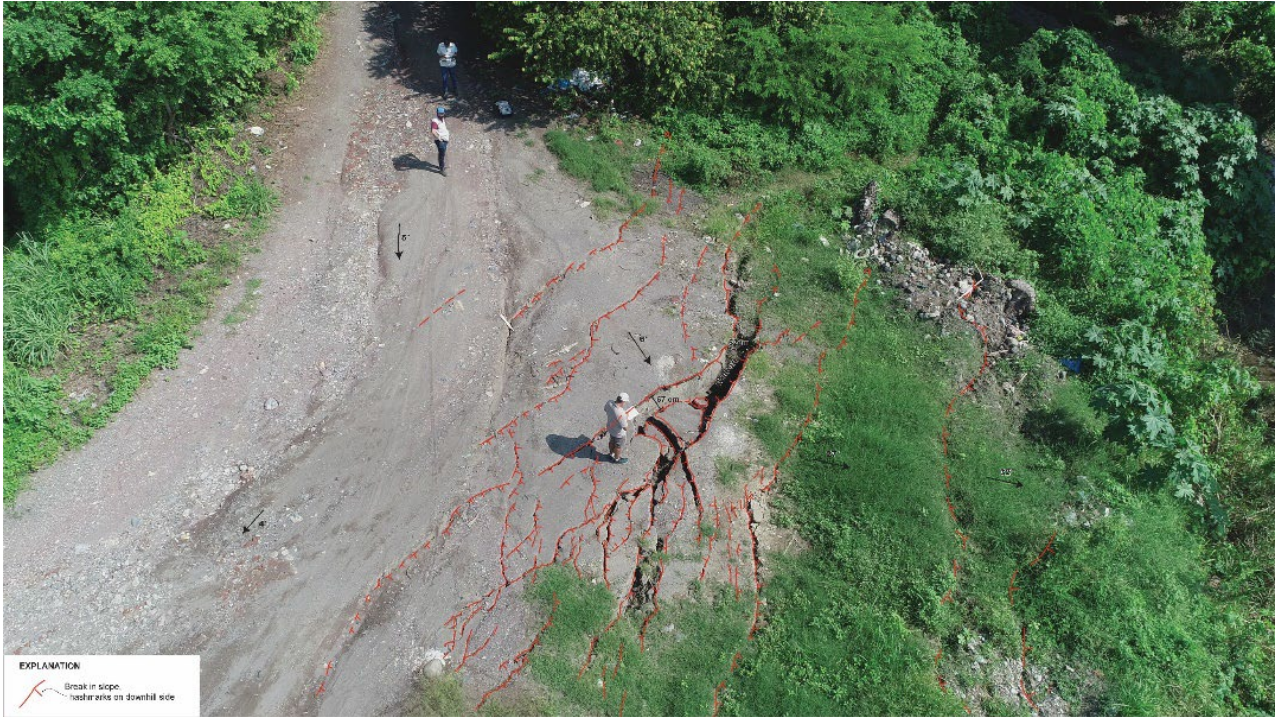
Figure 42. Lateral spread feature from Figure 41, La Zapotera, Colima. Red hash marks note cracks and lateral displacement of affected area. Waypoint Station 18 (Coordinates: 18.717472°, -103.716876°)
