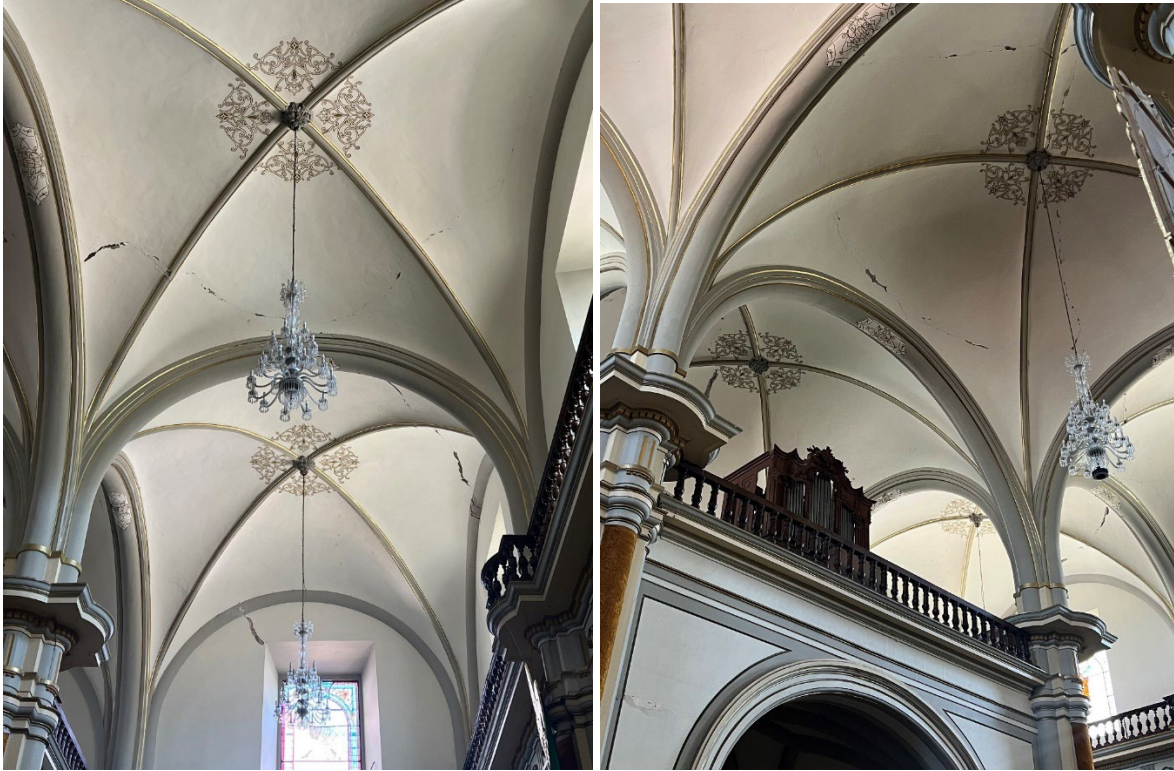
Figure 26. Roof cracking on church, Ciudad Guzman, Jalisco. Waypoint Station 37 (Coordinates: 19.703666°, -103.463191°)
