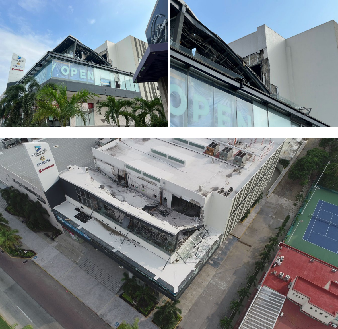
Figure 9. Collapse of roof in mall, Manzanillo, Colima, Waypoint Station 7 (Coordinates: 19.100552°, -104.325525°)
