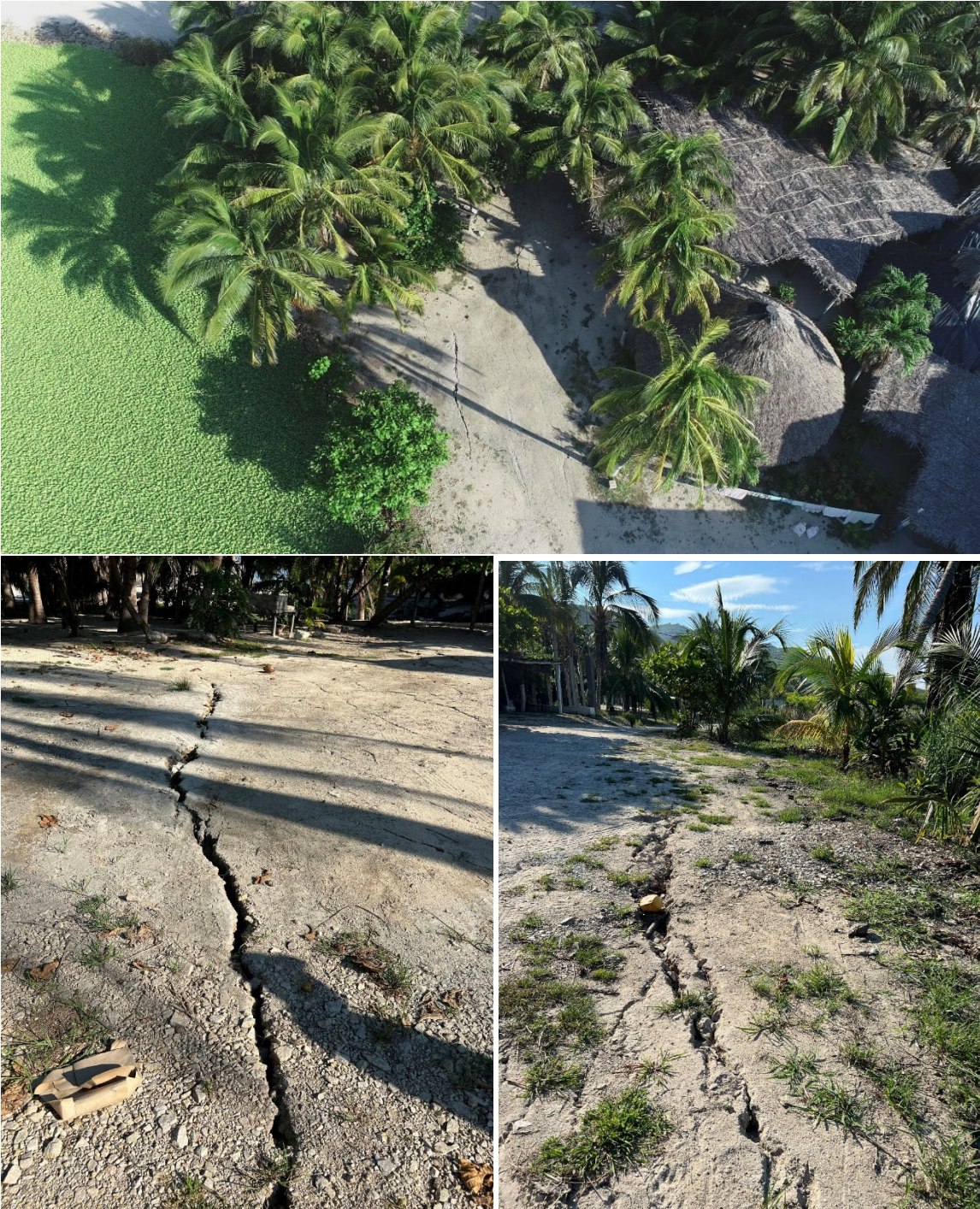
Figure 45. Lateral spreading and cracking in rural roads due to liquefaction, Maruata, Michoacan.
