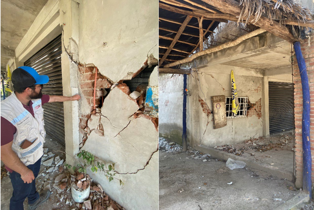
Figure 21. Collapse of masonry walls and damage to structural elements in community hospital and damaged column and wall of nearby masonry two story building, Maruata, Michoacan. Waypoint Station 28 (Coordinates: 18.27409°, -103.348231°)
