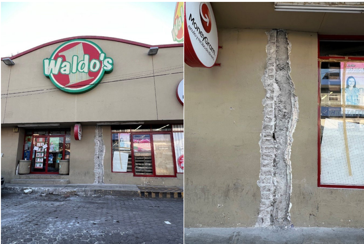
Figure 16. Column damage of supermarket, Tecoman, Colima Waypoint Station 14 (Coordinates: 18.910863°, -103.871611°)
