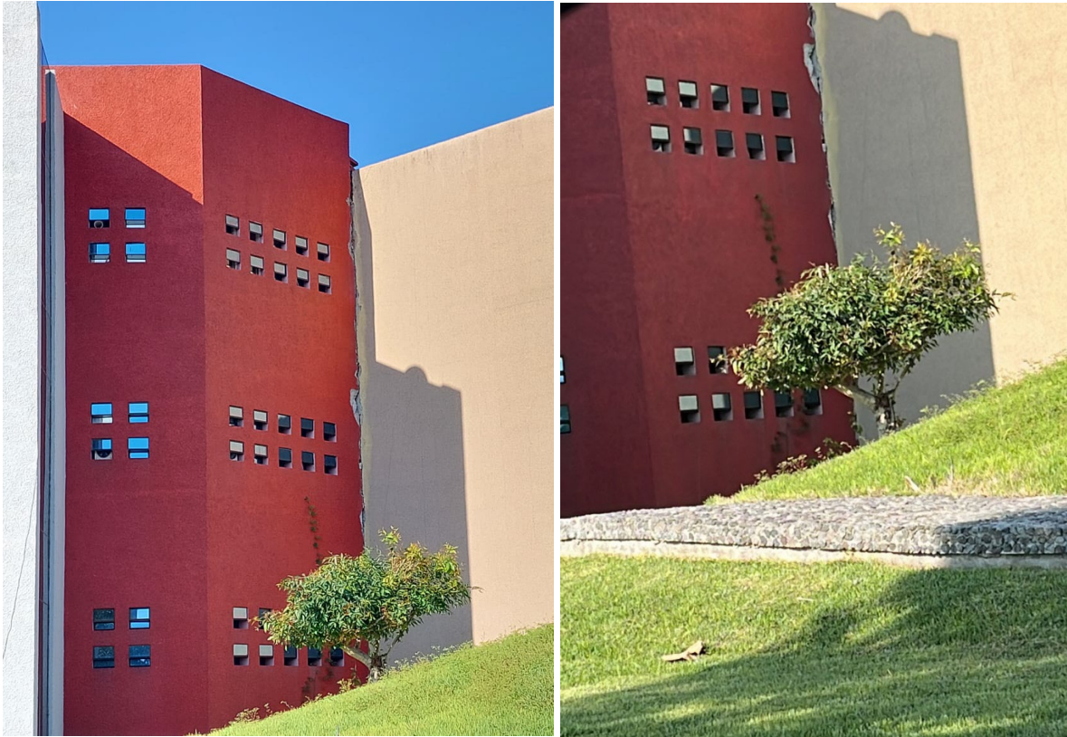
Figure 24. Vertical cracking in building, Colima, Colima. Waypoint Station 33 (Coordinates: 19.255976°, -103.687608°)
