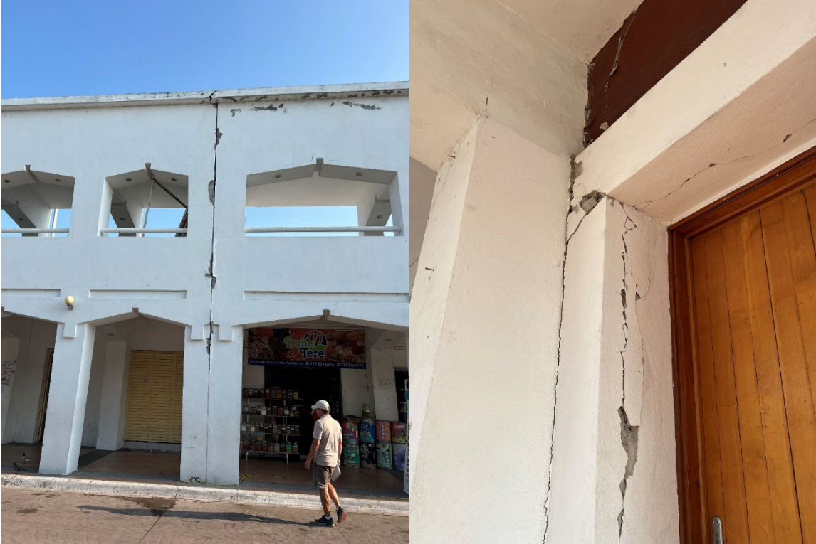
Figure 17. Damage in door frames and between structures, Tecoman, Colima Waypoint Station 15 (Coordinates: 18.910531°, -103.87186°)
