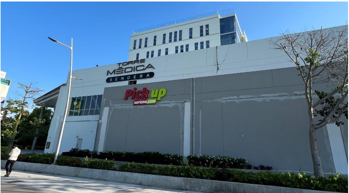
Figure 23. Cracking on non-structural elements with damage on the corner columns, Colima, Colima. Waypoint Station 32 (Coordinates: 19.275421°, -103.716969°)
