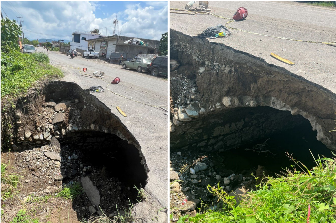
Figure 35. Collapse of the entrance of culvert made of masonry, Coahuayana, Michoacan. Waypoint Station 21 (Coordinates: 18.684114°, -103.669303°)
