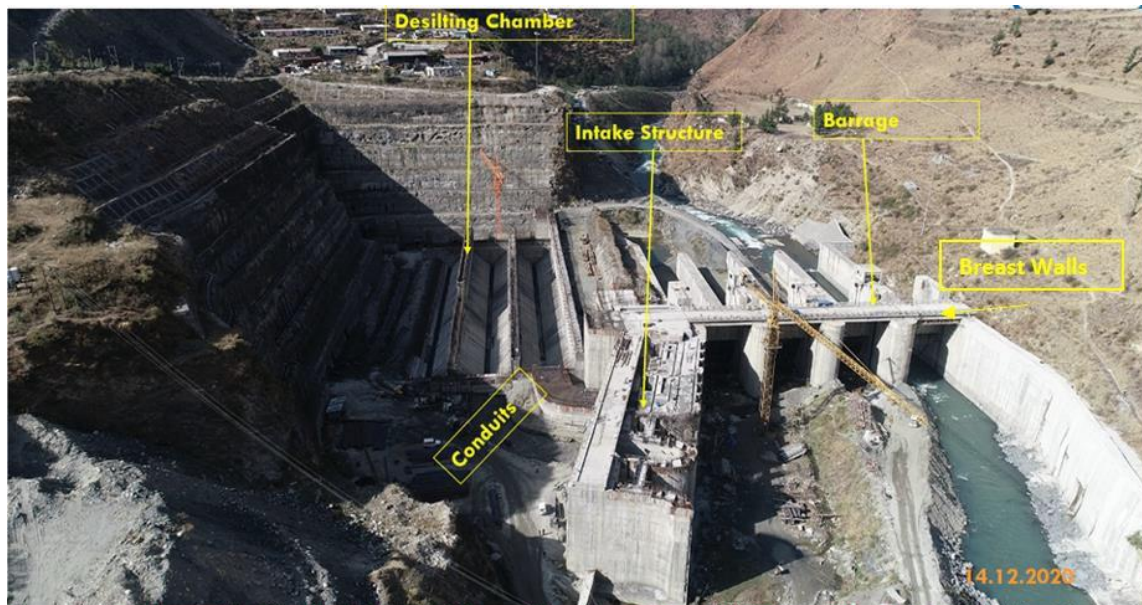
Figure 3.28 Close-up view of barrage site infrastructure (Source: NTPC Tapovan via National Institute of Disaster Management (NIDM), MHA-Webinar on Lessons from Chamoli Disaster 2021 https://www.youtube.com/watch?v=fE6vjZE6pUg&t=1709s ) @ 30°32'7.84"N 79°31'10.71" E
