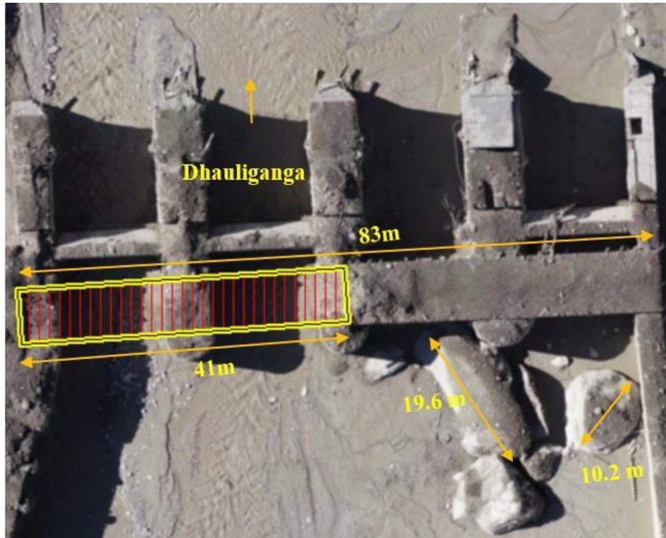
Figure 3.38 Dimensions of the existing and vanished portion of the breast wall (highlighted with red strips) along with the accumulated boulders. @ 30°29'35.89"N 79°37'41.67"E (Dated:11/02/2021)
