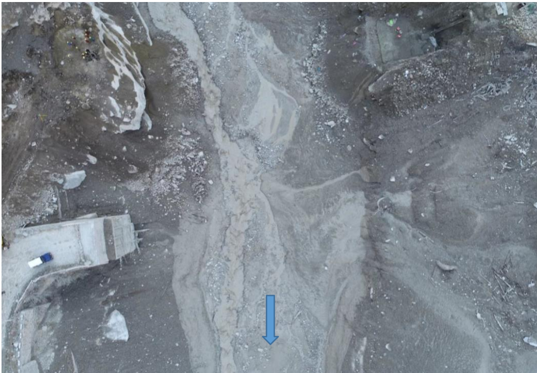
Figure 3.25 Damaged Raini bridge across the bank of Rishiganga River with only leftabutment and no decks. (30°29'7.95"N, 79°41'39.56"E) (Dated: February 11th, 2021)
