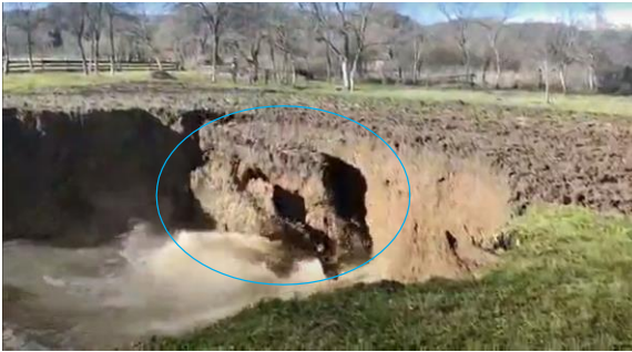
c) Large block collapse.
