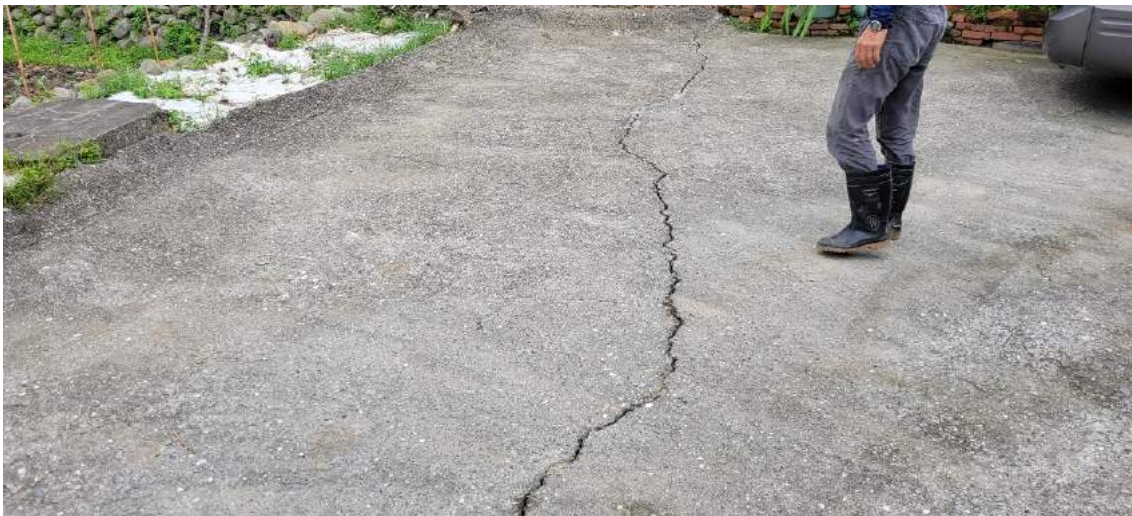
(a) Crack in pavement produced during mainshock. Lat: 23° 10' 28.945920", Lon: 121° 14' 54.936599"
