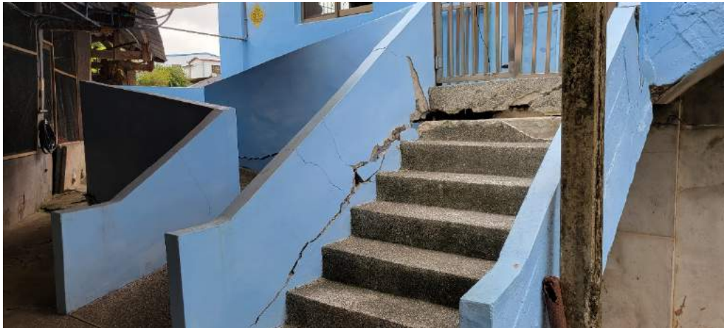
Figure 4.18 (c) Cracking in concrete stairs resulting from relative foundation displacement. Lat: 23^{\circ} 10' 28.512480'' , Lon: 121^{\circ} 14' 54.98628''
