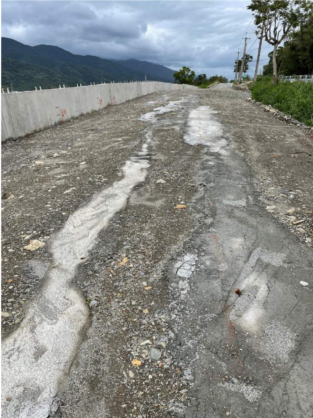
Figure 4.6: View looking north and ground cracking areas “repaired” with concrete. Failed retaining wall in upper left. Lat: 23° 8' 39.00048”, Lon: 121° 14' 12.52428”.
