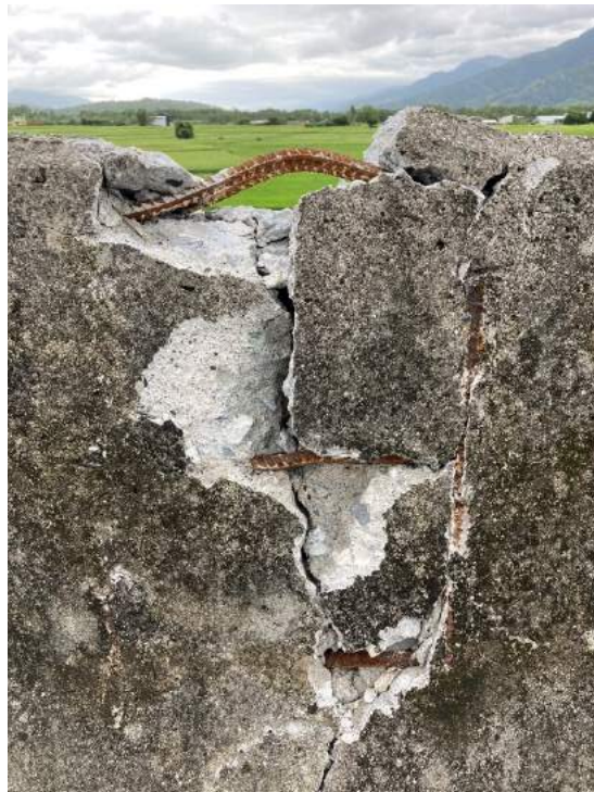
Figure 5.19. Compression buckling of concrete barrier steel reinforcement (23.26584° 121.29836°)
