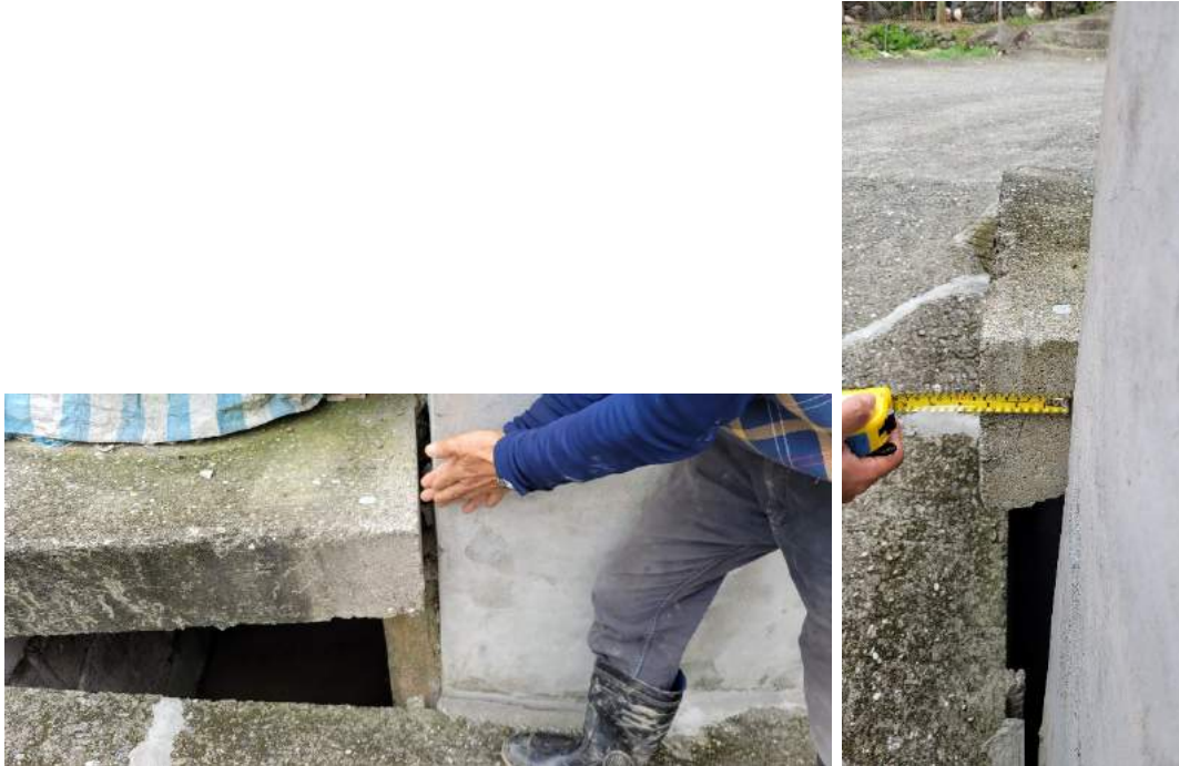
(e) Relative movement of foundation. Lat: 23° 10' 28.924320", Lon: 121° 14' 54.961080"
