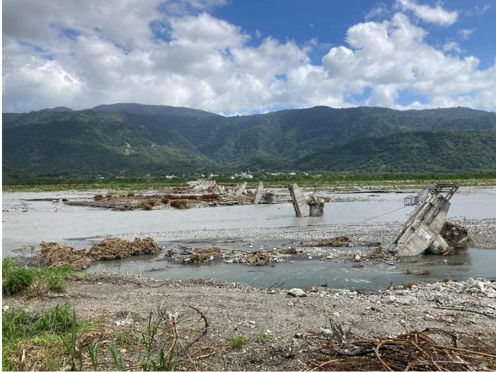
Figure 5.34. Looking towards the east abutment at the failed piers (23.38632° 121.33973°)
