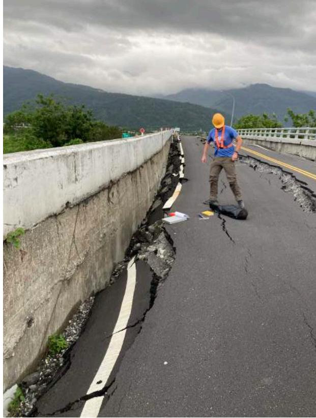
Figure 5.42. Roadway cracks and settlement in the east abutment looking west ( 23.38510^\circ 121.34767^\circ )
