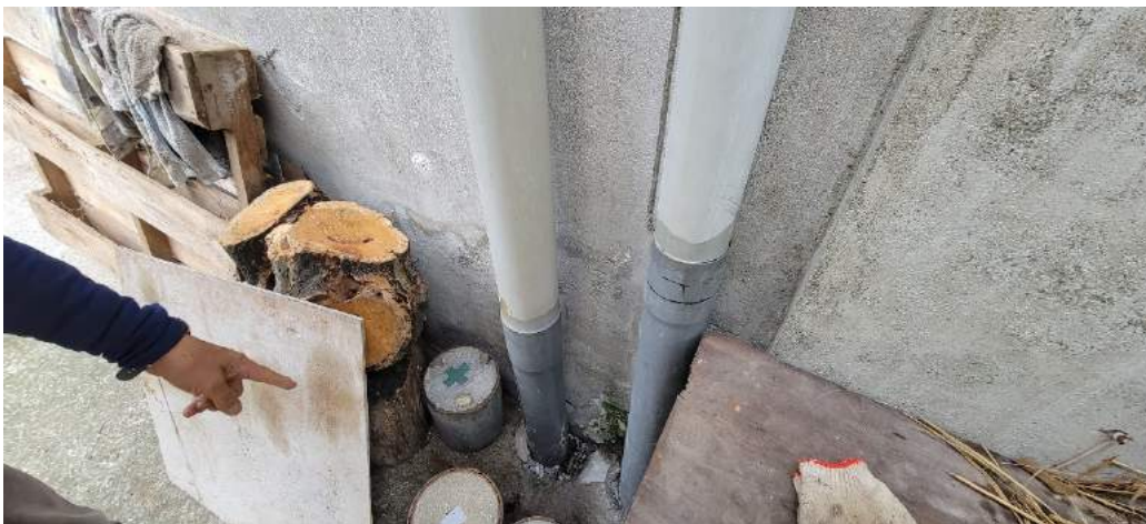
Figure 4.18 (a) Concrete damage due to relative foundation movement around water pipeline. Lat: 23° 10' 28.720199", Lon: 121° 14' 55.052159"
