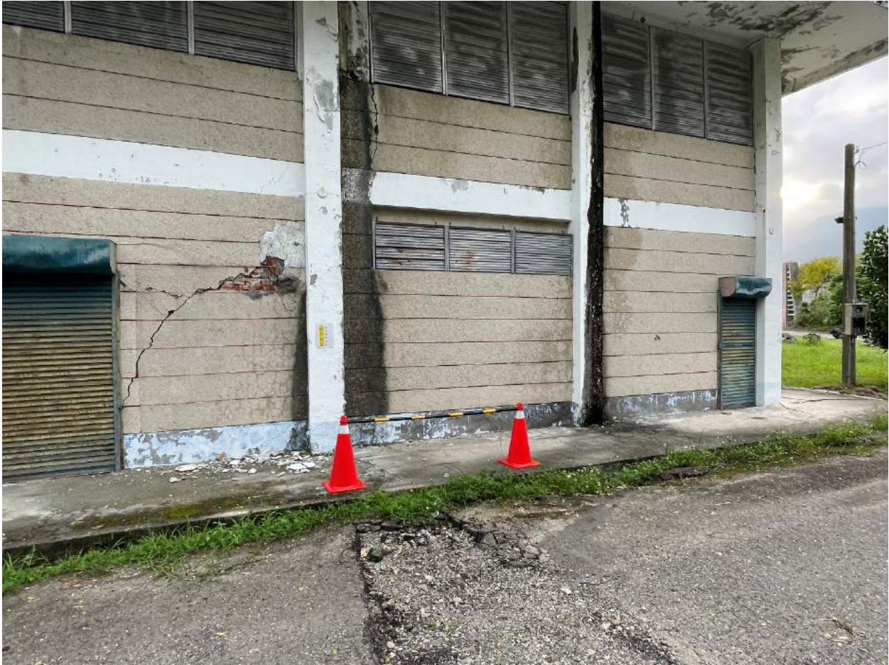
Figure 4.33: Damage to structure on the opposite side of the street from the retaining wall in the figure above. Cracking extends from the foundation to the roof, Lat: 23° 15' 46.403640", Lon: 121° 18' 9.362160"
