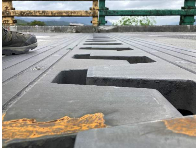
Figure 5.31. Typical differential movement at a Figure 5.joint. (23.32240°121.33194°)
