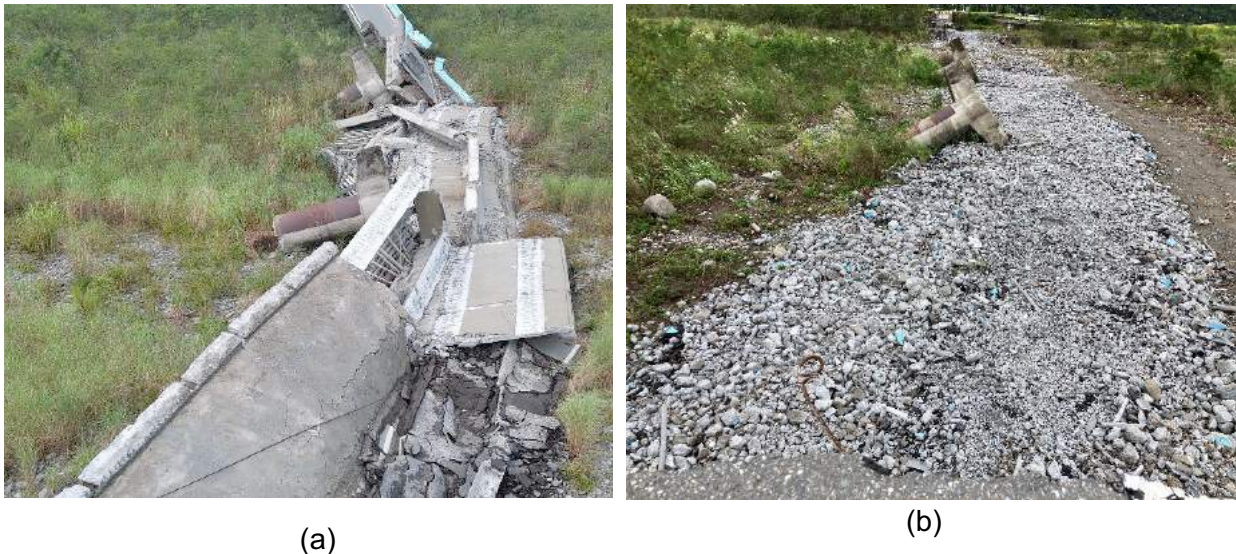
Figure 5.6. a) Failed spans and pier foundation supports at the Luntian Bridge (image curious of NCREE); b) view for concrete bridge piers after deck removal during GEER team visit in October 2022 (23.21726° 121.27172°)
