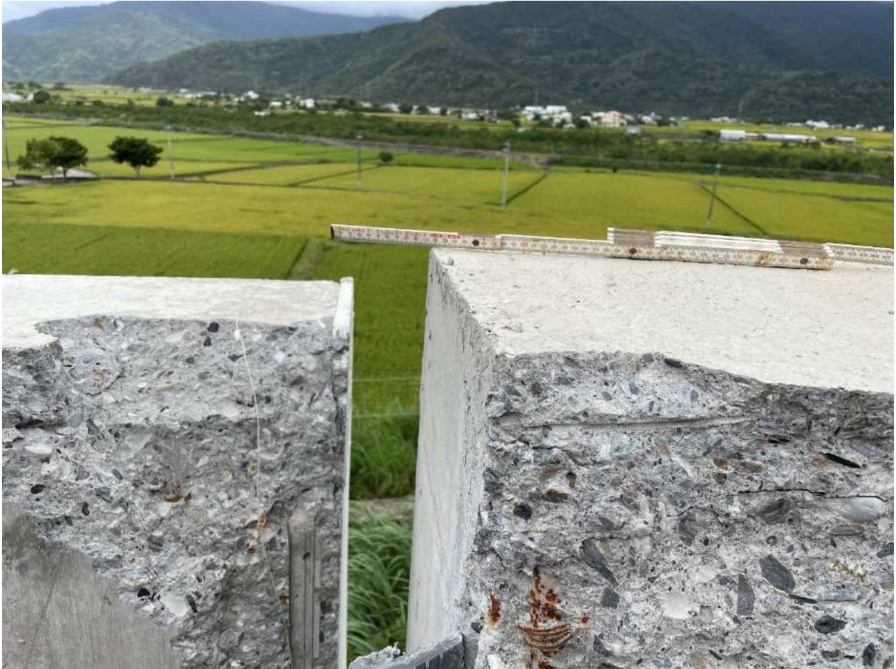
Figure 4.4: View looking west showing separation of joint between 20-m wall sections. Lat: 23° 8' 44.762279", Lon: 121° 14' 14.010719".
