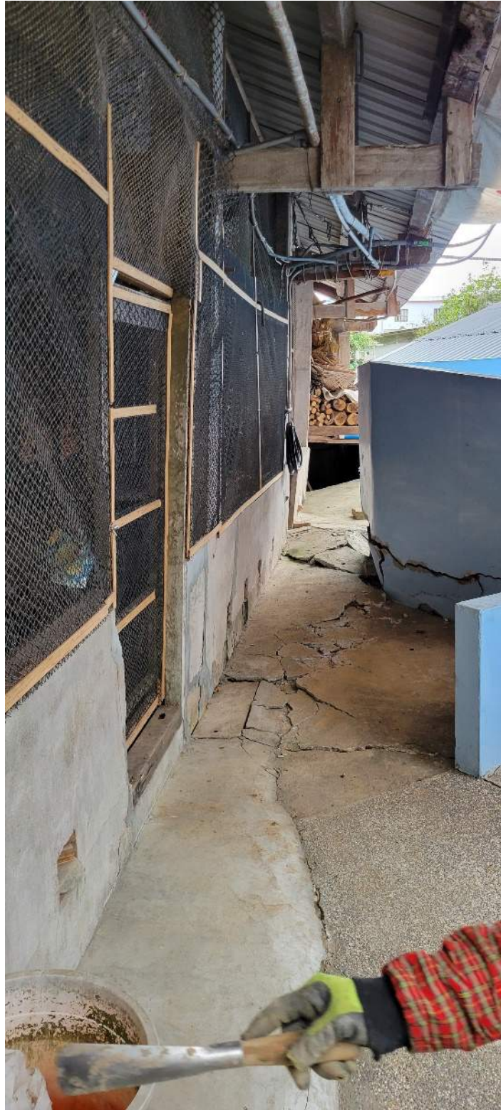
Figure 4.18 (d) Pavement buckling. Lat: 23° 10' 28.520039", Lon: 121° 14' 55.023719"
