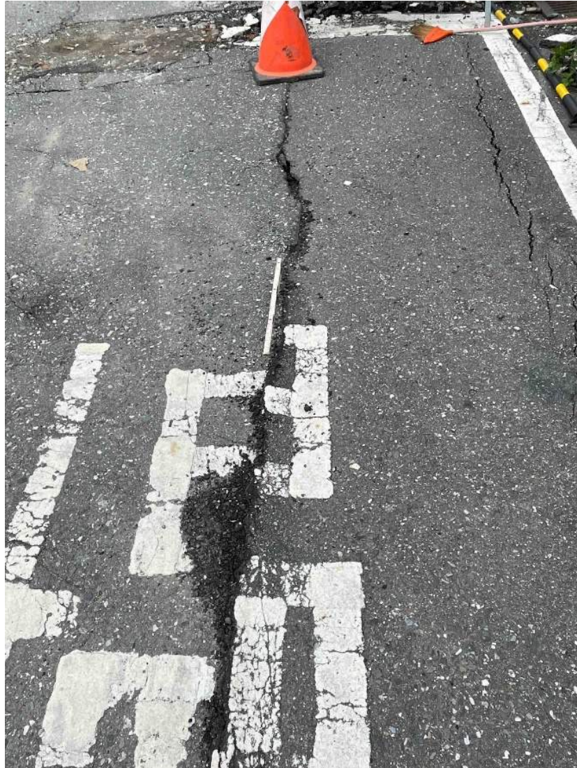
Figure 4.11: Surface rupture coincident with fault-parallel sewer line. Discrete LL offset is 18 cm. Lat: 23° 10' 24.693599", Lon: 121° 14' 54.185999"
