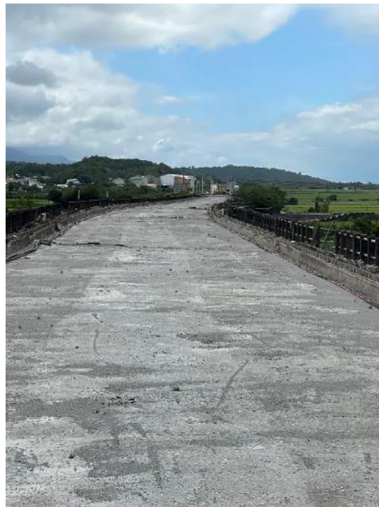
Figure 5.24. View from the bridge deck of the Dongli Railroad Bridge with the train rails removed. The twist in the deck was due to the lateral translation of the prestressed girders. (23.27829° 121.30669°)
