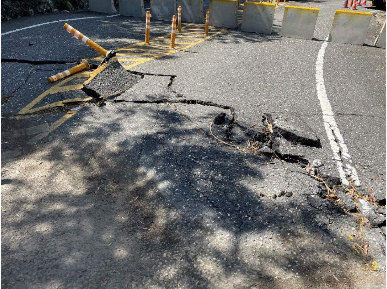
Figure 4.34: Surface rupture through the bridge approach near projected location of the LVF. Asphalt pavement buckled and locally detached. View looking southwest, Lat: 23° 15' 46.403640", Lon: 121° 18' 9.362160"
