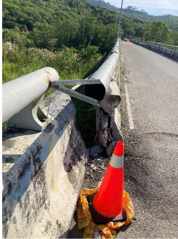
Figure 5.3. Lateral offset, looking towards the east abutment. (22.97484° 121.17017°)
