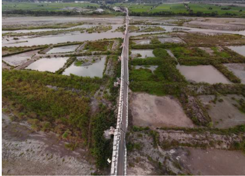
Figure 5.32. Failed spans of the Gaoliao bridge looking west (Image courteous of Zola Zhou, 23.38563° 121.34458°)
