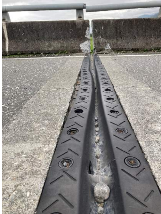
Figure 5.18. Damage to expansion joint, concrete and metal barriers (23.26557° 121.29901°)
