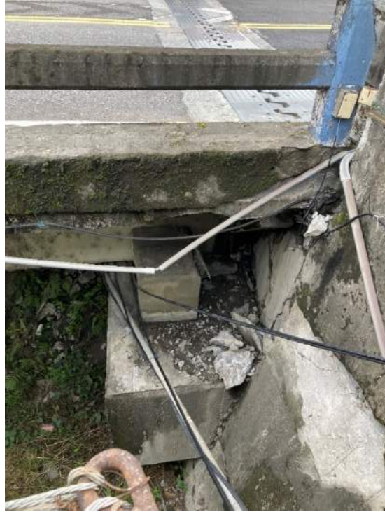
Figure 5.29. Damage to the North Yuli bridge east abutment and adjacent utility lines. (23.32233° 121.33240°)
