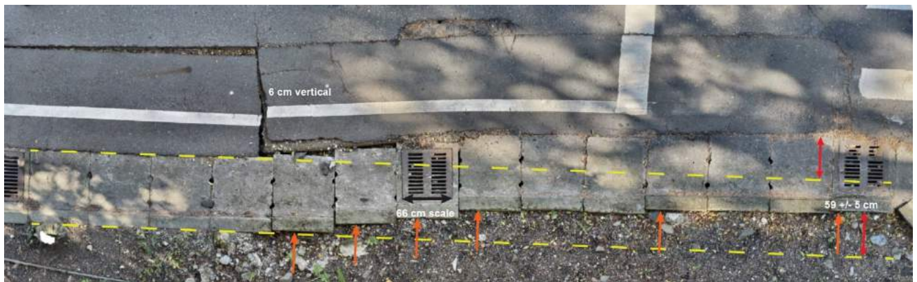
Figure 4.22: offset of sewer lateral in Fuli. The best estimate of total LL displacement is 59 cm, include possible pre-event creep and/or prior surface rupture on the LVF.
