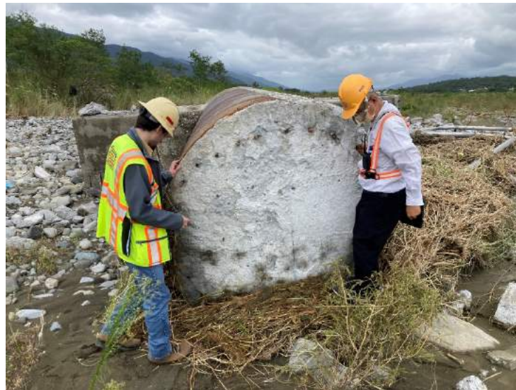
Figure 5.12. Typical view of one of the failed piers with irregular longitudinal rebar spacing. (23.21775° 121.27062°)
