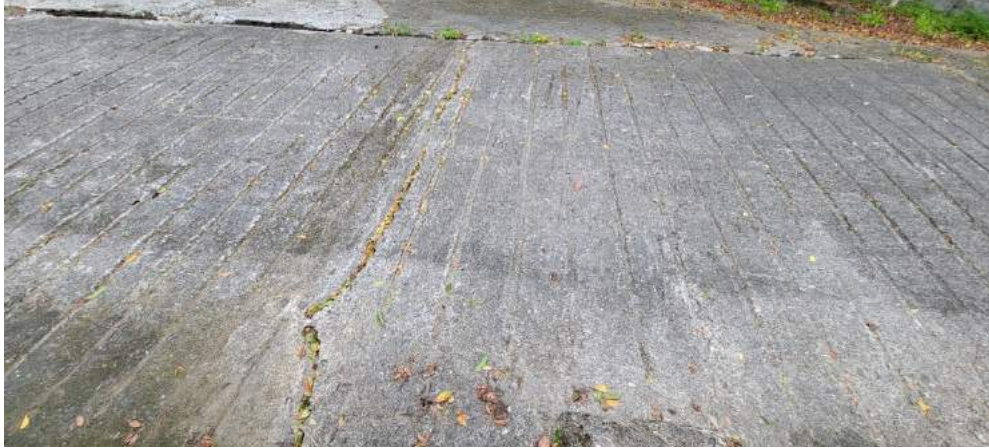
(d) Cracks in walkway between private property and Fuli Junior High School. Whether this crack was directly caused by the September 18 earthquake is uncertain. Lat: 23° 10' 28.848720", Lon: 121° 14' 56.038199"
