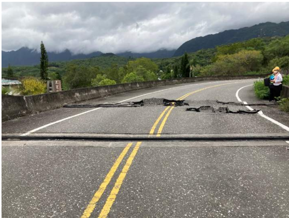
Figure 5.17. 41 cm lateral offset between bridge span and abutment. (Asphalt buckling due to surface fault rupture) (23.26452° 121.30089°)
