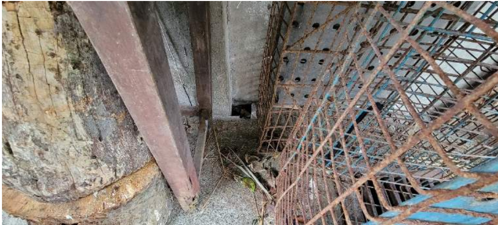
Figure 4.18 (b) Separation of concrete walls from foundation. Lat: 23^{\circ} 10' 28.626959'' , Lon: 121^{\circ} 14' 54.975479''
