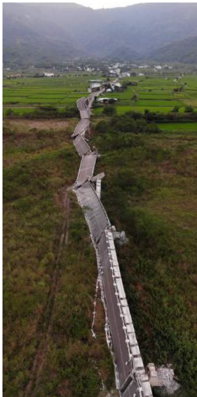
Figure 5.33. Failed spans of the Gaoliao bridge looking east (Image courteous of Zola Zhou, 23.38563° 121.34458°)
