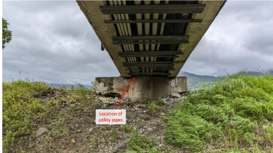
Figure 5.9. Looking west at the 2 nd pier from the east abutment following the earthquake. Note the north translation of the utility pipes from Figure 5.8. (23.21457° 121.27268°)
