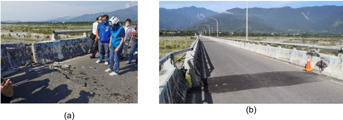
Figure 5.2. a) Damage between adjacent bridge spans buckling roadway, concrete barrier, and metal guardrail (United Daily News), looking south; b) repaired roadway and metal guardrail damage during GEER/NCREE visit looking northwest. (22.9748° 121.1702°)
