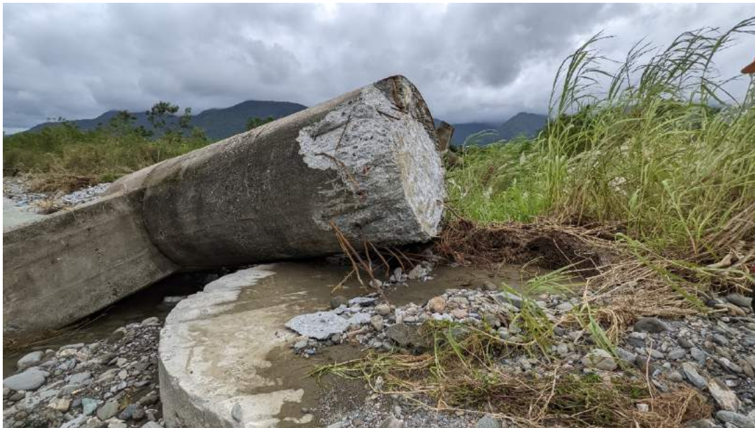
Figure 5.14. View of failed bridge pier and concrete pad. Note the yield longitudinal rebar connecting the pier to the concrete pad. (23.21771° 121.25425°)
