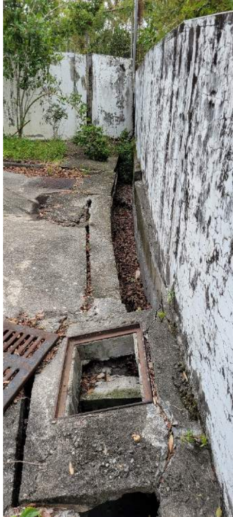
(g) Inward buckling of concrete wall. Uncertain as to whether this was a direct result of the September 18 earthquake. Lat: 23° 10' 28.223039", Lon: 121° 14' 56.014799"
