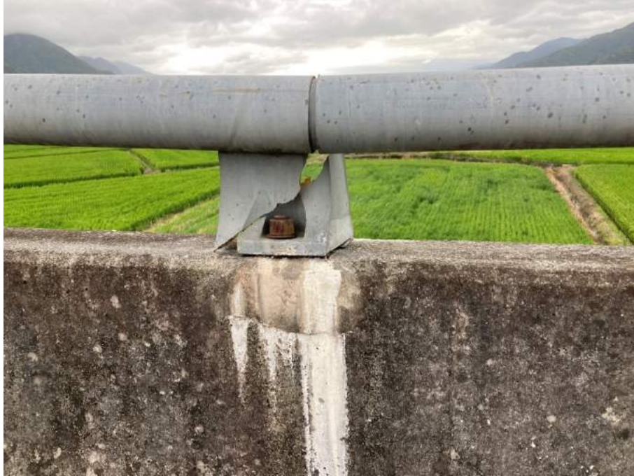
Figure 5.20. Shear failure in metal guardrail bracket caused by compressional loads. (The expansion joint preventing tensile loading) (23.26568° 121.29870°)
