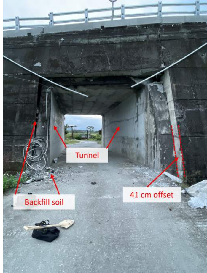
Figure 5.43. Tunnel beneath east bridge approach, 41 cm offset from gravity wall, and backfill soil that flowed from gap between the gravity wall and tunnel liner (23.38526° 121.34783°)
