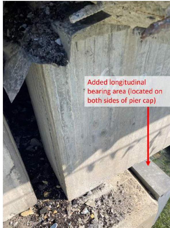
Figure 5.5. View of typical retrofit by adding additional bearing area to prevent longitudinal unseating (22.97479° 121.17059°)
