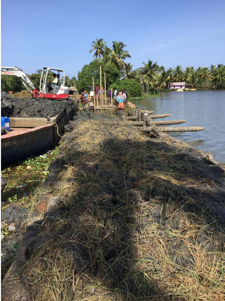
Figure 5.5: A major bund failure of roughly 50m long near Kainakari @ 9.5029947°N 76.3749555°E. The left side of the bund in the photograph is the lake and the right side of the bund is the flooded fields.
