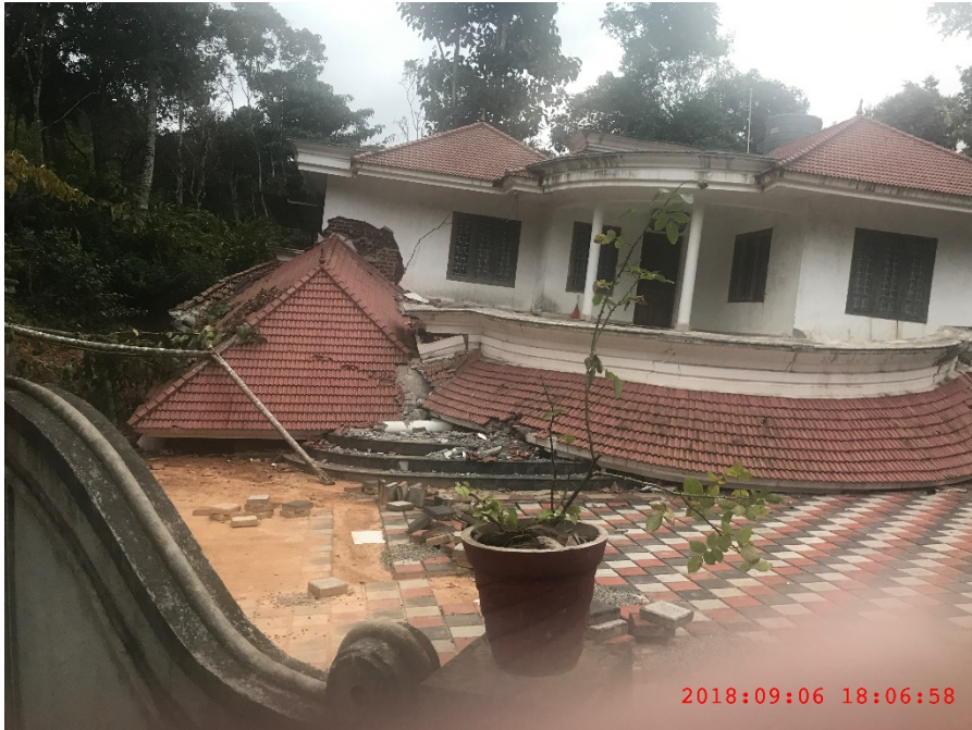
Figure C-4: Building destroyed due to ground movement. An entire floor has been subsided @ 9.8746102^{\circ} N 77.1193815^{\circ} E
