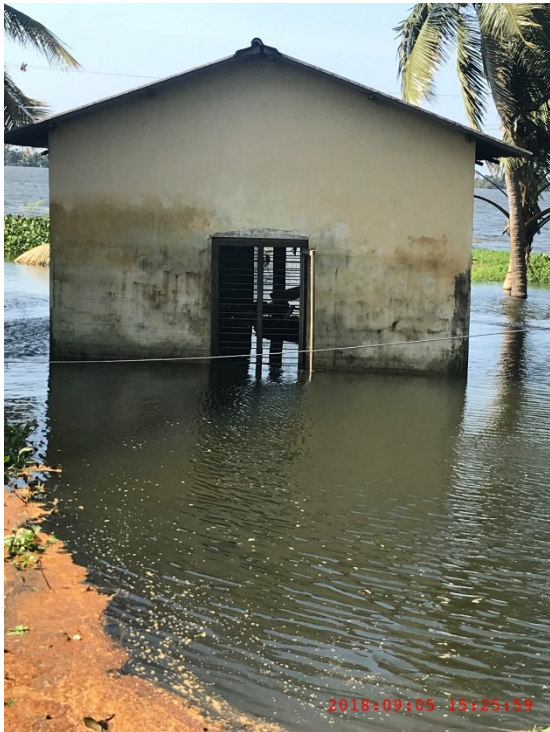
Figure 5.9: Flooded home due to bund failure @ 9.5032691^{\circ}\text{N } 76.3776221^{\circ}\text{E}
