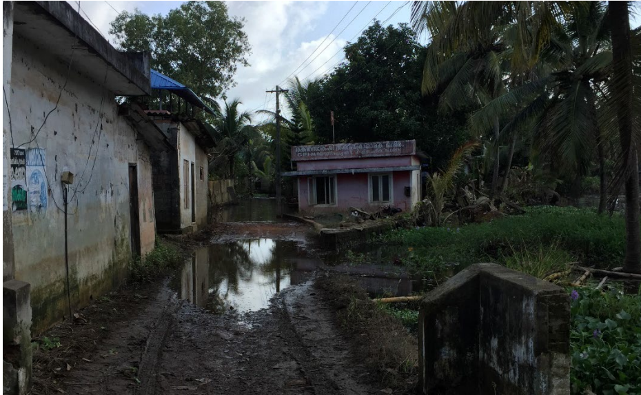
Figure 4.7: Photograph of building that tilted due to differential settlement following floodwater withdrawal (Latitude=9.453415°, Longitude=76.385143°).
