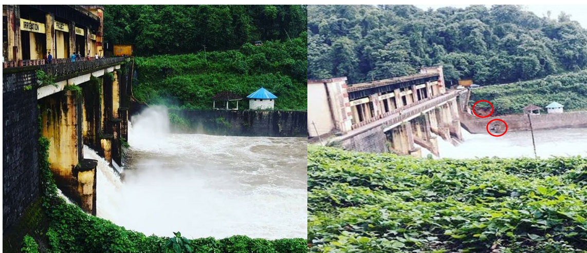
Figure 3.8: (Left) Downstream side of the Maniyar Dam with the shutters open on August 10th. (Right) Similar view as the left image taken on August 25 th showing minor slope failure and damage to the retaining structure (failures are circled in red). Source of photograph: Instagram
