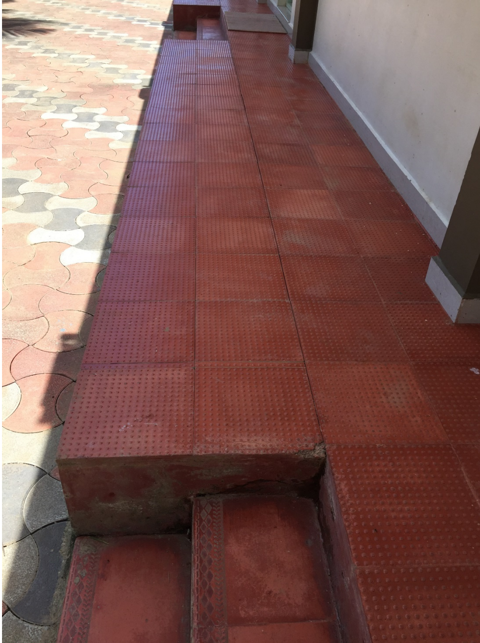
Figure 4.18: Photograph of cracking occurring in the concrete pavers surrounding the pile supported Mar Sleeve Church of Ponga building.
