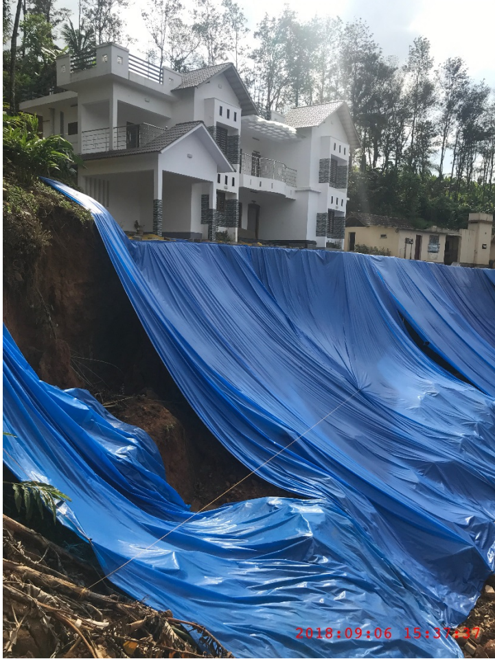
Figure A-11: Large landslide in front of the newly built house @ 9.7925061^{\circ} N 77.0680952^{\circ} E
