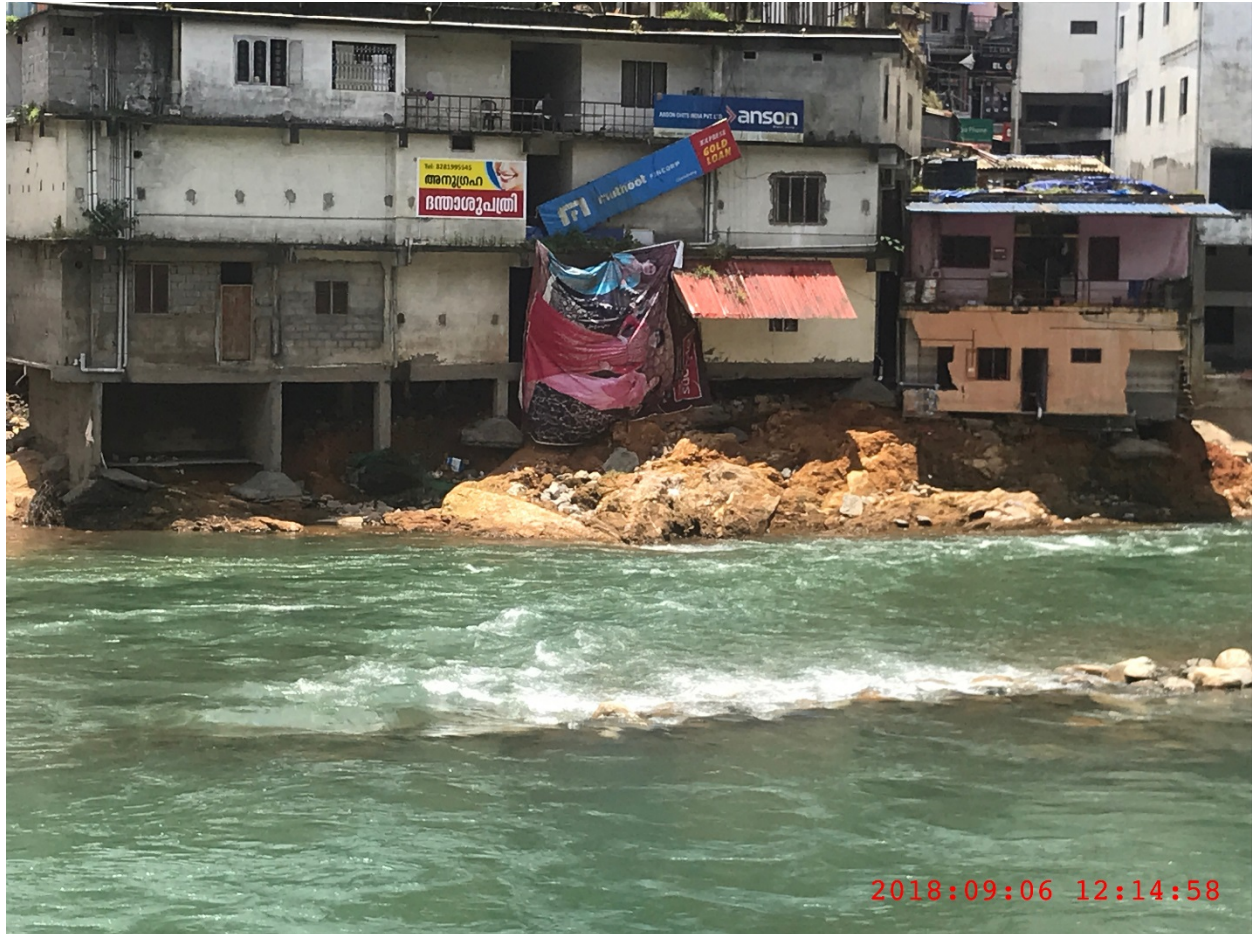
Figure B-1: River erosion @ 9.8575718° N 76.9636035° E
