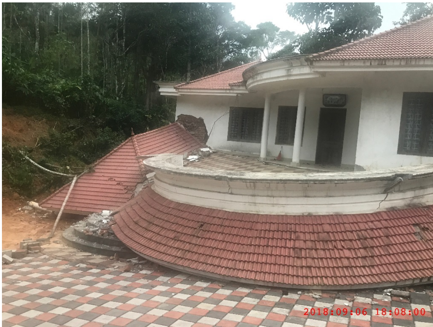
Figure C-5: Building destroyed due to ground movement. An entire floor has been subsided @ 9.8747156^{\circ} N 77.1193791^{\circ} E
