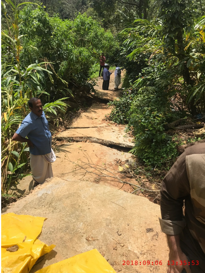
Figure A-8: Driveway to the house destroyed in landslide @ 9.7962622^{\circ} N 77.0681814^{\circ} E
