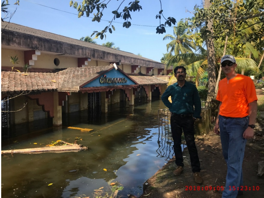
Figure 5.8: Entrance of the flooded community hall @ 9.5033389^{\circ}\text{N } 76.3772861^{\circ}\text{E}
