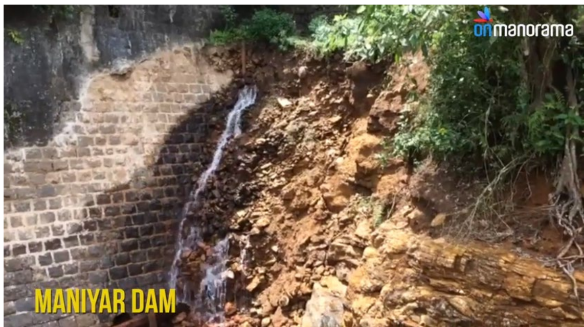
Figure 3.9: Closer view of the slope failure and seepage at the downstream side of the Maniyar dam (Source: manoramaonline.com).
