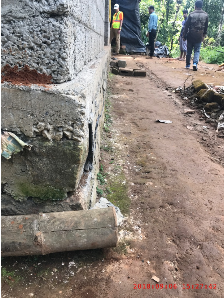
Figure C-3: Another view of the foundation crack @ 9.7918219^{\circ} N 77.0688023^{\circ} E
