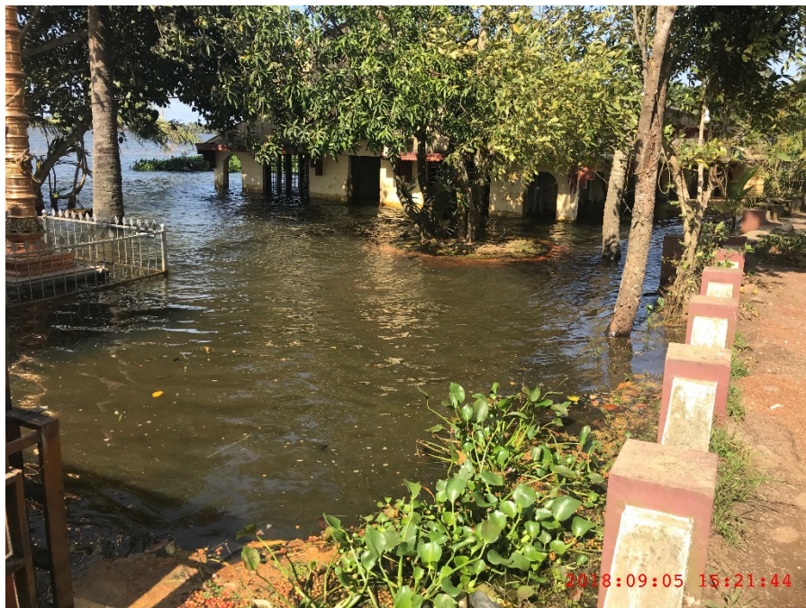
Figure 5.7: Flooded community hall from the bund failure @ 9.5033444 0 N 76.3770758 0 E
