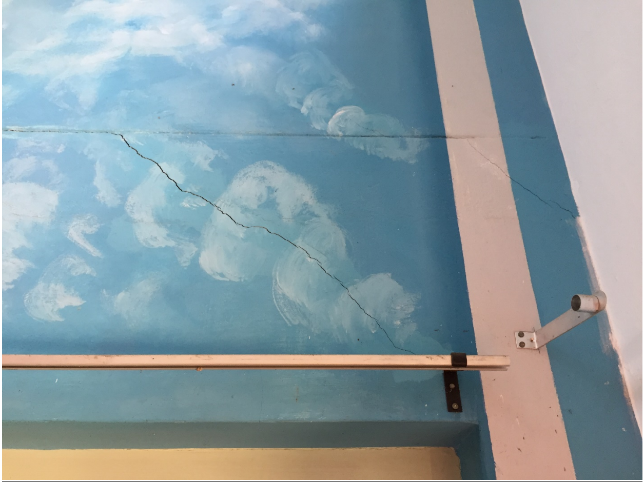
Figure 4.17: Photograph of cracking observed within the back wall of the Mar Sleeva Church or Ponga.
