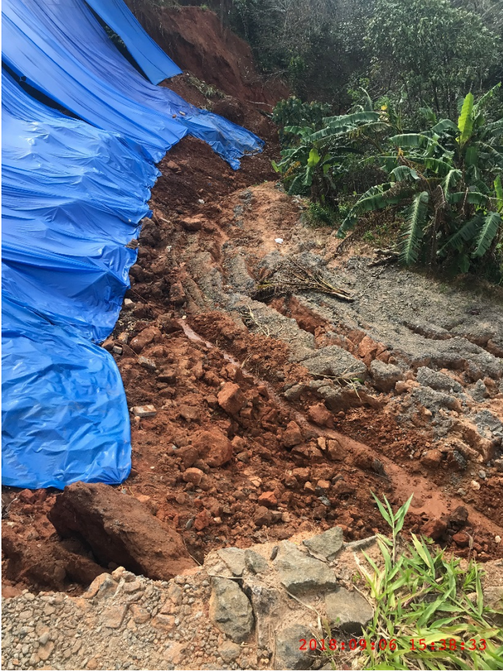
Figure A-12: Head of the landslide @ 9.7925131^{\circ} N 77.0680889^{\circ} E
