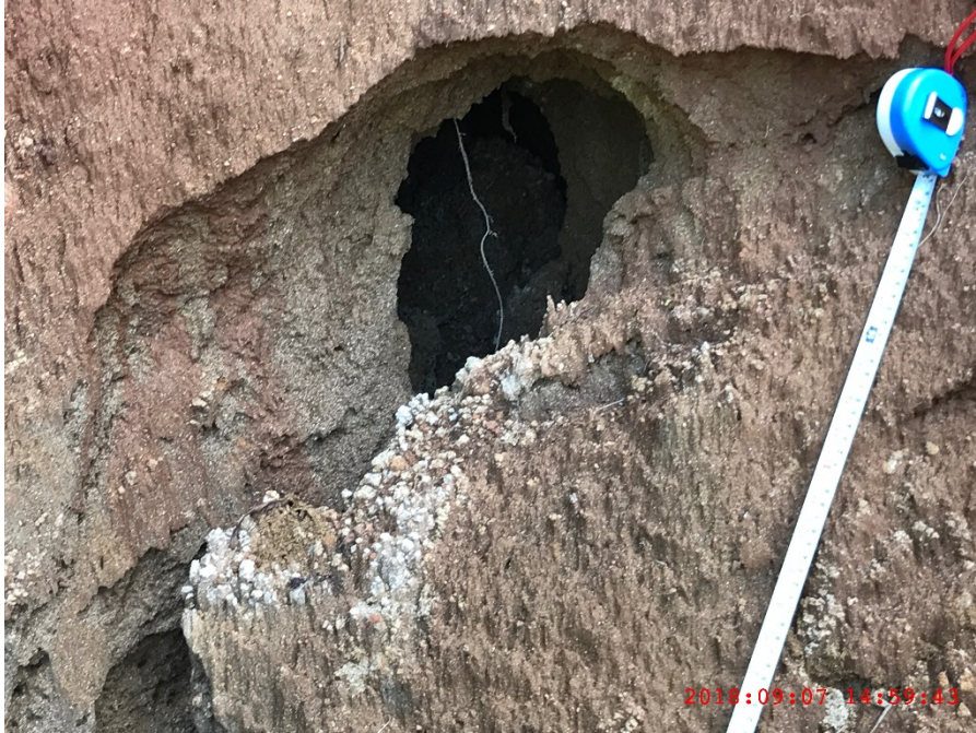
Figure A-20: Example of soil pipping @ 10.0088136° N 77.0257626° E
