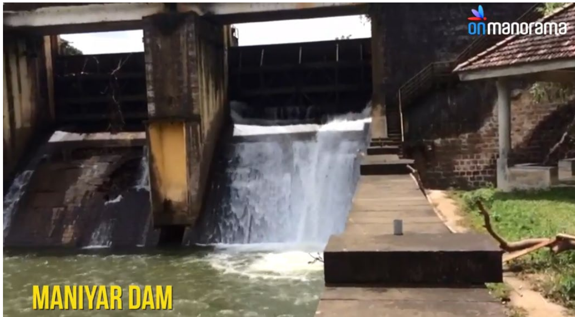
Figure 3.10: Photograph showing one shutter of the dam being closed and the surface concrete blocks been damaged (Source: manoramaonline.com).
