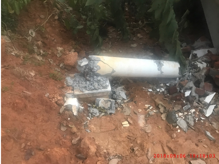
Figure C-6: Column of the building destroyed due to ground movement @ 9.8746397^{\circ} N 77.1193175^{\circ} E
