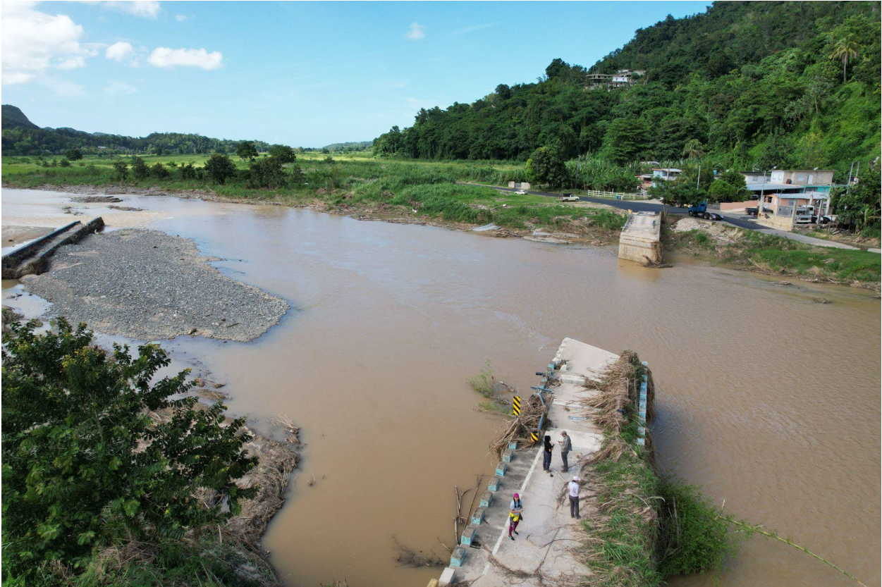
Figure 33: Aerial view of a temporary bridge failure along the Río Grande de Arecibo in Arecibo (18.3917, -66.6805). View is looking North. Note large amounts of vegetation that was caught by the bridge and the section of bridge washed away at the left center of the photo. Humans on bridge for scale
