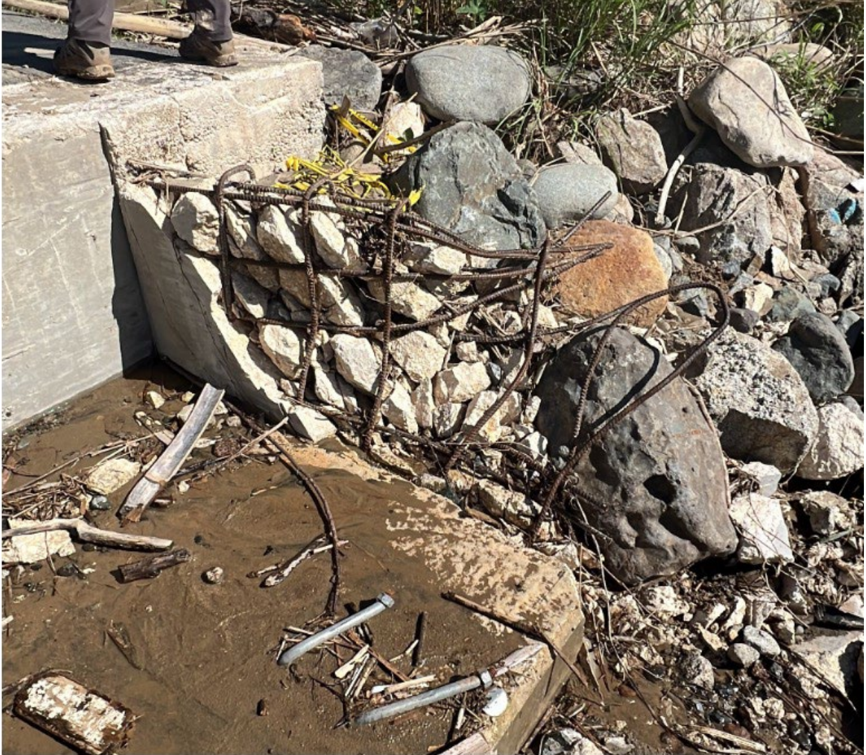
Figure 32: Destroyed concrete structure with rebar (deflected in downstream direction) on the western abutment of the temporary bridge in Utuado that was washed away during Hurricane Fiona
