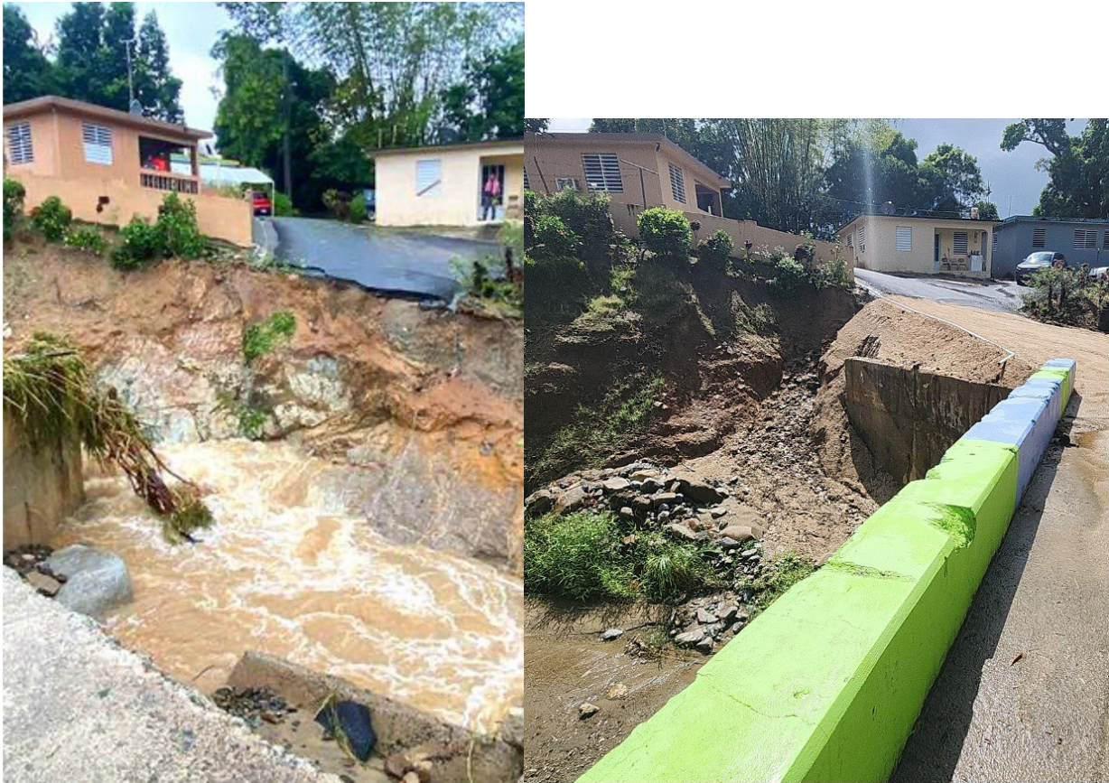
Figure 39: Example of bank erosion along the abutment of a small bridge over the Rio Maunabo in Maunabo (18.0289, -65.9475). The bridge did not suffer but the complete abutment and river bank was washed away. The area washed out was replaced with fill material to provide access to residents of a small isolated community beyond the bridge crossing.
