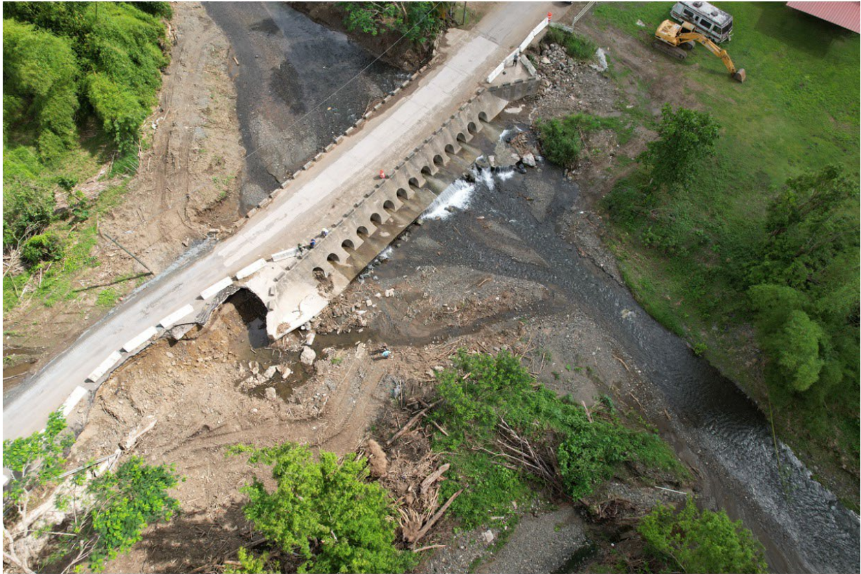
Figure 38: Aerial view of the PR-358 bridge over the Rio Hoconuco in San Germán (18.116, -67.071). The bridge structure did not fail, however, the abutments on both sides partially failed due to high discharge over and around the bridge during Hurricane Fiona.
