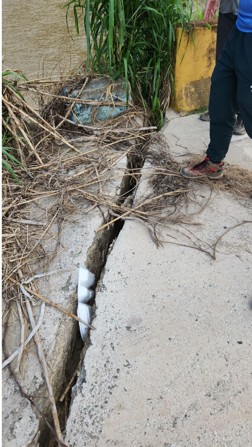
Figure 34: Horizontal separation of bridge segments along the Rio Grande de Arecibo bridge failure site in Arecibo. Separation is wider on the upstream side of the structure, indicating downstream rotational movement.
