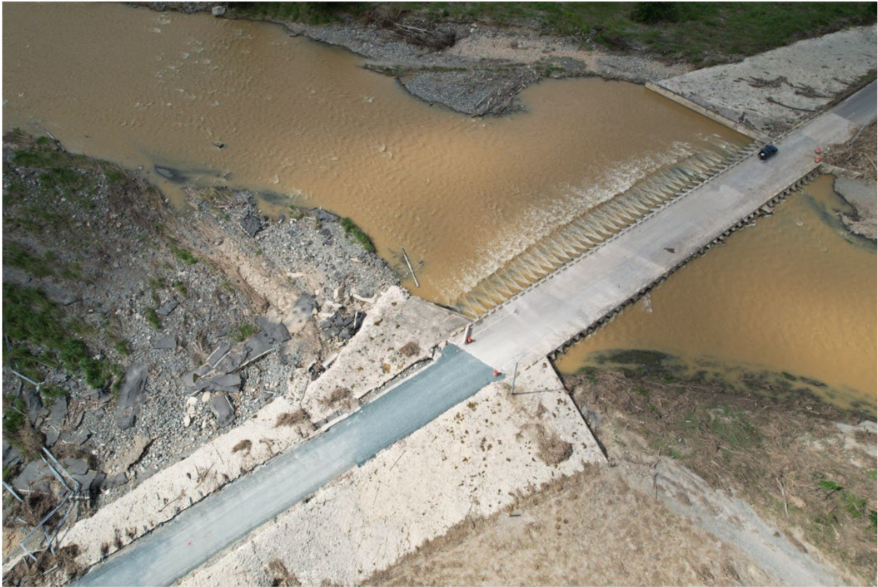
Figure 36: PR-123 bridge over the Rio Grande de Arecibo in Arecibo (18.368, -66.684). This bridge did not fail during Hurricane Fiona but the approaching abutments on either side had to be rebuilt following the storm. View is looking Northwest.
