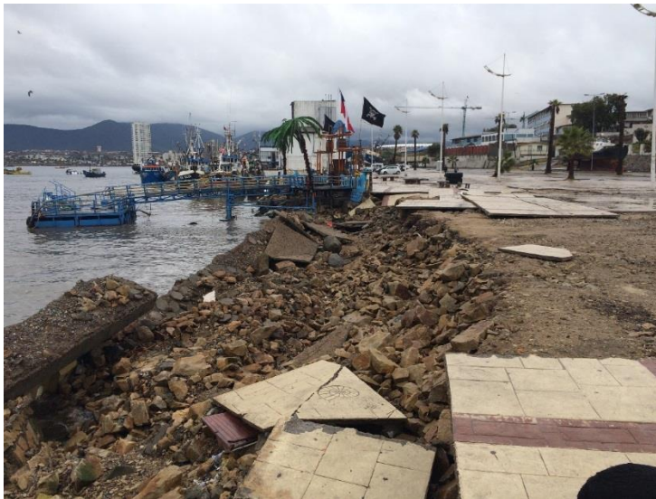
Figure 3.2. Failure of gravity walls at Coquimbo's waterfront (29.951370S; 71.335721W).
