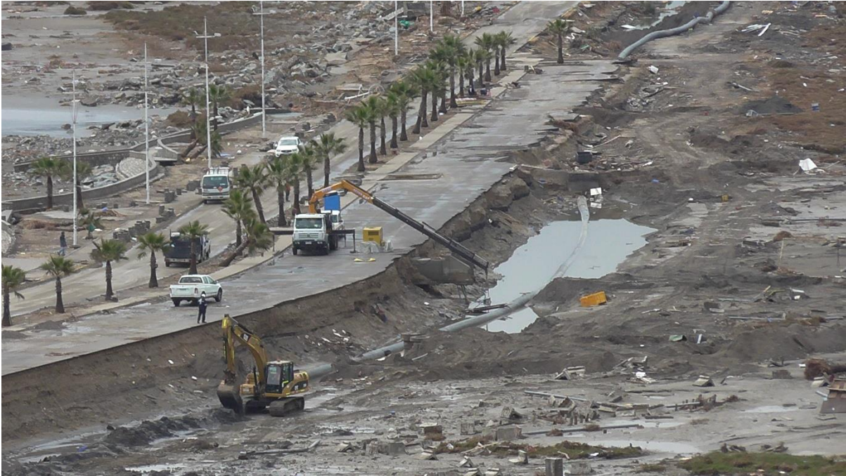
Figure 6.3. Tsunami erosion and scour along Avenida Costanera, Coquimbo (29.960589S; 71.328062W).
