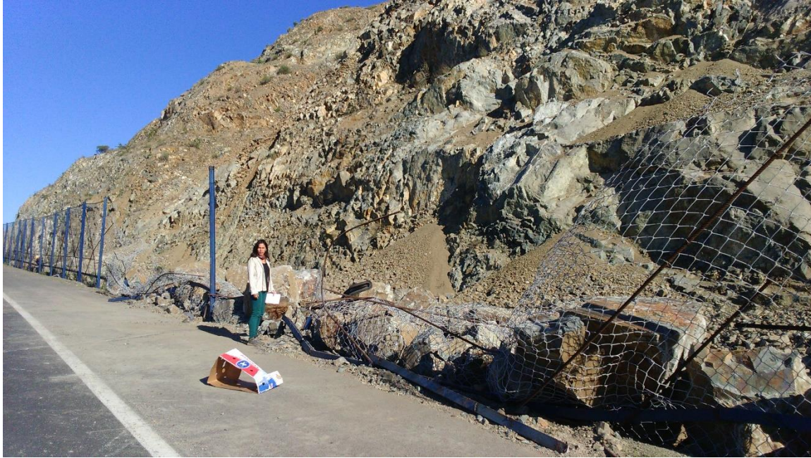
Figure 4.5. Km 305, northbound lane Route 5 showing failed rockfall mitigation fences (debris in the road had previously been cleaned up by highway department (GPS RF5: 31.23193S; 71.58976W).
