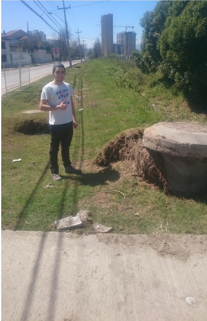
Figure 5.14. Field photograph looking northeast along Los Pescadores street. Note services have floated to the surface (uplifting the soil in blocks on to the right of person). Sewer top is now 70 cm above around surface. Note the second sewer portal behind person. Ground subsidence is also clear with the ground subsiding 20-30 cm relative to the road at this location. Surface water channel (runoff) runs directly behind the main sewer portal and parallel with the road (29.95068S; 71.29456W).
