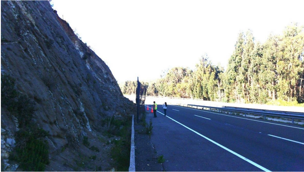
Figure 4.3. Km 295 northbound lane showing how the rockfall mitigation fences functioned well at this location and protected the road (GPS RF4: 31.31521S; 71.59444W).
