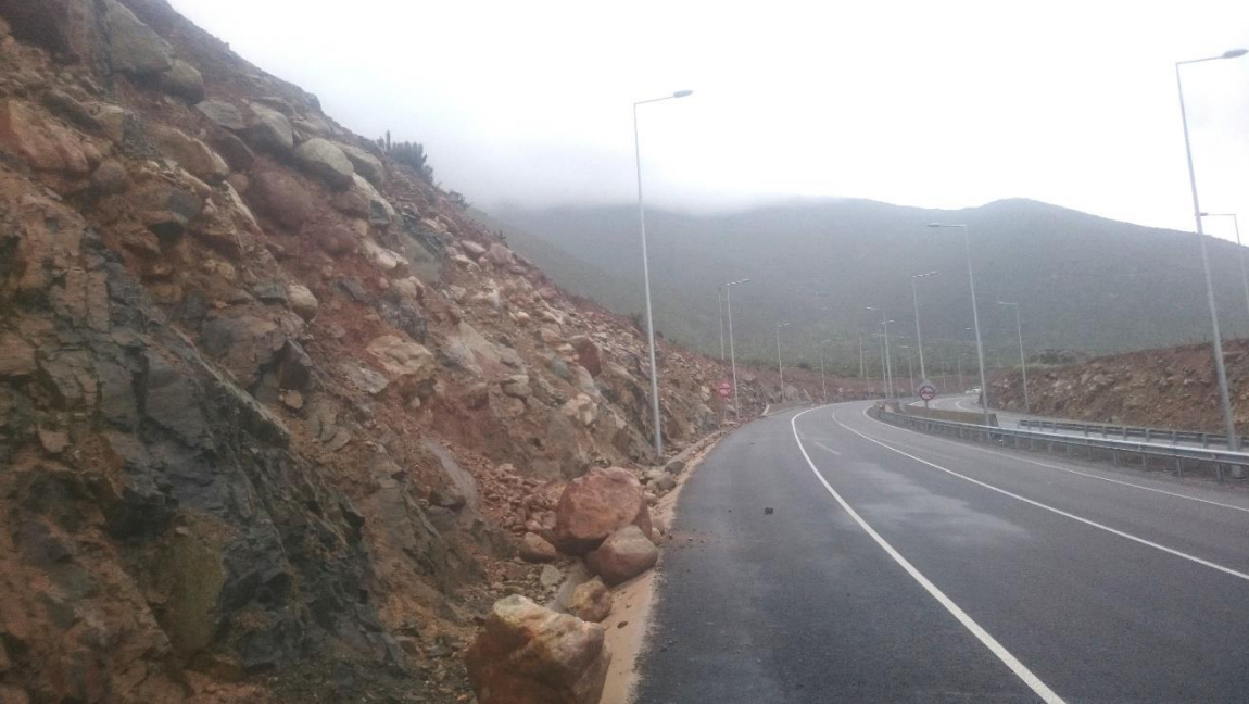
Figure 4.9. Km 508, northbound lane, alluvium (boulders), that fell from the road cut (looking south). Some of these boulders were previously in the road and pushed into the drainage (GPS RF10: 29.62911S; 71.27890W).
