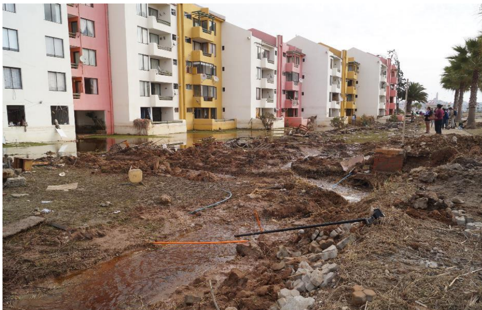
Figure 6.10. Flooded buildings at Avenida Costanera in the area of Coquimbo and tsunami debris.
