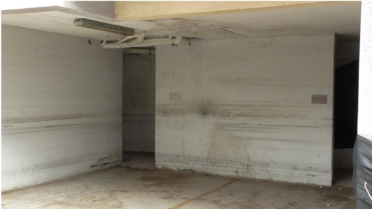
Figure 6.8. Flooding of the first story at Costa Mansa building (29.960144S; 71.332698W). Estimated run-up depth of 4.5 m.a.s.l. The structure, a 26 story RC shear wall building, was not damaged by the ground motion, however basic utilities (water, gas, electricity) were discontinued and residents were forced to move out.
