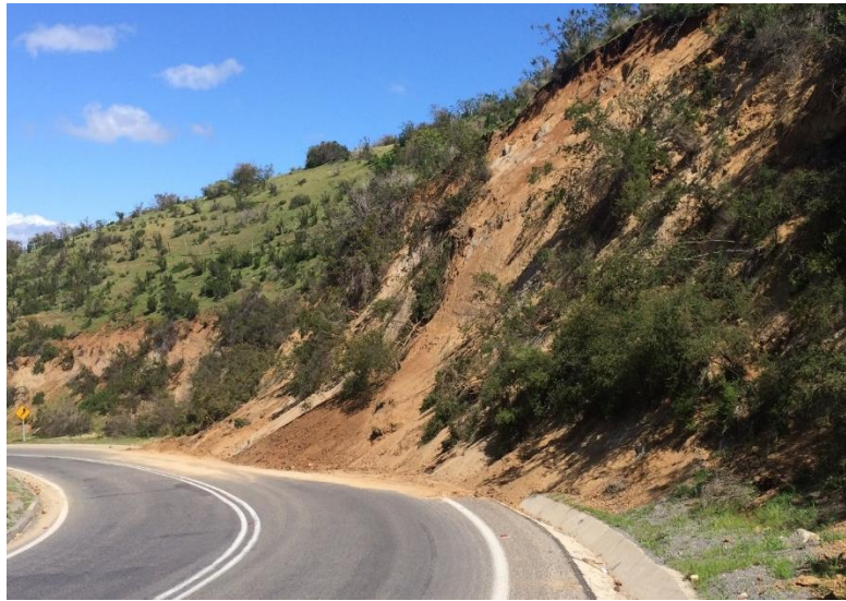
Figure 4.18. Mass-wasting in westbound of route D-85 (31.77599S; 71.32873W).
