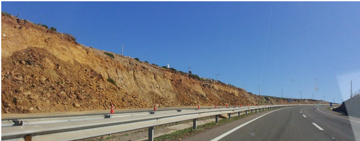
Figure 4.11. Km 338-339, southbound lane half closed from extensive slope collapse along Route 5. Field photograph looking north from the northbound lane. Cones indicate the closed southbound lane.
