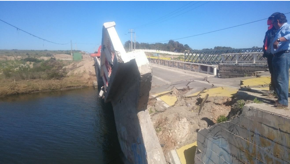
Figure 5.25. Field photograph looking south of the D-420 bridge. Northern end of the bridge has a vertical step where it failed during the earthquake, likely due to lateral spreading during liquefaction. People shown for scale (30.260784S; 71.481196W).
