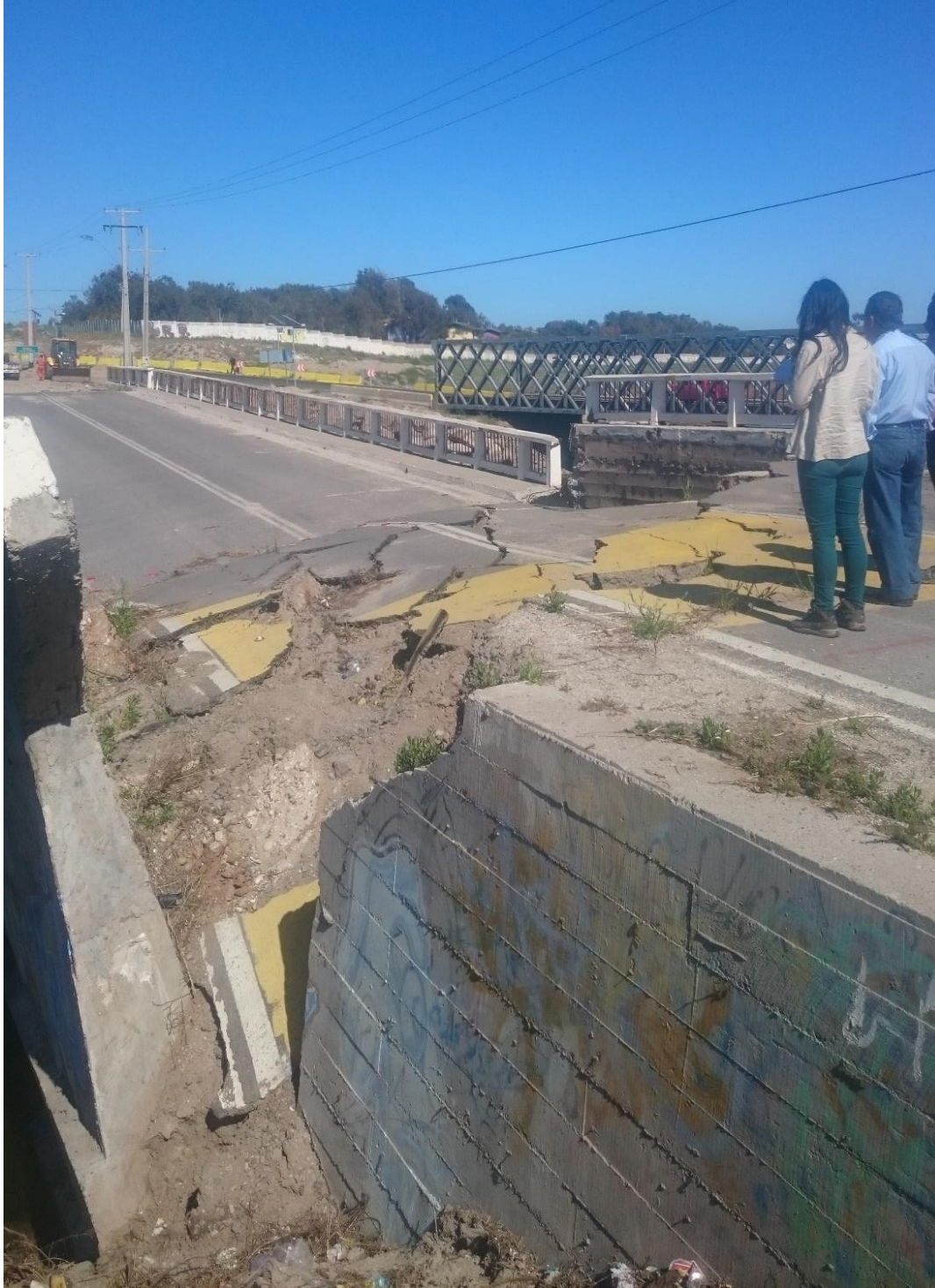
Figure 5.26. Field photograph looking south of the D-420 bridge. Northern end of the bridge has a vertical step where it failed during the earthquake – likely during liquefaction induced lateral spreading. Note the new steel bridge in the background on right (30.260784S; 71.481196W).
