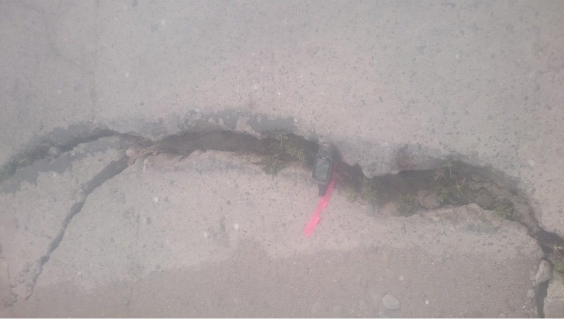
Figure 5.18. Field photograph showing concentric fractures in the concrete roadway which are accommodating the vertical and horizontal soil deformation underneath. GPS is 15.0 cm long and 5.5 cm wide for scale. Note the soil in the cracks and plants growing which suggests these cracks formed during previous earthquakes here (i.e., liquefaction during previous events took place here, which caused the formation of the cracks). The soil and plants lived here until the 2015 earthquake caused another round of liquefaction and further lateral spreading and subsidence (29.95068S; 71.29456W).
