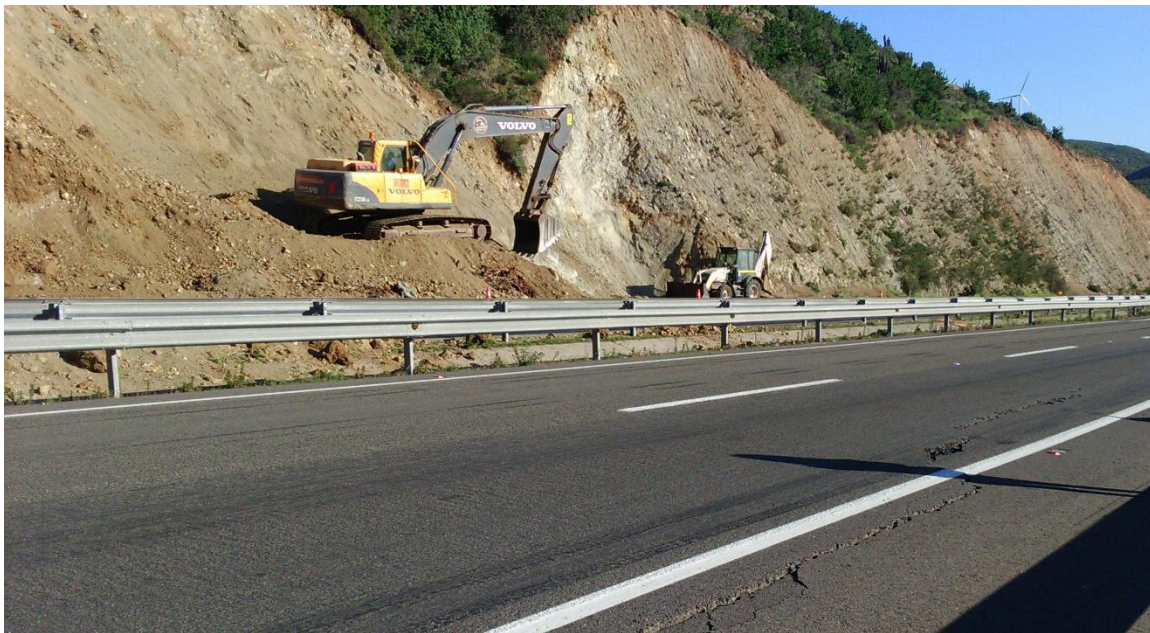
Figure 4.13. Km 287, southbound lane (photo looking north from northbound lane). Slope failure closed entire southbound lane, (note debris in median between lanes and excavator clearly the deposit). Deposit was estimated at 150-200 m 3 (based on discussions with clearing crew and evidence on the ground). Although not related to the slope failure note the cracks in the road due to slope settlement to the East in the foreground (GPS RF3: 31.37990S 71.58963W).
