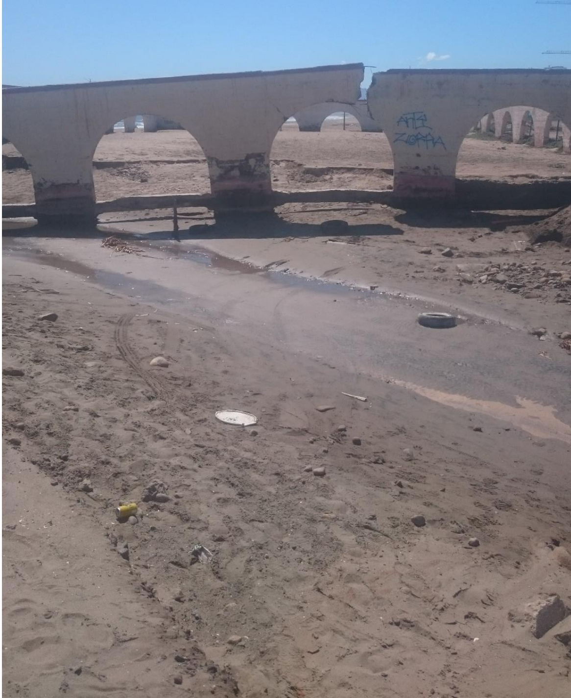
Figure 5.6. Field photograph looking north from El Faro towards the adjacent structure that shows clear differential settlement (down to the Southwest) with damage to the arc. Scour from waves as well as liquefaction was likely at this site (29.90541S; 71.27411W).
