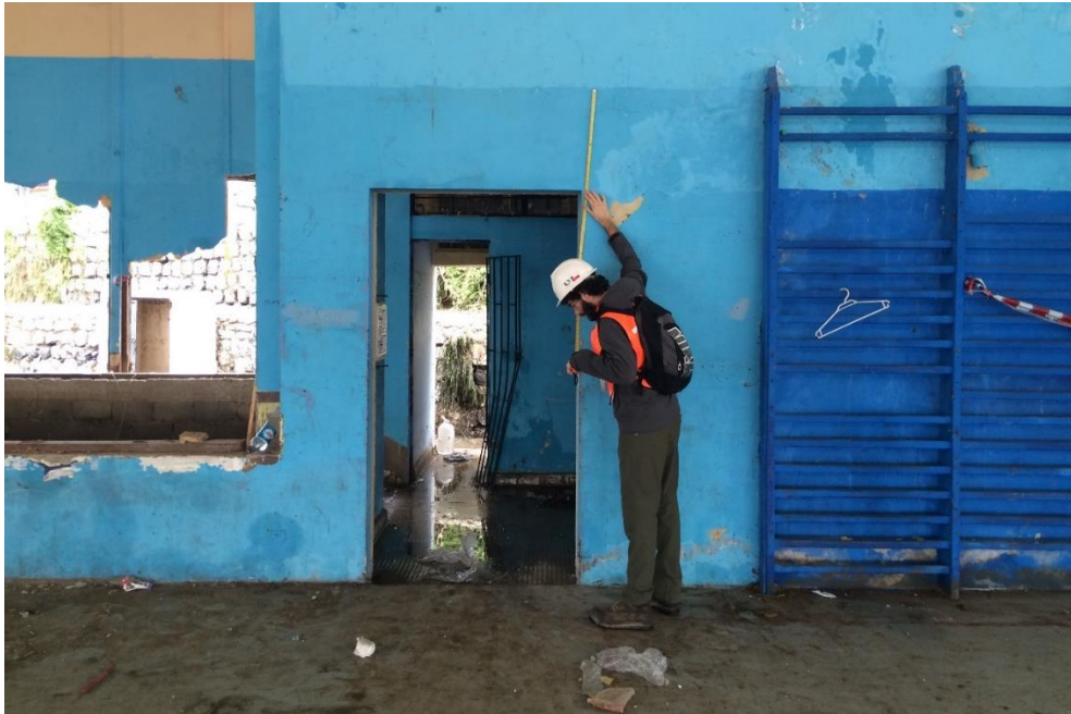
Figure 6.9. Flooding of Liceo Diego Portales's gymnasium located in Avenida Costanera, Coquimbo (29.953371S; 71.336161W). The structure is a steel frame building which sustained no structural damage from the earthquake; non-structural components such as division panels, peripheral fences and utilities were washed away by the waves
