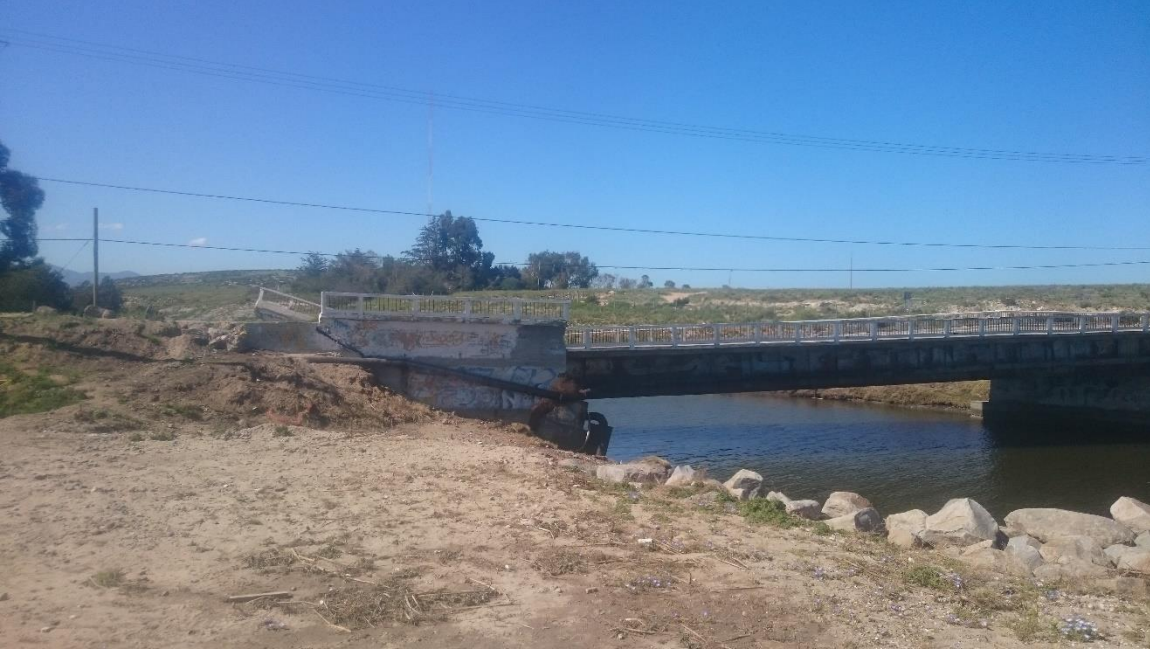
Figure 5.24. Field photograph looking east of the D-420 Bridge. Northern end of the bridge has a vertical step where it failed during the earthquake likely during liquefaction (30.260784S; 71.481196W).
