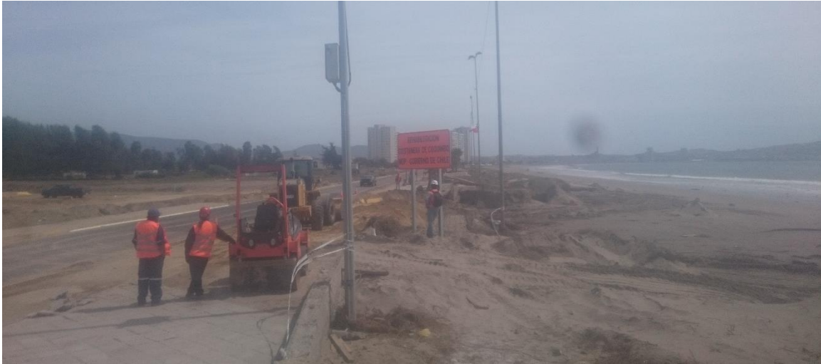
Figure 5.11. Field photograph of the destroyed road location on October 5, after the road was repaired and fully functioning (29.95368S; 71.30173W).
