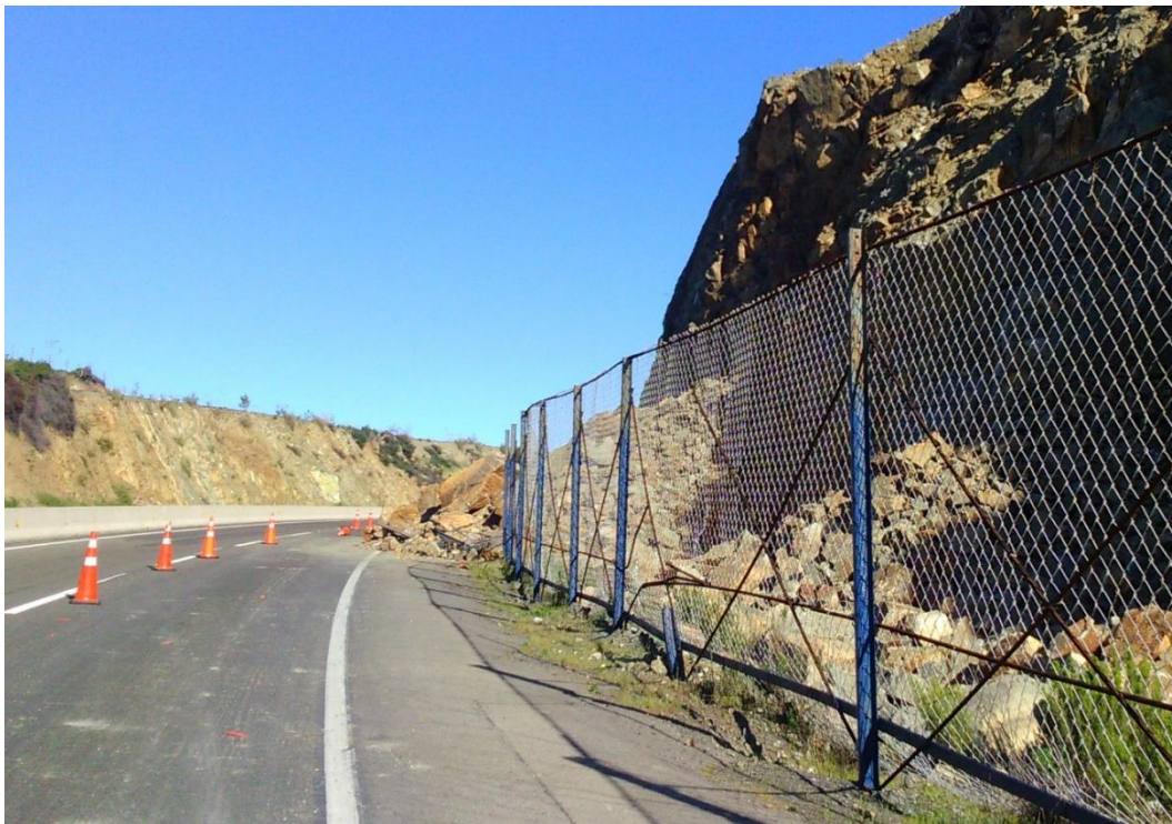
Figure 4.4. Km 305 northbound lane looking north showing how the rockfall fences failed during a cut slope collapse (GPS RF5: 31.23193S; 71.58976W). Note the fresh rockfall in the foreground, behind the fence) of the photo which then builds to a large debris cone in the background.
