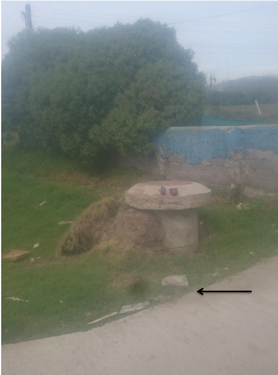
Figure 5.21. Field photograph of the same Los Pescadores street sewer portal however 8 days after the first photograph (and after a number of M_w 6+ aftershocks). Note that the services have continued to float and is now ~25 cm higher than the first photos (Black arrow indicates a line in the concrete portal that was below ground surface during first set of observations). The top of the manhole is also more tilted ( >5 degrees) during this second set of observations. This shows that liquefaction occurred during some of the aftershocks of this sequence (29.95068S; 71.29456W).
