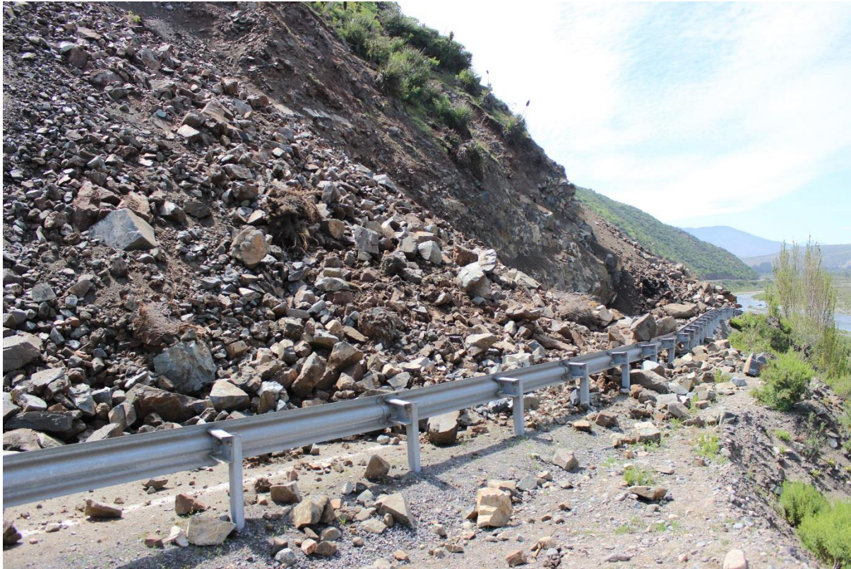
Figure 4.21. (Photo courtesy of Alondra Chamorro – CIGIDEN). As a result of massive rockfall, traffic was discontinued on Route D-75, north rim of Choapa River (31.59S; 71.41W).
