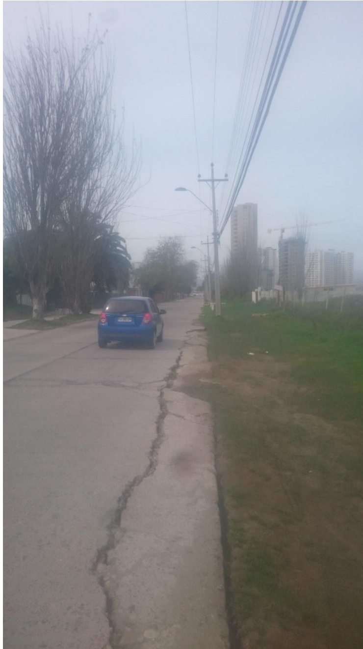
Figure 5.16. Field photograph looking north along Los Pescadores road. Note that the edge of the road has road parallel cracks where the road has failed to accommodate vertical subsidence and horizontal deformation of the soil during lateral spreading. Also note that the power lines in the back are tilted (29.95068S; 71.29456W).
