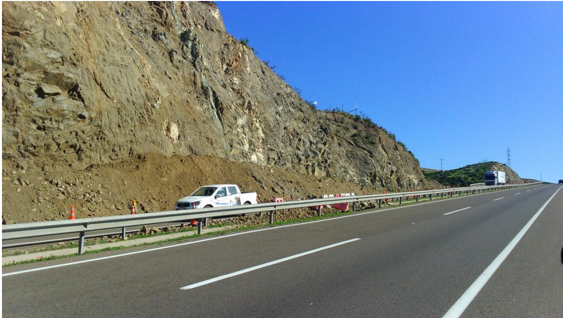
Figure 4.10. Km 350, southbound lane (photo taken looking north from northbound lane) slope failure impacted the northbound Route 5 and destroyed the mitigation fences closing the entire southbound lane. Note the debris in the median between lanes (GPS RF9: 30.87033S; 71.60181W).
