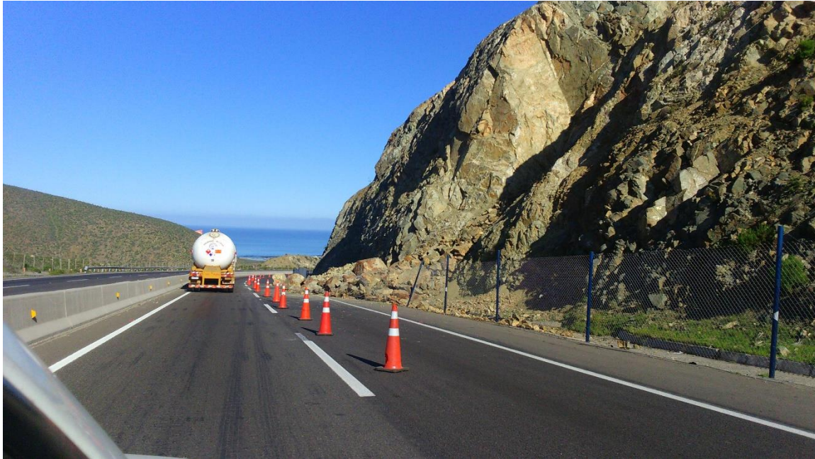
Figure 4.7. Km 334, northbound lane, rock slope failure looking north. Rockfall mitigation fences were destroyed on the northbound Route 5 with closure of both lanes after earthquake and one lane for at least 10 days later (GPS RF7: 31.00348S; 71.62430W).
