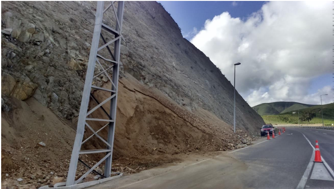
Figure 4.15. Km 280, southbound lane (photograph looking north from the southbound lane). Rockfall closed one lane, damaged streetlight and exit sign (GPS RF2: 31.44367S 71.56376W). Note that much of the deposit had been cleared prior to this photo being taken.
