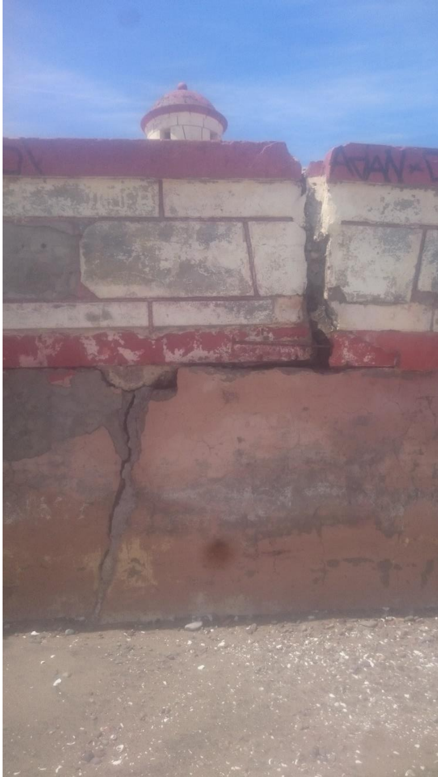
Figure 5.5. El Faro outer wall (Western, adjacent to sea) showing open fractures due to differential settlement during liquefaction perhaps in conjunction with wave scour (29.90541S; 71.27411W).
