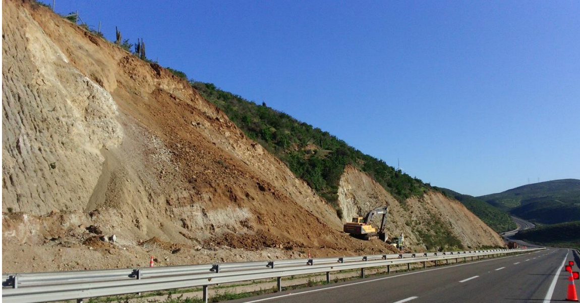
Figure 4.12. Km 287, southbound lane (photo looking north from northbound lane). Slope failure closed entire southbound lane, (note debris in median between lanes and excavator clearly the deposit). Deposit was estimated at 150-200 m 3 (based on discussions with clearing crew and evidence on the ground) (GPS RF3: 31.37990S; 71.58963W).
