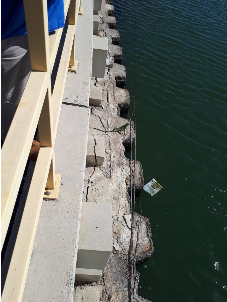
Figure 30: Looking south. The wall of the Costa Sur facility's cooling water outflow channel suffered fractures parallel to the water line. Adolescent iguana for scale (18.002N, 66.754W).
