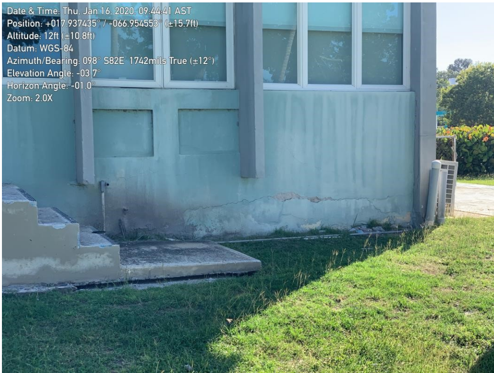
Figure 21. Separation between ground surface and staircase in the back of the building due to ground settlement
