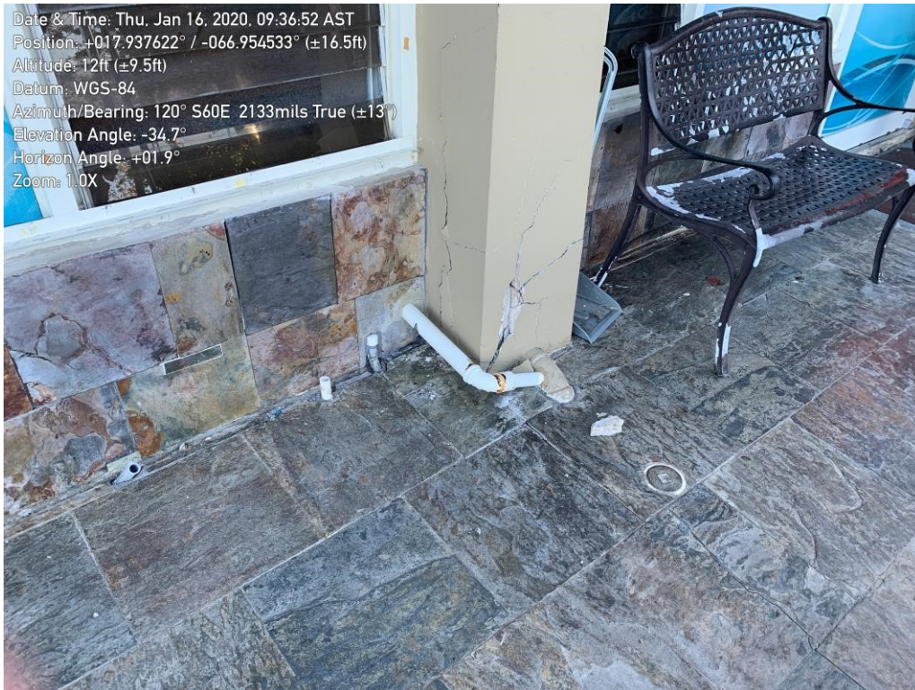
Figure 26. Cracks in column and broken PVC pipe due to ground settlement.
