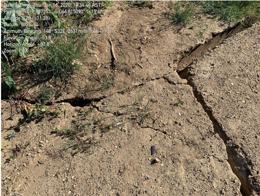
Figure 66. Detail of the ground settlement in the main road and north abutment connection shown in previous figure.
