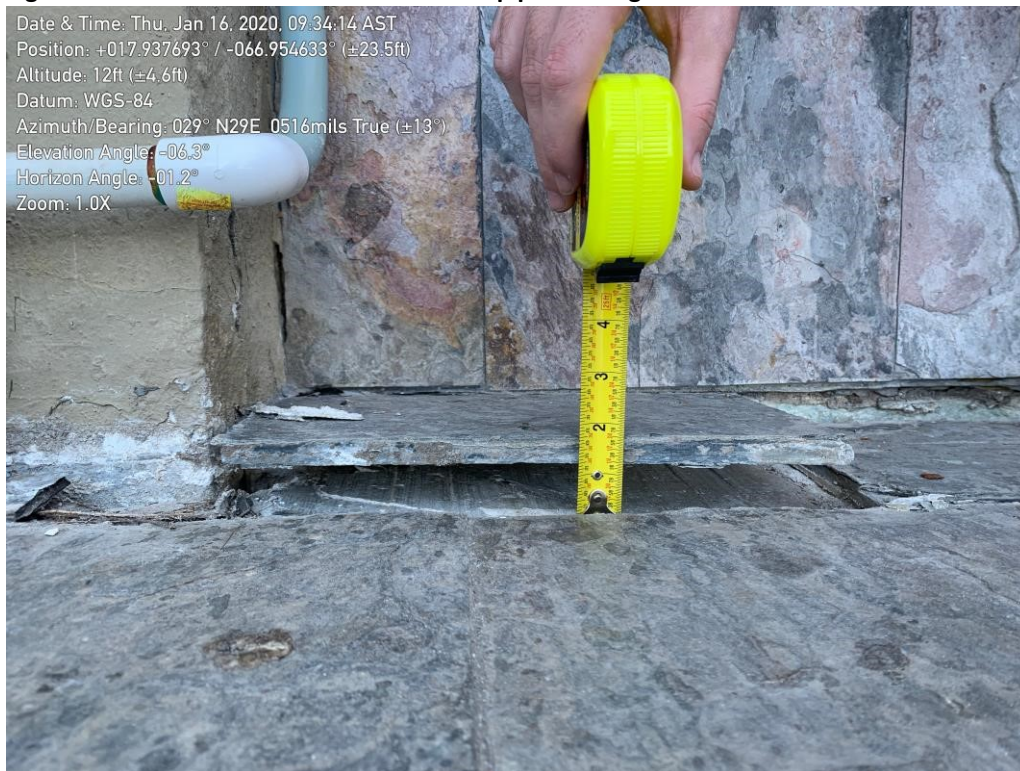
Figure 27. Hanging tile due to ground settlement. Gap in between the floor slab and the wall of approximately 1.5 inches.
