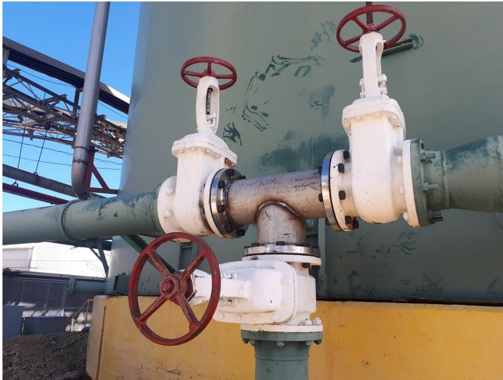
Figure 34. At one of the two water tanks immediately adjacent to the plant the center pipe piece (seen here without paint) was damaged and resulted in water discharge around the base of the tank. At Costa Sur facility (18.002N, 66.754W).
