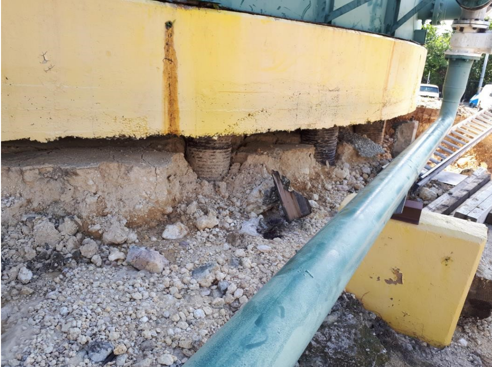
Figure 35. Scour of earthen material between pile cap and corrugated piles. New replacement section (pipe) seen in upper right of photograph (without paint). Scour was mainly on the north side of the structure (18.002N, 66.754W).
