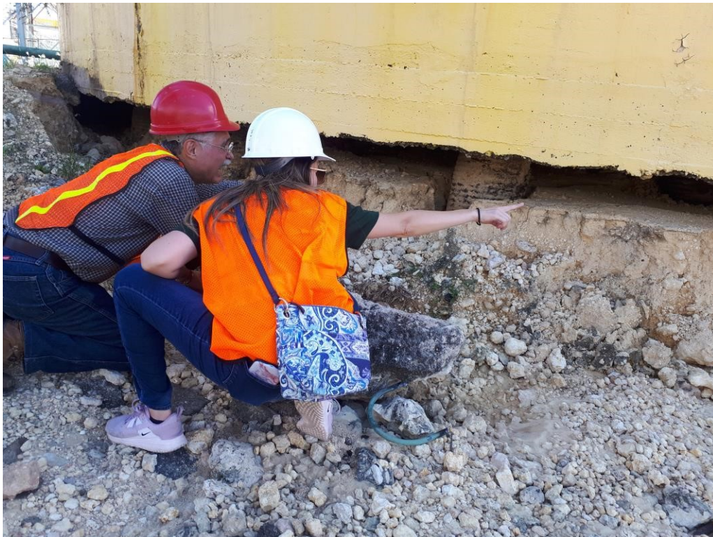
Figure 36: Members of the GEER team study the foundation scour site. Pile tilting seems to have occurred during pile driving (18.002N, 66.754W).
