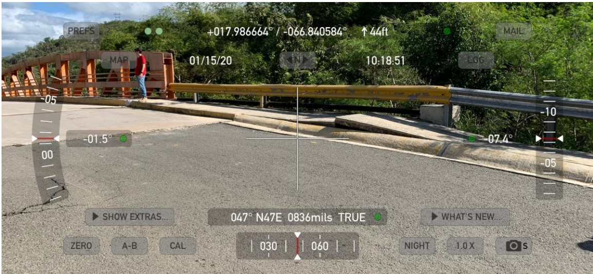
Figure 58. Side view of the sidewalk displacement.
