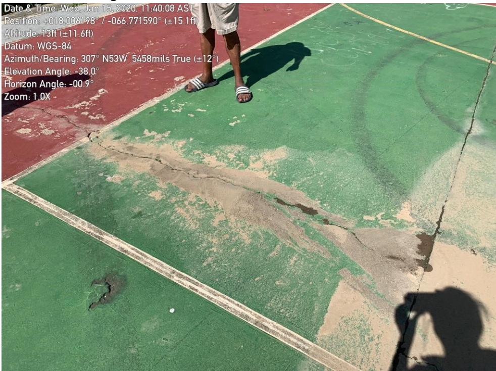
Figure 46. More ground cracks and sand ejecta at the community basketball court.
