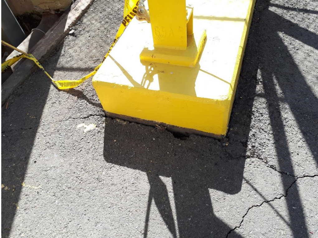
Figure 32. Similar to the previous photograph, pavement settlement at the base of a support structure. At the Costa Sur facility (18.002N, 66.754W).
