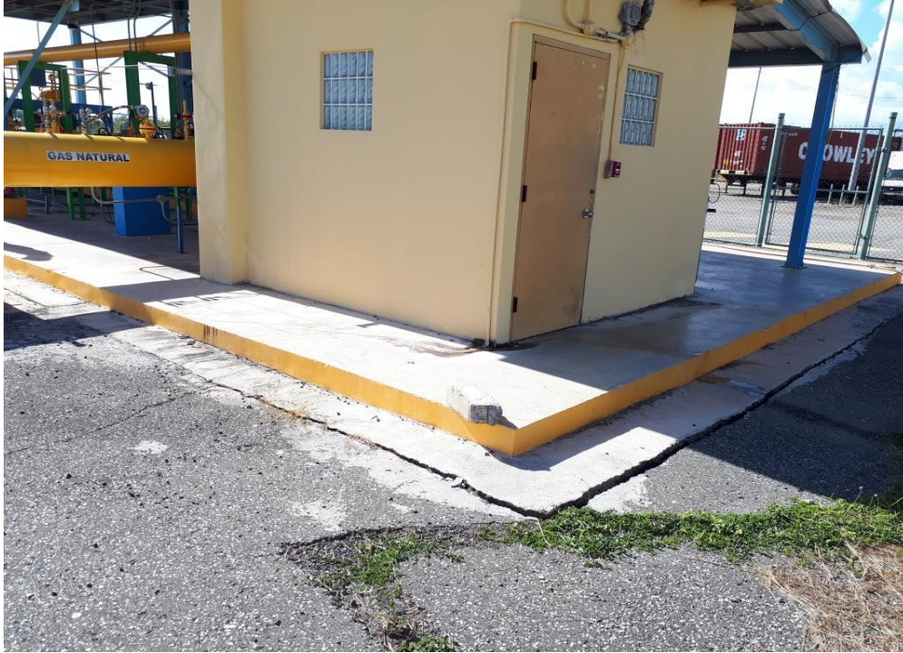
Figure 33. Settlement around the foundation of a small building near the natural gas pipeline at the Costa Sur facility (18.002N, 66.754W).
