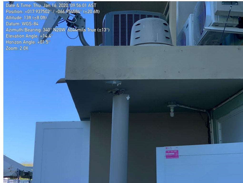
Figure 23. Displacement between a column and the main structure.
