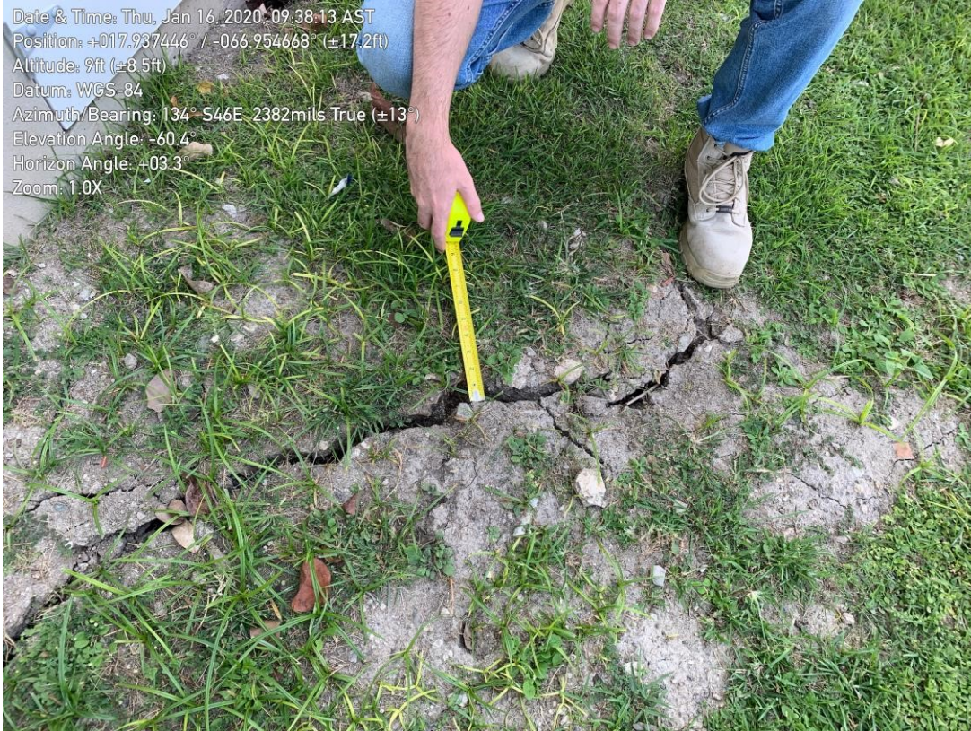
Figure 20. Cracks due to ground settlement at the site. Cracks like this were observed all around the perimeter of the structure.
