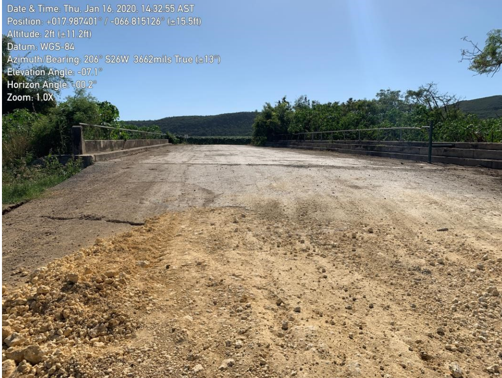
Figure 64. Settlement and ground cracks due to lateral spreading in the mango fields bridge in Tropical Fruit farm that gives access to Playa Ventana.
