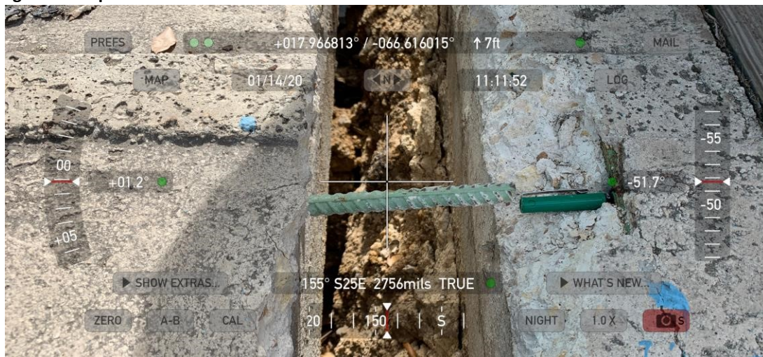
Figure 18. Exposed rebar at the joint of the concrete-wood structure.
