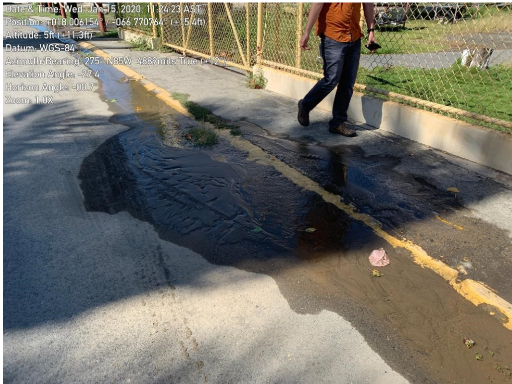
Figure 49. Broken water pipe and sand ejecta.
