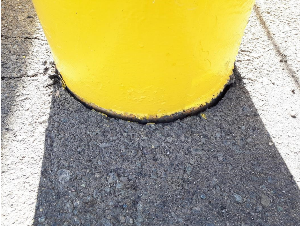
Figure 31. Looking southwest. One of the columns near the waterline. Pavement has detached and settled, as visible along paint line. At the Costa Sur facility (18.002N, 66.754W).
