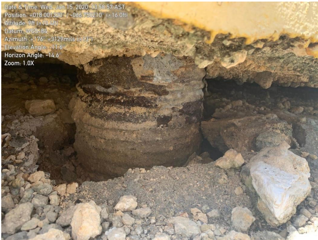
Figure 37: Close view of one of the piles showing some corrosion at the scour site. At the Costa Sur facility.
