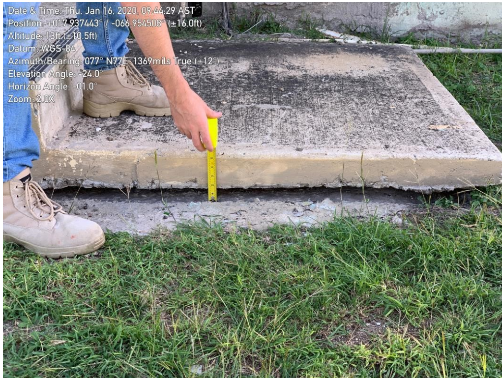
Figure 22. Detail of the separation shown in the previous figure. A gap of approximately 2 inches can be observed.
