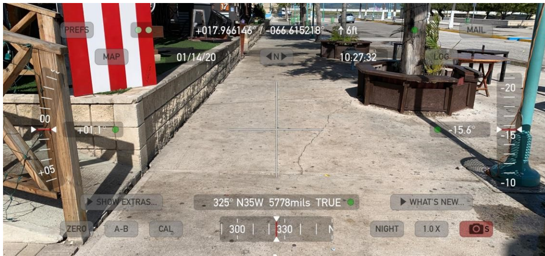
Figure 16. Ground cracks and separation of the boardwalk structure and sidewalk slab.
