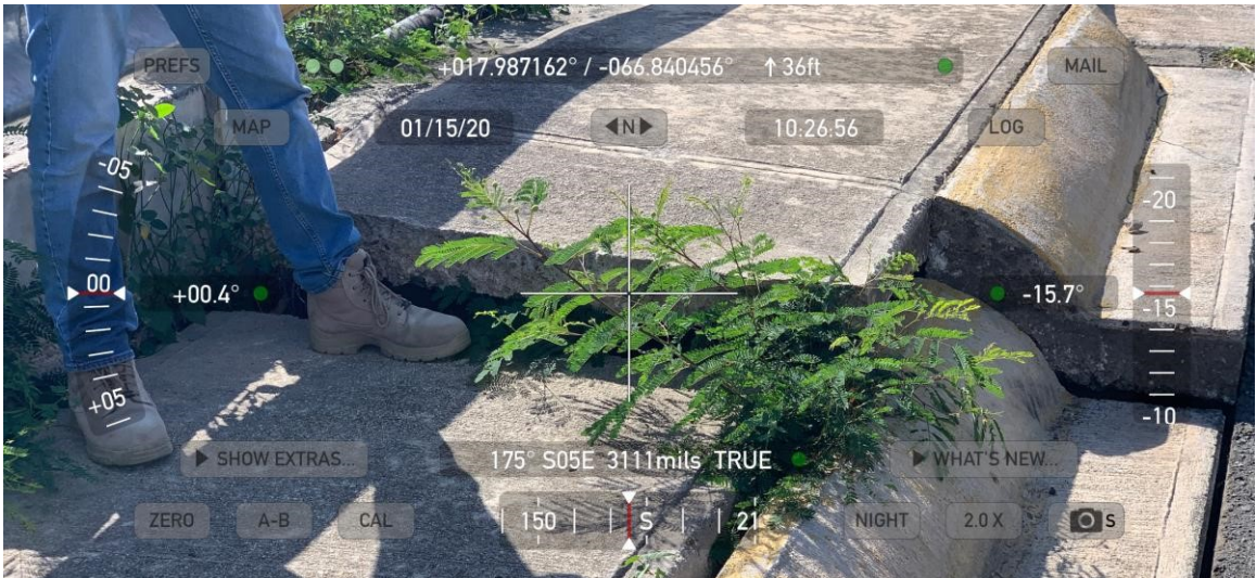
Figure 62. Detail of the sidewalk damage in the north abutment of PR-335R bridge over the Rio Yauco.
