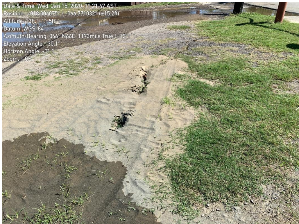
Figure 48. Sand ejecta in the parking lot of a restaurant.
