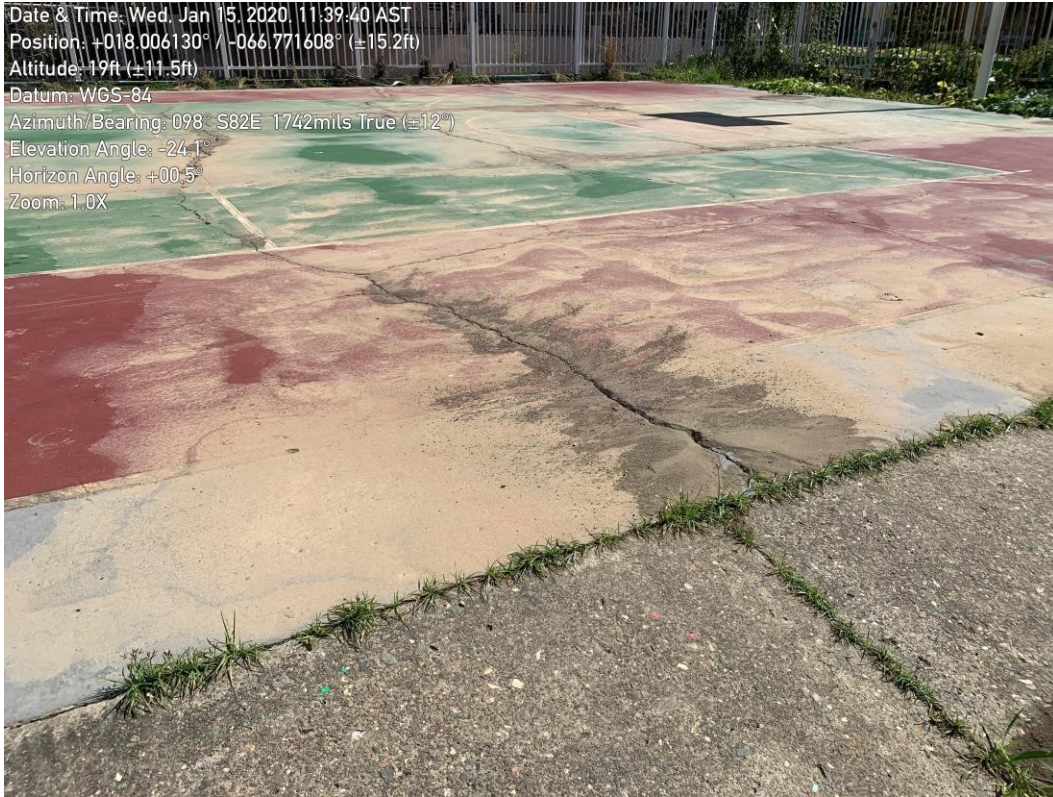
Figure 45. Ground cracks and sand ejecta at the community basketball court. Sand at this site was a silty sand. This crack ran through the whole width of the basketball court.
