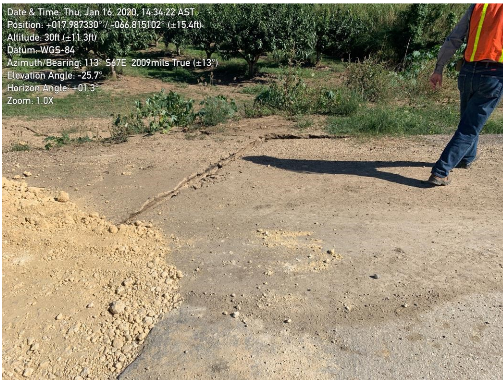
Figure 65. Ground settlement in the bridge north abutment also seen in Figure 64.
