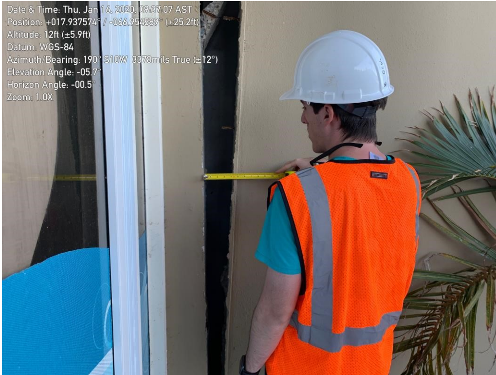
Figure 24. Gap in the connection of the original structure and the added structure in the back side of the building.
