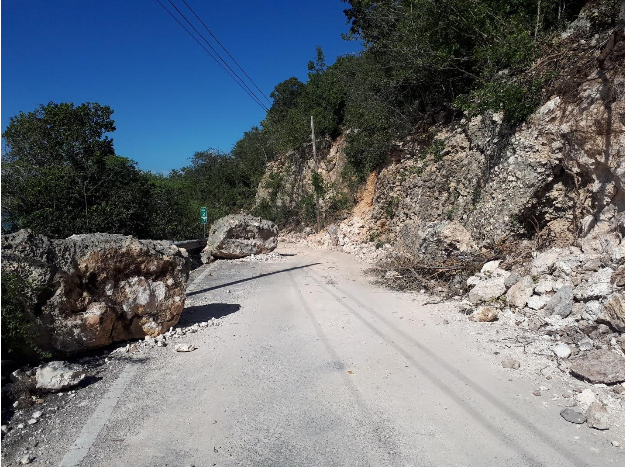
Figure 54: Rock fall along PR-333 km 2.7 in Guánica.
