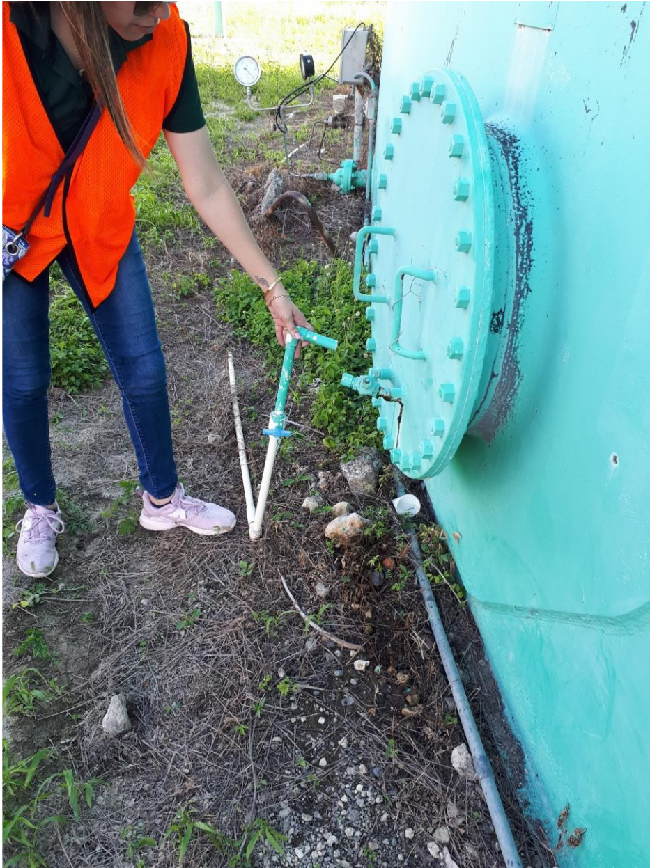
Figure 39: On the eastern base of the tank seen in previous figure, a severed PVC pipe displays a few inches of offset, suggesting minor settling of the structure (18.002N, 66.754W).
