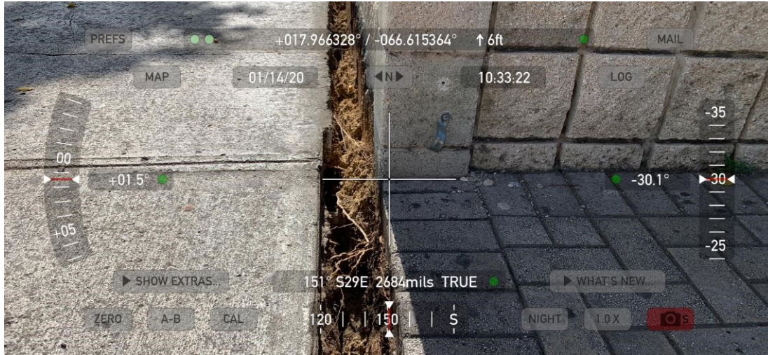
Figure 17. Separation of the sidewalk slab and the boardwalk structure.
