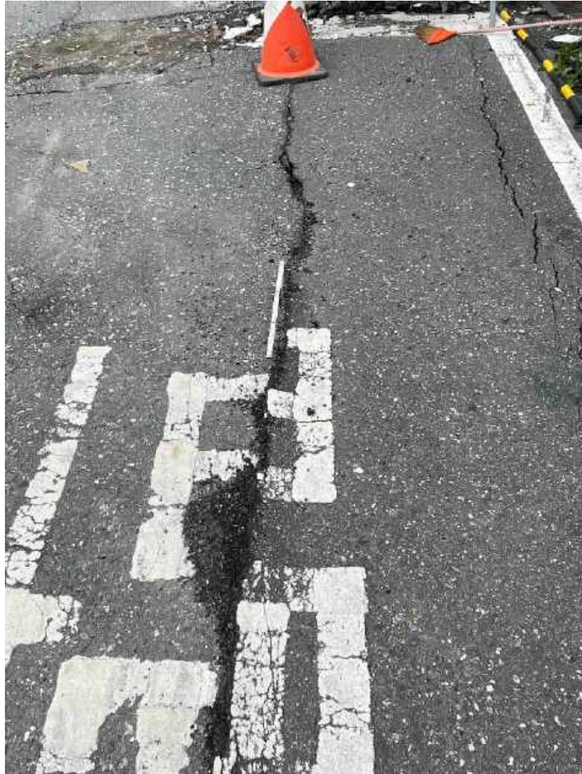
Figure 4.11: Surface rupture coincident with fault-parallel sewer line. Discrete LL offset is 18 cm. Lat: 23° 10' 24.693599", Lon: 121° 14' 54.185999"
