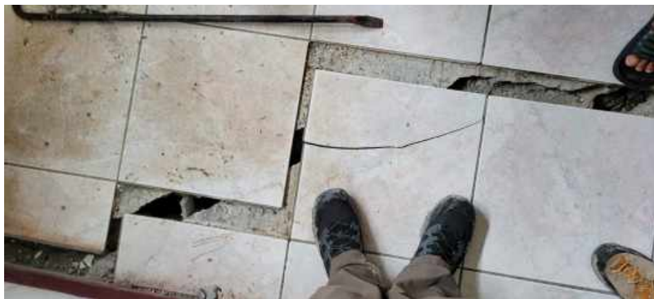
Figure 4.14: Partial collapse of URM structure along the LVF. Rupture propagated beneath the house. Lat: 23° 10' 26.201999", Lon: 121° 14' 54.605400"
