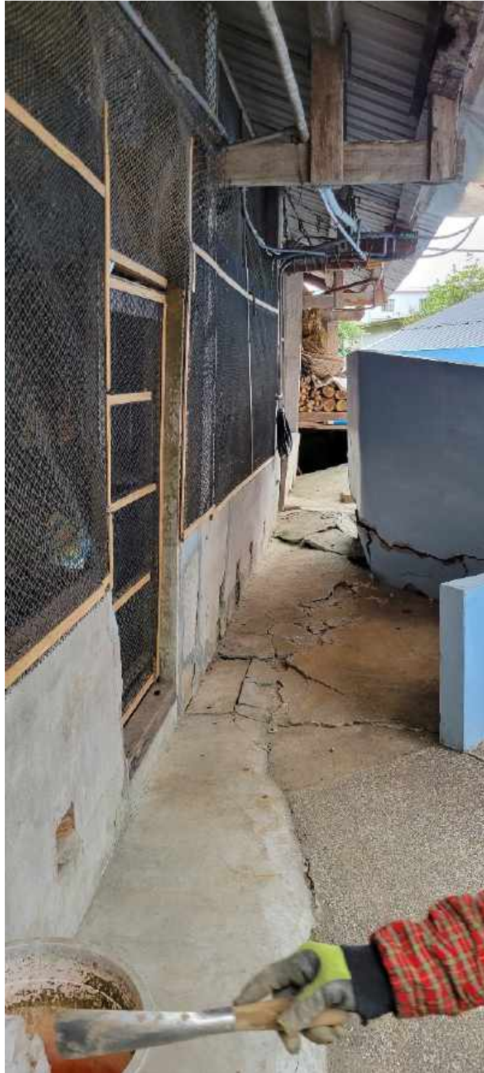
Figure 4.18 (d) Pavement buckling. Lat: 23° 10' 28.520039", Lon: 121° 14' 55.023719"
