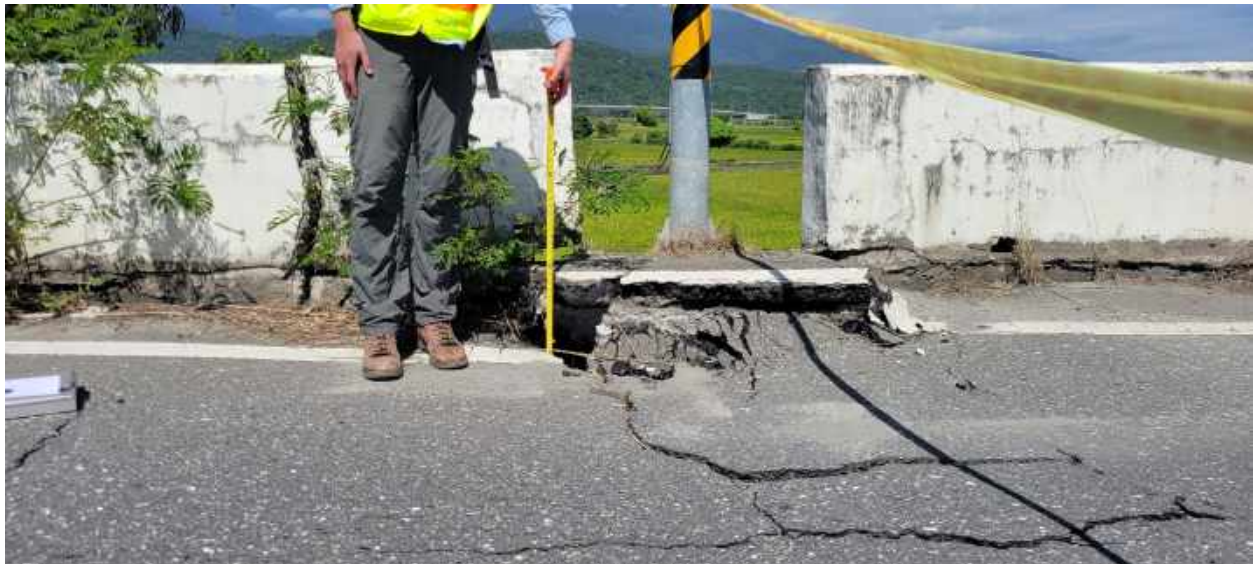
Figure 5.38. Settlement near the light post foundation in the east abutment (23.38617° 121.33741°)
