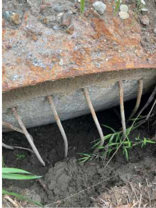
Figure 5.11. View from the bottom of one of the failed pier foundations. The longitudinal rebar yielded and relatively smooth base suggesting a cold joint (23.21753° 121.27116°)
