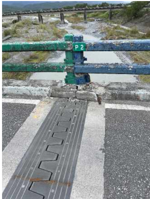
Figure 5.30. Typical damage in concrete railing at finger joints. (23.32317° 121.32758°)
