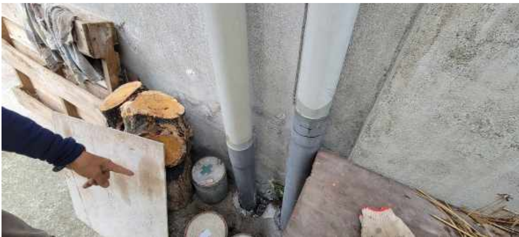
Figure 4.18 (a) Concrete damage due to relative foundation movement around water pipeline. Lat: 23° 10' 28.720199", Lon: 121° 14' 55.052159"
