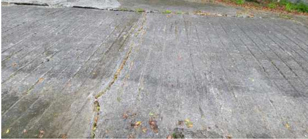
(d) Cracks in walkway between private property and Fuli Junior High School. Whether this crack was directly caused by the September 18 earthquake is uncertain. Lat: 23° 10' 28.848720", Lon: 121° 14' 56.038199"
