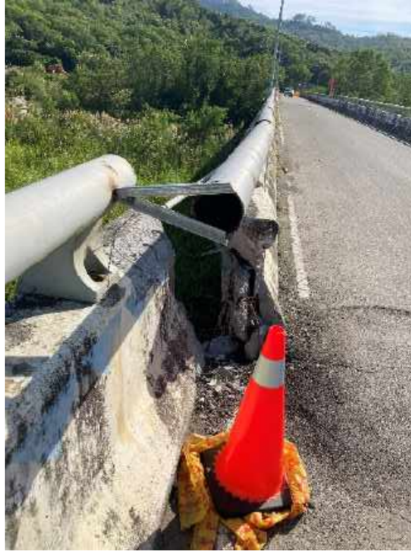
Figure 5.3. Lateral offset, looking towards the east abutment. (22.97484° 121.17017°)
