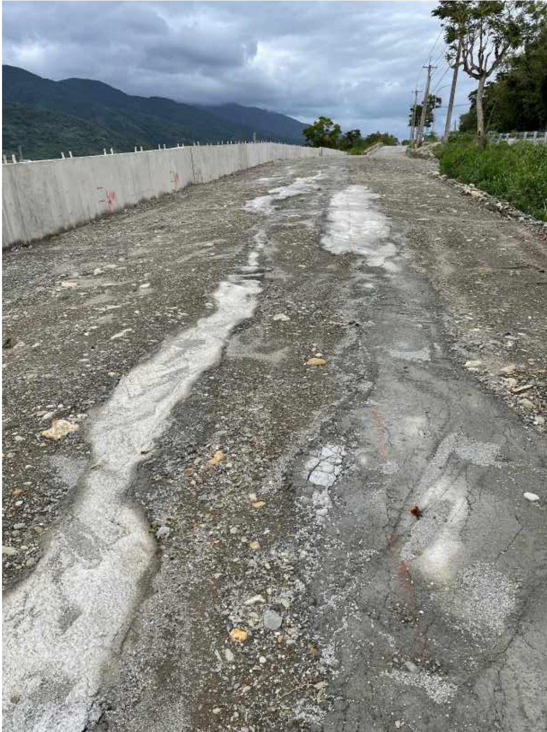
Figure 4.6: View looking north and ground cracking areas “repaired” with concrete. Failed retaining wall in upper left. Lat: 23° 8' 39.00048”, Lon: 121° 14' 12.52428”.
