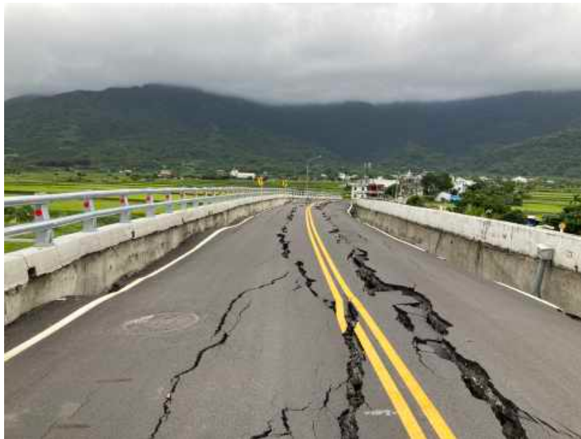
Figure 5.41. Roadway cracks and settlement in the east abutment looking east (23.38520° 121.34710°)
