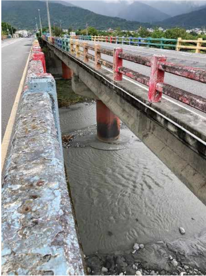
Figure 5.28. View of the substructure of the North Yuli bridge. Similar structural components on the south bridge. (23.32320° 121.32780°)
