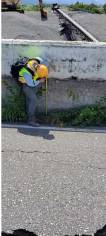
Figure 5.37. Roadway settlement at the south back-to-back concrete gravity wall in the west abutment (23.38629° 121.33811°)
