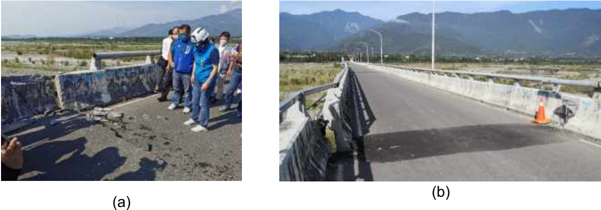
Figure 5.2. a) Damage between adjacent bridge spans buckling roadway, concrete barrier, and metal guardrail (United Daily News), looking south; b) repaired roadway and metal guardrail damage during GEER/NCREE visit looking northwest. (22.9748° 121.1702°)
