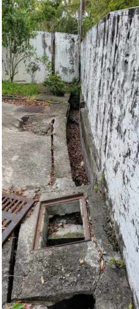
(g) Inward buckling of concrete wall. Uncertain as to whether this was a direct result of the September 18 earthquake. Lat: 23° 10' 28.223039", Lon: 121° 14' 56.014799"
