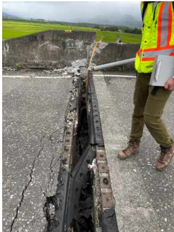
Figure 5.21. Extension of bridge joint at the west abutment. Gap approximately 25 cm. (23.26574° 121.29864°)
