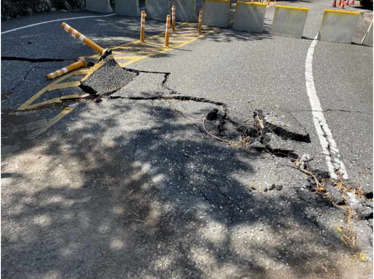
Figure 4.34: Surface rupture through the bridge approach near projected location of the LVF. Asphalt pavement buckled and locally detached. View looking southwest, Lat: 23° 15' 46.403640", Lon: 121° 18' 9.362160"
