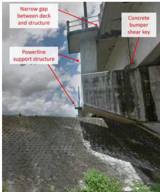
Figure 5.26. Google Street view from 2012 showing the intact powerline support structure and concrete bumper shear key (23.27468°, 121.30489°)
