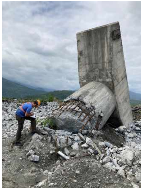
Figure 5.35. Typical view of the plastic hinges in the concrete piers (23.38630° 121.33930°)
