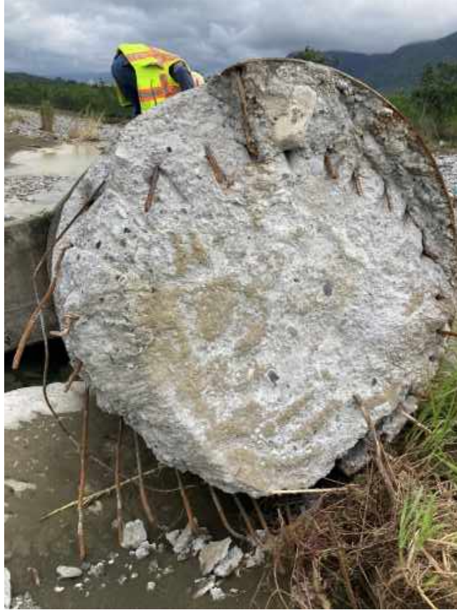
Figure 5.13. View of a failed pier with irregular longitudinal rebar spacing. Same pier as and concrete pad as Figure 5.14. (23.217653° 21.270928°)
