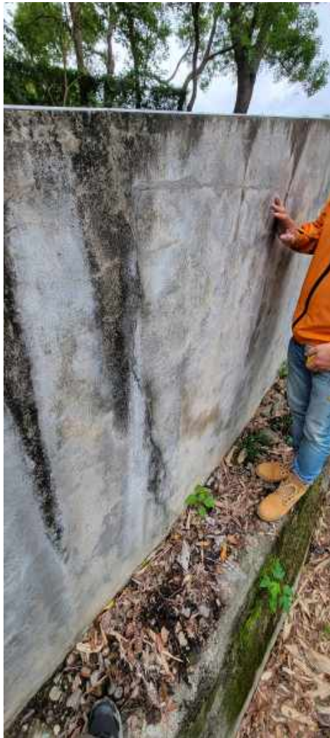
(c) Hairline fracture in concrete wall uphill from (b). Lat: 23° 10' 28.858440", Lon: 121° 14' 56.000759"
