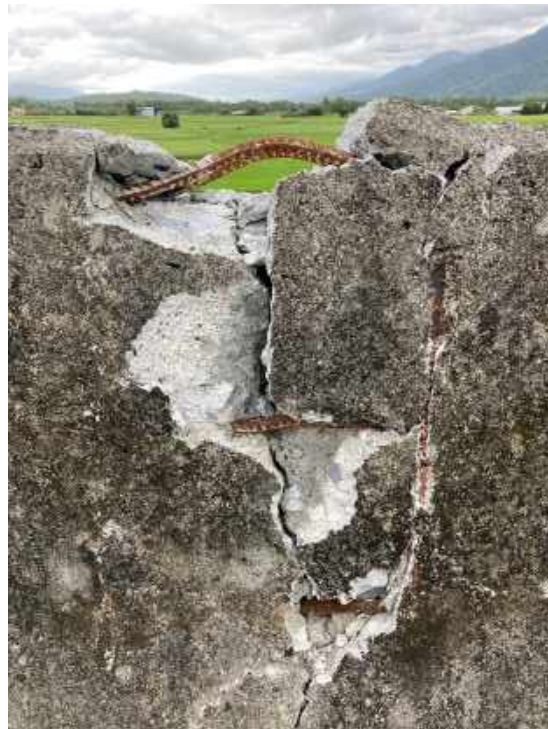
Figure 5.19. Compression buckling of concrete barrier steel reinforcement (23.26584° 121.29836°)
