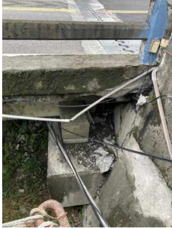
Figure 5.29. Damage to the North Yuli bridge east abutment and adjacent utility lines. (23.32233° 121.33240°)
