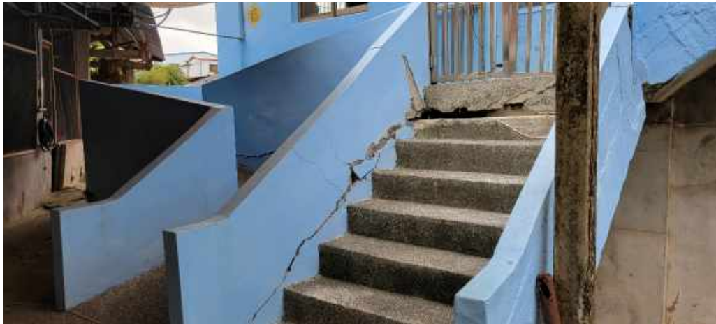
Figure 4.18 (c) Cracking in concrete stairs resulting from relative foundation displacement. Lat: 23° 10' 28.512480", Lon: 121° 14' 54.98628"
