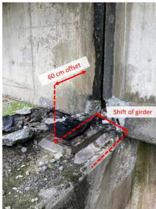
Figure 5.10. 60 cm transverse translation of the bridge girder north, and longitudinal shift of the girder towards the east abutment. (23.21459° 121.27268°)
