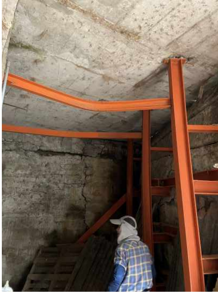
Figure 4.17: Deformation of braced concrete structure built into the LVF scarp. Deformation was largely coseismic based on owner's account. Lat: 23° 10' 27.884280", Lon: 121° 14' 54.895199"
