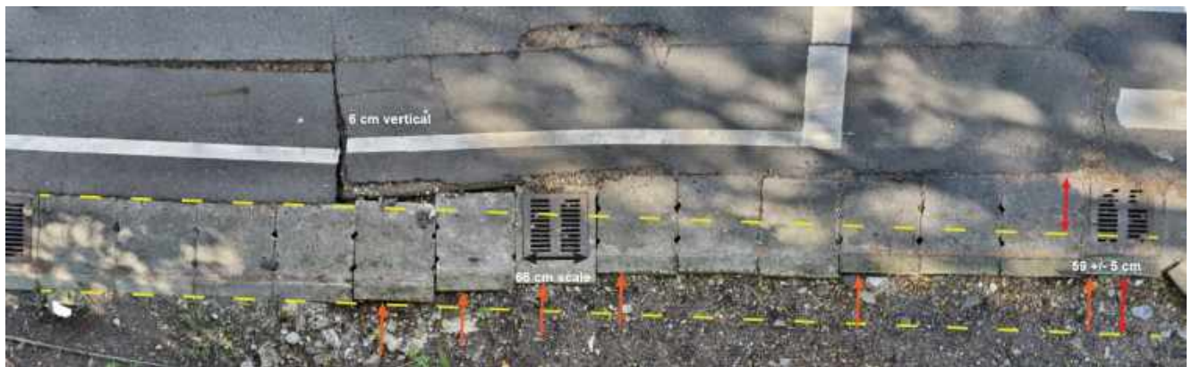
Figure 4.22: offset of sewer lateral in Fuli. The best estimate of total LL displacement is 59 cm, include possible pre-event creep and/or prior surface rupture on the LVF.
