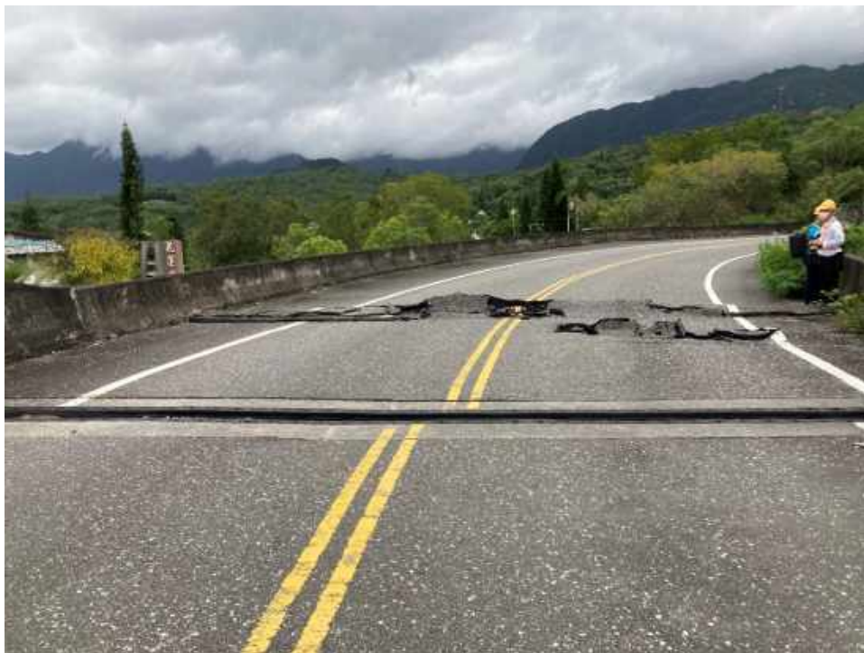
Figure 5.17. 41 cm lateral offset between bridge span and abutment. (Asphalt buckling due to surface fault rupture) (23.26452° 121.30089°)
