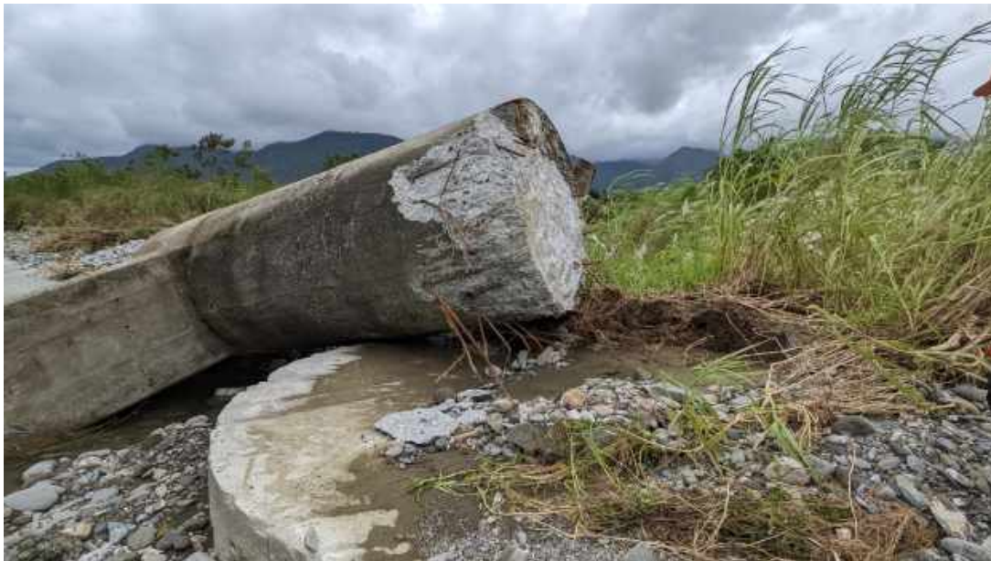
Figure 5.14. View of failed bridge pier and concrete pad. Note the yield longitudinal rebar connecting the pier to the concrete pad. (23.21771° 121.25425°)
