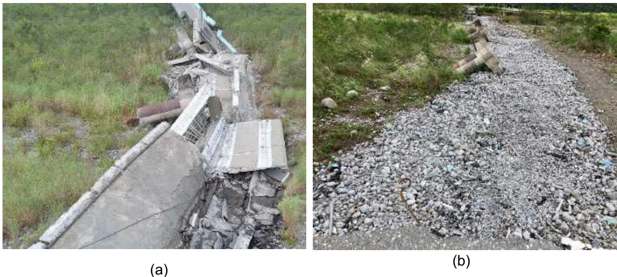
Figure 5.6. a) Failed spans and pier foundation supports at the Luntian Bridge (image curious of NCREE); b) view for concrete bridge piers after deck removal during GEER team visit in October 2022 (23.21726° 121.27172°)
