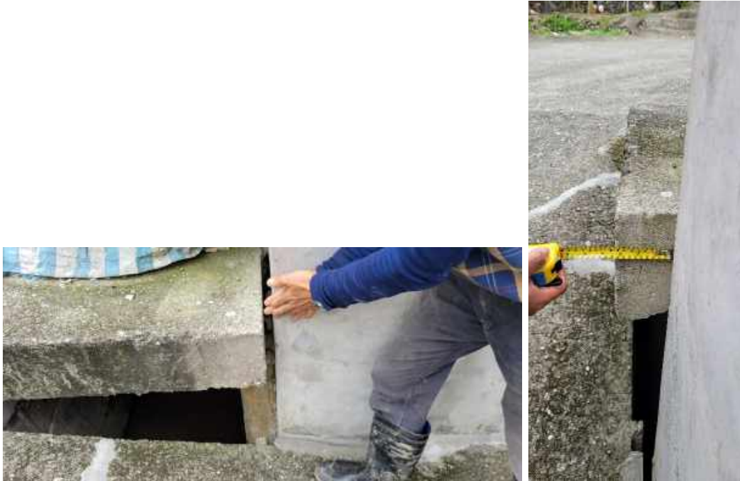
(e) Relative movement of foundation. Lat: 23° 10' 28.924320", Lon: 121° 14' 54.961080"
