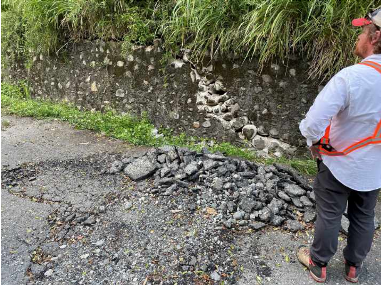
Figure 4.32: Reverse faulting through unreinforced cobble and concrete retaining wall, Lat: 23° 15' 46.403640", Lon: 121° 18' 9.362160"
