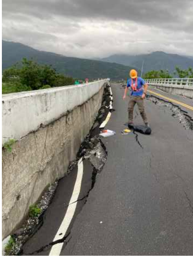
Figure 5.42. Roadway cracks and settlement in the east abutment looking west (23.38510° 121.34767°)
