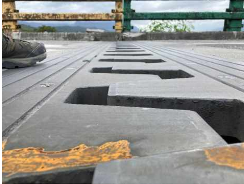
Figure 5.31. Typical differential movement at a Figure 5.joint. (23.32240°121.33194°)
