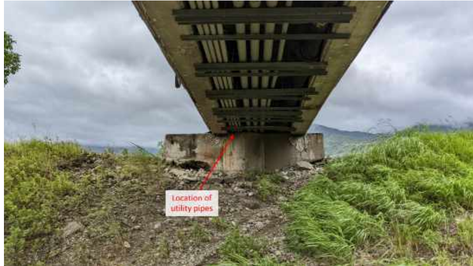
Figure 5.9. Looking west at the 2 nd pier from the east abutment following the earthquake. Note the north translation of the utility pipes from Figure 5.8. (23.21457° 121.27268°)
