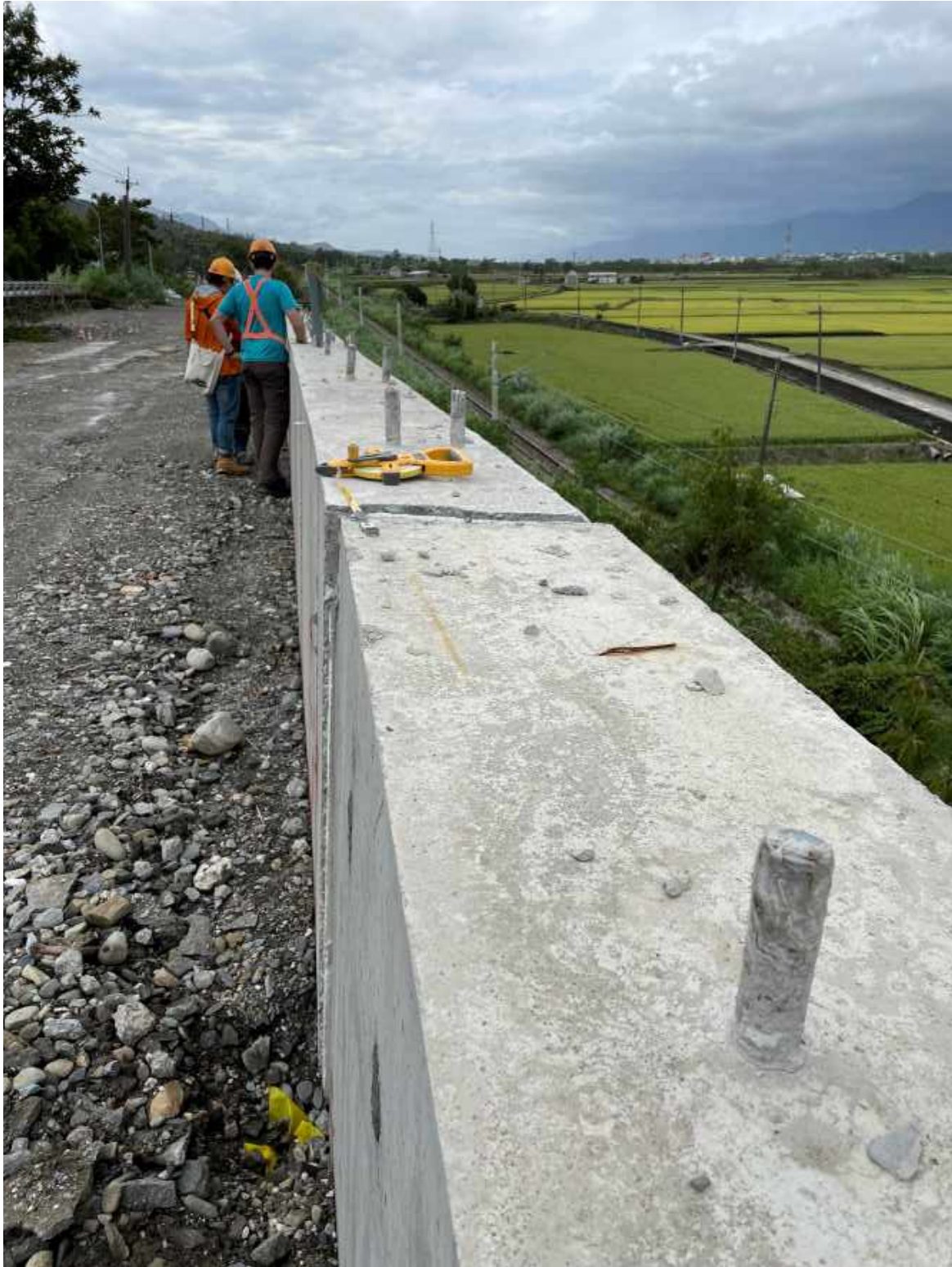
Figure 4.3: View looking south along retaining wall showing displacement of joint between 20-m wall sections. Backfill composed of river gravel, locally emplaced in lifts between geotextile. Lat: 23° 8' 43.47456", Lon: 121° 14' 13.727399".
