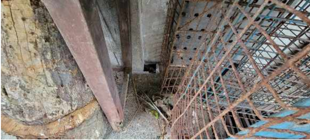
Figure 4.18 (b) Separation of concrete walls from foundation. Lat: 23° 10' 28.626959", Lon: 121° 14' 54.975479"
