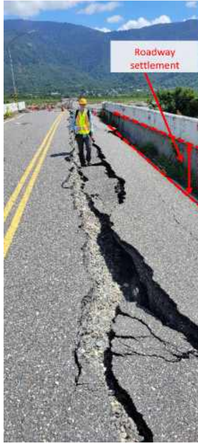
Figure 5.36. Roadway cracks and settlement in west abutment. Note (23.38625° 121.33806°)
