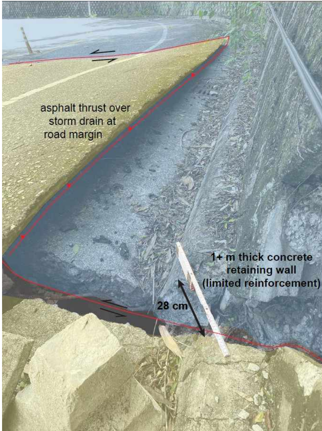
Figure 4.35: Annotated photo showing view of buckled pavement on bridge approach. Net horizontal displacement of the 1-m-thick concrete retaining wall (sparse reinforcement) was ~28 cm, Lat: 23° 15' 46.403640", Lon: 121° 18' 9.362160"
