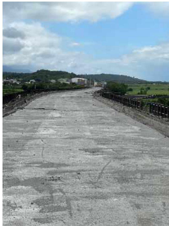
Figure 5.24. View from the bridge deck of the Dongli Railroad Bridge with the train rails removed. The twist in the deck was due to the lateral translation of the prestressed girders. (23.27829° 121.30669°)
