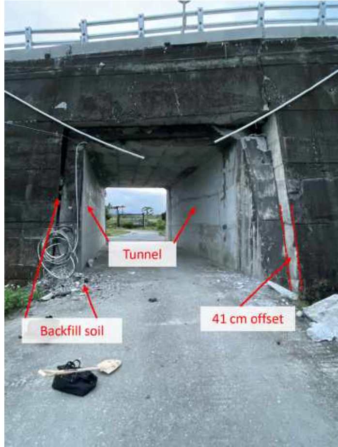
Figure 5.43. Tunnel beneath east bridge approach, 41 cm offset from gravity wall, and backfill soil that flowed from gap between the gravity wall and tunnel liner (23.38526° 121.34783°)
