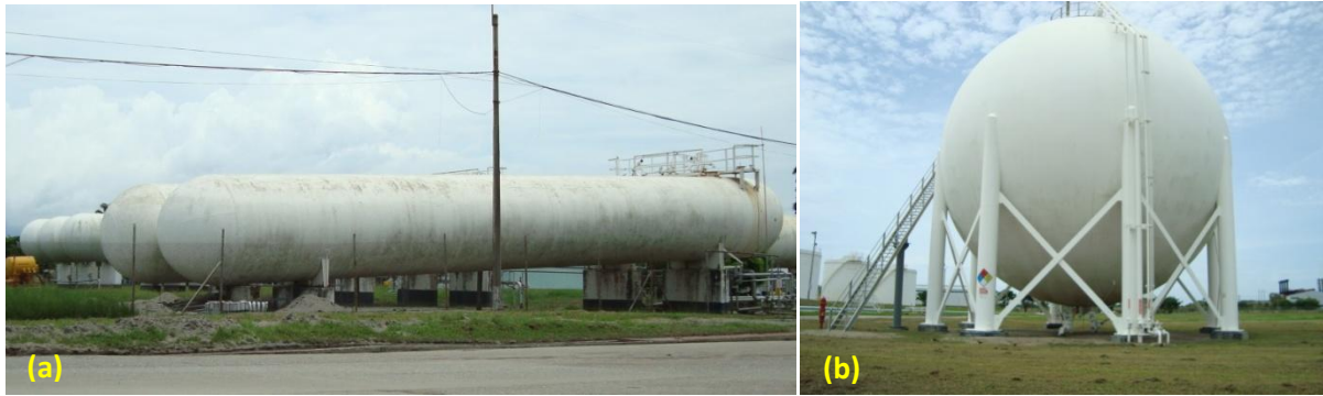
Figure 4 – (a) Tanks supported on shallow foundations sank and tilted, notice sand boil piled up next to foundation on left [6/20/2009, 1:12PM, 15.851061, -87.956882], and (b) those supported on piles performed well [06/20/2009, 1:16 PM, N15.851226, W87.958534].
