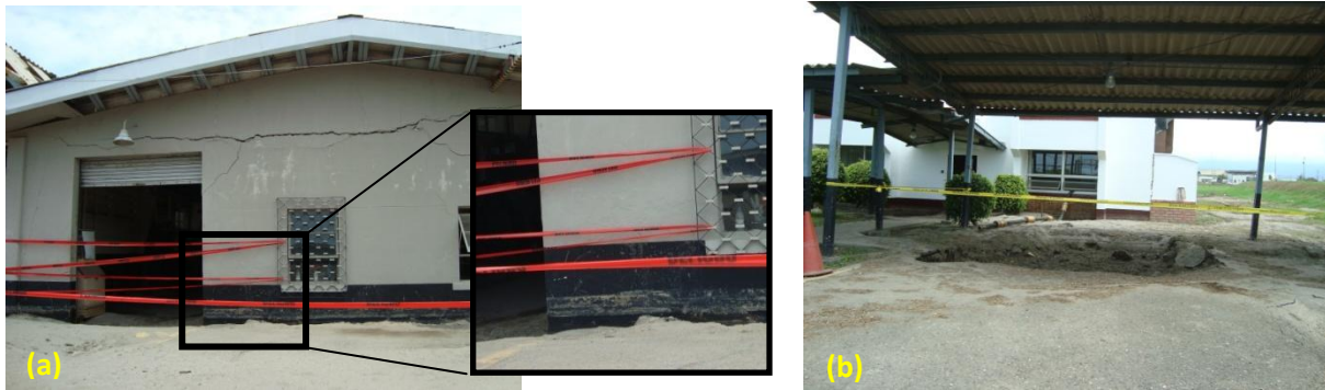
Figure 5 – (a) Buildings and small structures sank up to 3 ft and were flooded with liquefied sand [06/20/2009, 1:08 PM, N15.849851, W87.95793], and (b) vehicles sank into sand boils, see carport automobile was already extracted [06/20/2009, 1:25 PM, N15.848216, W87.958604].
