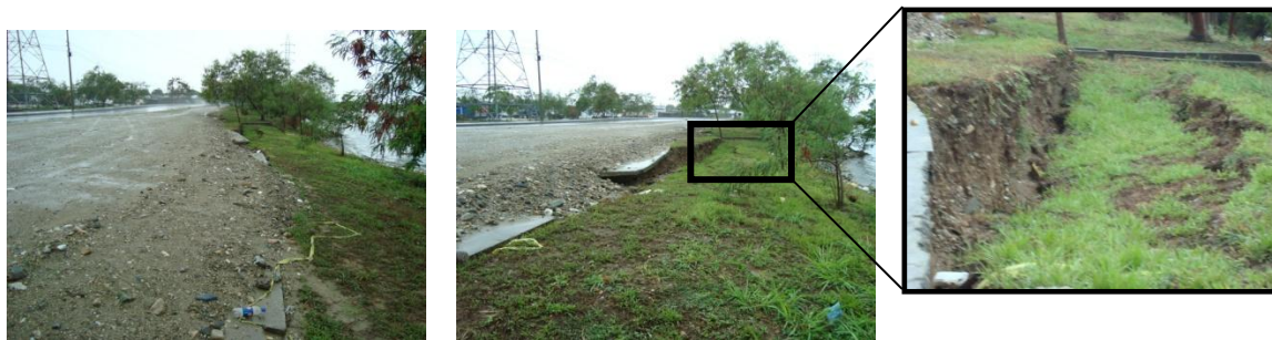
Figure 6 – Temporary repair of roadway embankment, due to lateral spreading [06/20/2009, 1:25 PM, N15.848216, W87.958604].
