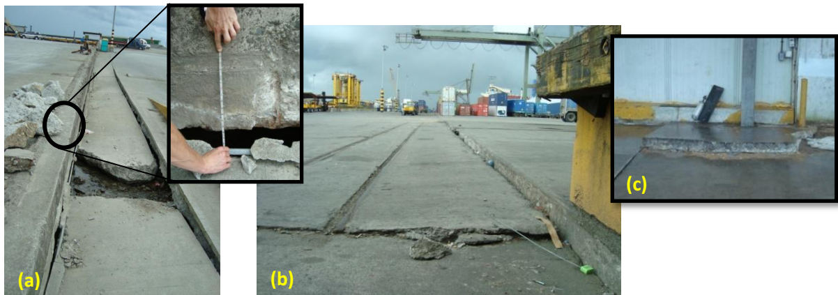
(a) Up to 0.46m at the main dock [06/20/2009, 3:37PM, N15.843718, W87.951739], (b) 0.2m near port warehouses [06/20/2009, 3:49PM, N15.8424, W87.94941], and (c) Relative foundation displacement up to 0.15m [06/20/2009, 4:00PM, N15.841912, W87.941644].
