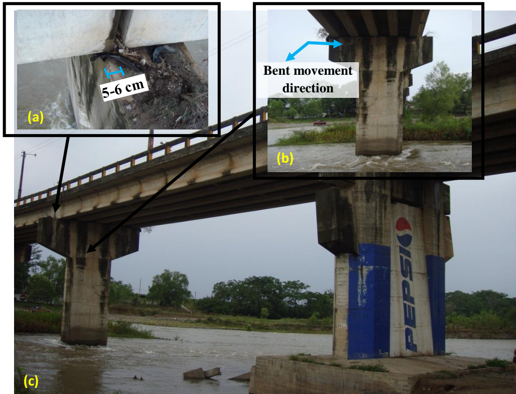
Figure 14 – Santa Rita Bridge over the Humuya River after the earthquake and before collapse
