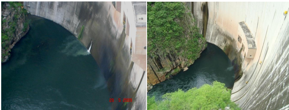
Figure 17 – (a) Turbid seepage at base of dam [05/28/2009, N15.03096, W87.747885], and (b) clear seepage at base of dam [06/21/2009, 11.55AM, 15.03096, -87.747885]
