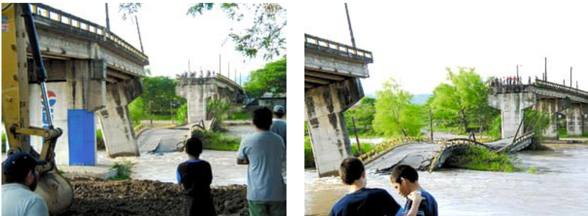
Figure 15 – Collapse of the 2 to 3 spans of the Sta. Rita Bridge over the Humuya River post-earthquake [06/28/2009, N15.191019, W87.892095] (source: LaPrensa.hn).
