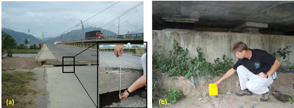
Figure 13 – Settlement of ground around abutments due to liquefaction (a) Old bridge westbound [06/19/2009, 6:36PM, N15.404409, W87.821095], and (b) New bridge, eastbound [06/19/2009, 6:52PM, N15.40422, W87.821021].
