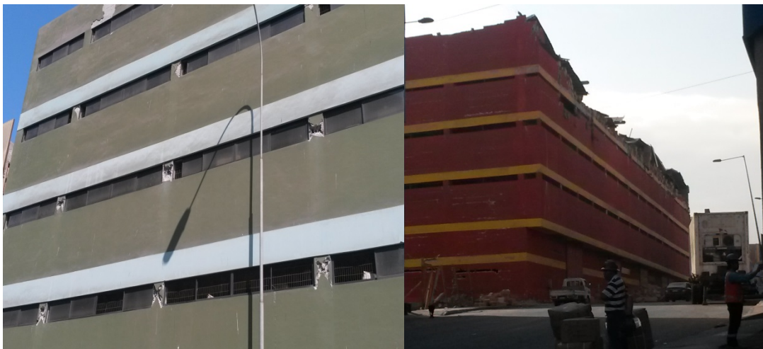
Fig. 5.7 (left) Typical short column structural damage and (right) fallen roof parapets in the ZOFRI zone.
