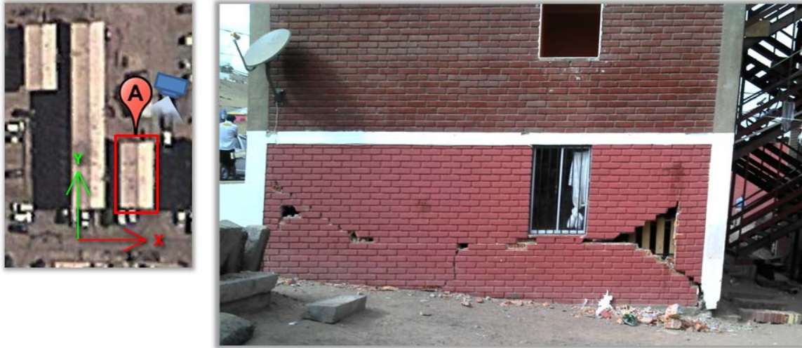
Fig. 5.14. Observed damage in buildings type A
