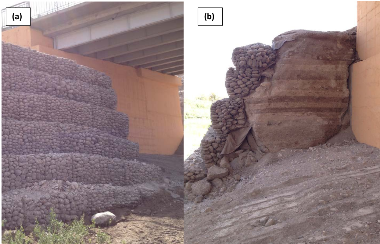
Fig. 3.8 (a) Gabion wall adjacent to the north bridge abutment and (b) tension crack adjacent to abutment behind gabion wall. (19.454265°, -69.946496°)
