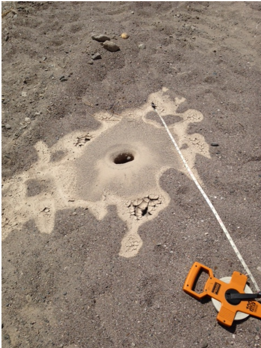
Fig. 3.19 Sand boil observed at the Camarones Bridge (-19.157366°, -70.186806°).
