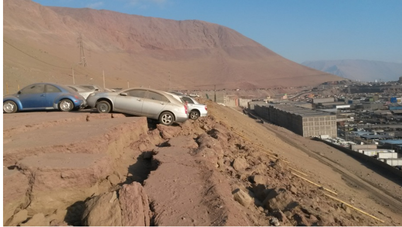
Fig. 5.8. Observed landslides in the ZOFRI area (-20.200965°, -70.128995°)
