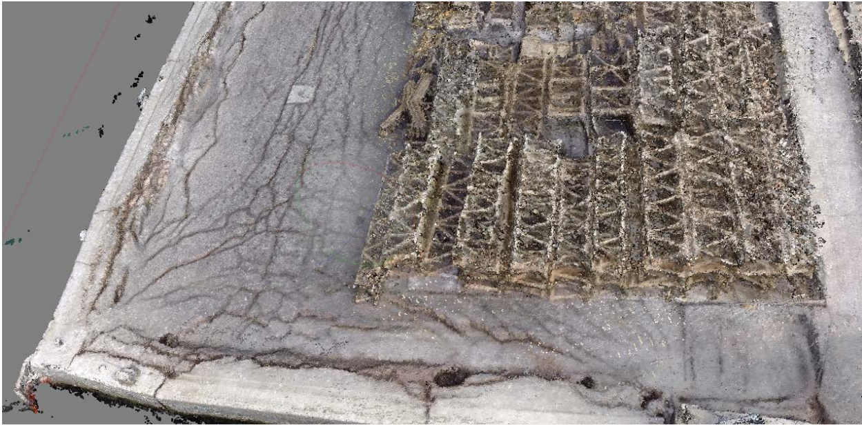
Fig. 2.15 Screenshot of corner cracking and deformation from the dense point cloud
