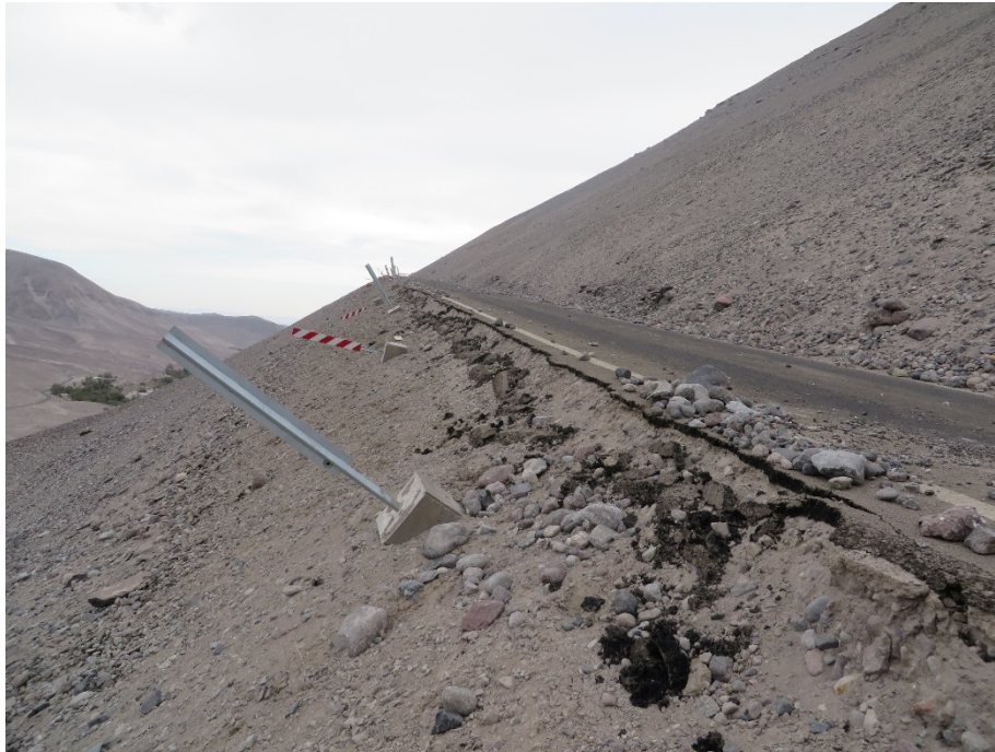
Fig. 6.12 Damage on shoulders of Route A-555 induced by rock falls along unimpeded traffic. (-19.884222°, -69.468258°)
