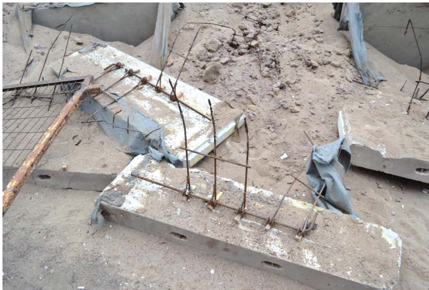
Fig. 4.11. Advanced corrosion of the galvanized steel bars (20.273889°, - 70.123889°) (photograph courtesy of Ramon Verdugo)
