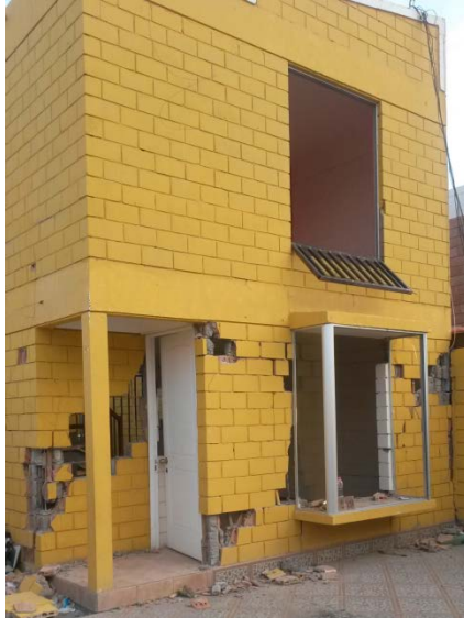
Fig. 5.11. Observed damage for case 2 of Fig. 5.9.
