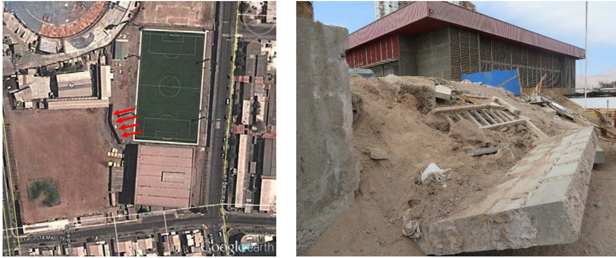
Fig. 4.6. Left: Aerial view of retaining walls at the Municipal Stadium (-20.243611°, - 70.132222°). Right: overturning failure of masonry walls at the Municipal Stadium
