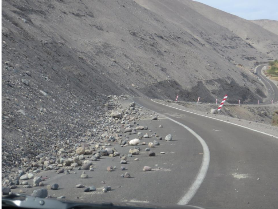
Fig. 6.11. Rock falls along Route A565, unimpeded traffic. (-19.942006°, -69.533139°)
