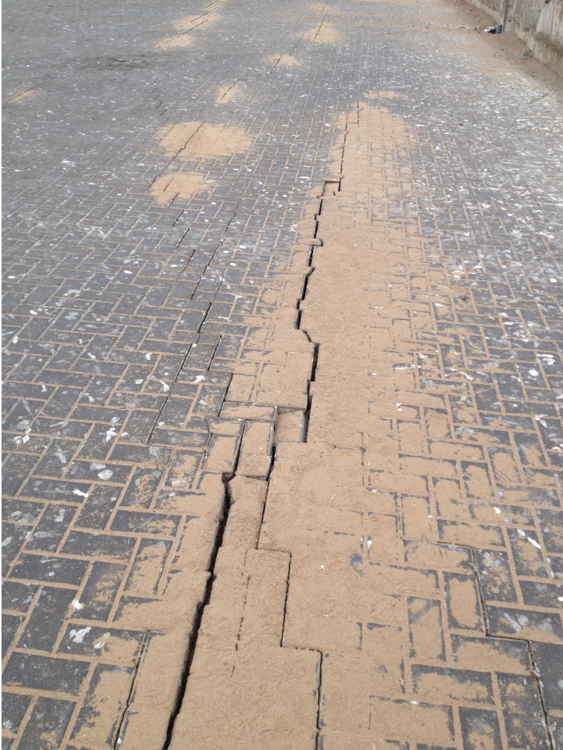
Fig. 2.6 Photograph showing liquefaction ejecta (sand) which vented upward through brick pavement after formation of cracks from lateral spreading. (-20.202451°, -70.158441°)
