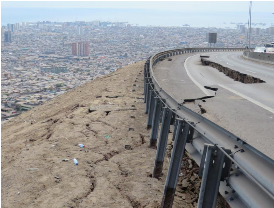
Fig. 6.1 Deep seated slope failure on Route A-16 (-20.243028°, -70.124056°).
