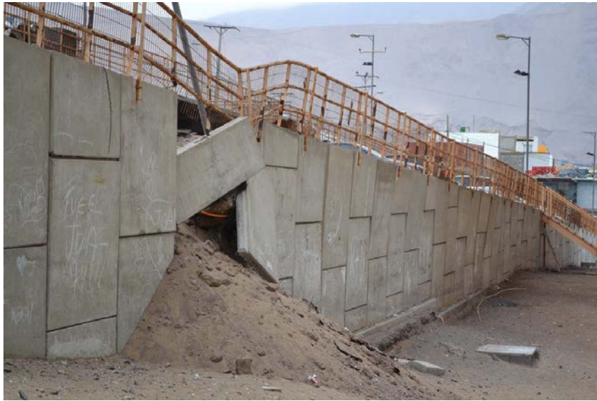
Fig. 4.10. Localized failure in the 1 st level and backfill flow (20.273889°, - 70.123889°) (photograph courtesy of Ramon Verdugo)
