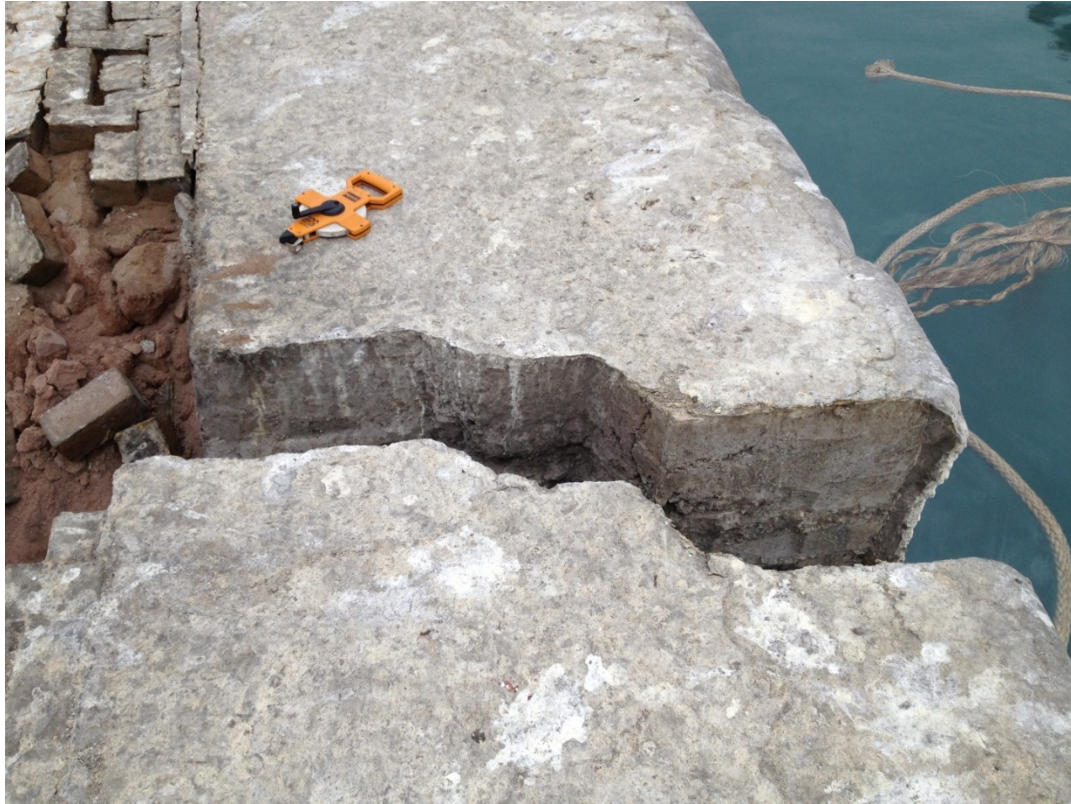
Fig. 2.7 Longitudinal offset in the concrete block quay wall along the perimeter of the Molo pier. (-20.200806°, -70.157416°)
