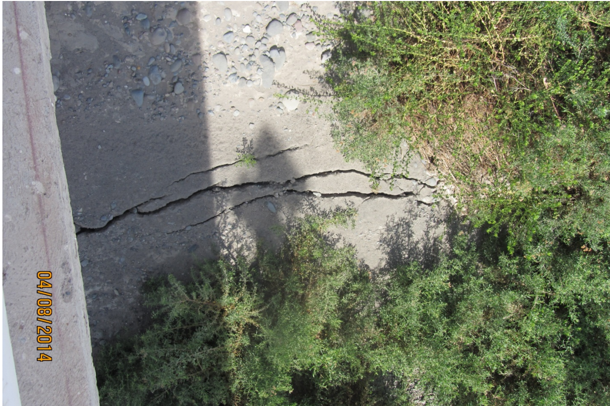
Fig. 3.4 Photograph showing cracks paralleling the stream channel below the Tiliviche bridge (-19.551966°, -69.940921°).
