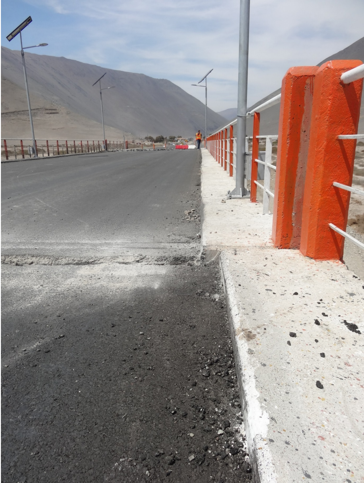
Fig. 3.17 Photograph of lateral offset observed at the Camarones Bridge. (-19.007839°,-70.002497°)
