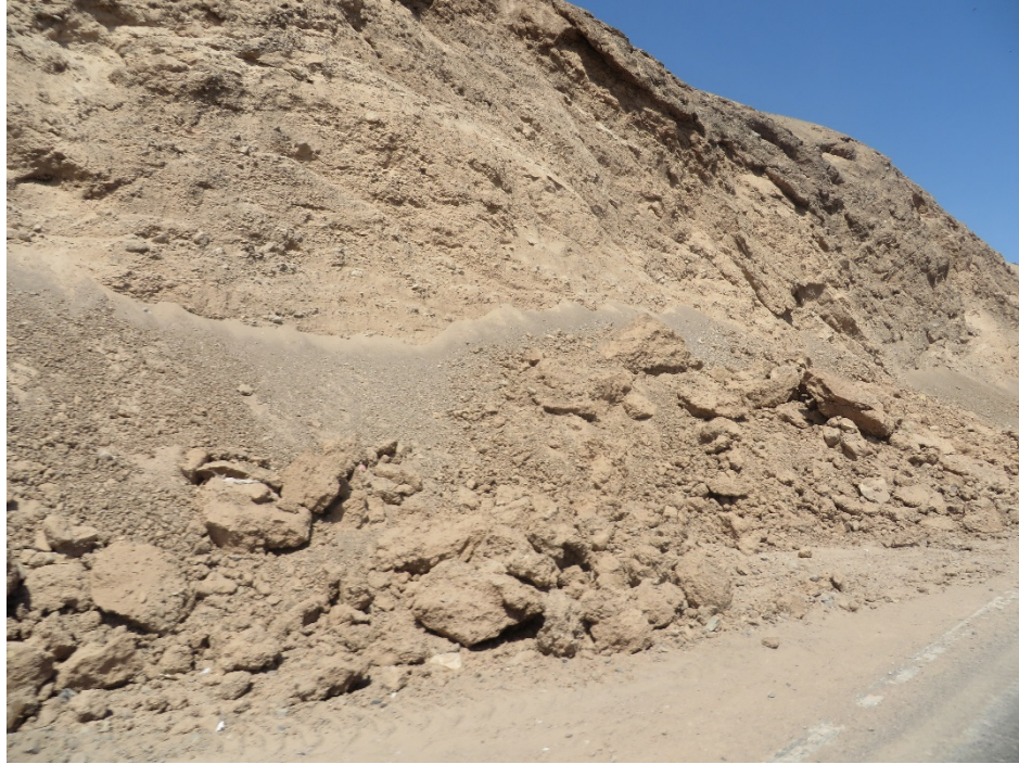
Fig. 6.6. Disaggregated rock slides on Route A-16 (-20.264989°, -70.112106°)
