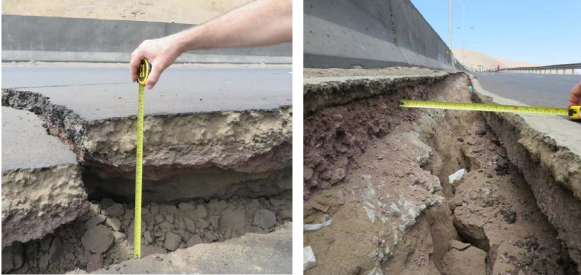
Fig. 6.2 Measured displacements of 40 cm (vertical) and 30 cm (horizontal) on the slope displacement of Route A-16. (-20.243028°, -70.124056°).
