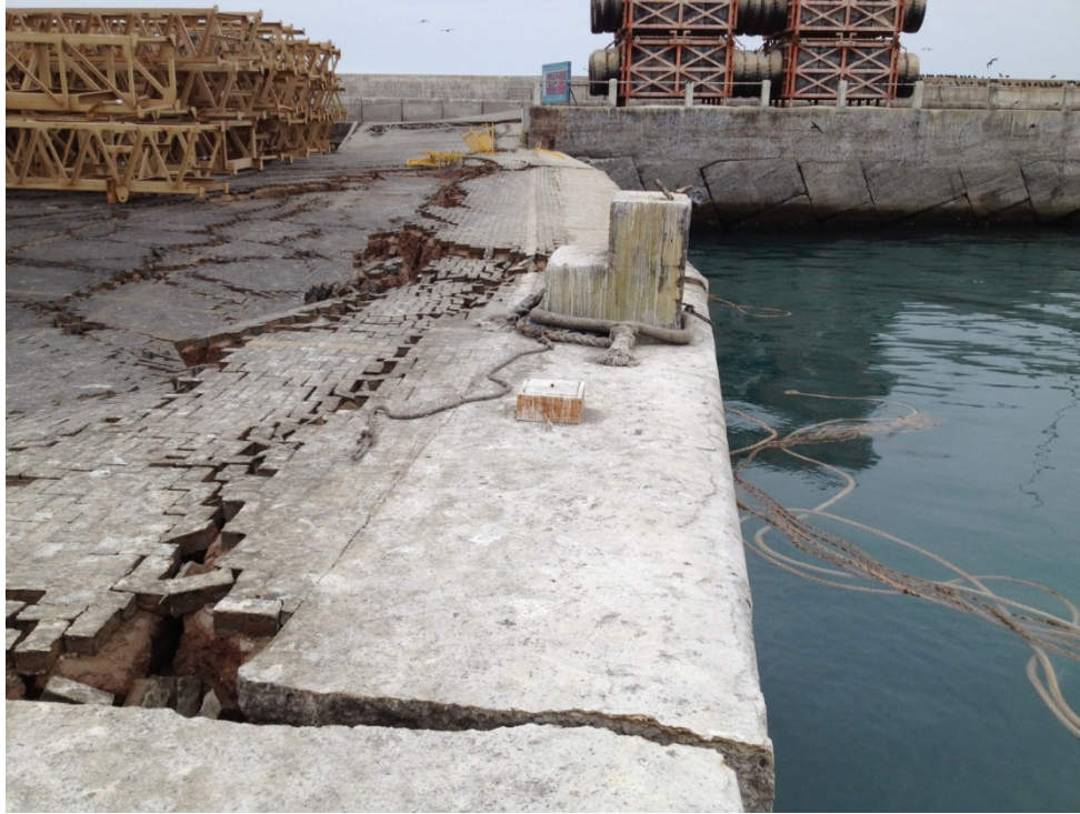
Fig. 2.8 Lateral displacement in the longitudinal and transverse directions near the end of the Molo pier. Horizontal displacement in the transverse and longitudinal direction was about 0.6 m and 0.45 m, respectively. The displacement created offsets in the block perimeter wall. (-20.200916°, -70.157139°)
