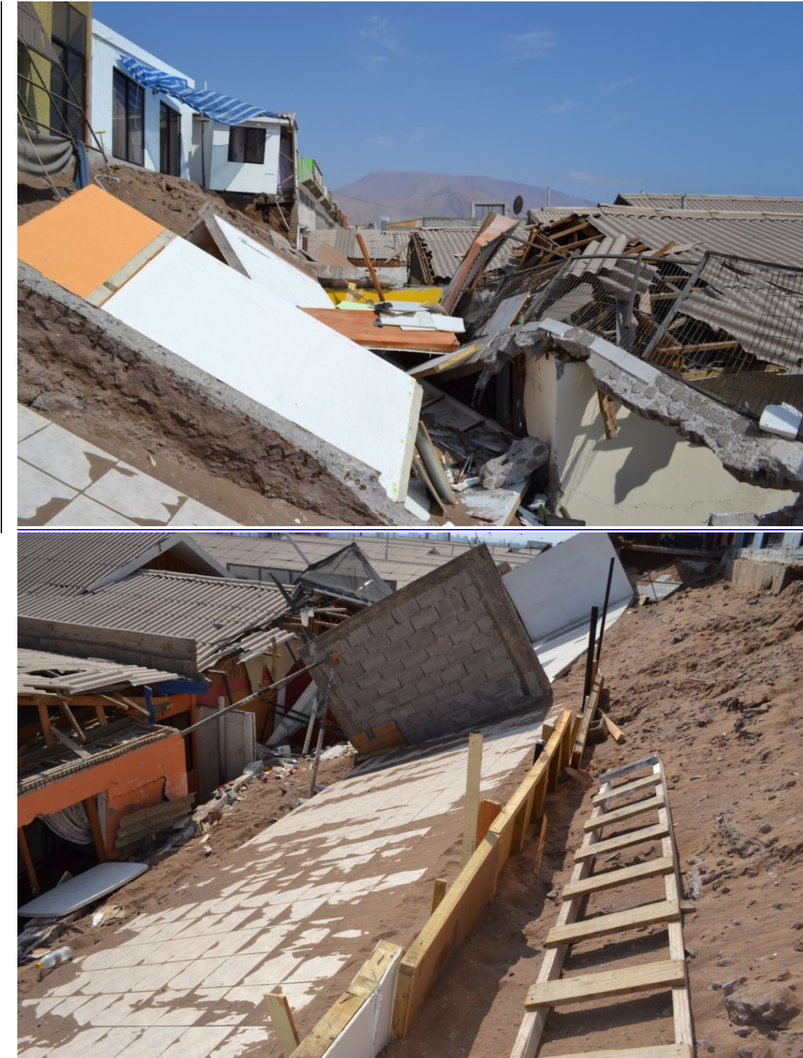
Fig. 4.5 Failure of unreinforced non-engineered retaining walls. (-20.246503°, -70.129301°)
