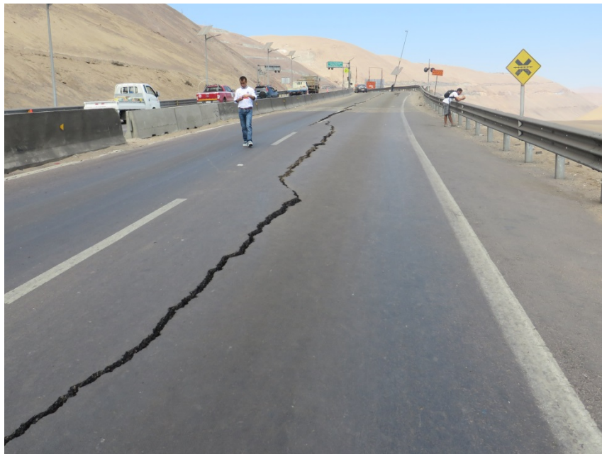
Fig. 6.3 Minor slope displacements and surface cracks extending 300 m past the principal slope displacement on Route A-16. (- 20.243028°, -70124056°).
