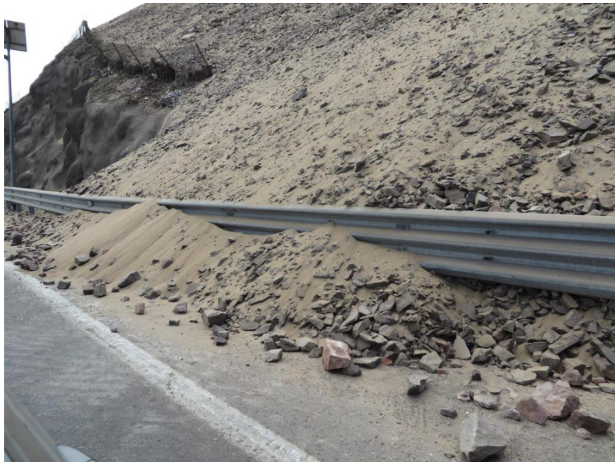
Fig. 6.5 Raveling failure on non-stabilized slopes overtopping the guardrails in Route A-16. (-20.249944°, -70.117747°)
