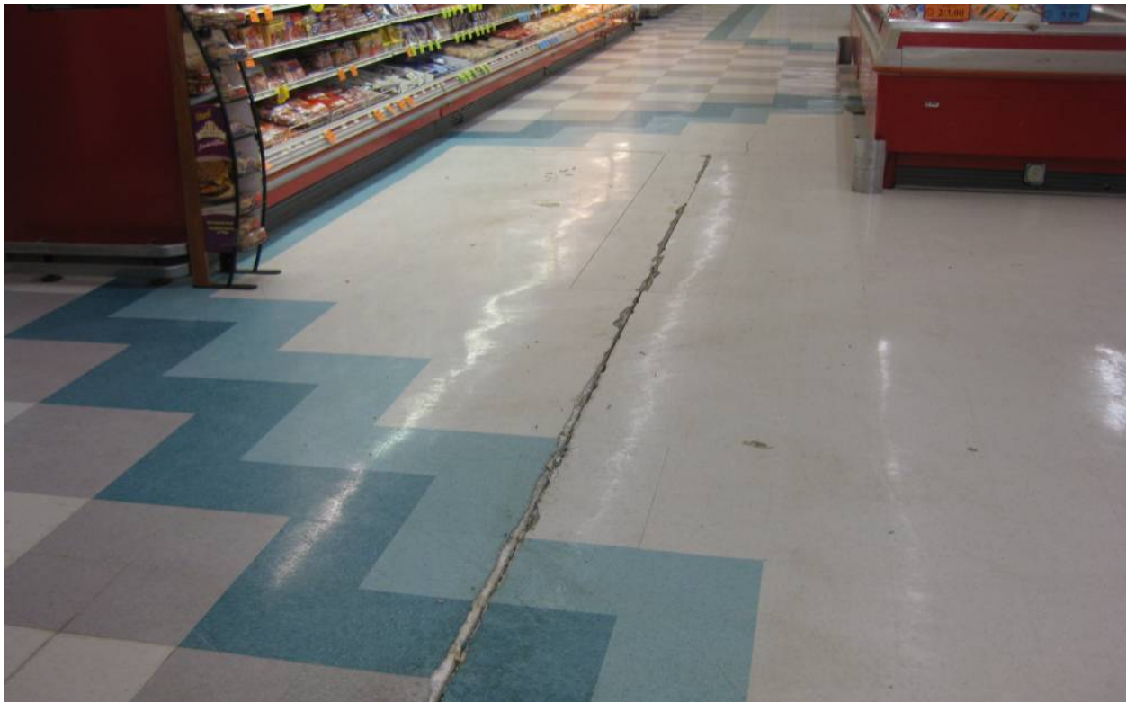
Figure 14 Cracking of the slab on grade concrete slabs at cold joints indicating differential settlement of foundation soils at Ray's Food Place Market (40.776538N; 124.192284W).
