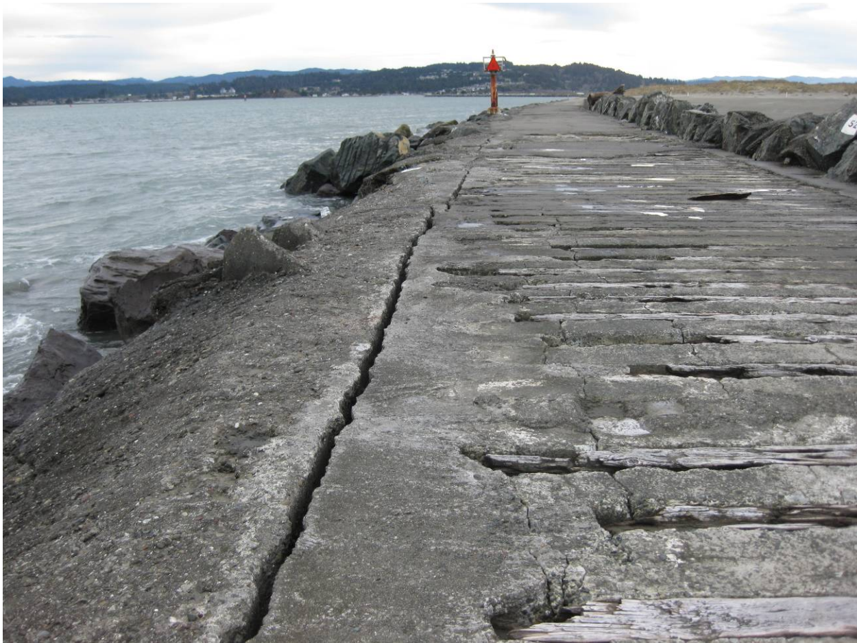
Figure 21 Deformations were observed in the Humboldt South Jetty. Some apparently fresh concrete spalling was observed; however, it was not apparent that this cracking was a caused by the Jan. 9 earthquake (40.75770N;124.234943W).
