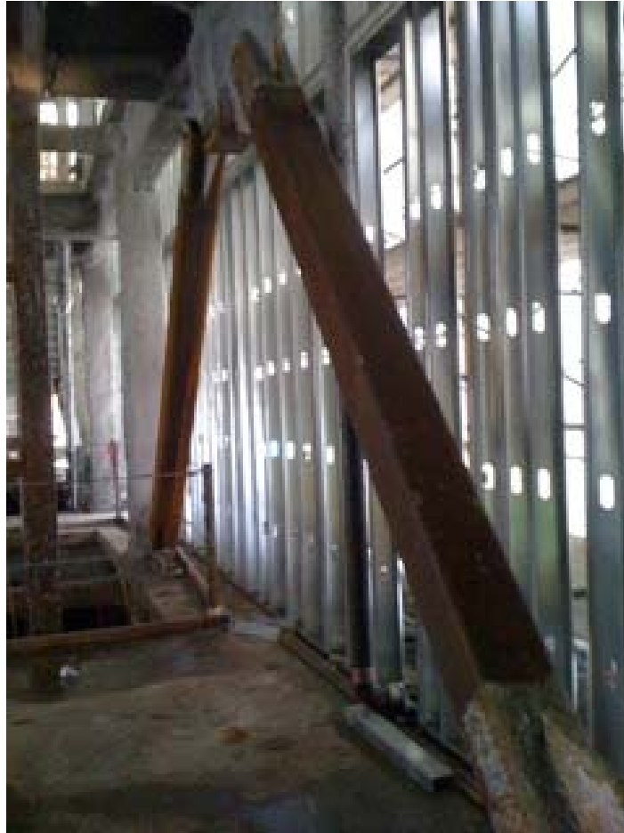
Figure 30 No evidence of damage to the new building (St. Joseph's Hospital) and the braces do not appear to have yielded or buckled
