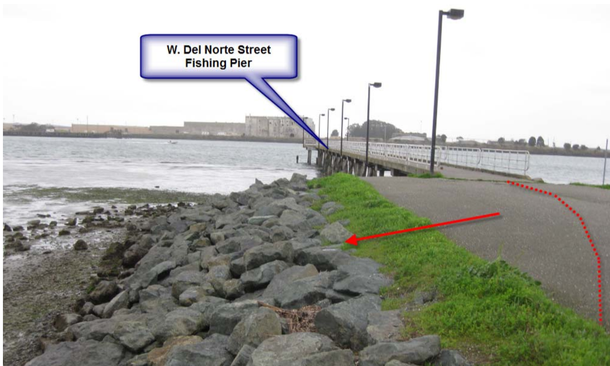
Figure 13 W. Del Norte Street Fishing Pier fractures in pavement indicated near-onset of slope failure (40.790688N; 124.187810W). Arrow indicates directly of movement of embankment and dashed line shows outline of cracking.
