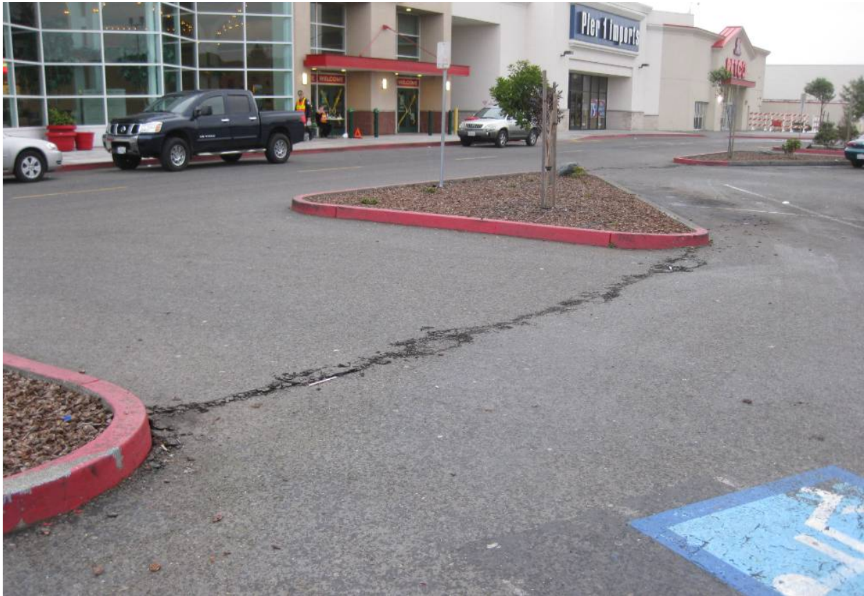
Figure 15 Ruptures in the Bayshore Mall parking lot (40.778562N; 124.190219W).
