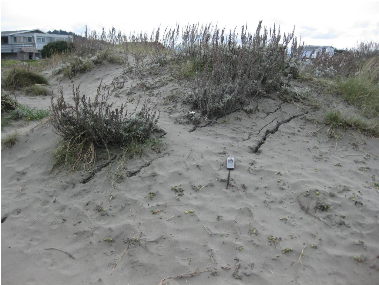
Figure 19 Ground cracking at the King Salmon region at Buhne Drive and King Salmon Avenue. Figure 20 shows the approximate extents of these ‘cracking’ features (40.741957N; 124.216385W).
