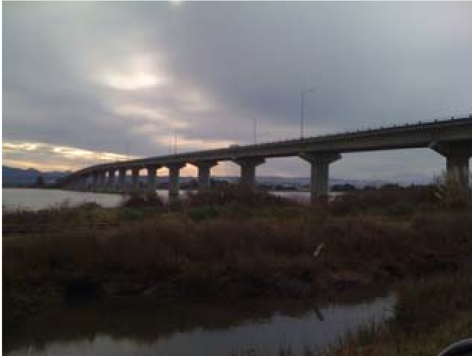
Figure 32 There was no evidence of any damage to the Samoa Bridges, other than very minor working at the end expansion joints and some cracking in the end diaphragms, used to restrain the precast concrete I-girders.
