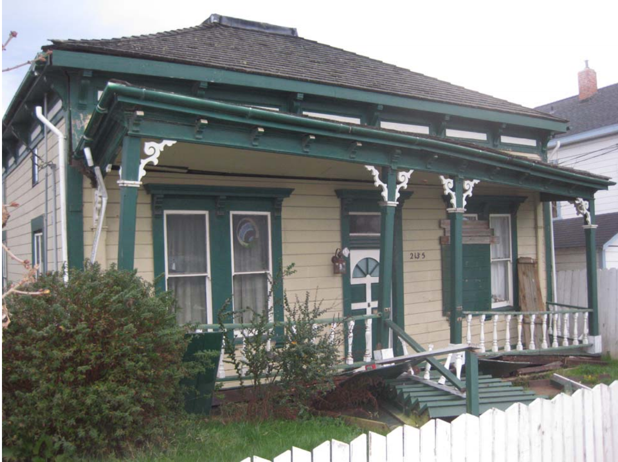
Figure 26 This home was knocked from its foundation (2135 California Street, Eureka, California).
