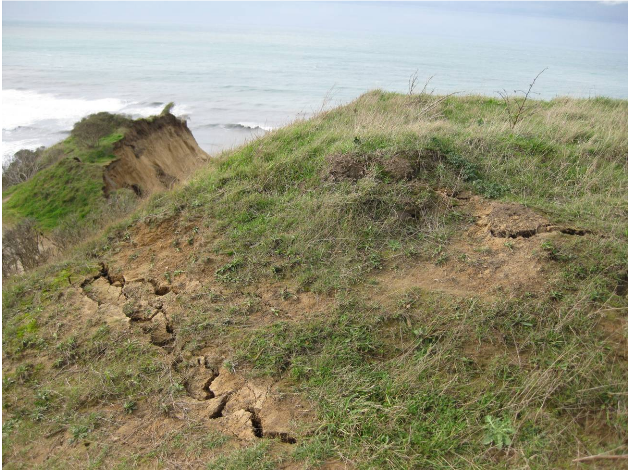
Figure 24 Some lateral displacement cracking was observed on the bluffs immediately south of Centerville Beach; however, this is an area of active bluff erosion (40.560943N; 124.353851W).
