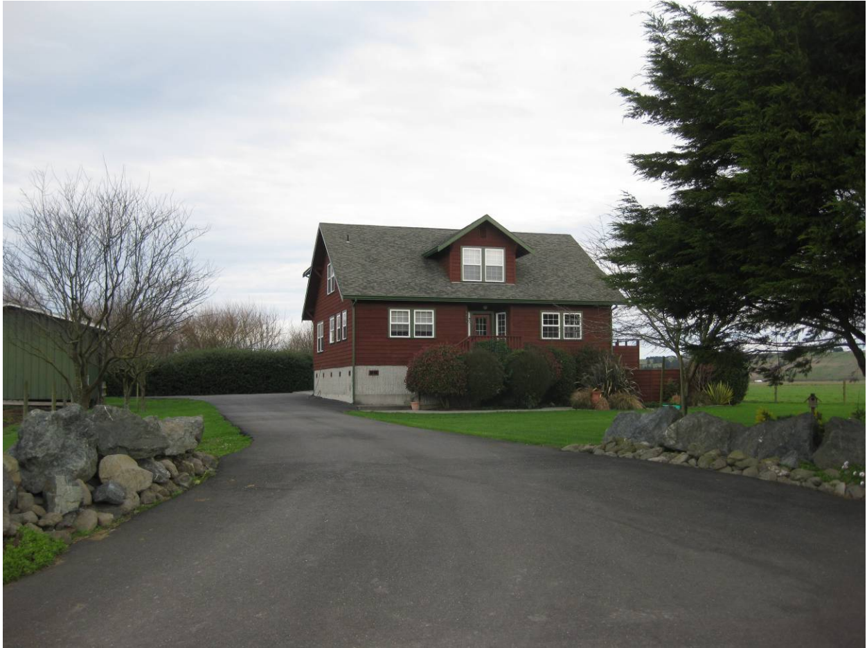
Figure 22 No significant structural damage and or ground features were observed in the Eel River valley along Cannibal Island Road (40.642967N; 124.262067W).
