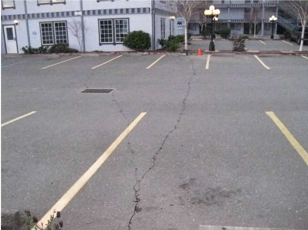
Figure 16 Cracking in AC pavement in the parking lot at the Best Western, NW corner of Broadway Street and Truesdale Street (40.775312N; 124.1919019W).
