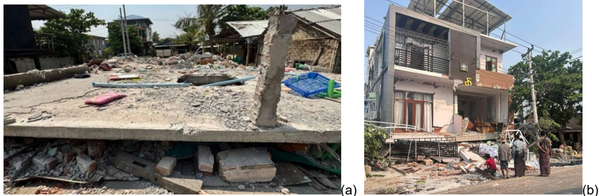
Figure 5.3.1. Collapsed reinforced concrete frames of private schools in Kyaukse (a) and Sagaing (b) (Source: Htet Naing Zaw, BBC Burmese (a); BBC Burmese (b)).
