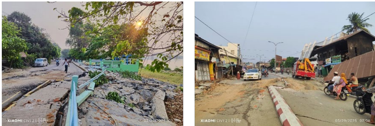
Figure 2.15. Roadways with offset of several feet (21°52'49.27"N, 95°59'5.57"E) (Source: HMSon @heungburma on X ).
