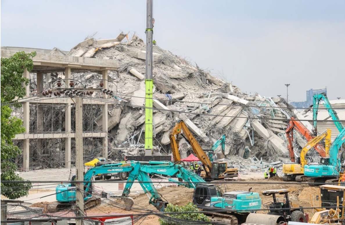
Figure 5.5.1 The site of 30-story building collapse showing debris pile next to an undamaged ground plus two-story concrete frame building also under construction (Source: Thai Post News ).
