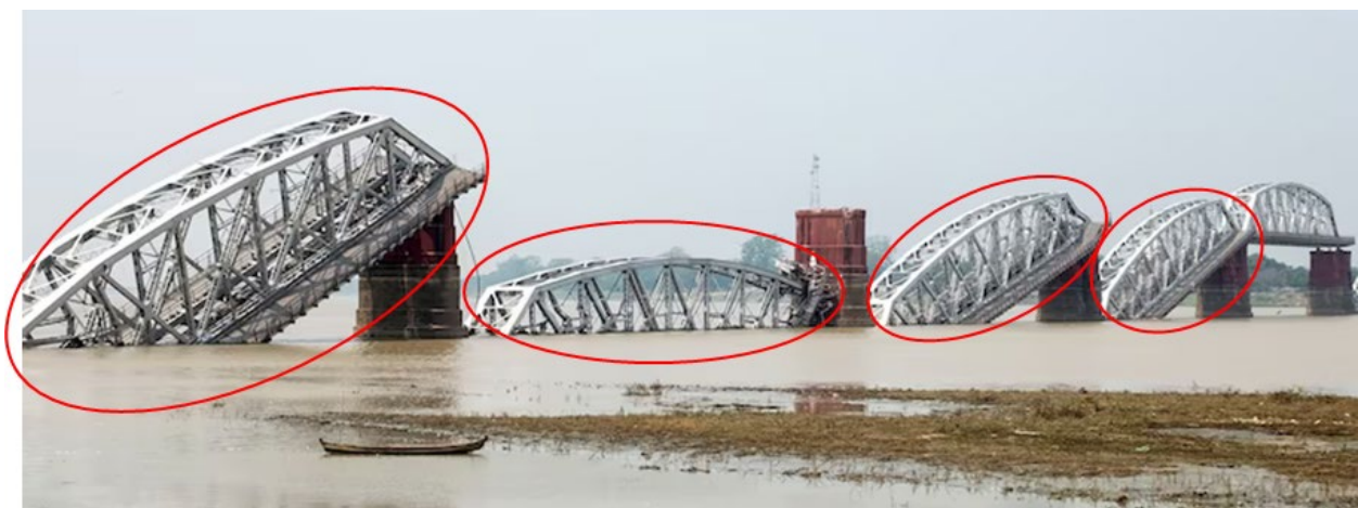
Figure 6.2.2. Unseated bridge decks of the Ava Bridge, noting undamaged piers and fully intact bridge deck sections (Deliso 2025).
