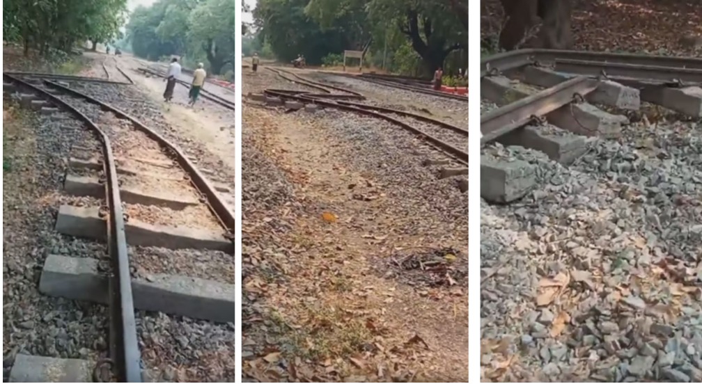
Figure 6.2.5. Track deformation at Thayetkon Railway Station (Source: Facebook ).
