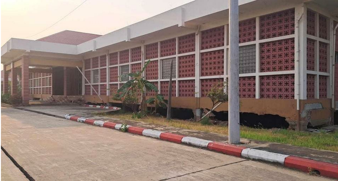
Figure 5.2.4. Wachat Jivitadana Sangha Hospital in Sagaing [Coordinates: 21.915215, 96.001606] was closed due to physical damage at the base of the structure (Source: Than Lwin Khet News on Facebook ).
