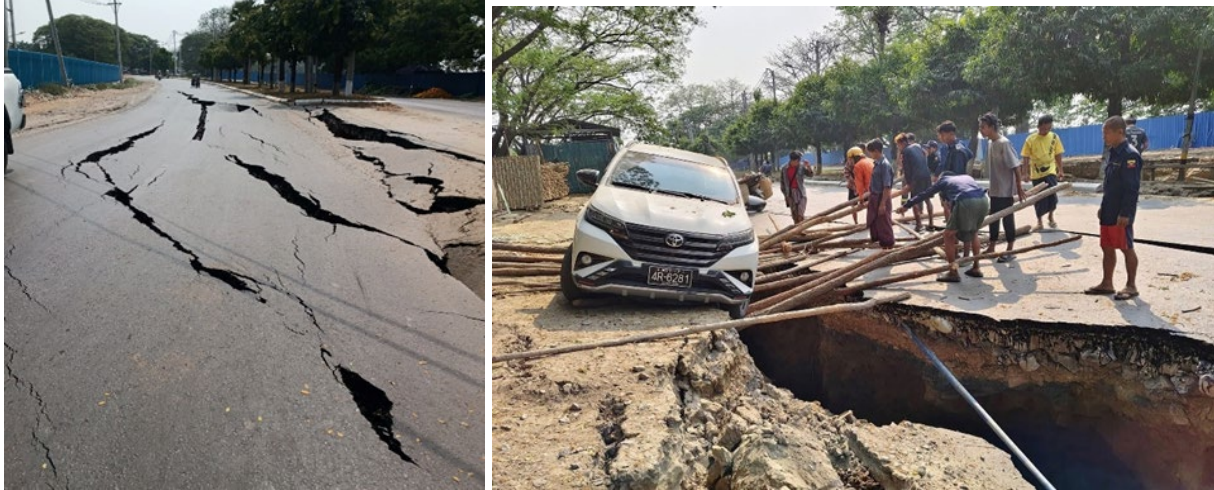
Figure 4.3.3. Extension in pavements along Myo Patt Road [Approximate Location 21.9260, 96.0546] (Credit: ZoMung Thawng).
