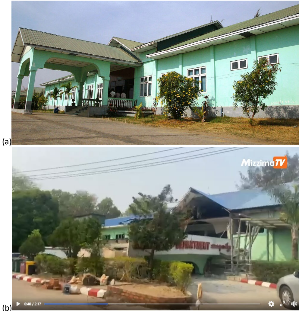
Figure 5.2.2. Nay Pyi Taw General Hospital: (a) back view of the building shows one of the typical reinforced concrete entrance canopies before the earthquake; (b) canopy collapsed at the Emergency Department (Sources: (a) Wikimedia Commons , (b) Mazzina Myanmar , 2025).
