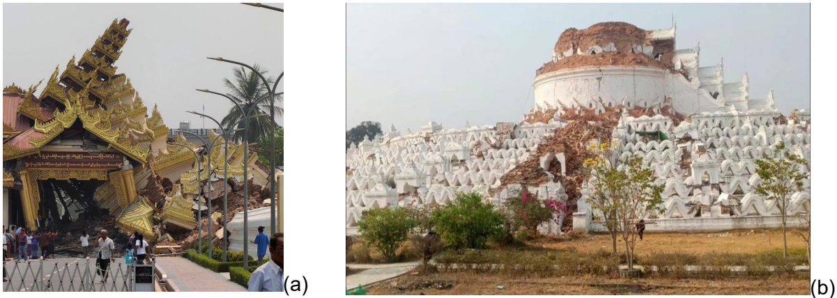
Figure 5.4.2. Damage to religious sites in Myanmar: (a) Mahamuni Pagoda (Source: @SaadAbedine on X ); (b) collapse of the Myatheindan Pagoda (or Hsinbyume Pagoda) (Source: Vietnam ).
