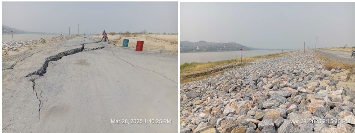
Figure 4.3.2. Evidence of lateral spreading along riverbank [Approximate location 21.9260, 96.0546]: fissures in the road at the crest of the slope (left) and extension cracking near the toe of slope (right) (Credit: ZoMung Thawng).
