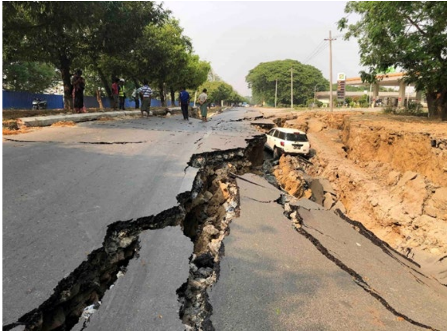
Figure 4.6.2. Severe ground deformation along Myo Patt Road next to Amarapura Urban Development Project site (Credit: ZoMung Thawng).
