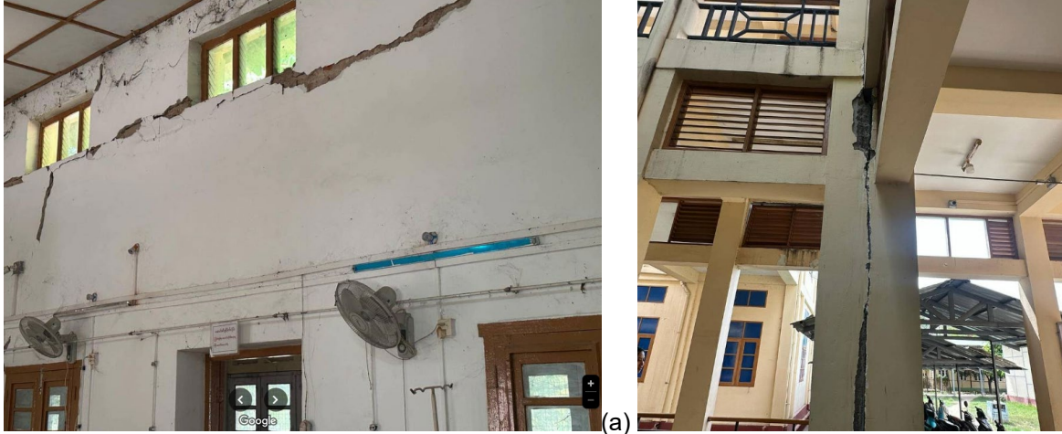
Figure 5.2.5. Evidence of physical damage in the interiors of a building at the Sagaing General Hospital: (a) non-structural damage in facade walls and (b) concrete cover detachment in reinforced concrete columns due to apparent pounding (Source: See Clearly via GoogleMaps ).
