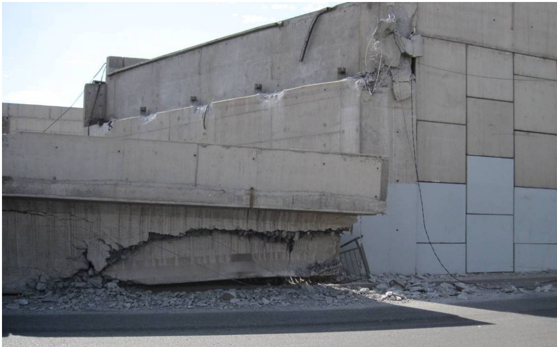
Figure 12.1. Intersection of Americo Vespucio Norte and Independencia. Abutment of a collapsed bridge. (33°21'57.83"S, 70°41'17.71"W)
