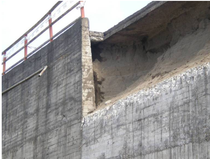
Figure 12.9. Granular fill soils and water seepage evident behind failed portion of wall.
