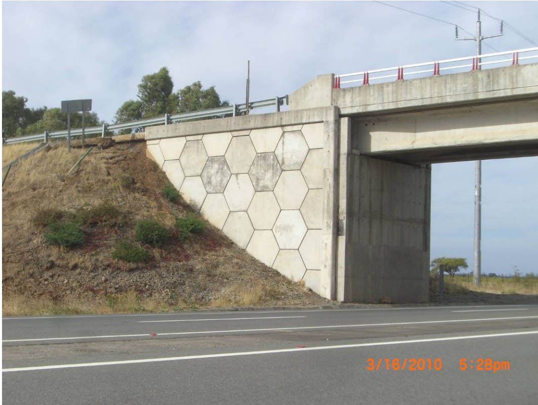
Figure 12.4 Undamaged MSE wingwall on overpass structure over highway 152 west of Chillan despite sliding of adjacent fill slope (S36.6588, W72.2776).
