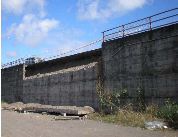
Figure 12.7. Failed reinforced concrete retaining structure in San Pedro.
