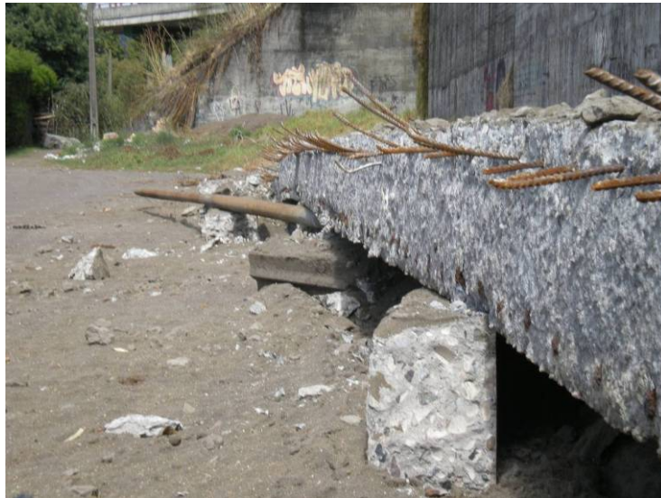
Figure 12.8. Toppled portion of 16-inch thick wall showing bent compression bars and snapped tension bars.
