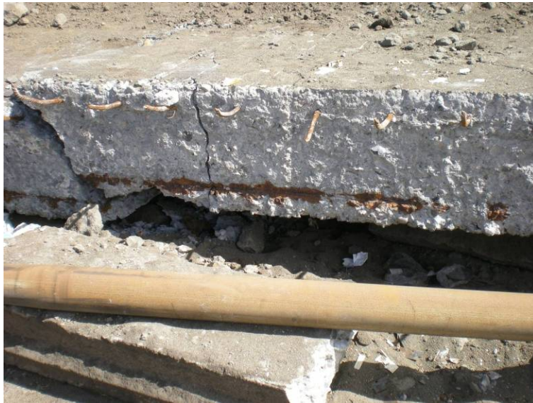
Figure 12.10. Corrosion of horizontal reinforcing steel where water entered the joint.
