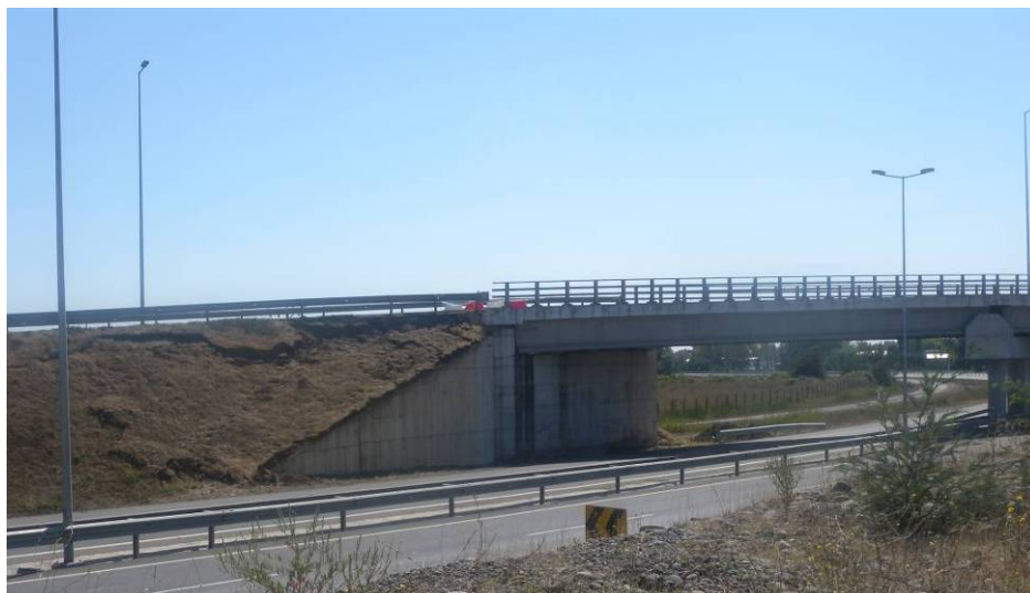
Figure 12.6. Surficial sloughing on a bridge approach embankment, with the abutment showing no evidence of damage, Route 5, north of Chillan.
