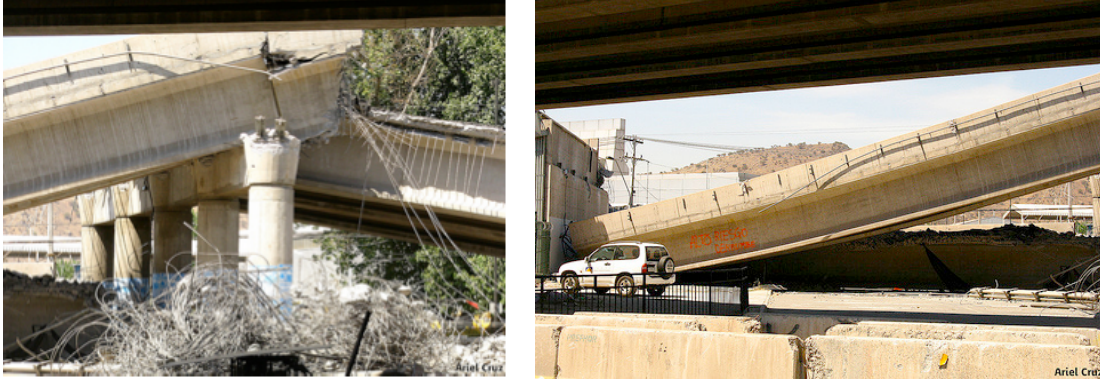
Figure 5.6. Paso Superior Lo Echevers (S33.3759° W70.7476°). Collapse of the eastbound deck of the Americo Vespucio Norte ring road (Source: http://www.flickr.com/photos/consulta_recorridos/ ).
