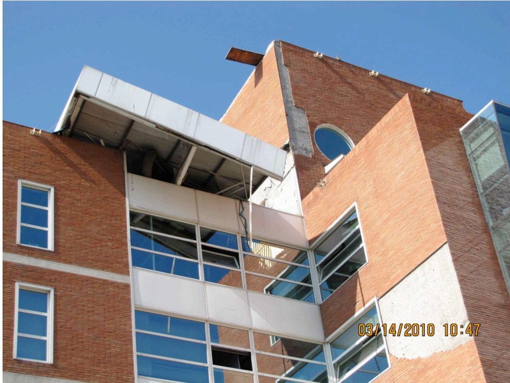
Figure 5.12. Site DA004 (S33.387652° W70.617122°, 1047 hrs on 03/14/2010) Identical 7-story buildings connected; damage was observed in only one of the two.
