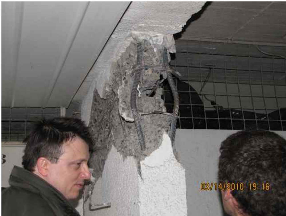
Figure 5.24. Site DA019 (S33.016045° W 71.551990°, 1916 hrs on 03/14/2010). Damaged 10-story building. Lack of confinement beam-column joints and low quality concrete.
