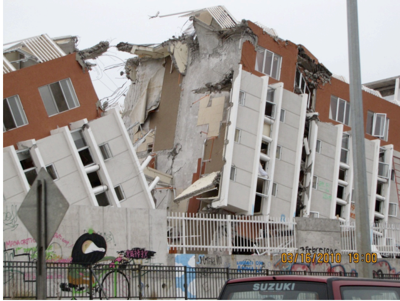
Figure 5.34. Collapsed structure (S 36.828067° W73.061639°, 1900 hrs on 03/16/2010) designed using Soil Type II conditions.
