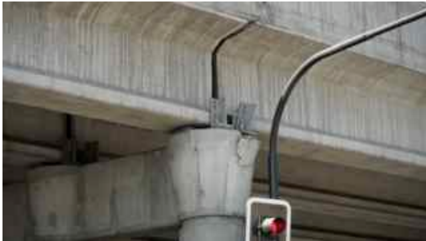
Figure 5.7. Paso Lo Boza (S33.3865° W70.7601°). Minor structural damage of shear keys (Source: Dr. Roberto Leon, personal communication).
