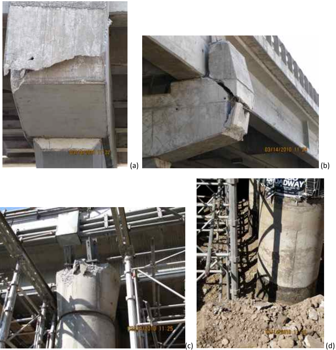
Figure 5.5. Paso San Martin (S33.3660° W70.6891°, 1122 hrs on 03/14/2010). Shear key failure and longitudinal, transverse deck displacement.
