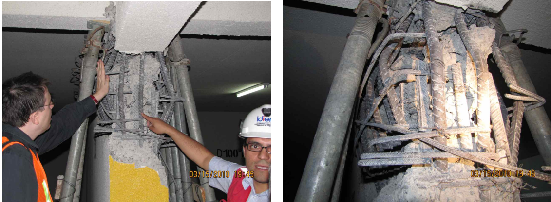
Figure 5.26. Site DA027 (S 33.020074° W 71.544055°, 1945 hrs on 03/15/2010). Heavily damaged 20-story building, lack of confinement at beam-column joints.
