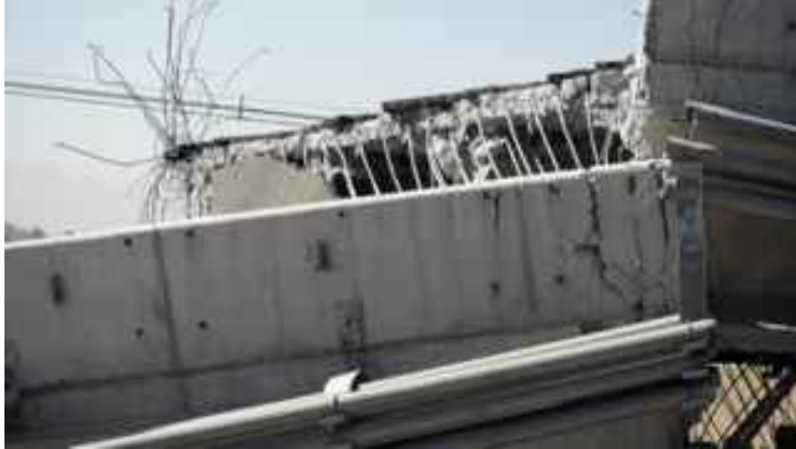
Figure 5.8. Paso Miraflores (S33.3945° W70.7700°). Deck collapse detail (Source: Dr. Roberto Leon, personal communication).
