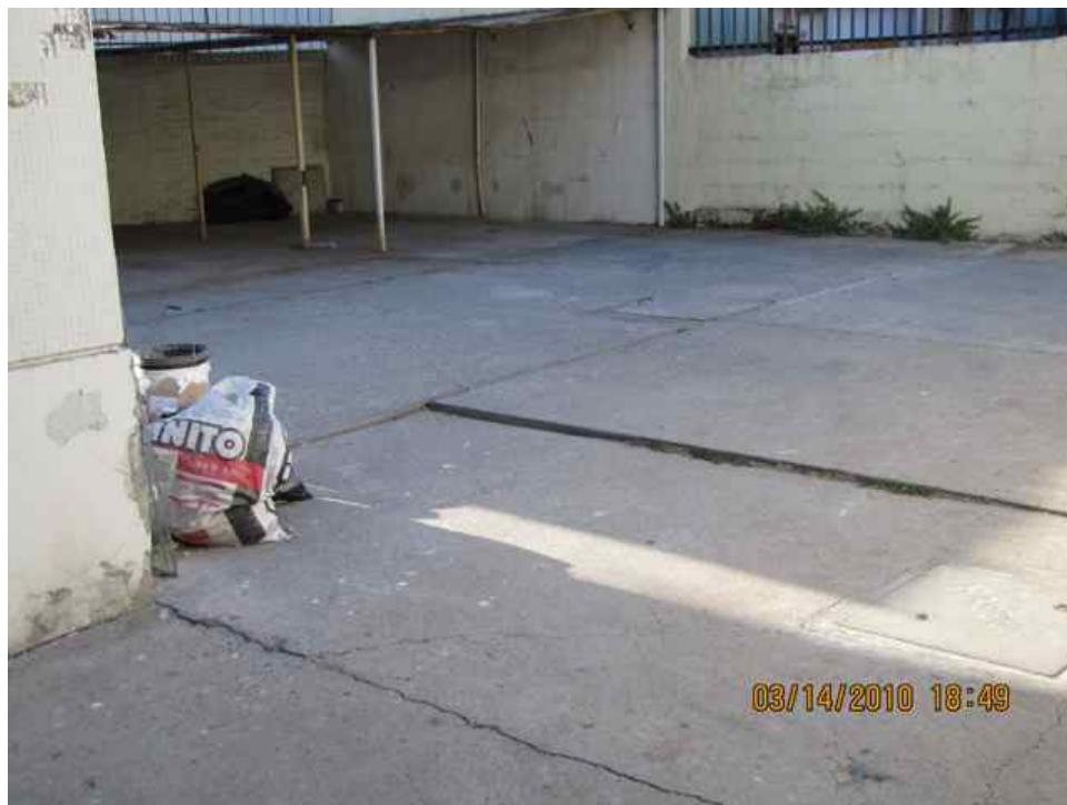
Figure 5.23. Site DA018 (S 33.017386° W 71.557107°, 18:48 hrs on 03/14/2010) Damaged 6-story building. Evidence of ground settlement.
