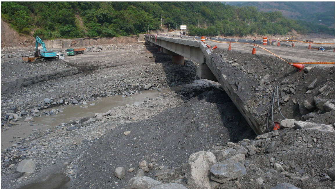
Photo 2-3-5. Damaged abutment and deck of Bridge #2 .
