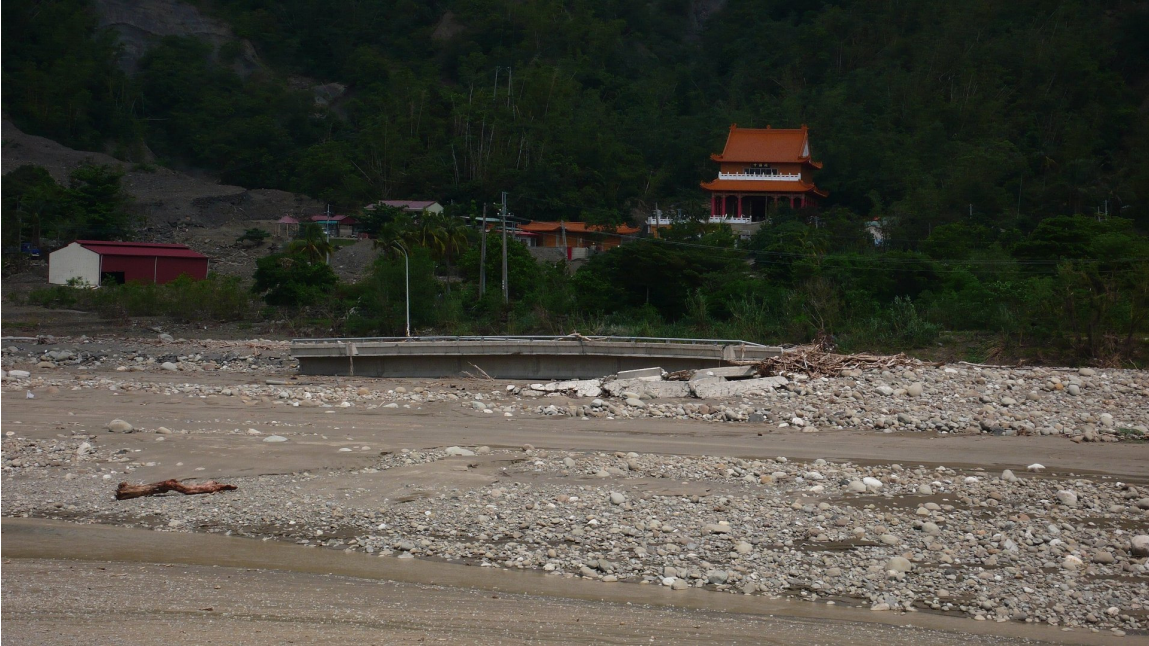
Photo 2-1-5. A span was washed downstream (Side Bridge)
