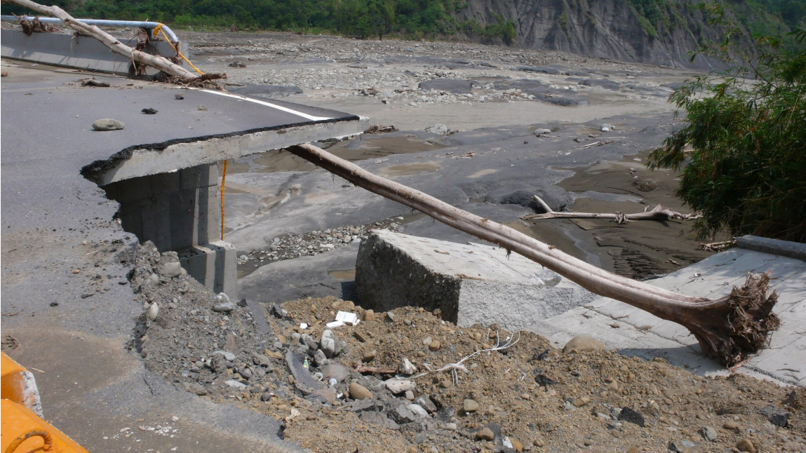
Photo 2-1-3. Collapse of retaining walls at the abutment of Jia Xian Bridge.
