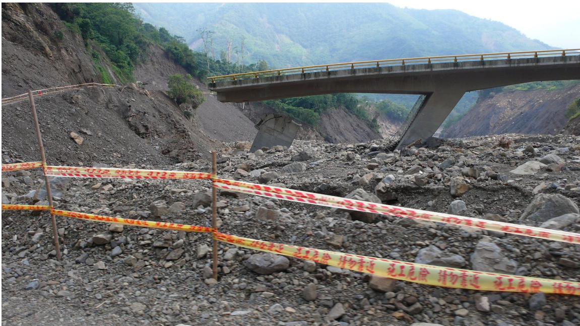
Photo 2-2-1. Failure of the abutment and superstructure of a bridge.
