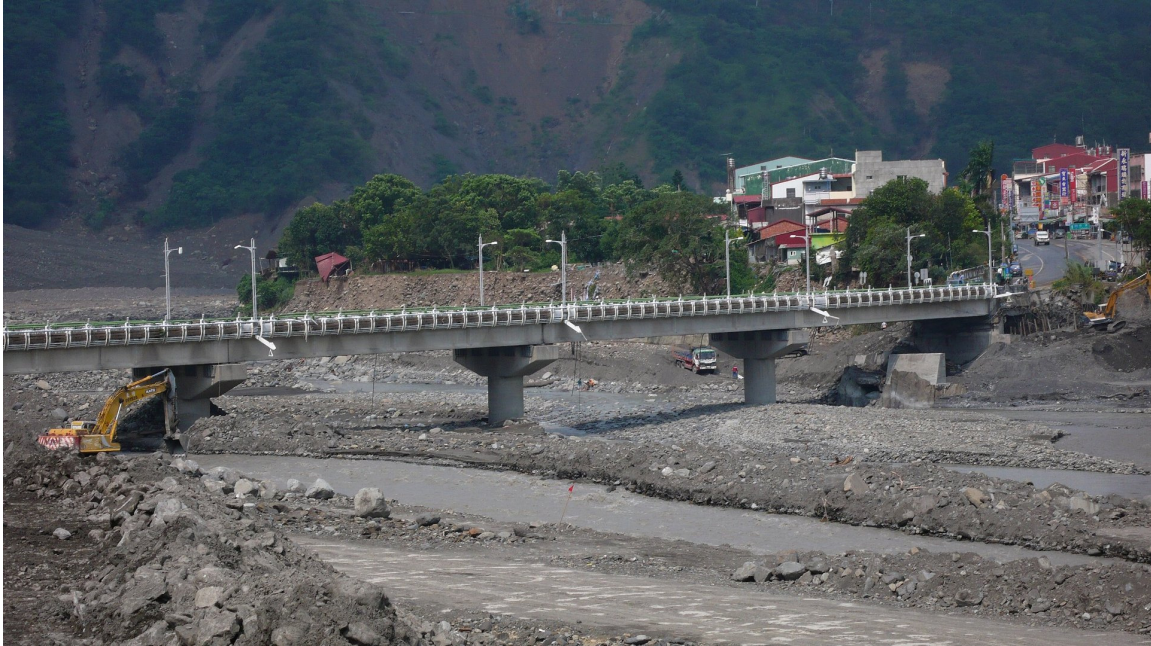
Photo 2-3-6. The vertical clearance of Bridge #2 was significantly reduced by debris deposition.
