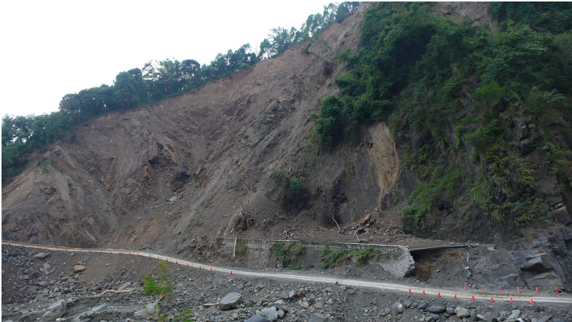
Photo 2-2-2. Significant slope failure on both sides of the road in Jia Xian Village.
