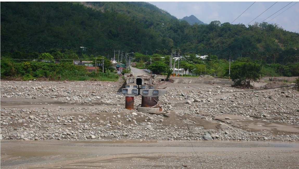
Photo 2-1-4. Part of the superstructure and pier foundation disappeared (Side Bridge).
