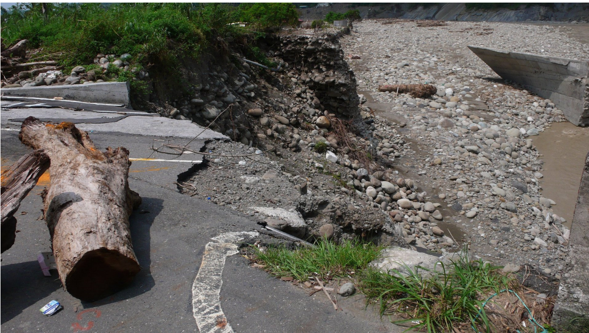
Photo 2-1-6. Scouring of the river bank and road. Note that part of a retaining wall stayed in the riverbed (Side Bridge).
