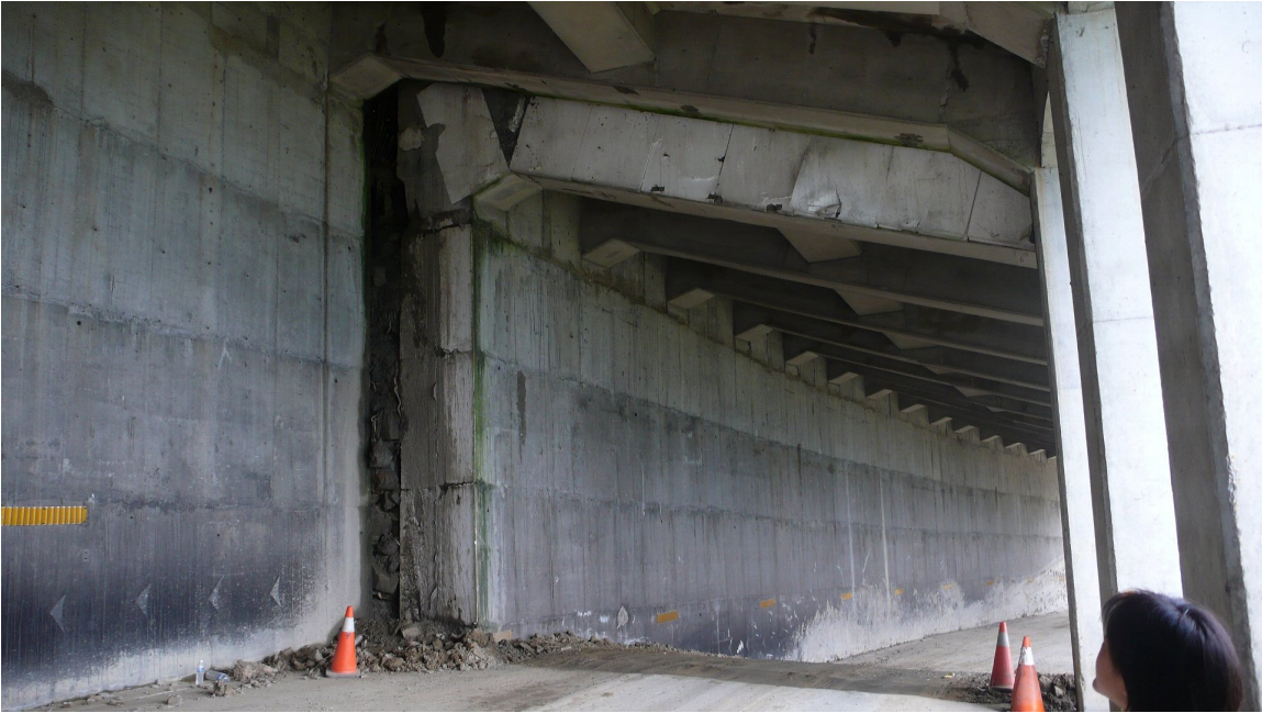
Photo 5-3-3. One of the sections of the shed displaced relative to the stable section.
