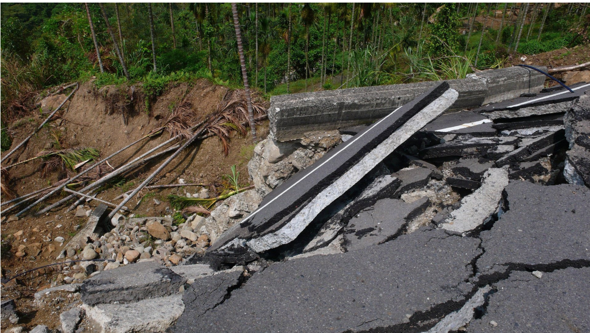
Photo 5-2-5. Pavement damaged by slope movement.
