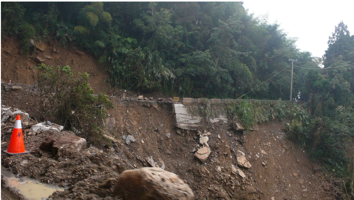
Photo 5-6-6. The loss of foundation due to landslides led to the collapse of many retaining walls.
