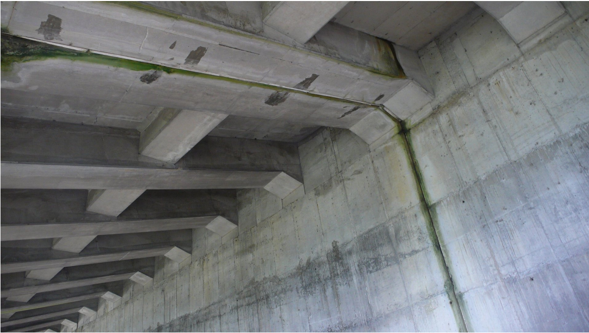
Photo 5-3-4. The other sections did not exhibit relative displacement.
