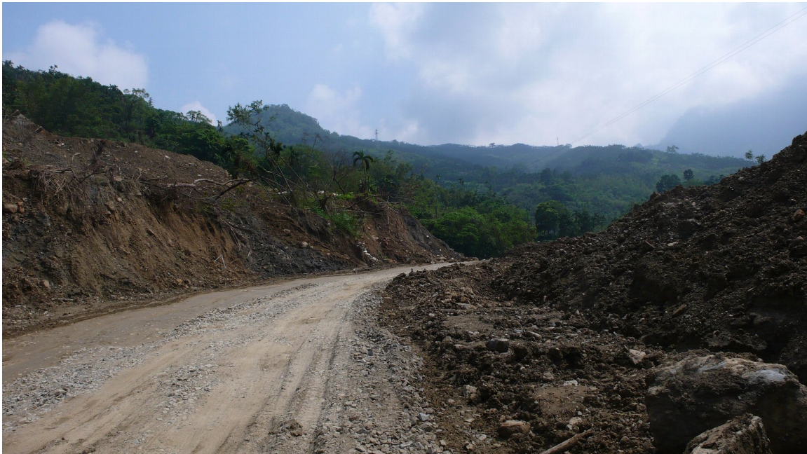
Photo 5-2-1. The road was buried by a debris flow which traveled from the top of a mountain down to a stream.
