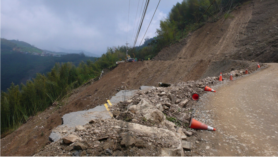
Photo 5-4-1. Landslides. Note the original location of highway and new access road
