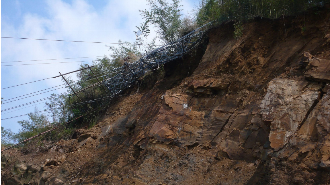
Photo 5-2-6. An electricity transmission tower damaged by landslides.
