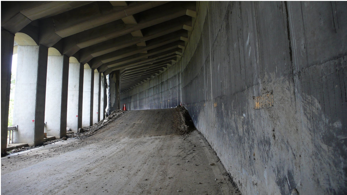
Photo 5-3-2. Differential settlement of road inside the shed.
