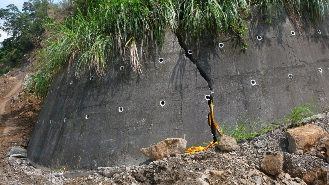
Photo 5-2-2. A retaining wall damaged by landslides.
