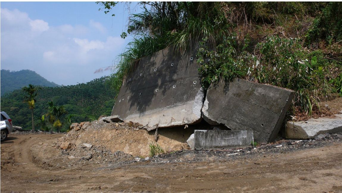
Photo 5-2-3. Another damaged retaining wall.
