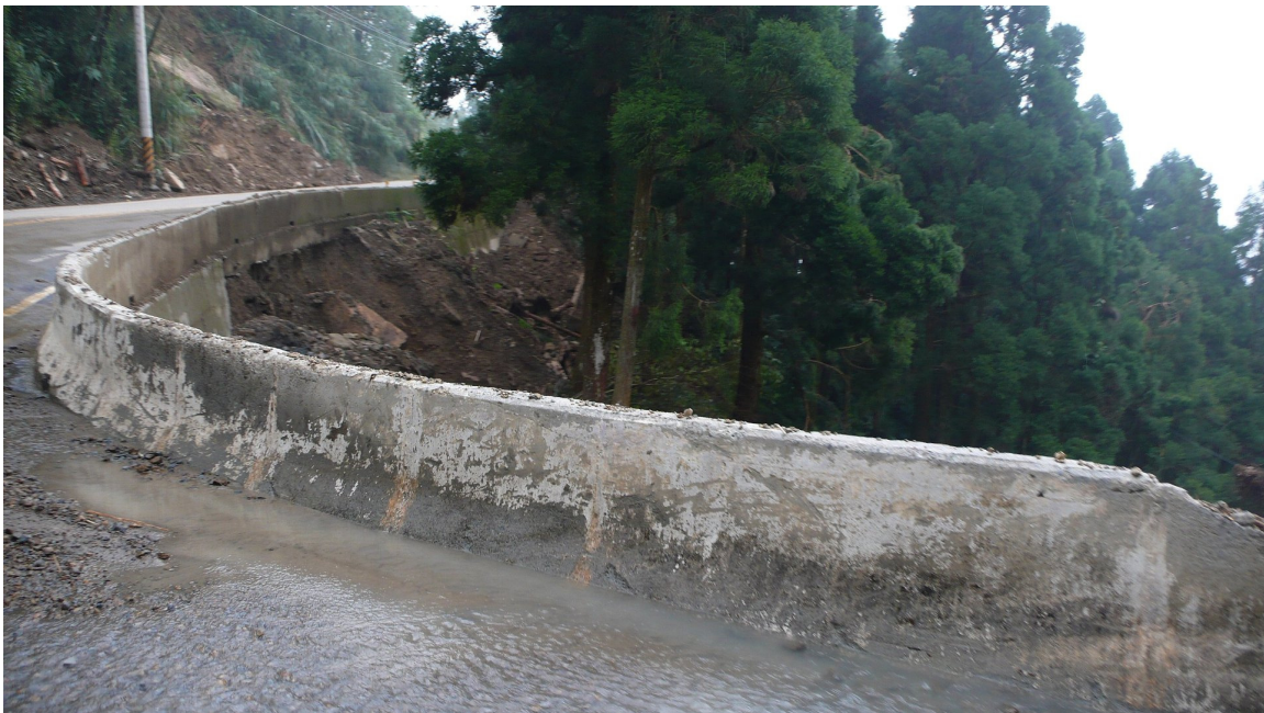
Photo 5-6-4. The Jersey Barrier was reported to have blocked the water from draining during heavy rainfall
