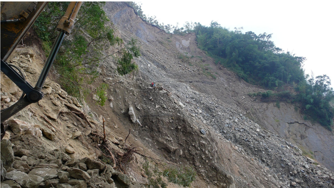
Photo 5-5-3. Several hundred meters of the highway were lost due to a landslide.
