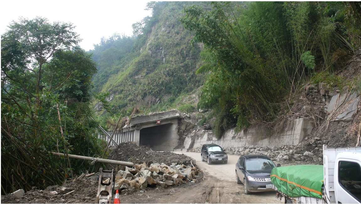
Photo 5-3-1. Debris flow was seen at one end of the shed. Part of the shed was buried.
