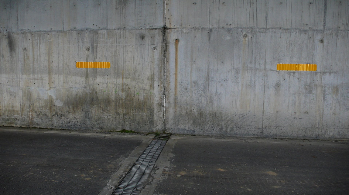
Photo 5-5-2. Construction joints remained intact; these did not show evidence of relative displacement.
