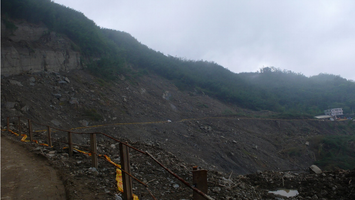
Photo 5-3-5. Landslides damaged several hundred meters of the existing roadway. The mountain was cut to create a new access road.
