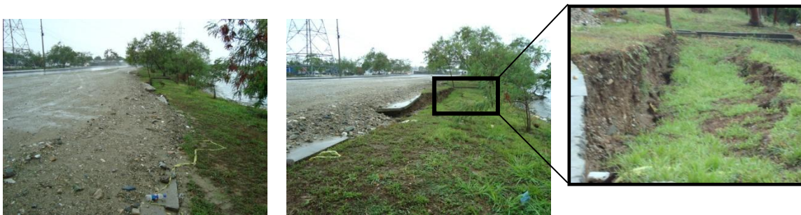
Figure 6 – Temporary repair of roadway embankment, due to lateral spreading [06/20/2009, 1:25 PM, N15.848216, W87.958604].
