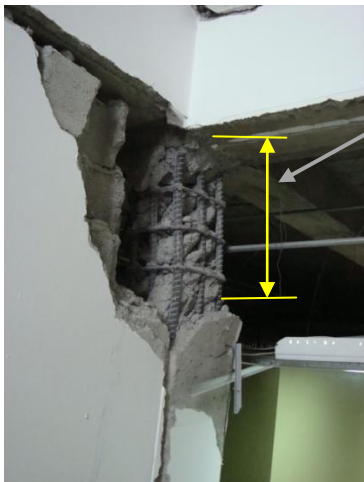
(b) Column failure at the infill wall frame interface [06/19/2009, 5:08PM, N15.473038, W88.018103]
