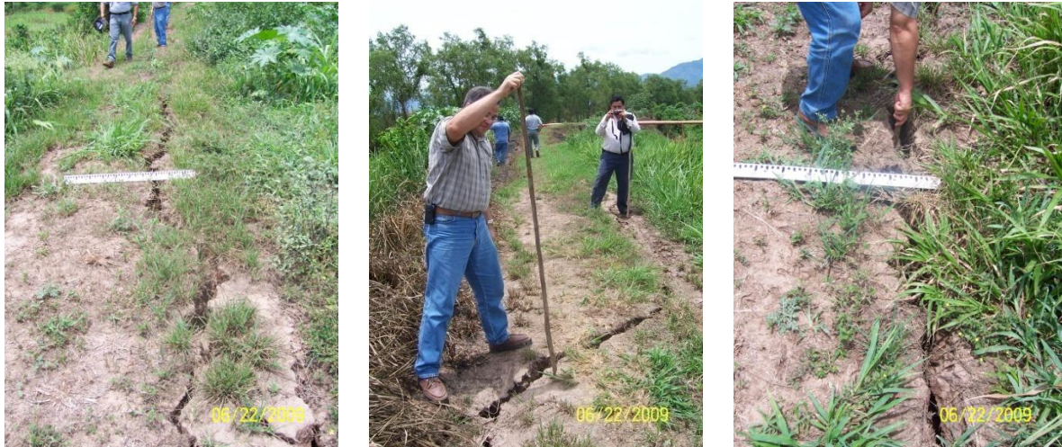
Figure 10 – Cracks at the crest of levees exceeding 1.5m deep [06/22/2009, 11:57AM, N15.344505, W87.868515].
