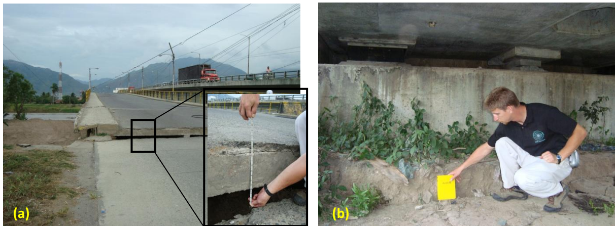
Figure 13 – Settlement of ground around abutments due to liquefaction (a) Old bridge westbound [06/19/2009, 6:36PM, N15.404409, W87.821095], and (b) New bridge, eastbound [06/19/2009, 6:52PM, N15.40422, W87.821021].
