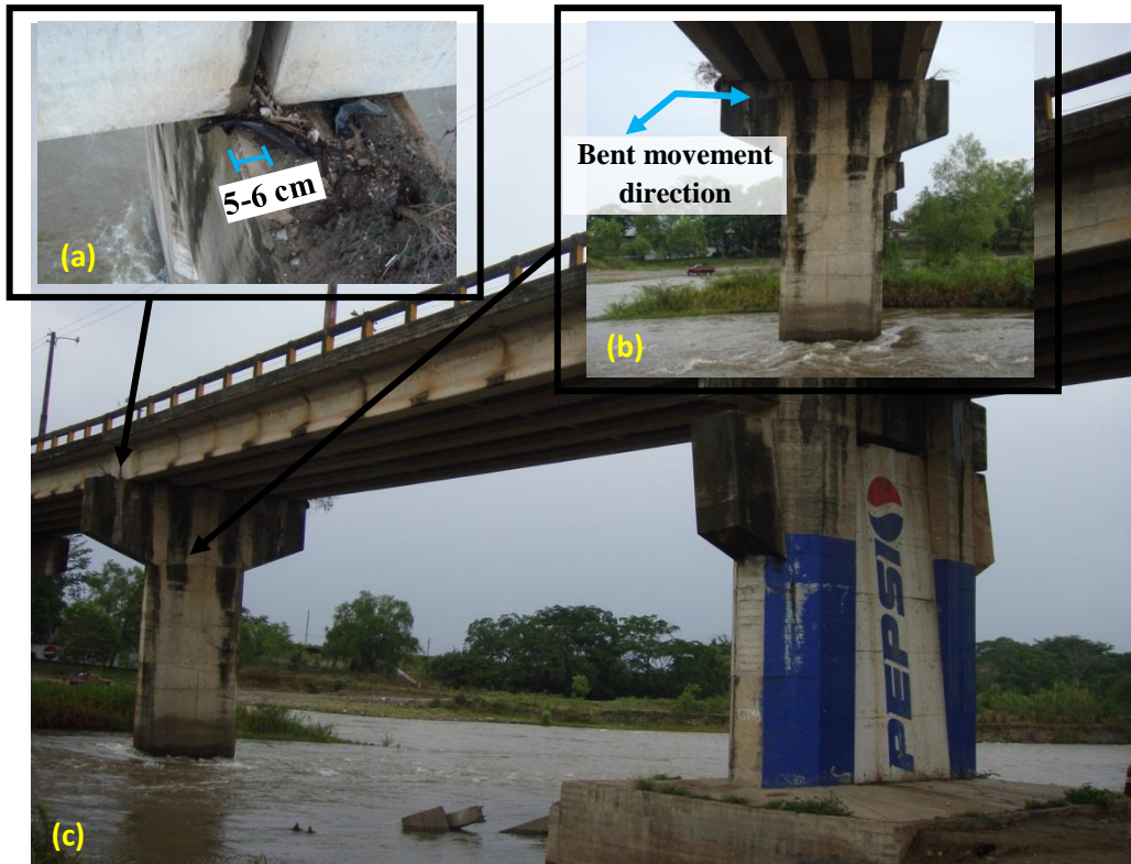
Figure 14 – Santa Rita Bridge over the Humuya River after the earthquake and before collapse (a) [06/21/2009, 6:08PM, N15.191548, W87.82559] (b) [06/21/2009, 5:43PM, N15.191017, W87.8922393] (c) [06/21/2009, 5:40PM, N15.190907, W87.892658]
