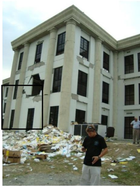
(a) Overall damage including out-of-plane failure of masonry infill wall [06/19/2009, 5:53PM, N15.472899, W88.018565].
