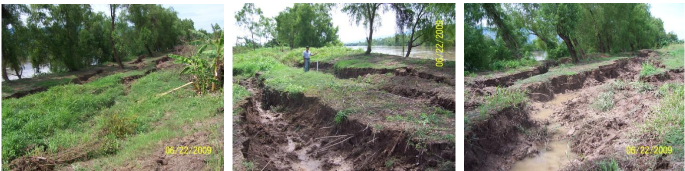
Figure 9 – Multiple views of severe lateral spreading between levees and river [06/22/2009, 10:25AM, N15.391266, W87.845191].
