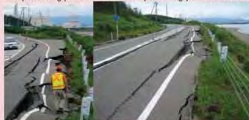
Road Embankment and Pavement Failure
