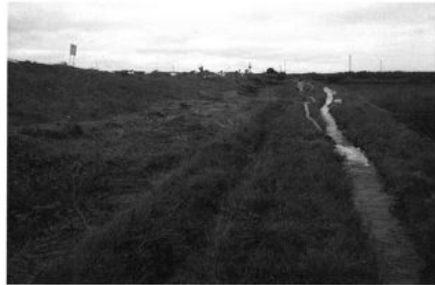
Figure 6-59 Dike along north bank of Assabu River: westward view showing irrigation ditch that was pushed outward and settled. A hose carries water past the damaged section.
